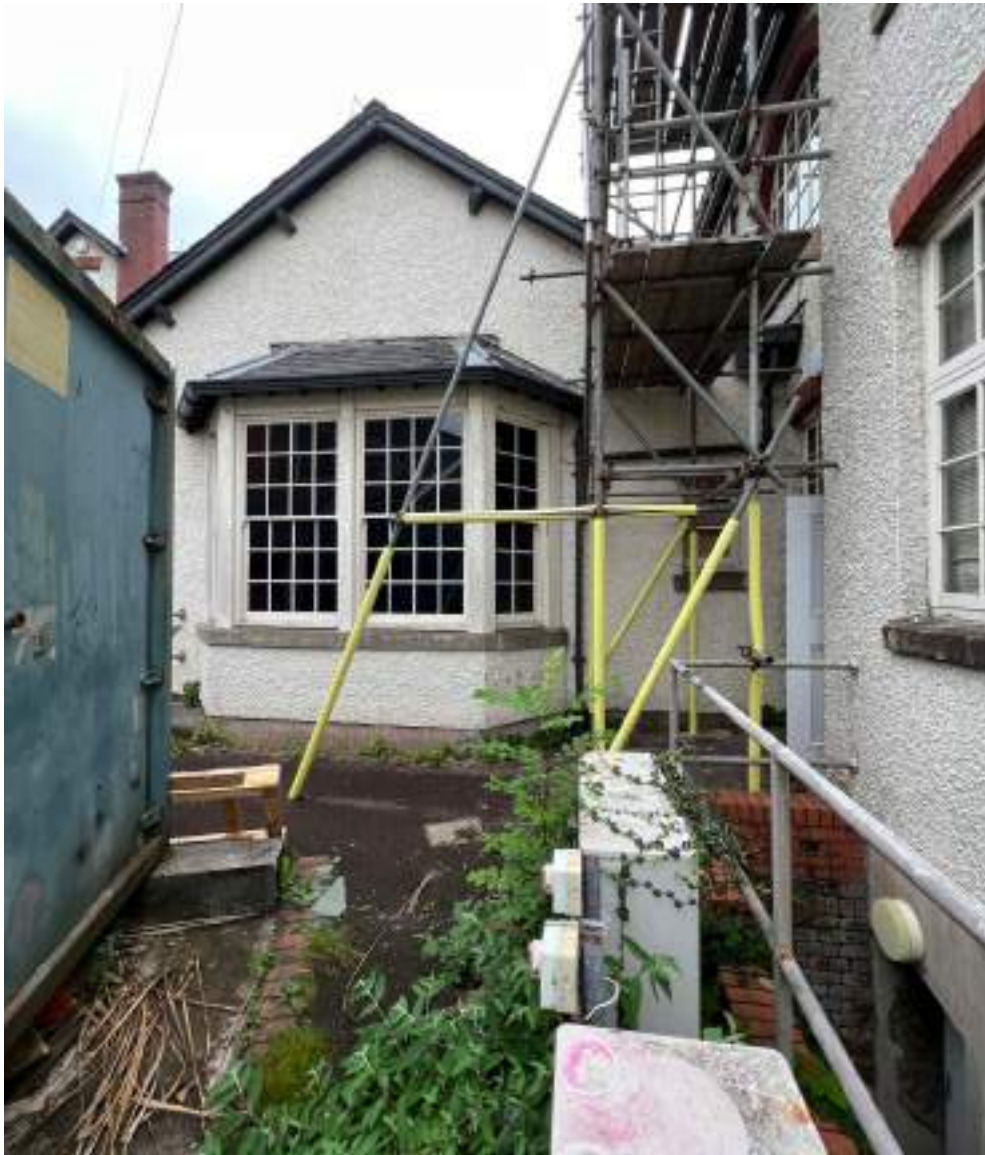
Photograph 124: Shipping container to the left of the image with bay window to ground for studio with timber sash windows in front
