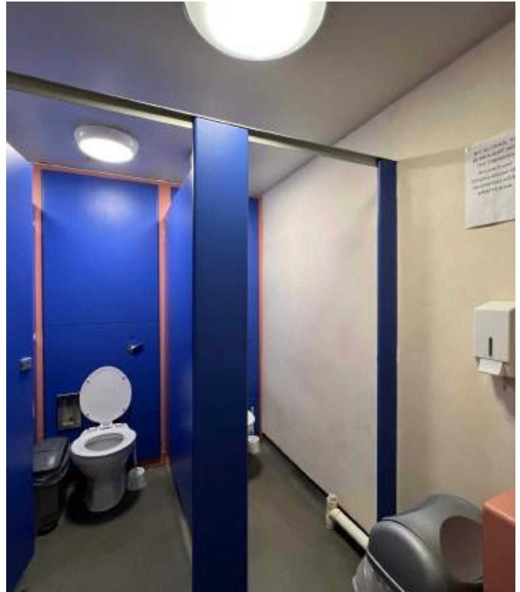
Photograph 82: Modern toilet cubicle system and finishes
