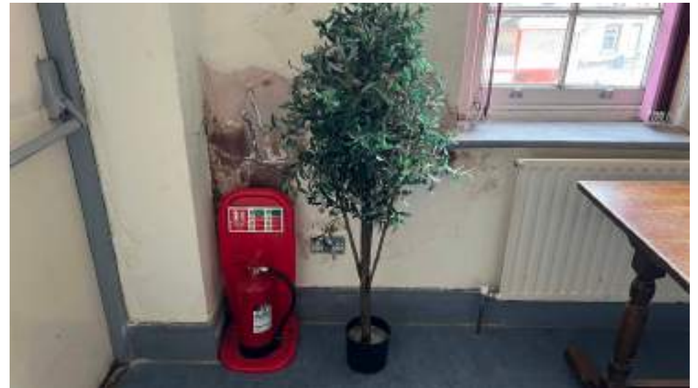
Photograph 96: Signs of significant water ingress from west facade
