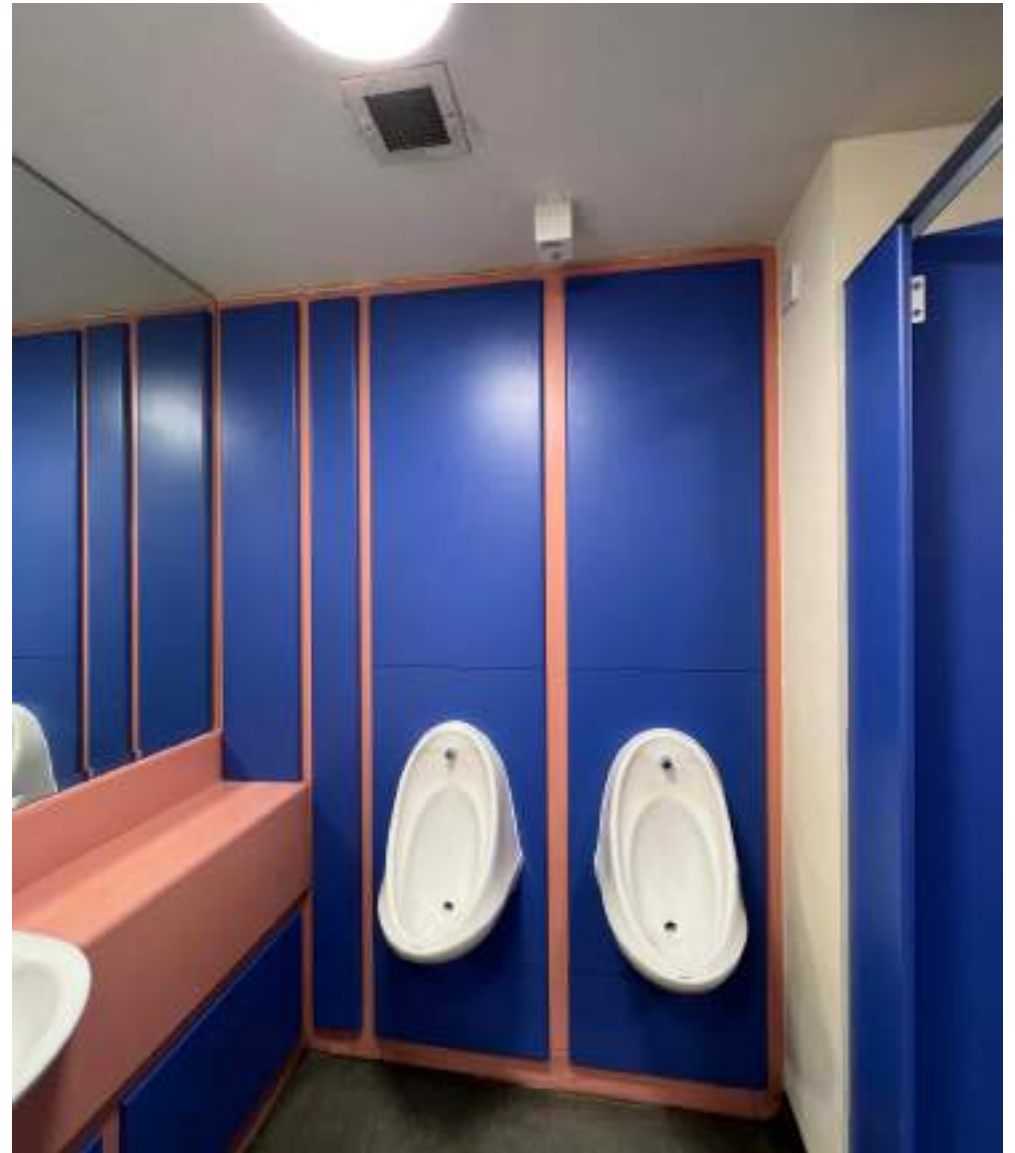
Photograph 84: Modern toilet cubicle system and finishes
