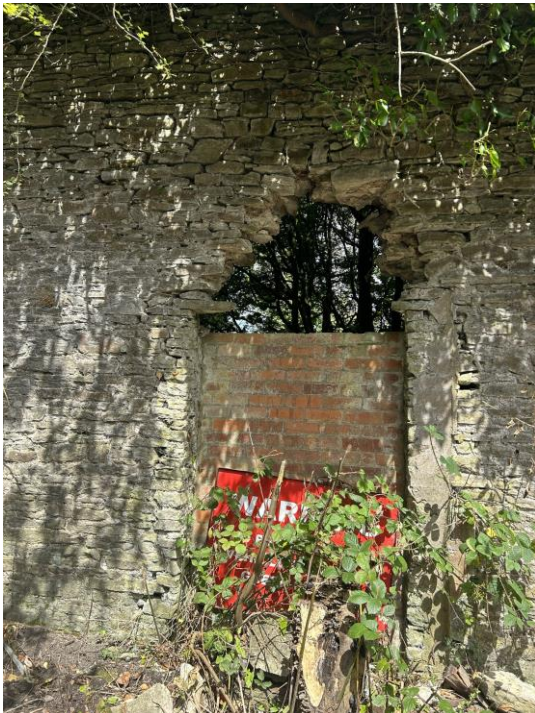
Figure 4.6: Partially collapsed opening along the north-west wall.
