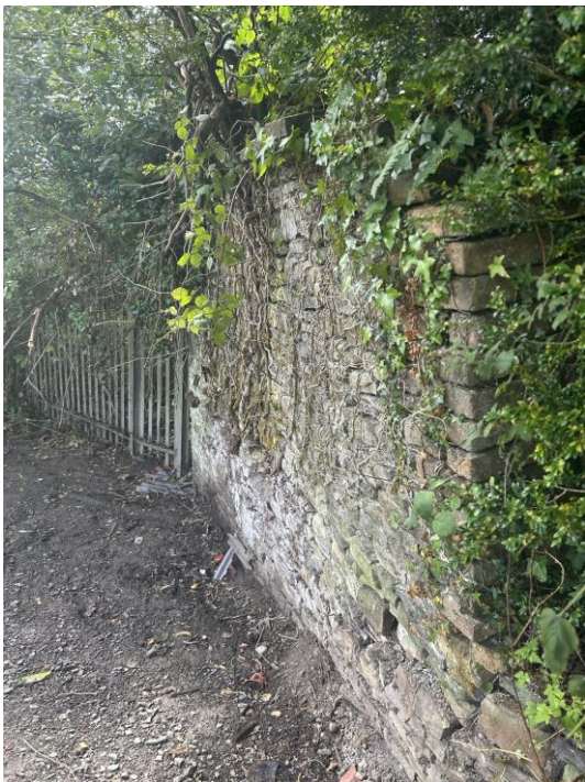
Figure 4.8: Wall A – Side view, providing some indication of the section out of plumb and the large vegetation on top of the wall.
