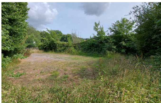
Area 1: ill maintained asphalt, with overgrown rear portion to the foreground, right of the photo.
