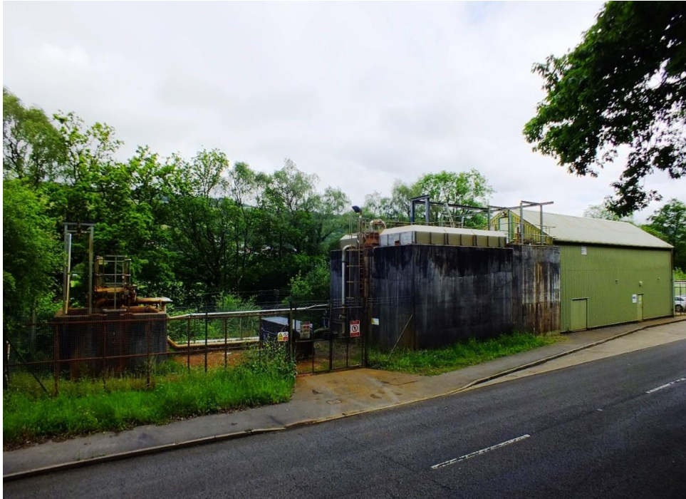
Photograph 3 – View looking south east towards the active treatment plant
