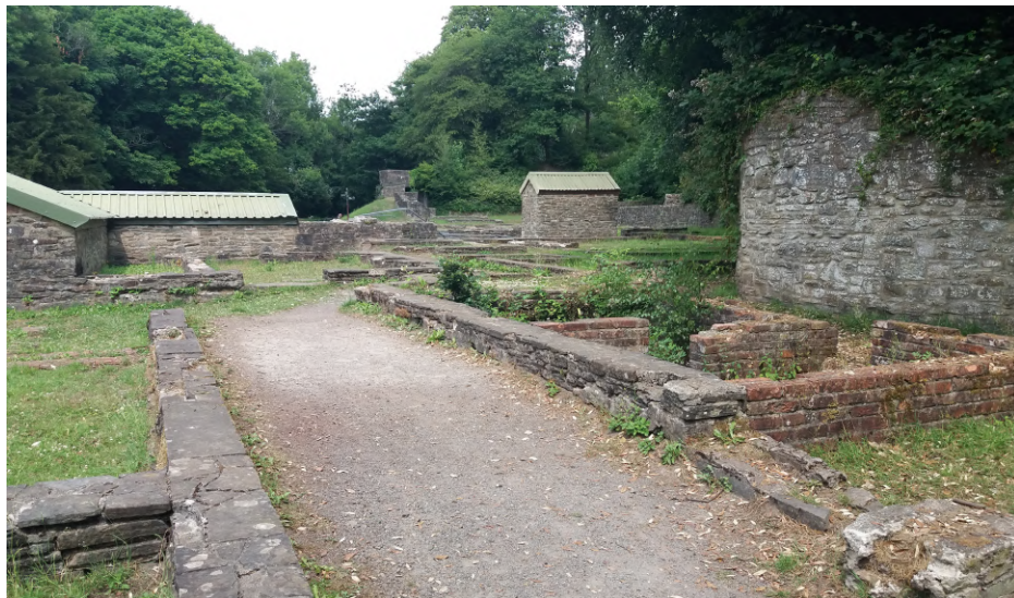
Stonework above ground uses modern cements and lacks maintenance
