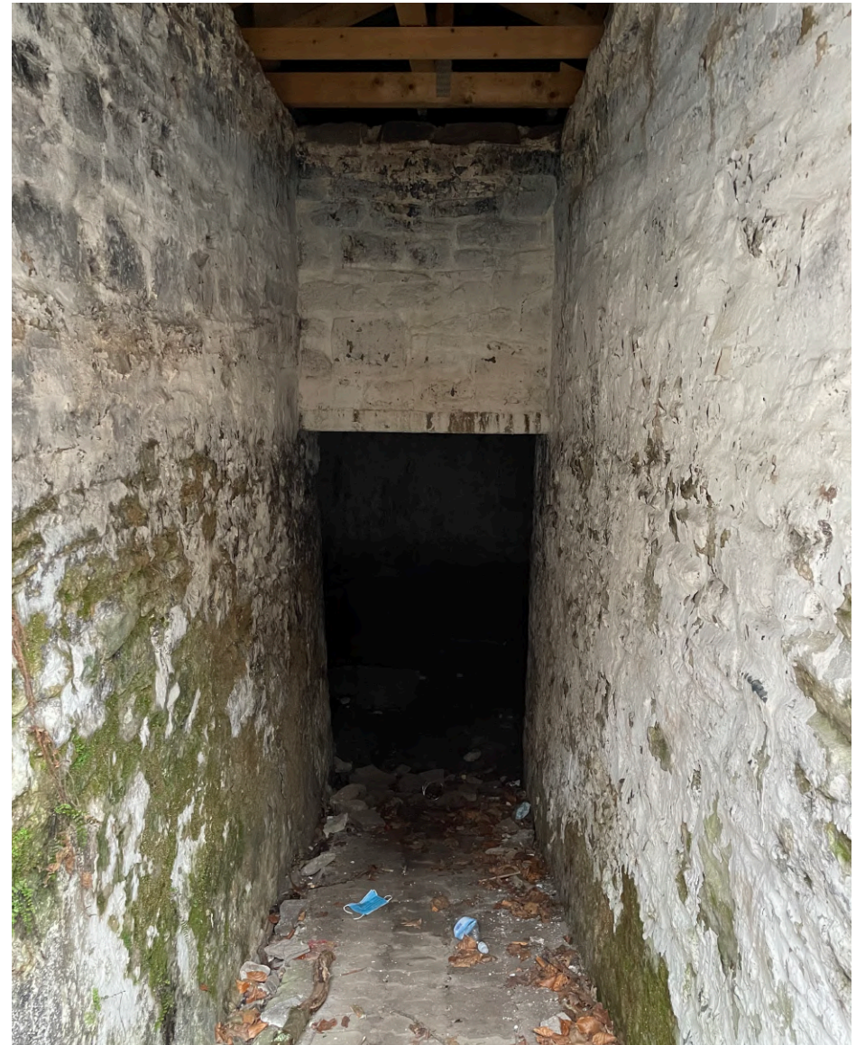
Improved lighting will make spaces more accessible and less intimidating
