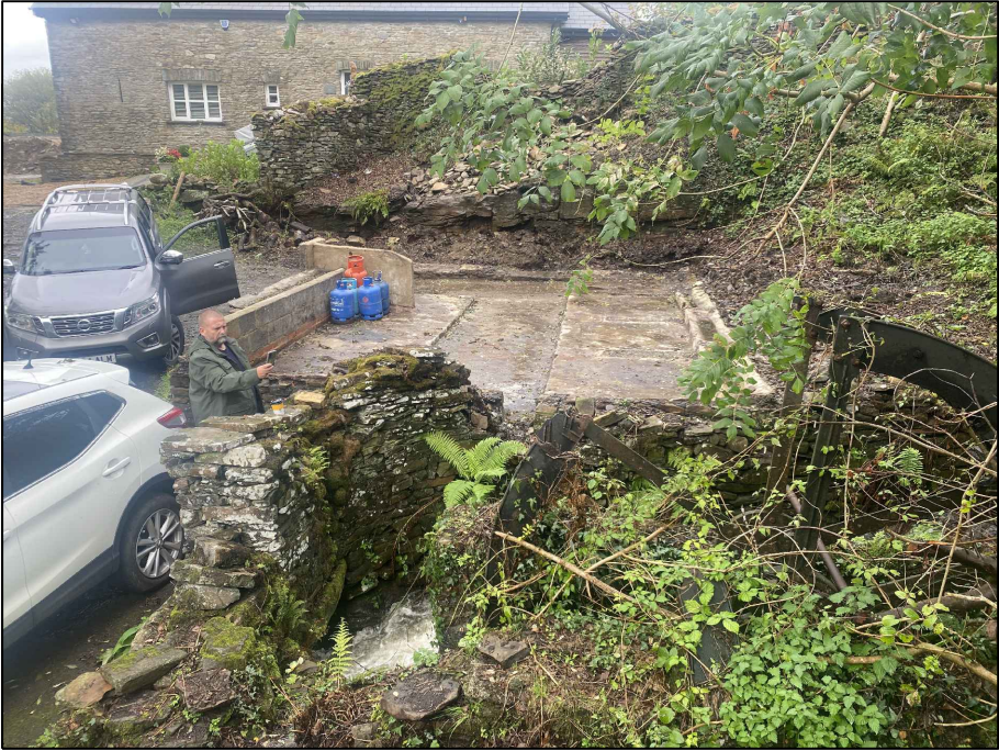
Pic.3 There is a concrete floor slab remaining that was designed for use as a milking shed, which has a central channel for collection of cattle waste that could be washed directly into the brook (which would no longer be allowed). The site slopes downward toward the brook, which has a dry stone wall facing to the bank. Building in such close proximity to the brook will add complexity.
