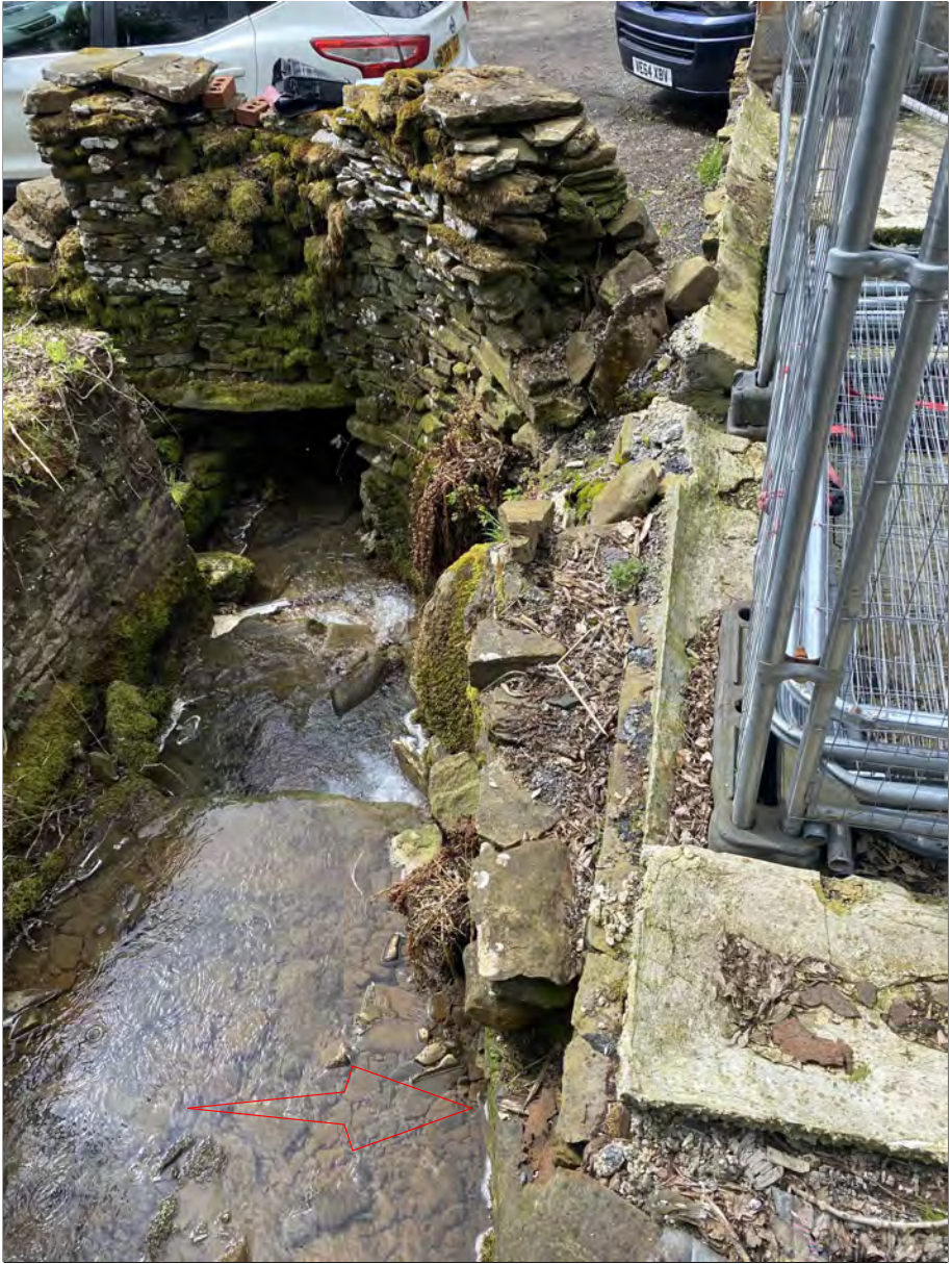
Pic.19 At its closest point to the vertical wall of the stream embankment the existing slab sits atop the embankment wall - with only 150mm or so of edge projection before the vertical face of the wall drops to the stream bed - a height of appx 1200 mm. The wall would need to be reduced in height to accommodate the depth of the concrete raft edge and associated formwork.
