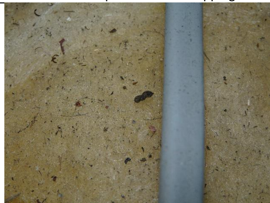
Photo 28: Close up view of bat droppings
