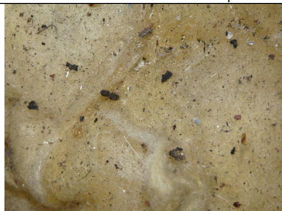
Photo 26: Close up view of bat droppings
