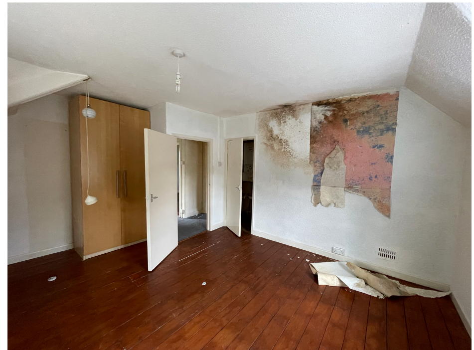
The interior of Pond Cottage has been 'modernised' with a variety of inappropriate materials, all of which serves to reduce the breathability of fabric
