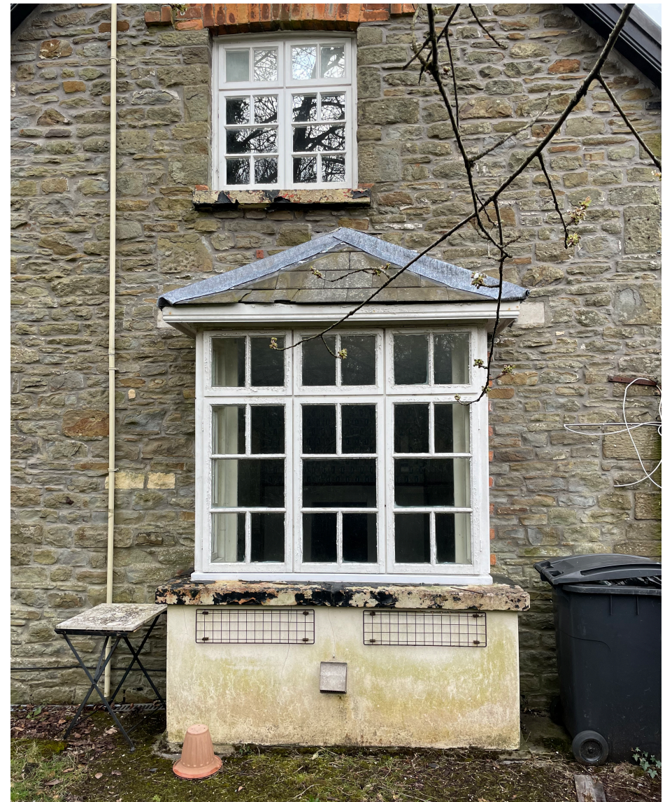
External walls to the property are extensively pointed in cement mortar with cements renders also being prevalent. These stop the fabric from 'breathing'
