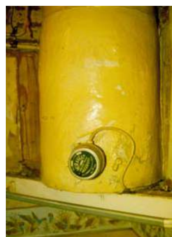
Figure 18 Domestic hot water cylinder lagged with asbestos
