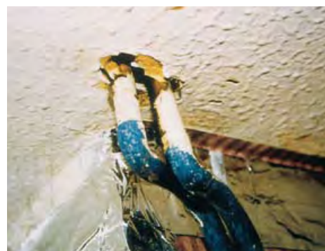
Figure 14 Decorative coating containing asbestos
