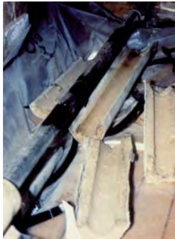
Figure 25 Sectional 'caposite' asbestos pipe lagging
