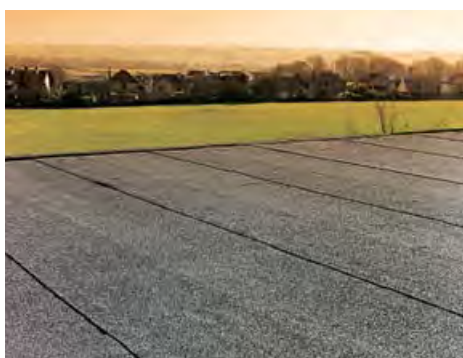
Figure 13 Built-up bituminous roofing containing asbestos
