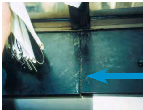
Figure 8 Window sill reinforced with asbestos
