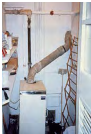
Figure 32 Asbestos cement flue on a domestic boiler
