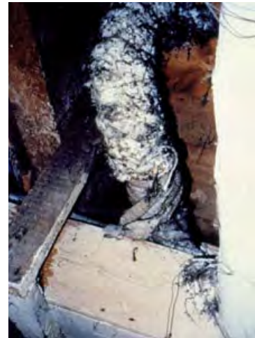
Figure 26 Asbestos rope pipe lagging
