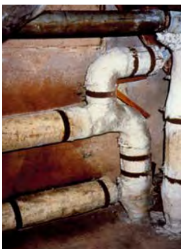
Figure 23 Asbestos pipe lagging
