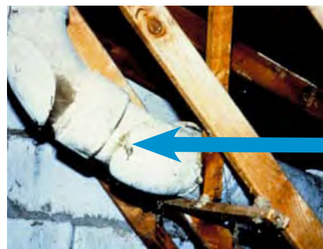
Figure 24 Asbestos cement flue in a ceiling void
