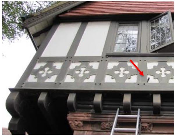
Detail of 1st floor's exposed timber frame, showing screwdriver pushed 120mm into void at decayed joint
