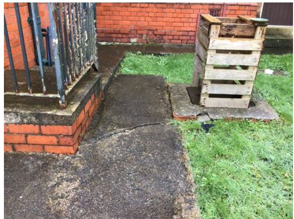
Defective concrete path and single step at NW corner of laundry
