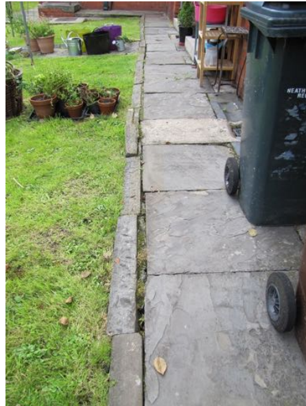
W rear path, showing displaced kerb stones & narrow width
