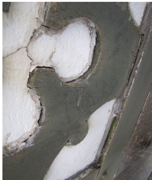
Cracked render & failed silicone mastic
