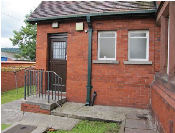
Laundry viewed from W, showing single step to be replaced
