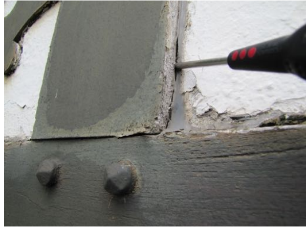
Typical decay within posts where hard render hinders drying out
