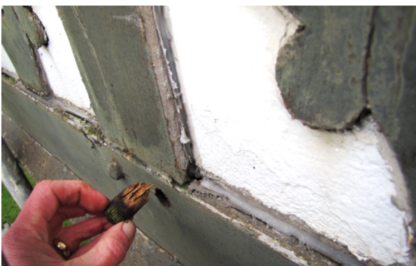
Decayed matching hardwood pegs (with shaped heads)
