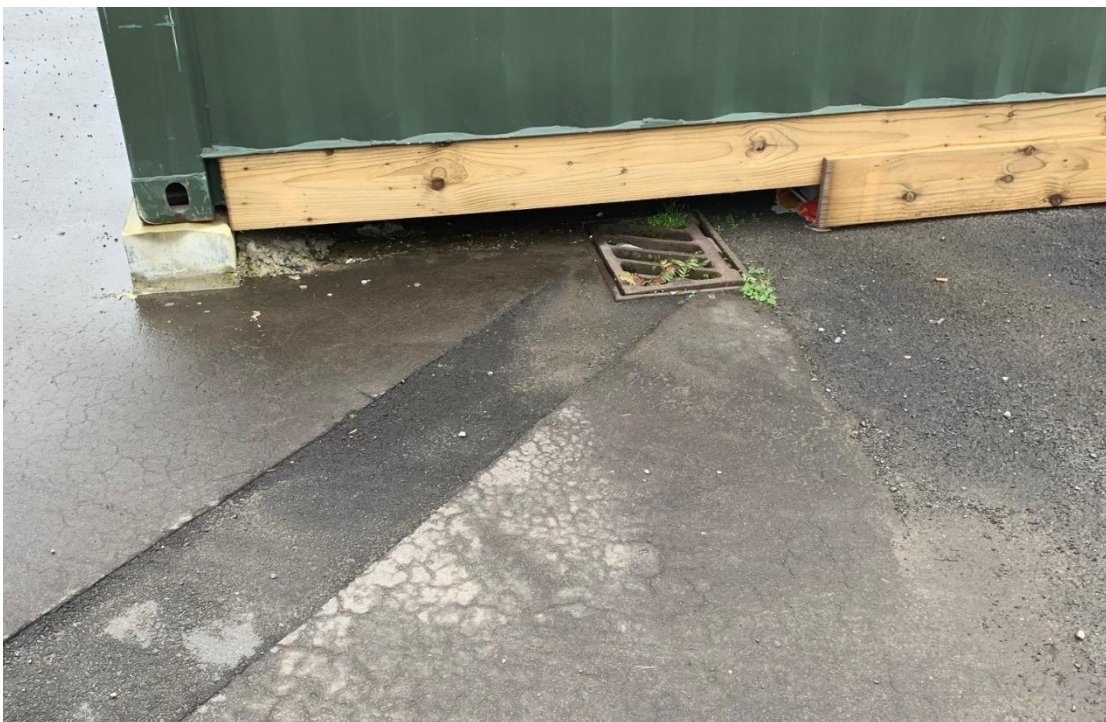
Figure 2-6 Void area under the raised container
