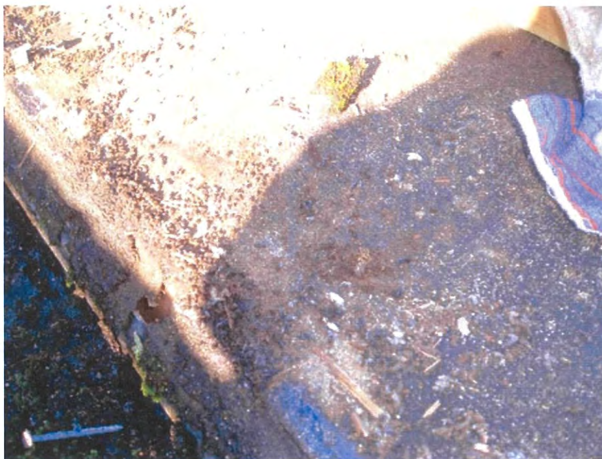
Droppings under the tiles on the southern pitch of the roof
