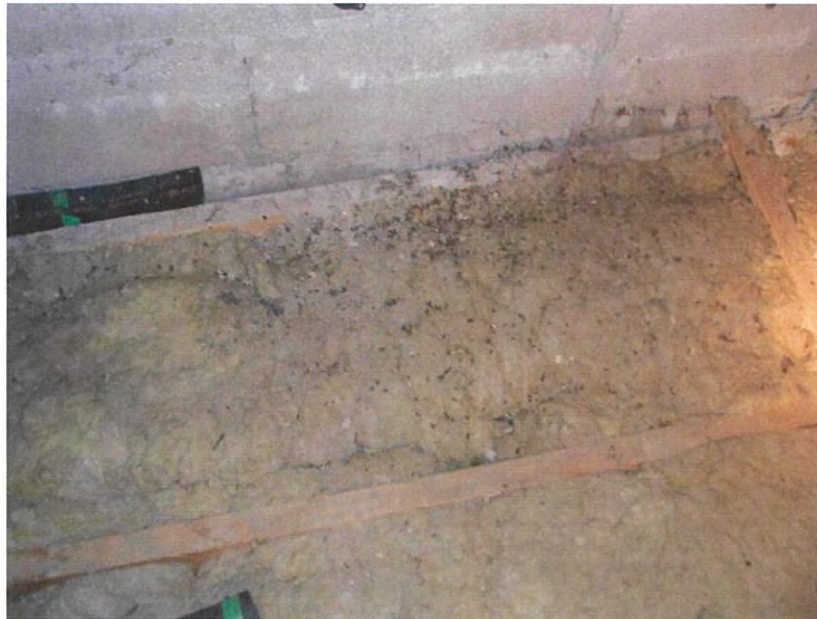
Typical scattering of old and fresh pipistrelle droppings at gable wall.
