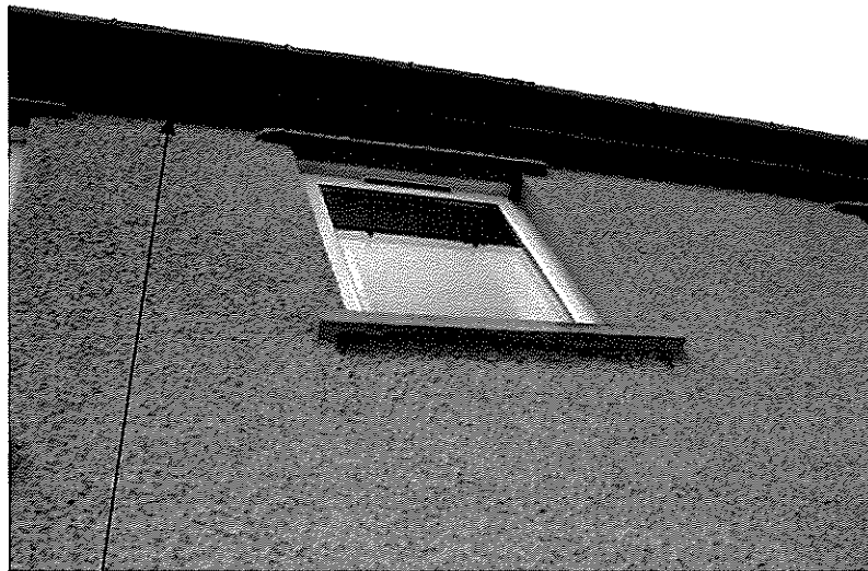
Significant gaps between render and soffits in western wing
