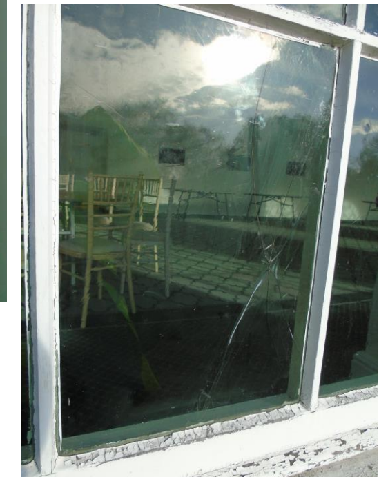
Figure 5: Cracked Cylinder Glass, Exterior
