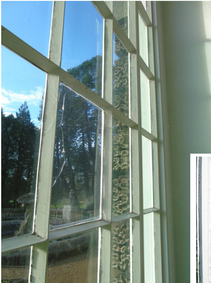
Figure 4: Cracked Cylinder Glass, Interior
