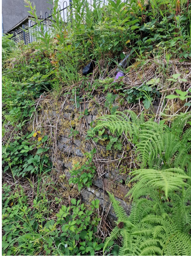
Overgrowth at top of wall
