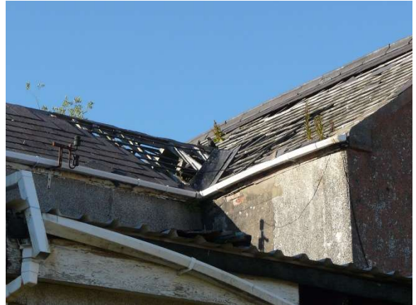
Image 5: Roof - viewed from south - large gaps
