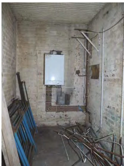
Fig 27: External store (east) housing gas fired boiler.
