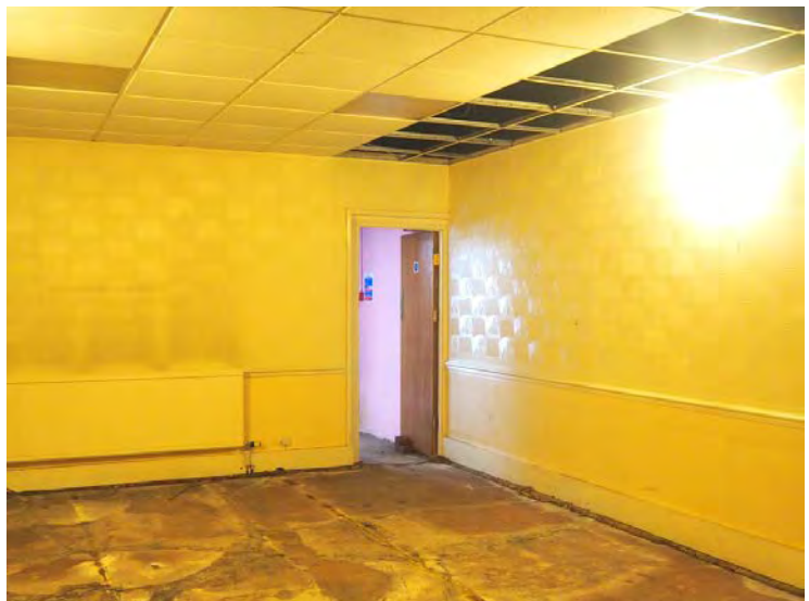
Fig 34: Ground floor social room with route through to kitchen store/stairs to first floor hallway. Image shows previous lay-in-grid ceiling/contemporary finishes and cracked concrete floor.
