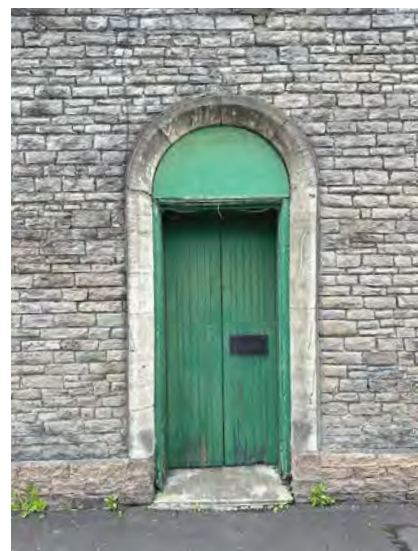
Fig 14: Principal entrance located on south elevation abutting Castle Street. Timber doors in poor condition throughout.
