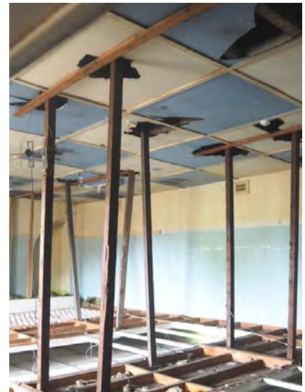
Fig 20: Void over lay-in-grid ceiling with cement tile ceiling, damaged by modern ceiling structure.
