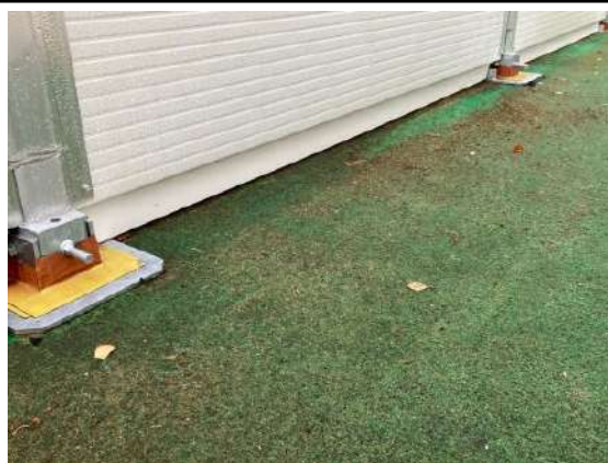
Photograph Five - Evidence that perimeters have now been protected with a PVC trim.
