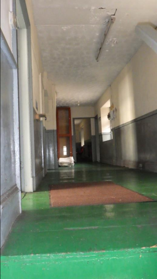
Areas need refurbishing.
