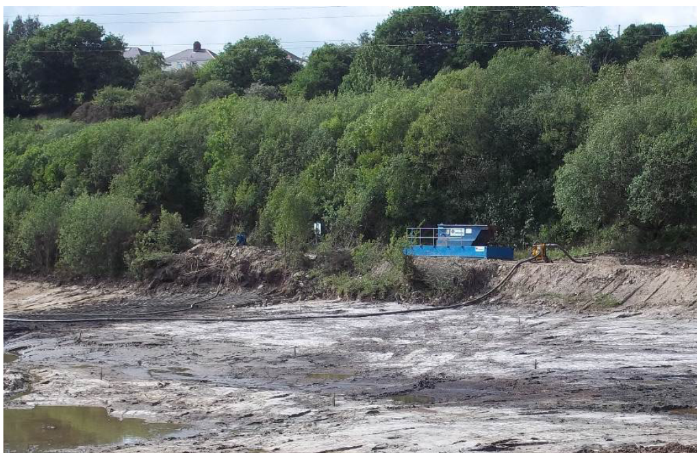
Photograph 10 – Water Treatment System at East Bay
