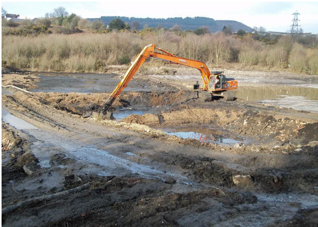
Photograph 17 – Mixing lagoon within Section 2 of East Bay
