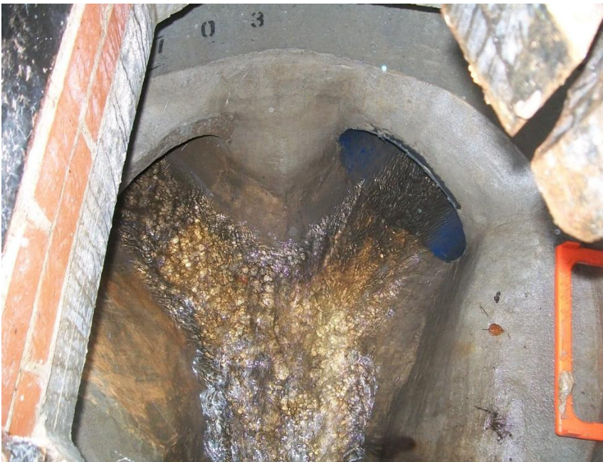
Plate 2. Manhole 000. Skewen drainage to the left, NSR drain to the right.
