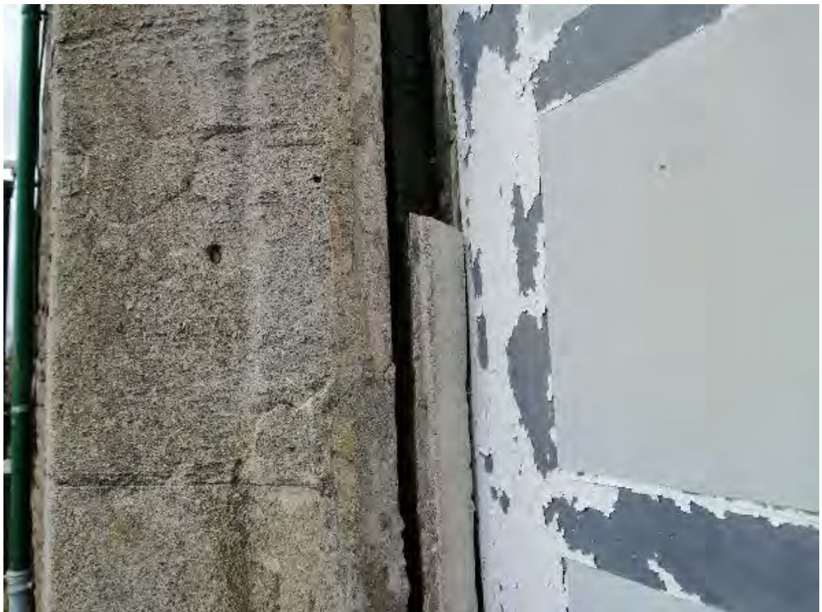
Photo 64 – Cracking and Gaps Around Timber Window Frames (Front Wall Elevation)
