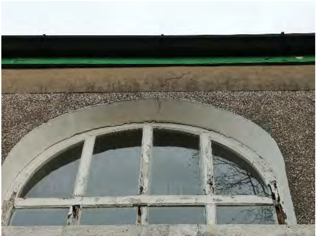
Photo 47 – Render Shrinkage Cracking (Left Wall Elevation)
