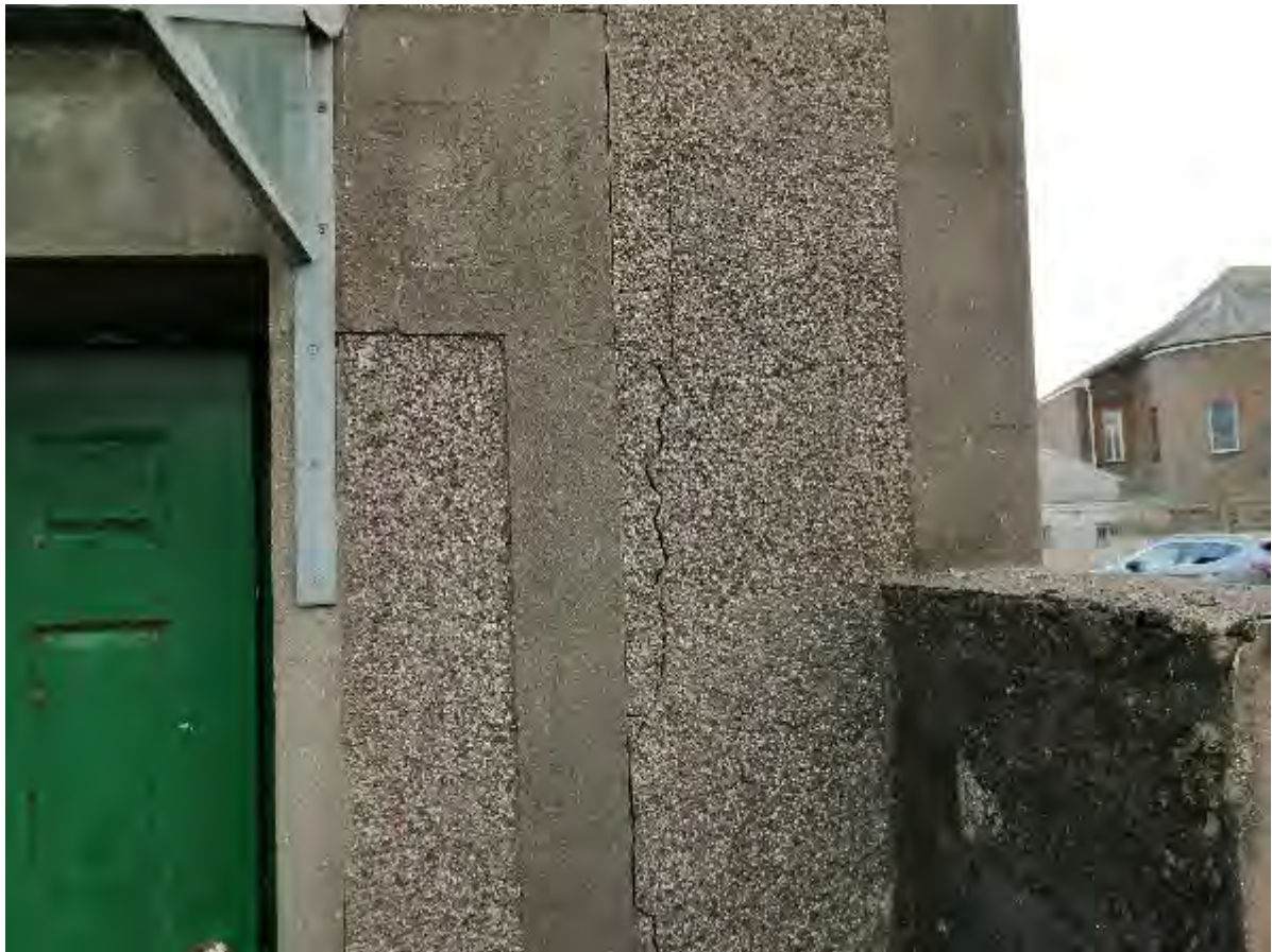
Photo 57 – Wall Crack (Left Wall Elevation)
