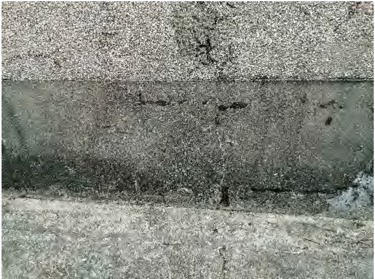
Photo 44 – Render Shrinkage Cracking (Left Wall Elevation)
