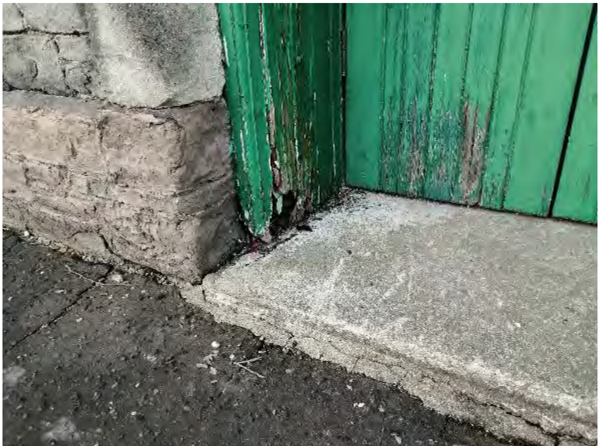
Photo 72 – Weathering and Rot to Timber Door Frame (Front Wall Elevation)
