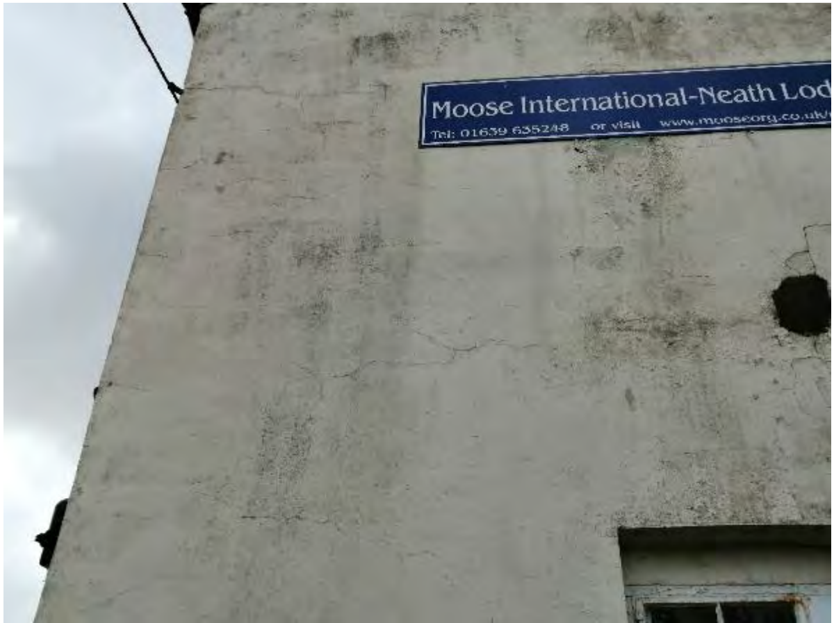
Photo 75 – Render Shrinkage Cracking (Right Wall Elevation)
