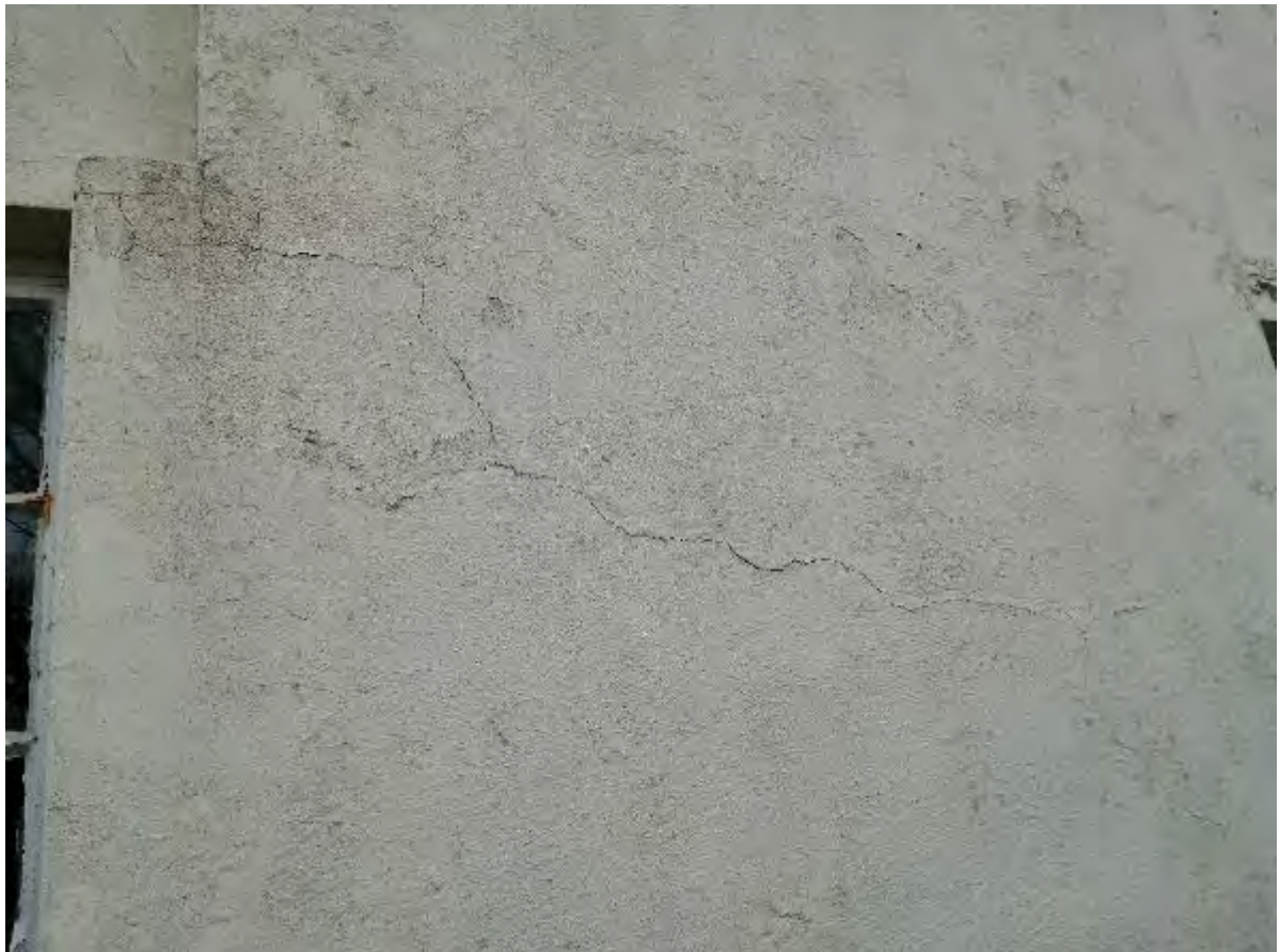
Photo 80 – Render Shrinkage Cracking (Right Wall Elevation)
