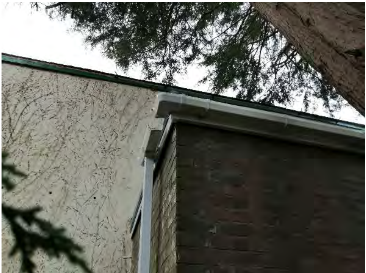
Photo 13 – Missing Guttering (Rear Roof Profile)
