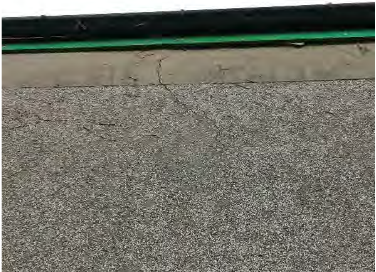
Photo 46 – Render Shrinkage Cracking (Left Wall Elevation)
