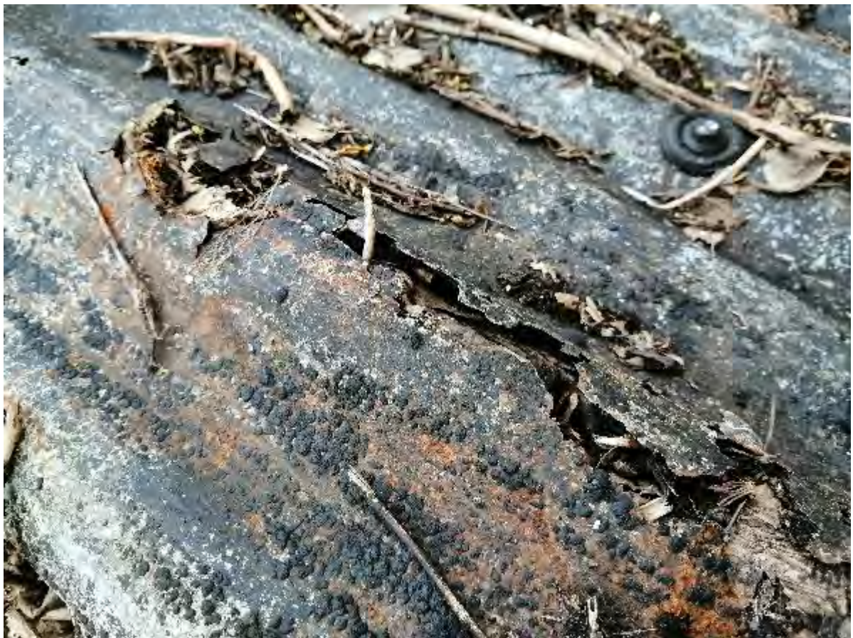
Photo 19 – Holes and Corrosion to Sheeting Material (Rear Roof Profile)
