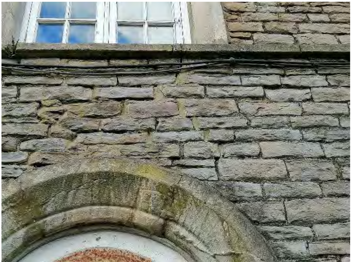
Photo 62 – Cracking to Mortar (Front Wall Elevation)
