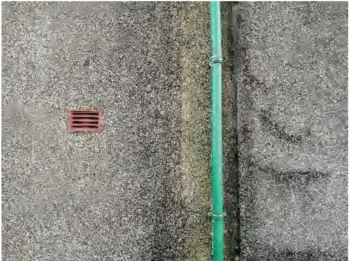
Photo 50 – Render Shrinkage Cracking (Left Wall Elevation)
