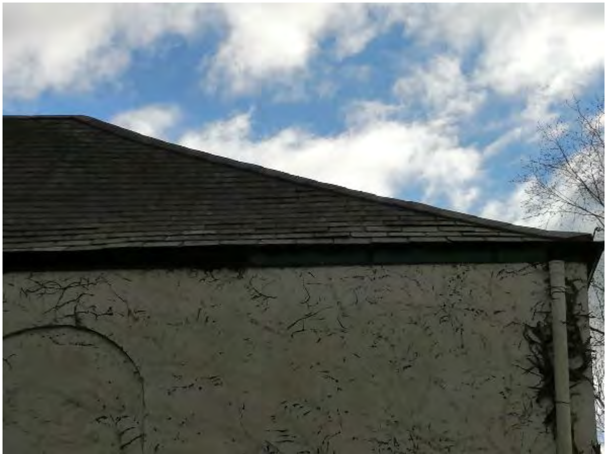
Photo 11 – Missing Guttering and Displaced Edge Tiles (Rear Roof Profile)
