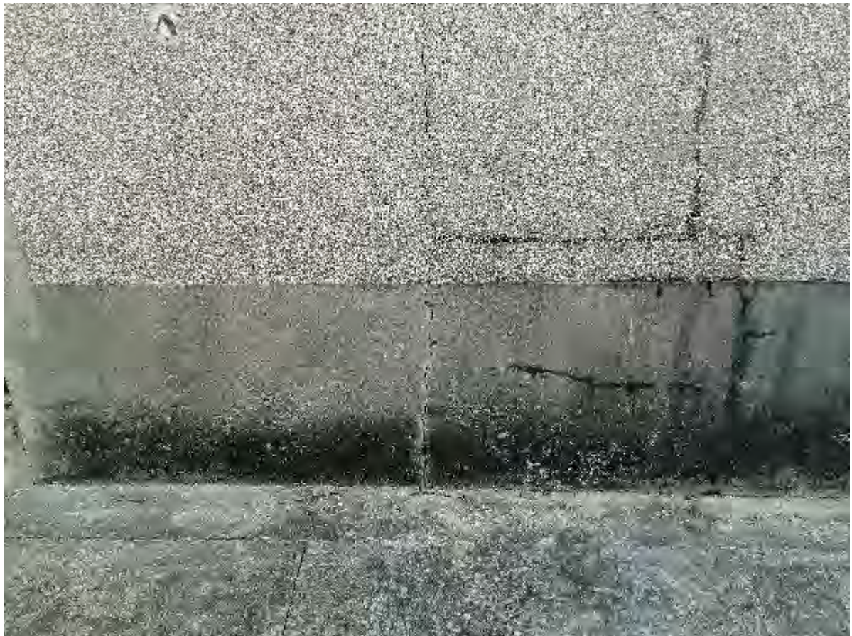
Photo 38 – Render Cracking Around Old Opening (Left Wall Elevation)
