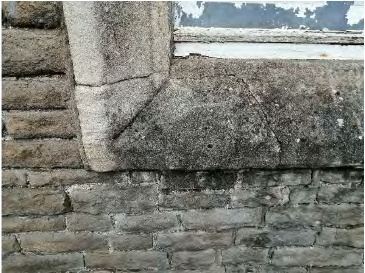
Photo 65 – Cracking to Stonework (Front Wall Elevation)
