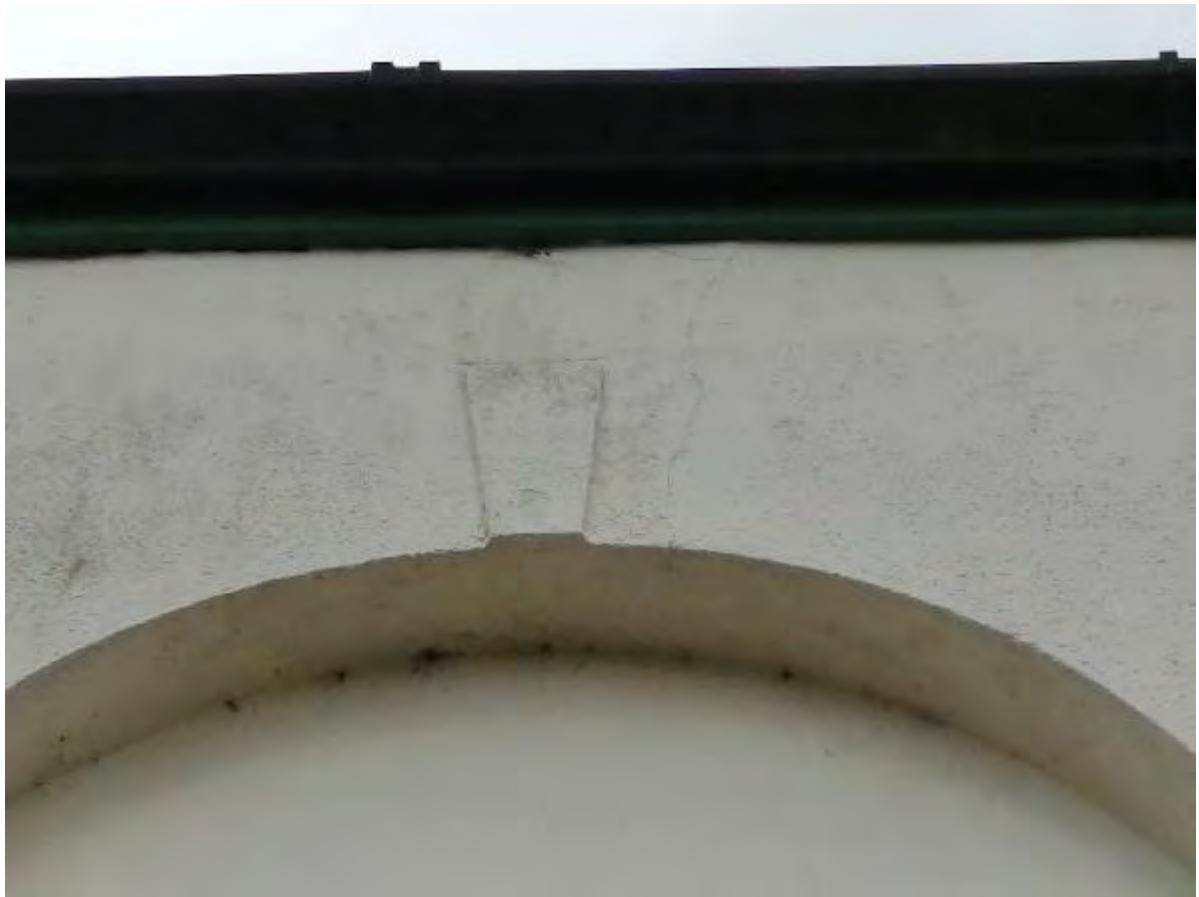
Photo 81 – Render Shrinkage Cracking (Right Wall Elevation)
