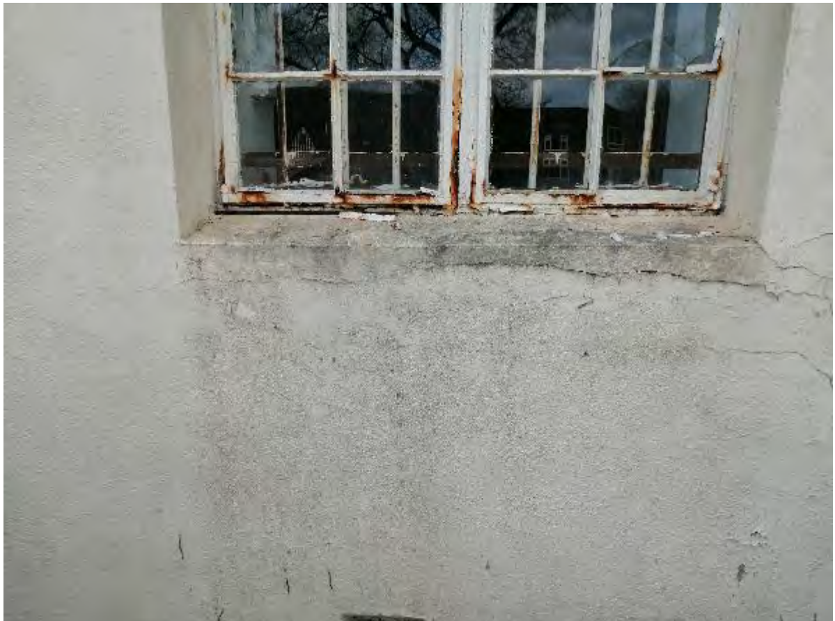
Photo 78 – Render Shrinkage Cracking (Right Wall Elevation)
