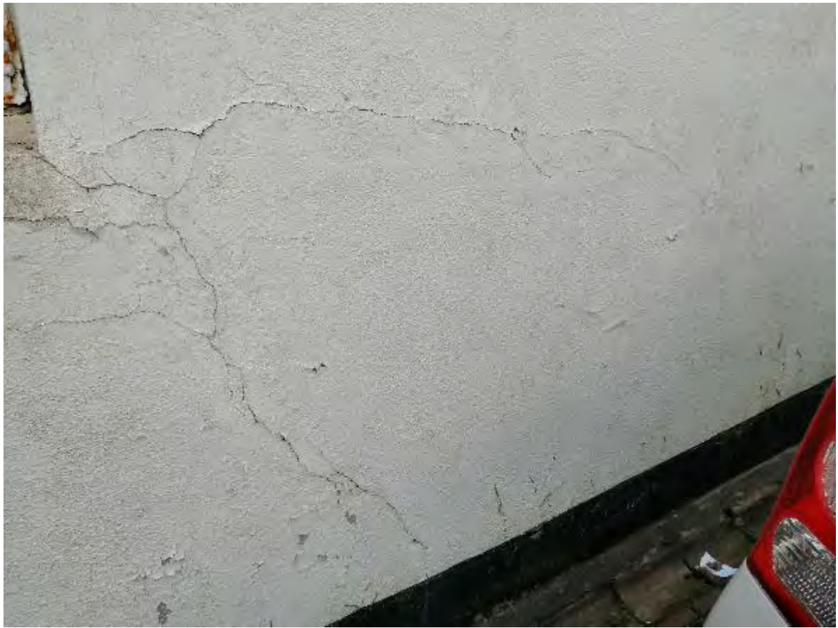
Photo 79 – Render Shrinkage Cracking (Right Wall Elevation)
