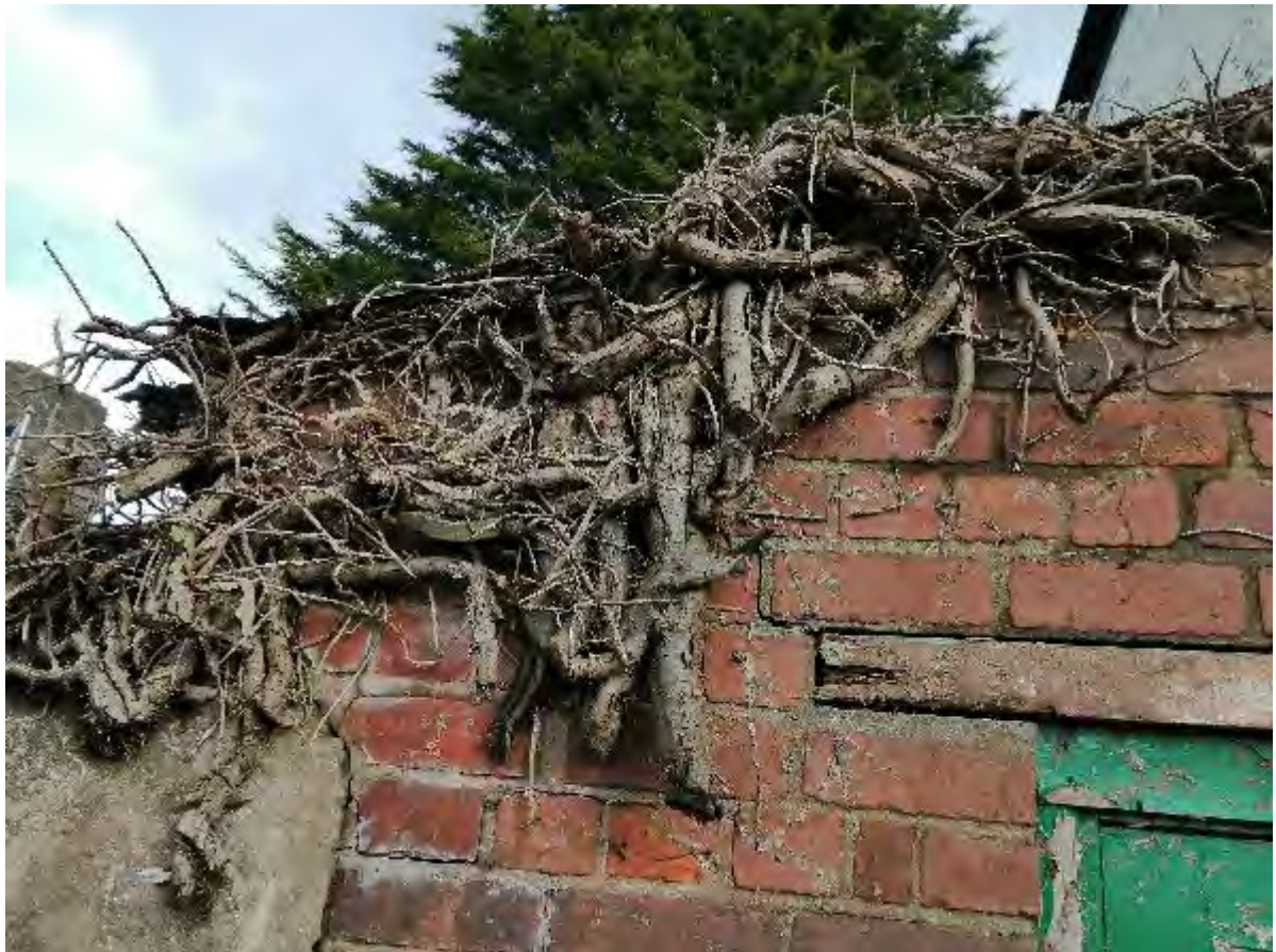
Photo 17 – Vegetation Growth Under Roof Tiles (Rear Roof Profile)
