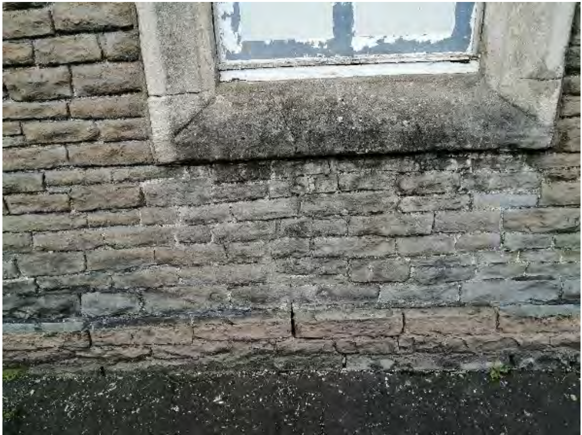
Photo 61 – Cracking to Mortar (Front Wall Elevation)
