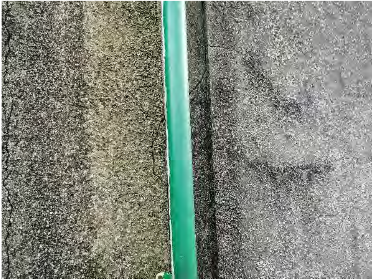
Photo 53 – Cracking Between Original Property and Front Extension (Left Wall Elevation)
