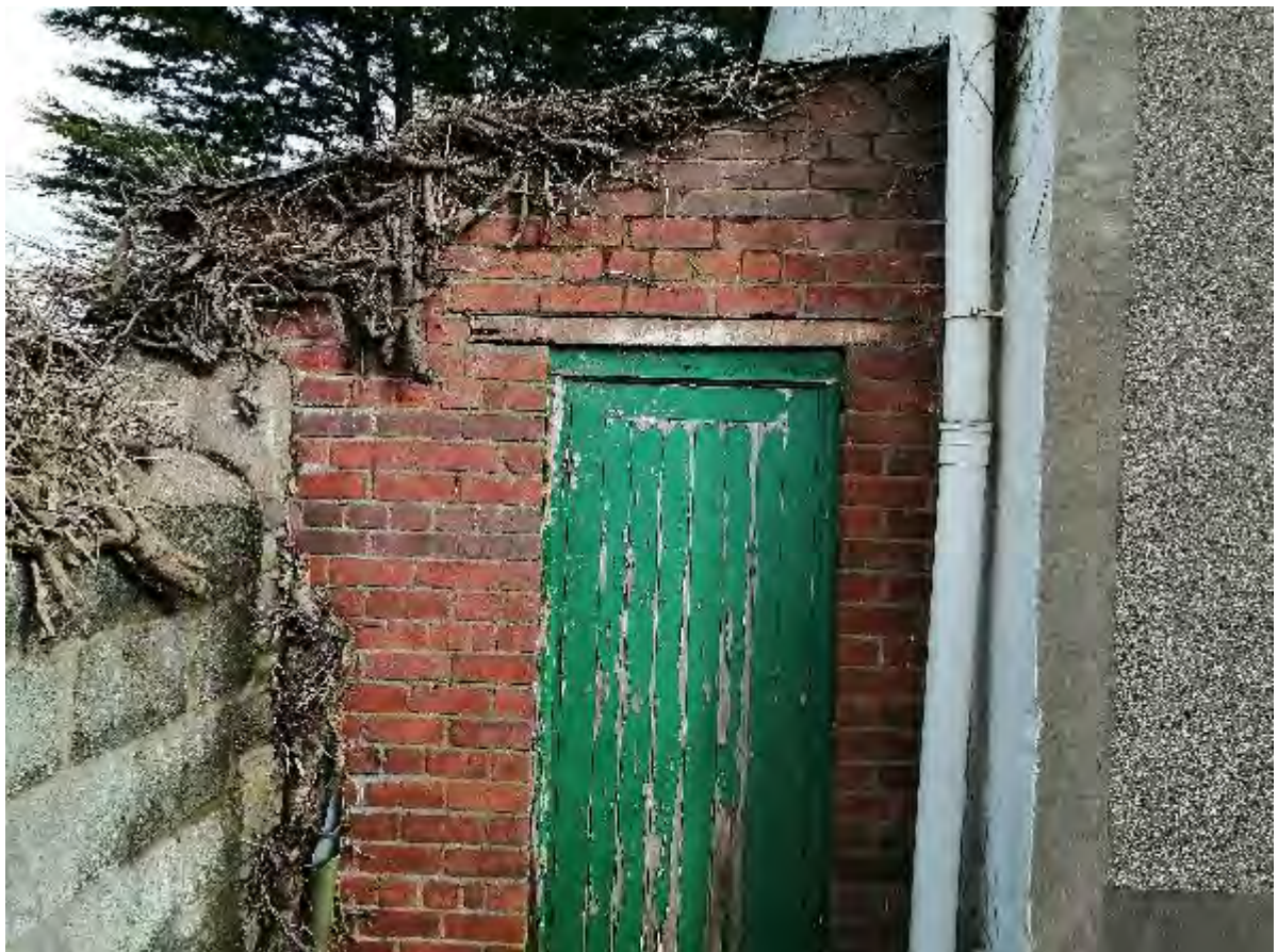
Photo 34 – Vegetation Growth (Left Wall Elevation)
