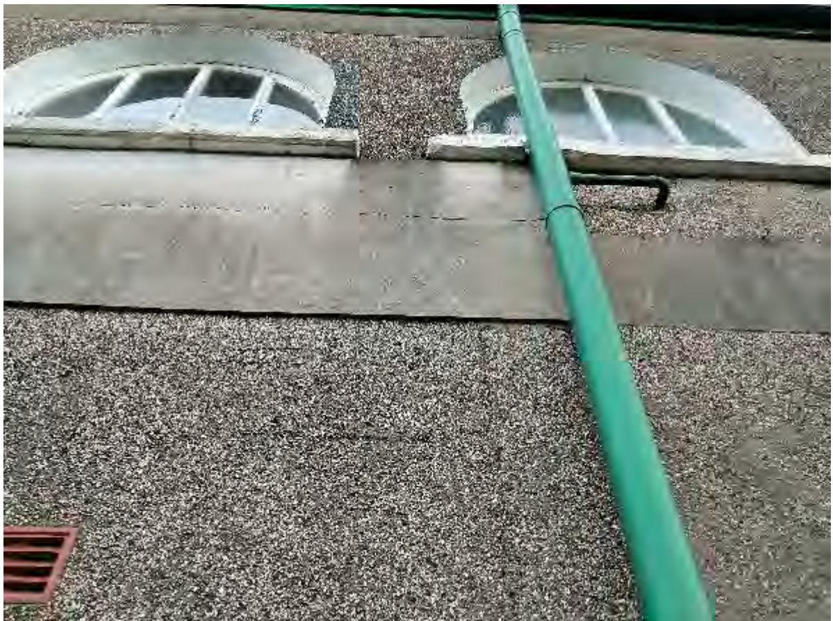
Photo 40 – Render Cracking Around Old Opening (Left Wall Elevation)
