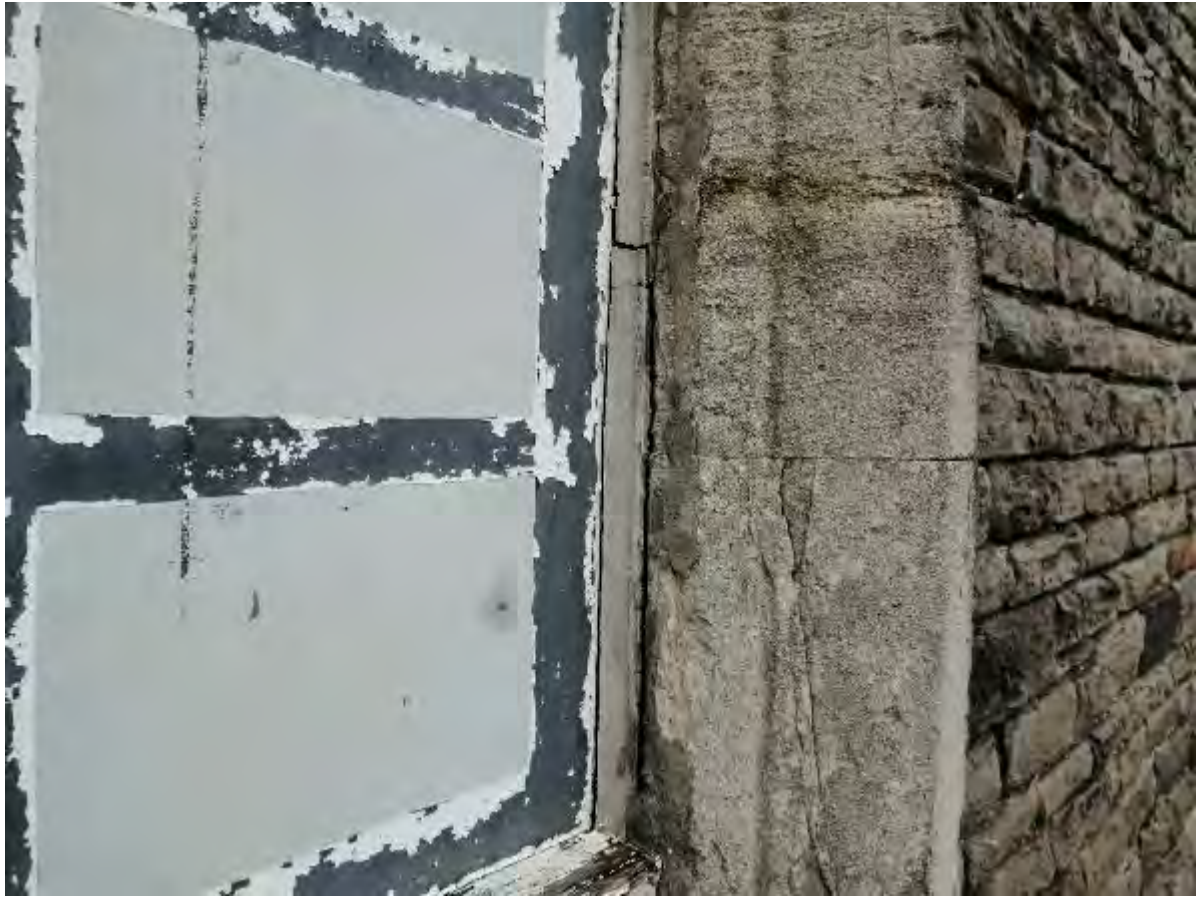
Photo 63 – Cracking and Gaps Around Timber Window Frames (Front Wall Elevation)
