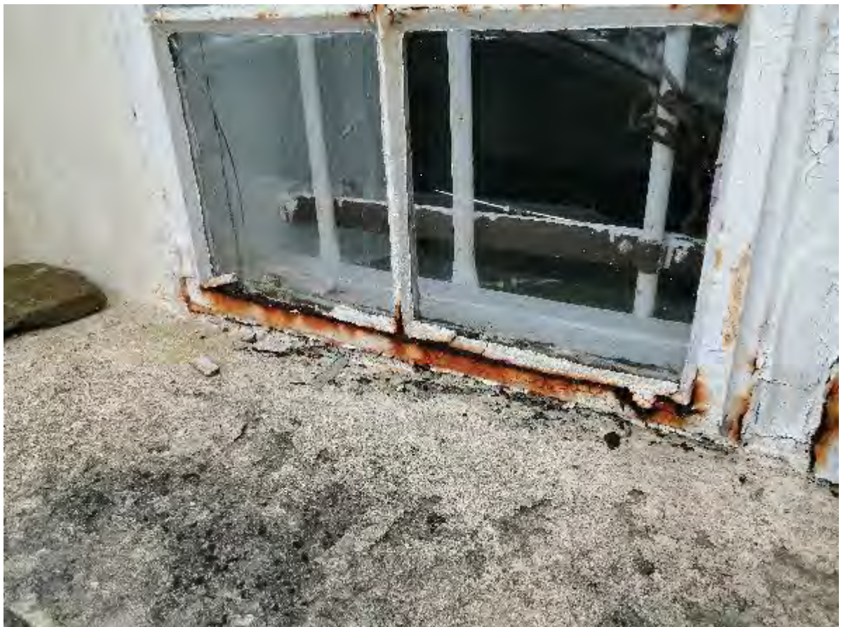
Photo 86 – Corrosion to Metal Window Frame (Right Wall Elevation)
