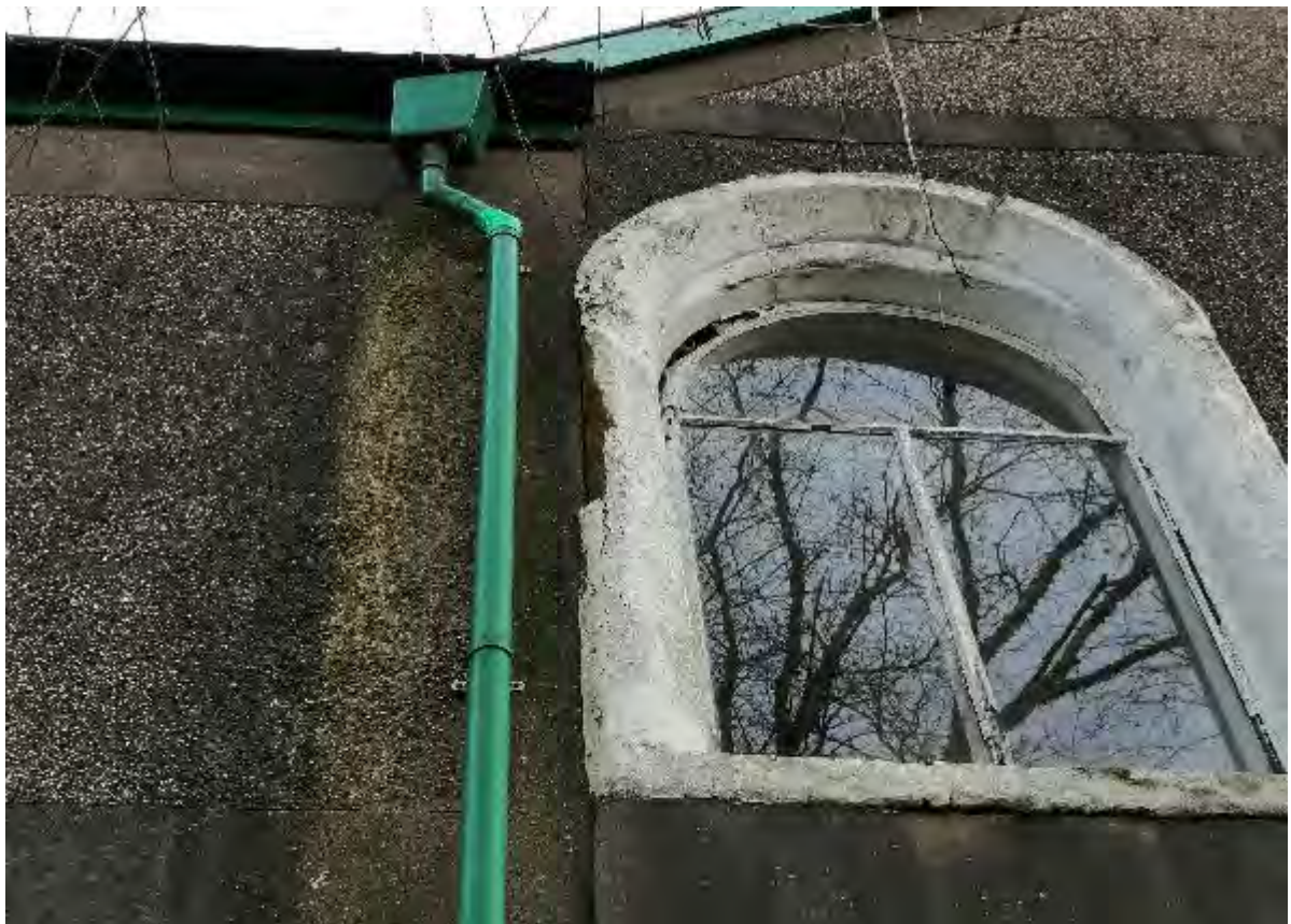
Photo 52 – Cracking Between Original Property and Front Extension and Rot to Timber Window Frame (Left Wall Elevation)
