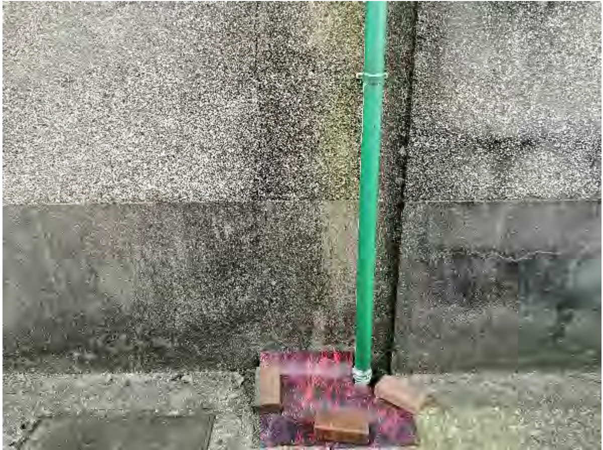
Photo 51 – Render Shrinkage Cracking (Left Wall Elevation)
