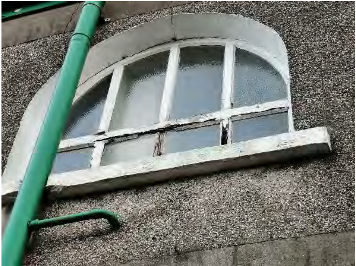
Photo 55 – Rot to Timber Window Frame (Left Wall Elevation)
