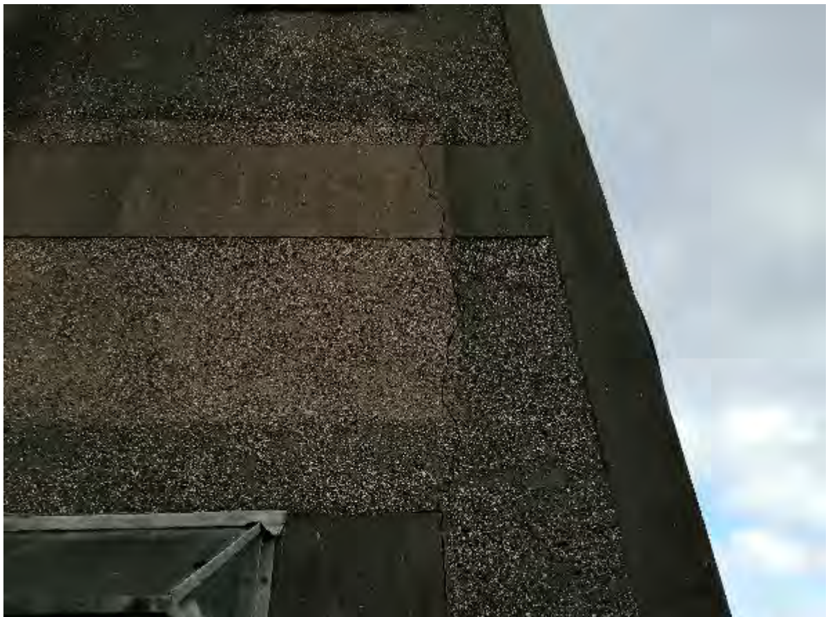
Photo 56 – Wall Crack (Left Wall Elevation)
