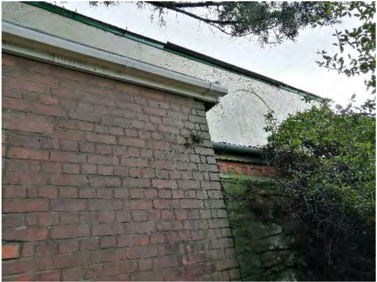
Photo 33 – Vegetation Growth (Rear Wall Elevation)
