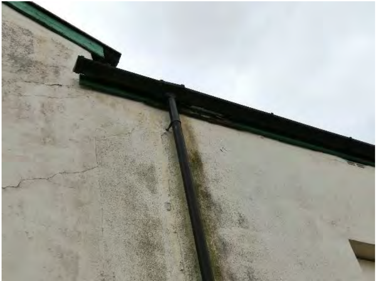
Photo 16 – Weathered Fascia Board (Right Roof Profile)
