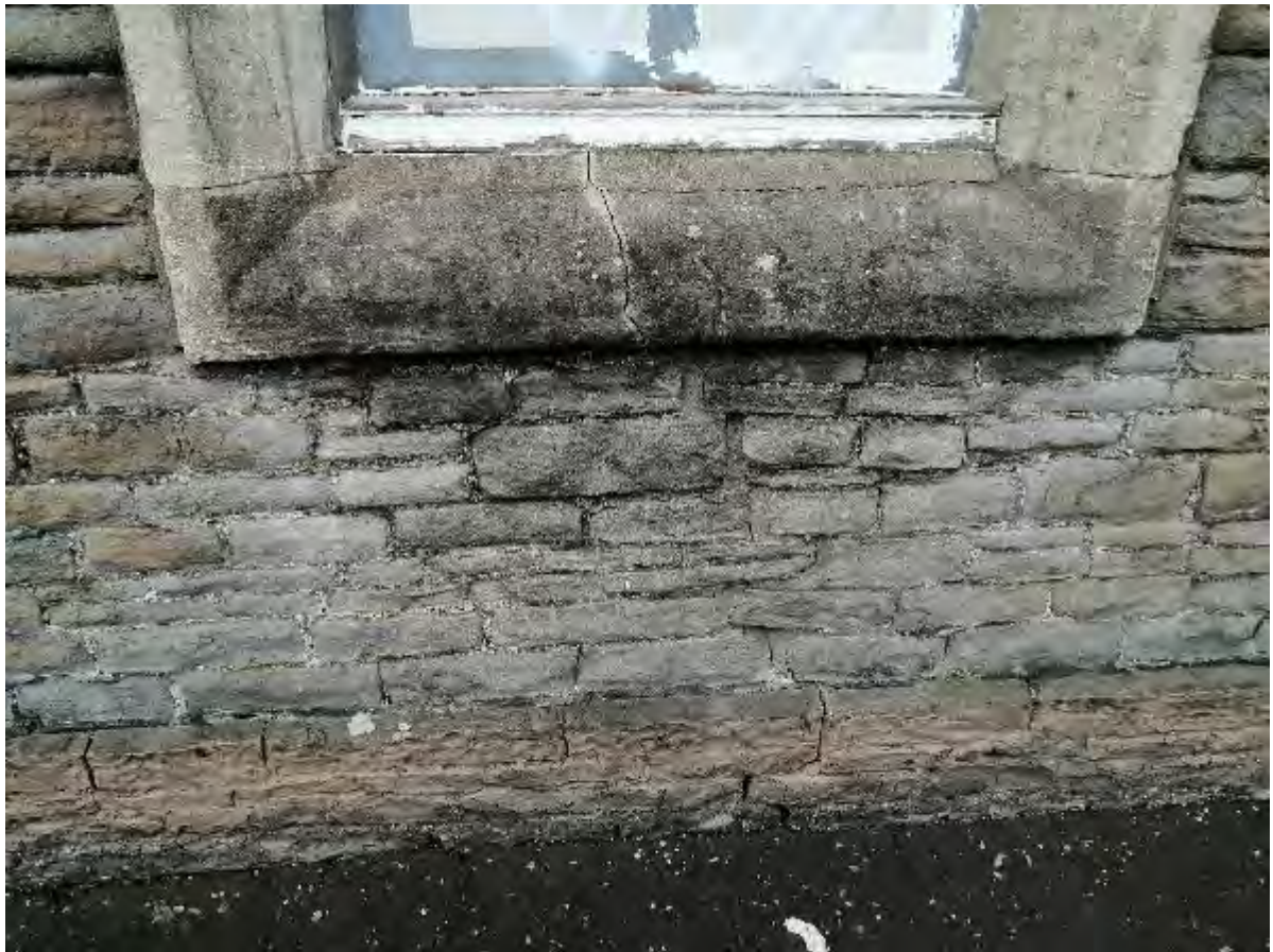
Photo 67 – Cracking to Mortar (Front Wall Elevation)
