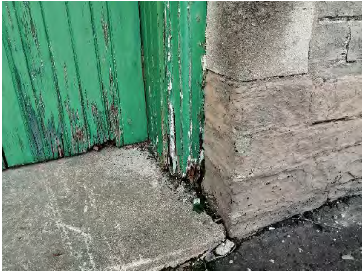
Photo 73 – Weathering and Rot to Timber Door Frame (Front Wall Elevation)
