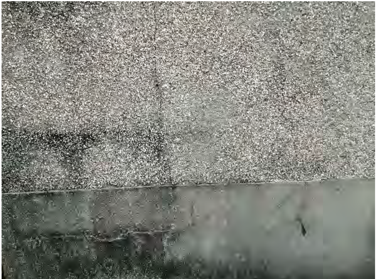
Photo 54 – Render Shrinkage Cracking (Left Wall Elevation)
