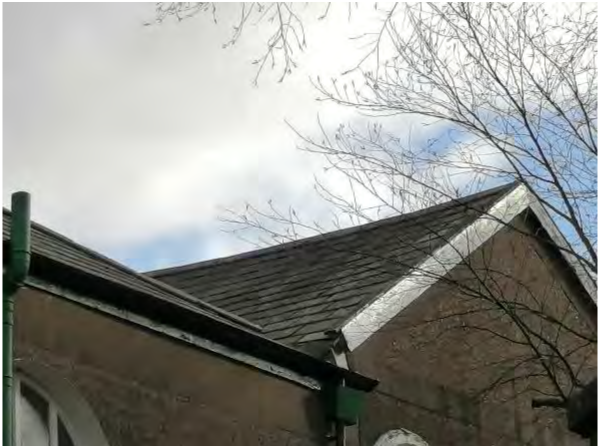
Photo 15 – Weathered Fascia Board (Left Roof Profile)
