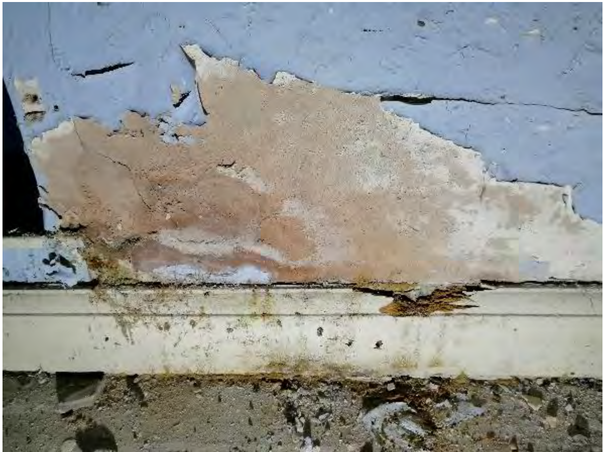
Photo 143 – Penetrating Damp (Rear Room)
