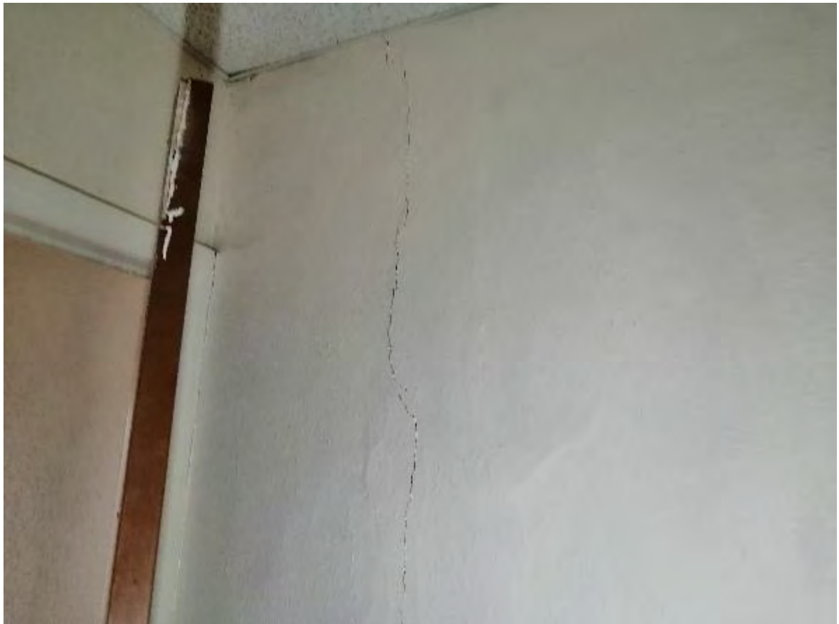
Photo 124 – Wall Plaster Crack (Front Room 1)
