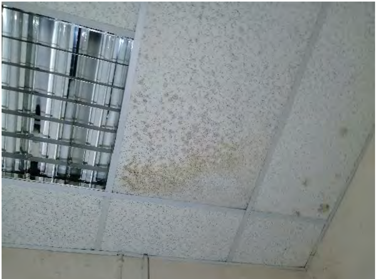
Photo 166 – Condensation Damp (Male Toilets)
