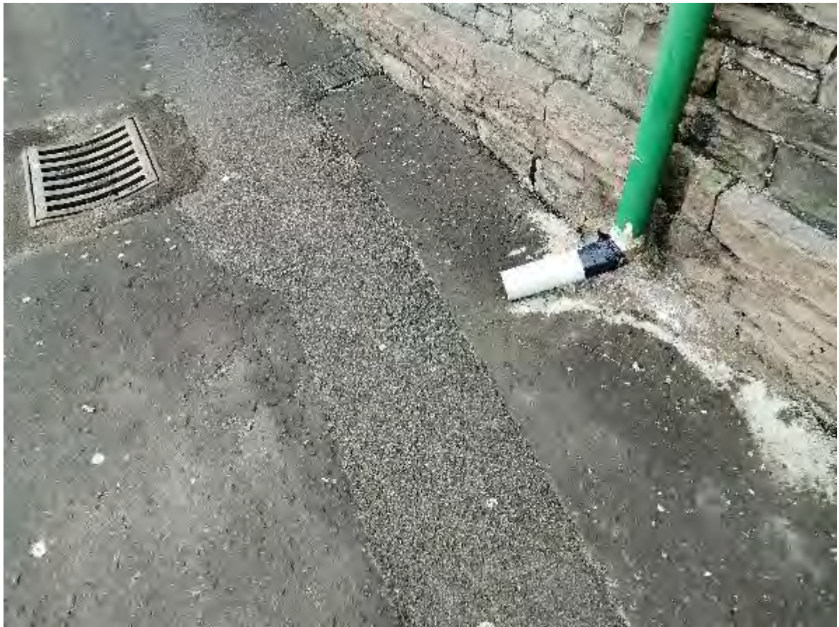
Photo 248 – No Drainage to Remove Water from Wall (Front Wall Elevation)
