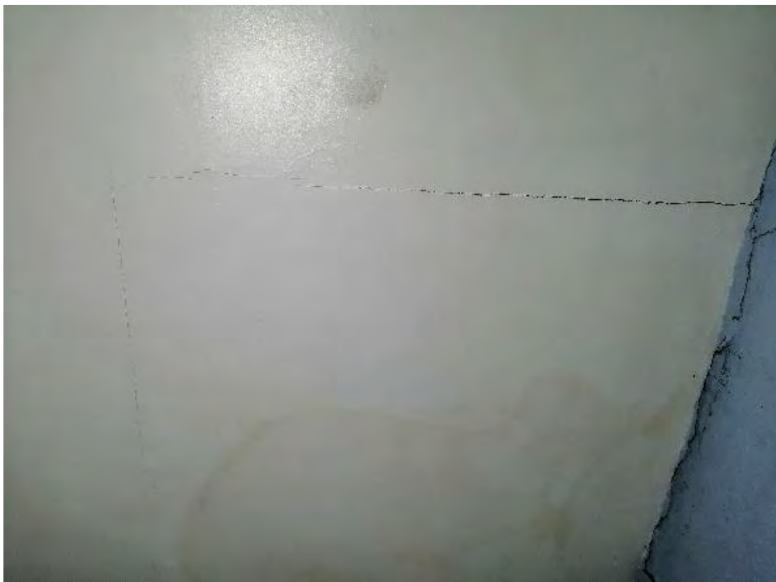
Photo 102 – Ceiling Cracking (Rear Room)
