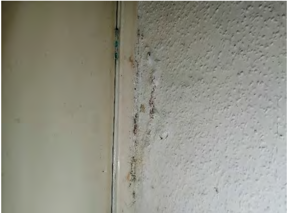
Photo 224 – Penetrating Damp (Corridor 1)
