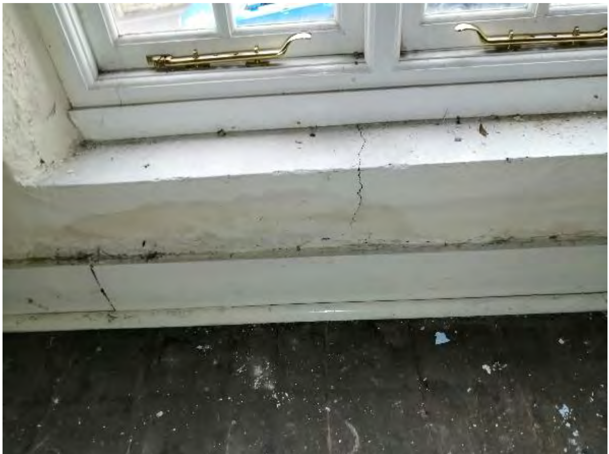
Photo 130 – Wall Plaster Crack (Front Room 1)
