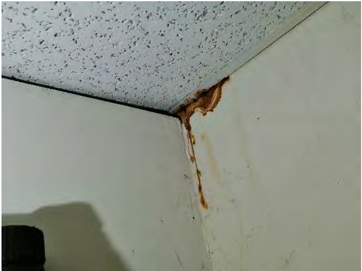
Photo 159 – Penetrating Damp (Front Room 1)
