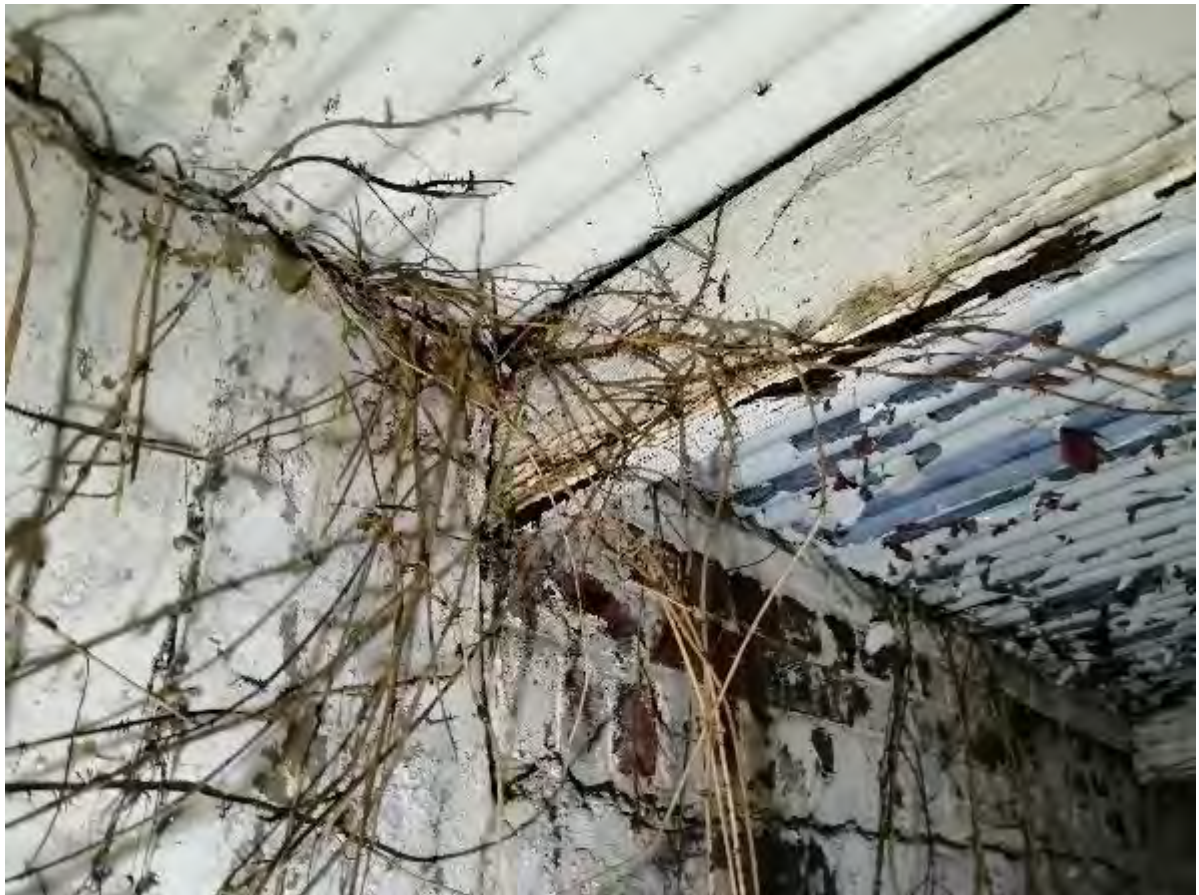
Photo 220 – Rot to Roof Purlin (Fire Exit Room)
