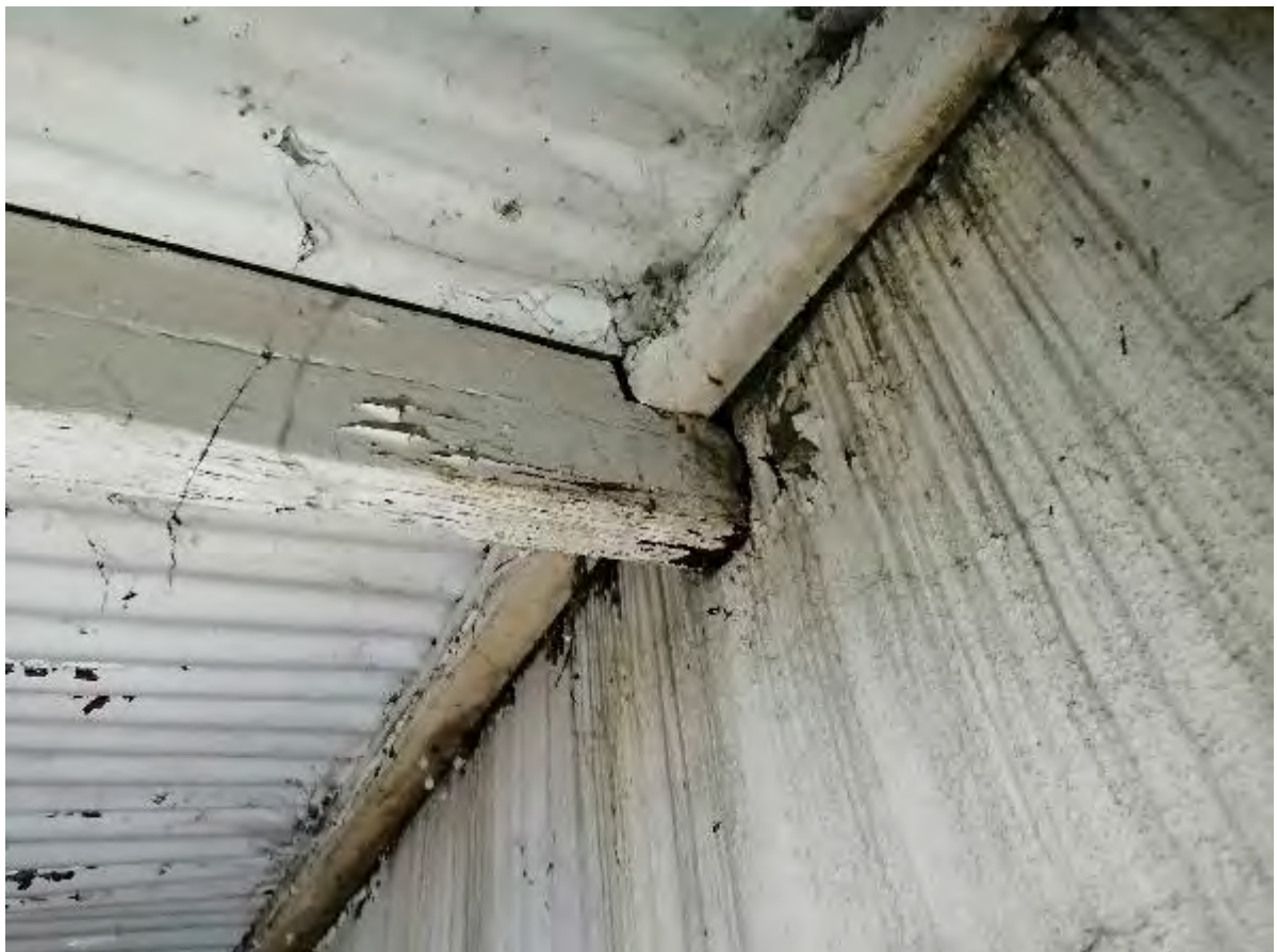
Photo 222 – Rot to Roof Purlin (Fire Exit Room)
