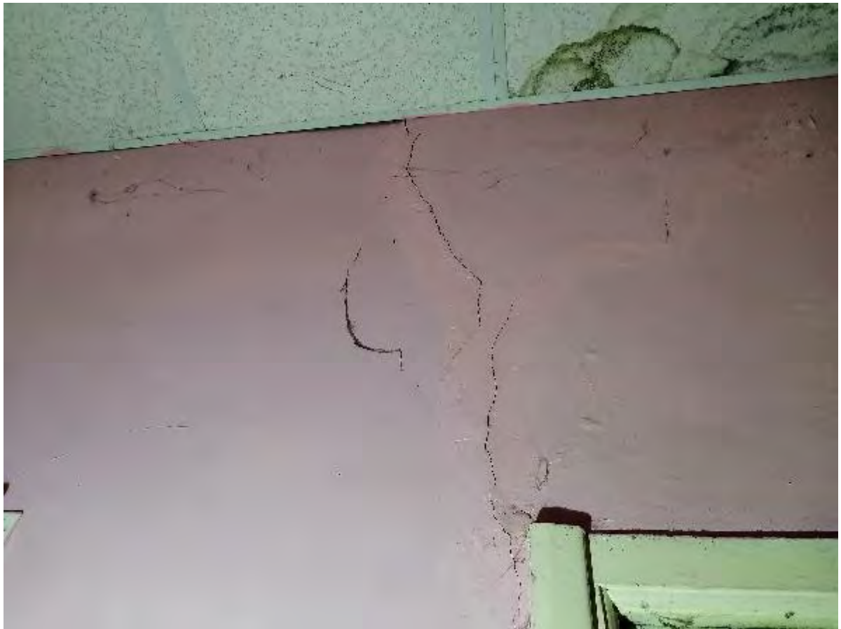
Photo 189 – Wall Plaster Cracking (Corridor 2)
