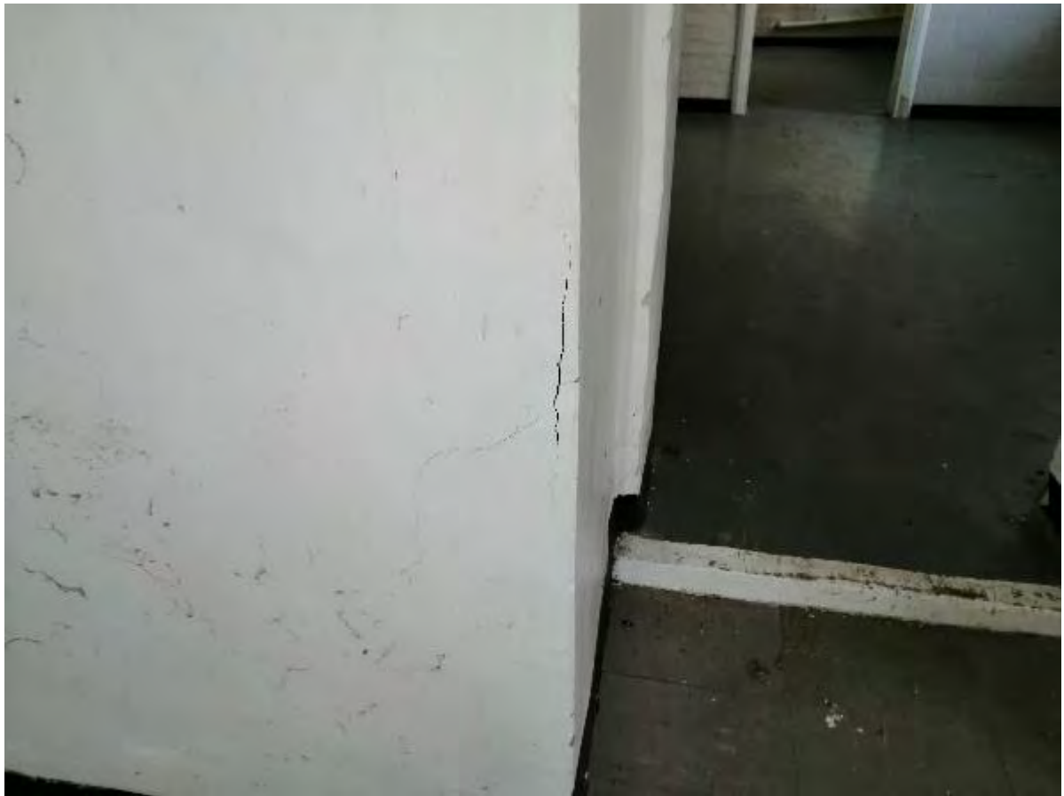
Photo 195 – Wall Plaster Cracking and Detached Plaster (Side Room 1)
