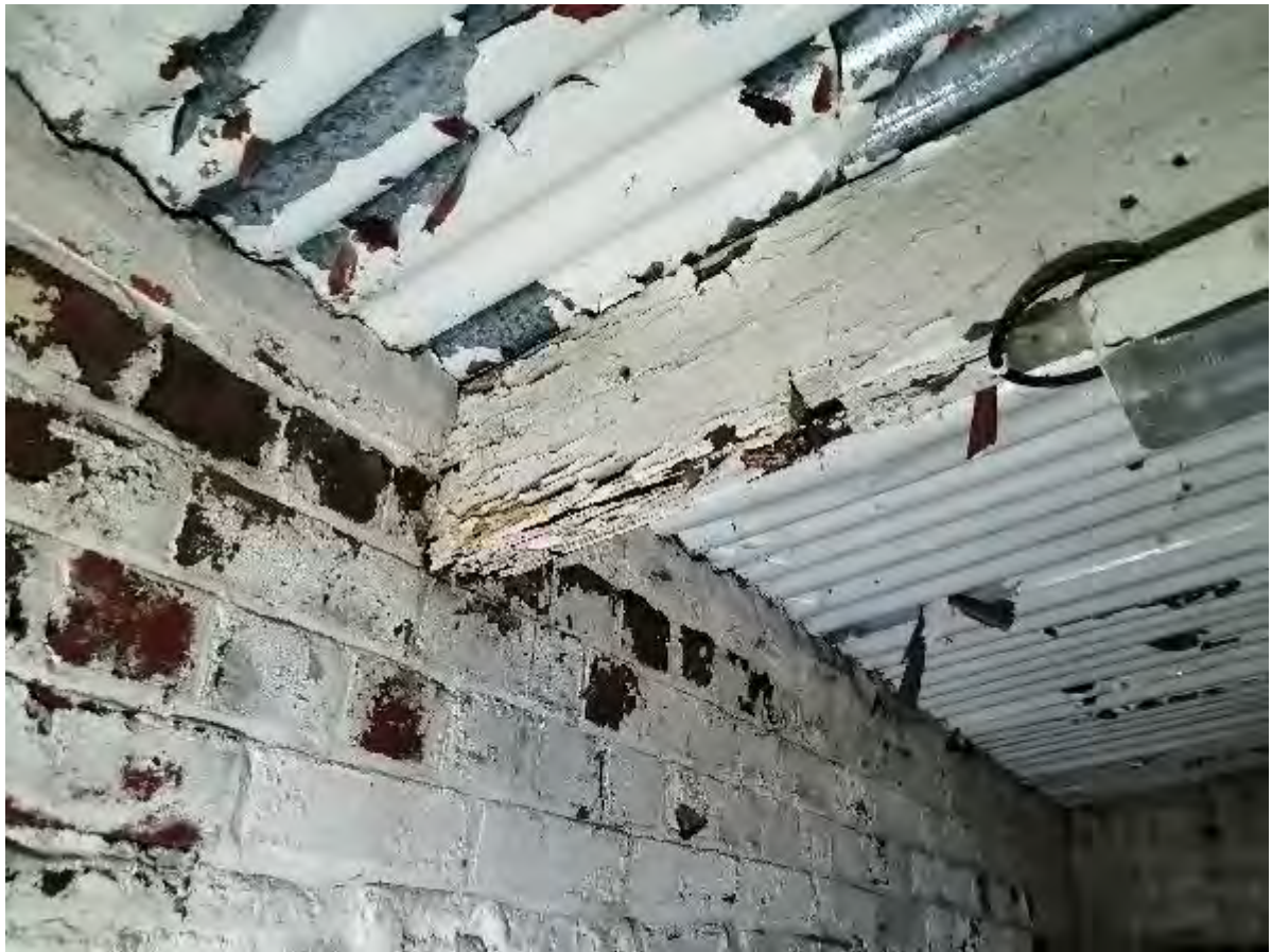
Photo 221 – Rot to Roof Purlin (Fire Exit Room)
