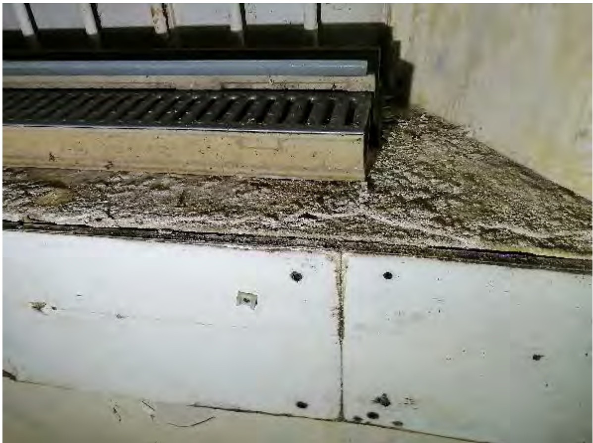
Photo 234 – Penetrating Damp (Utility Room 1)
