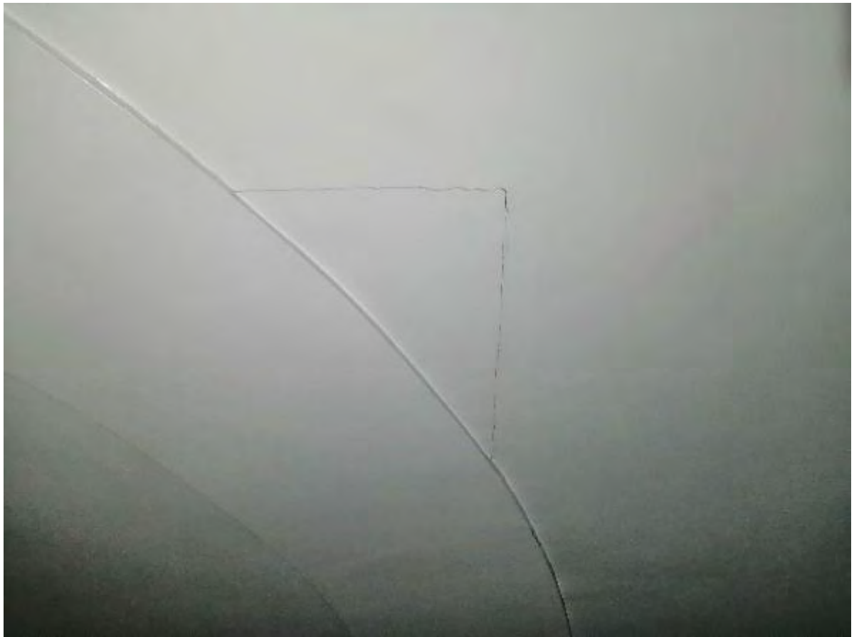
Photo 110 – Ceiling Cracking (Rear Room)
