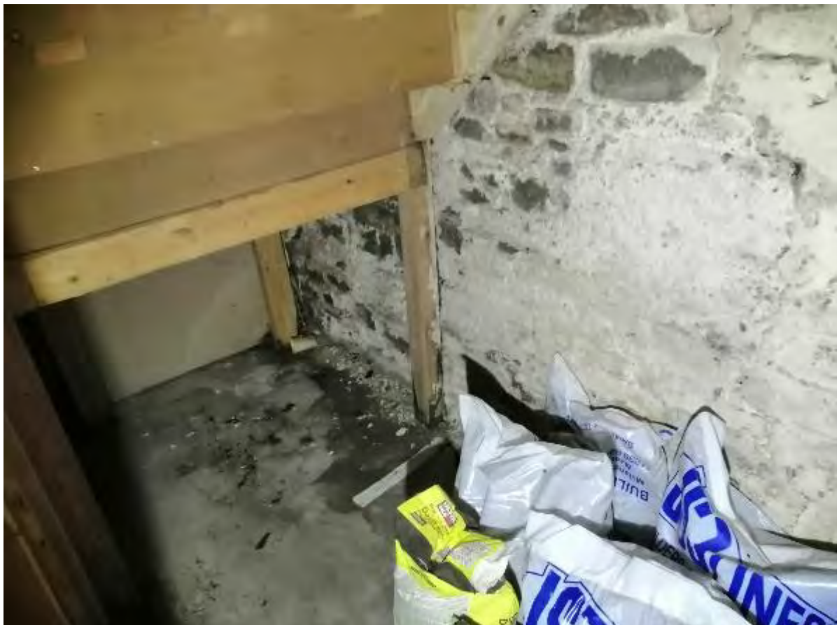
Photo 226 – Rising Damp (Under Staircase)
