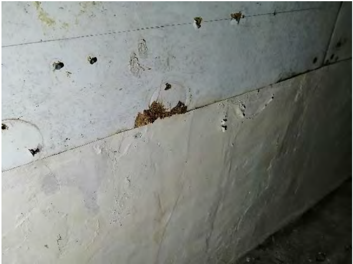
Photo 235 – Penetrating Damp (Utility Room 1)
