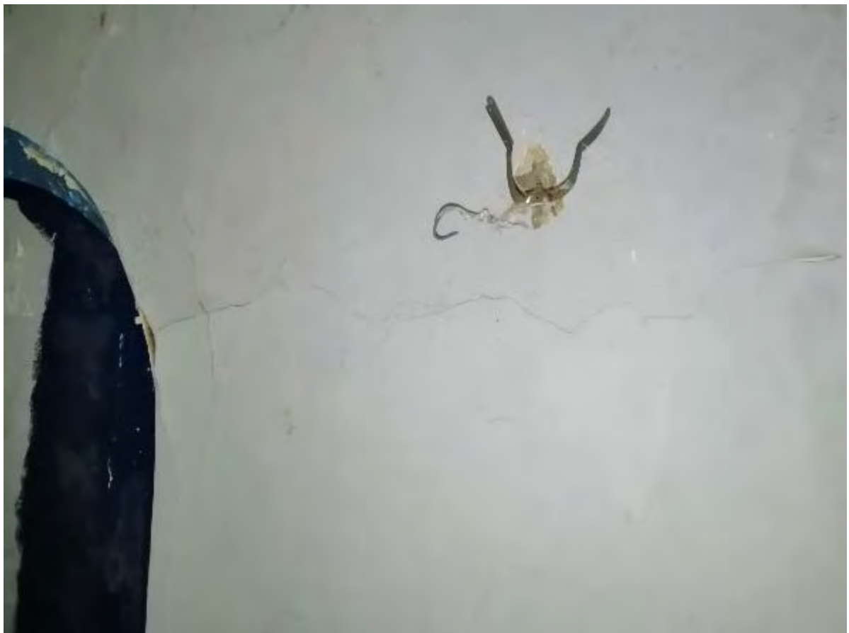
Photo 116 – Wall Plaster Crack (Rear Room)
