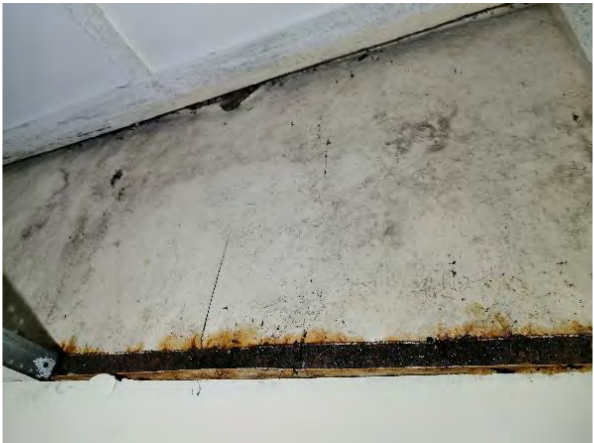
Photo 160 – Penetrating Damp (Front Room 1)
