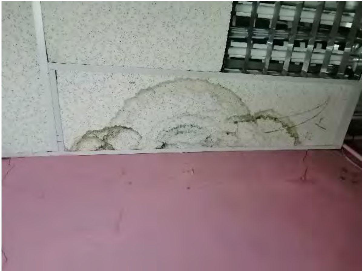
Photo 227 – Penetrating Damp (Corridor 2)
