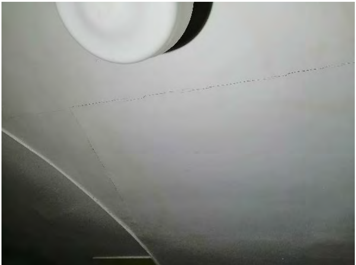
Photo 104 – Ceiling Cracking (Rear Room)
