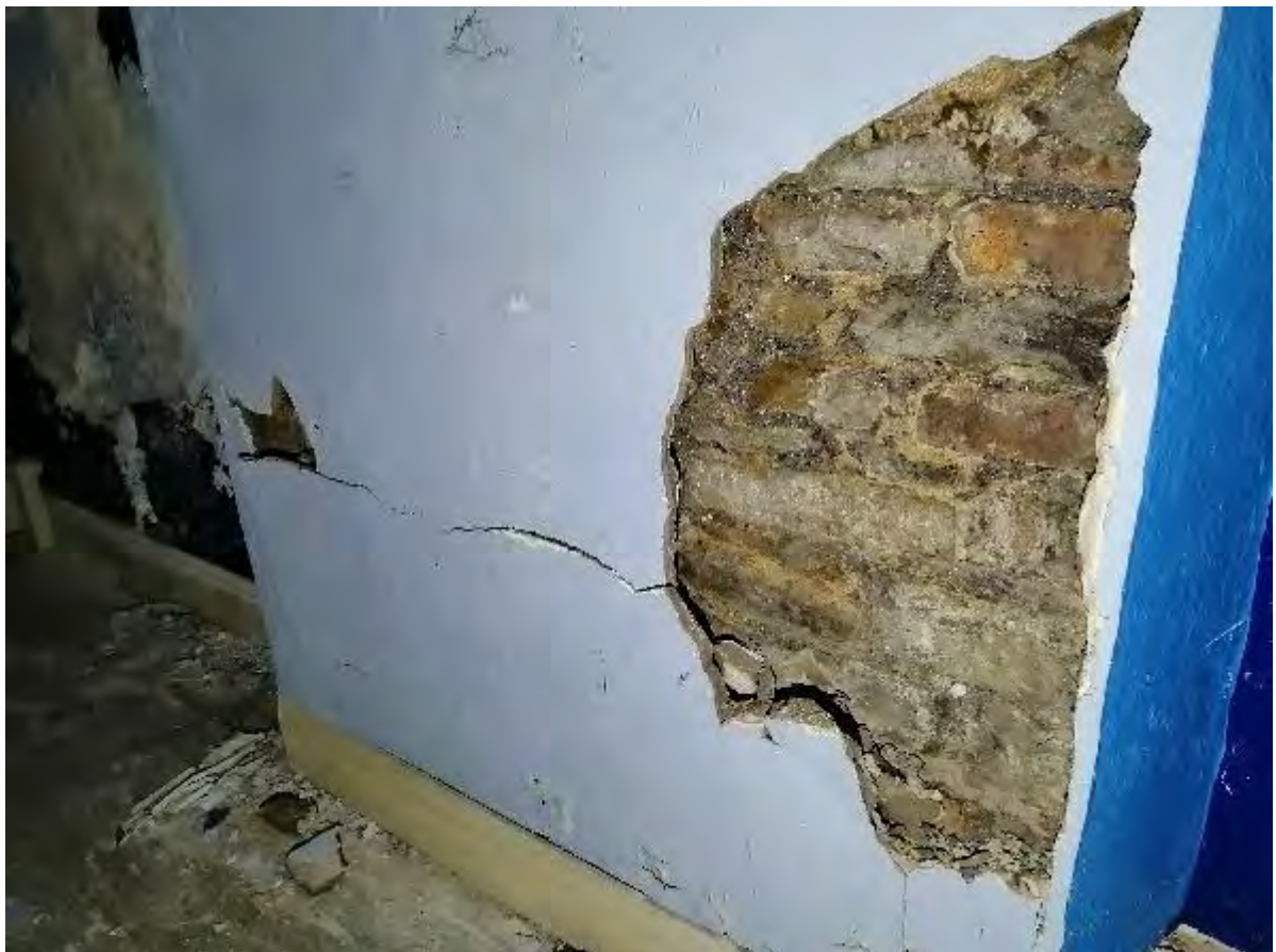
Photo 118 – Detached Wall Plaster (Rear Room)
