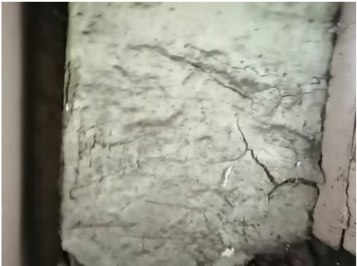
Photo 188 – Wall Plaster Cracking to Archway Behind Stud Wall (Front Room)
