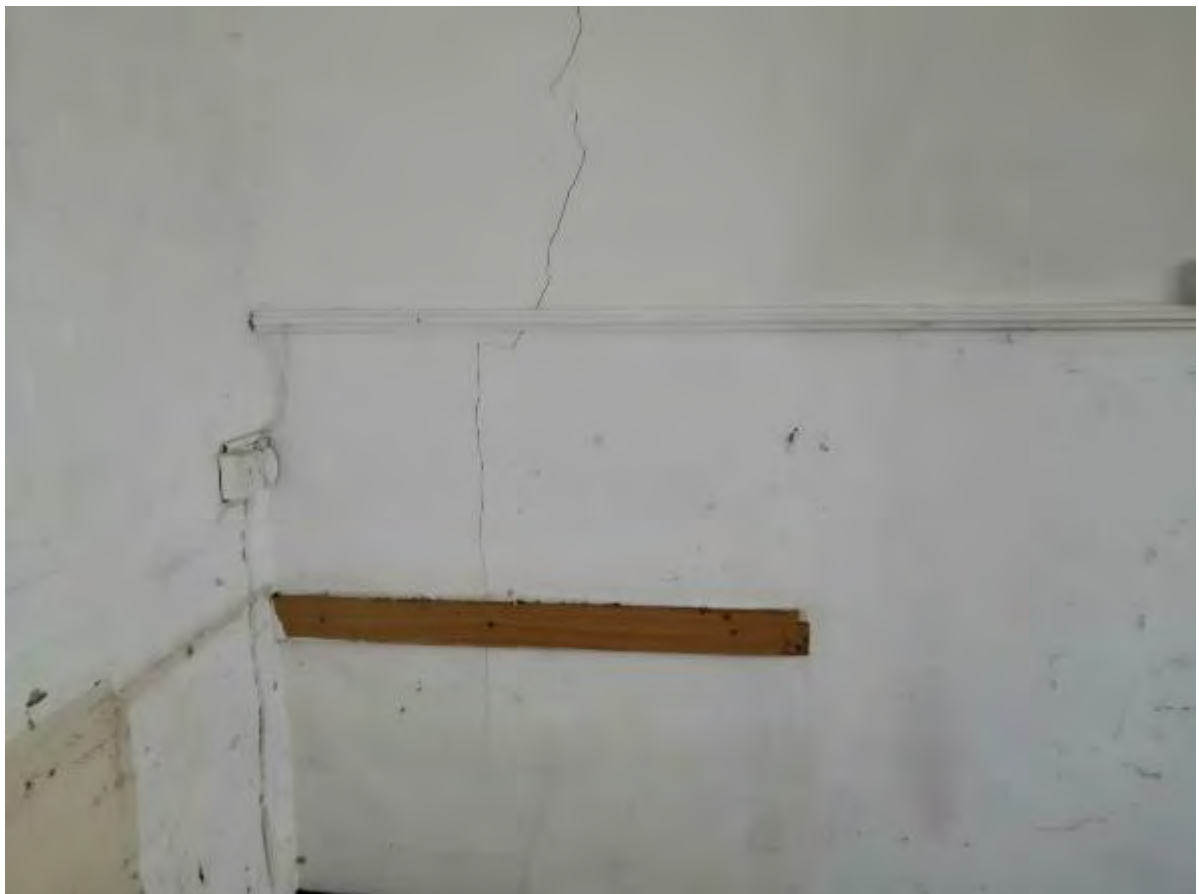
Photo 194 – Wall Plaster Cracking (Side Room 1)
