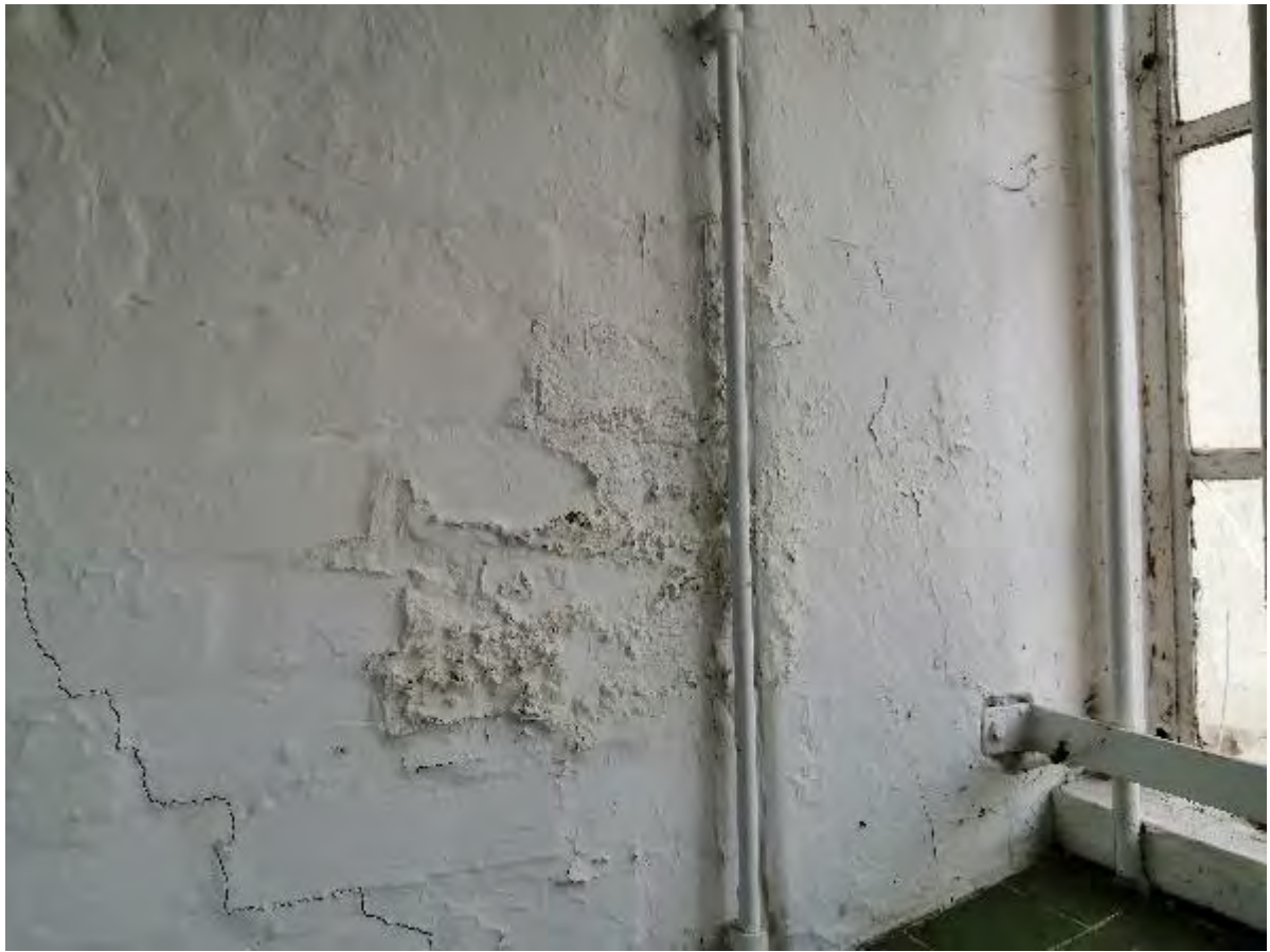
Photo 231 – Penetrating Damp (Kitchen)
