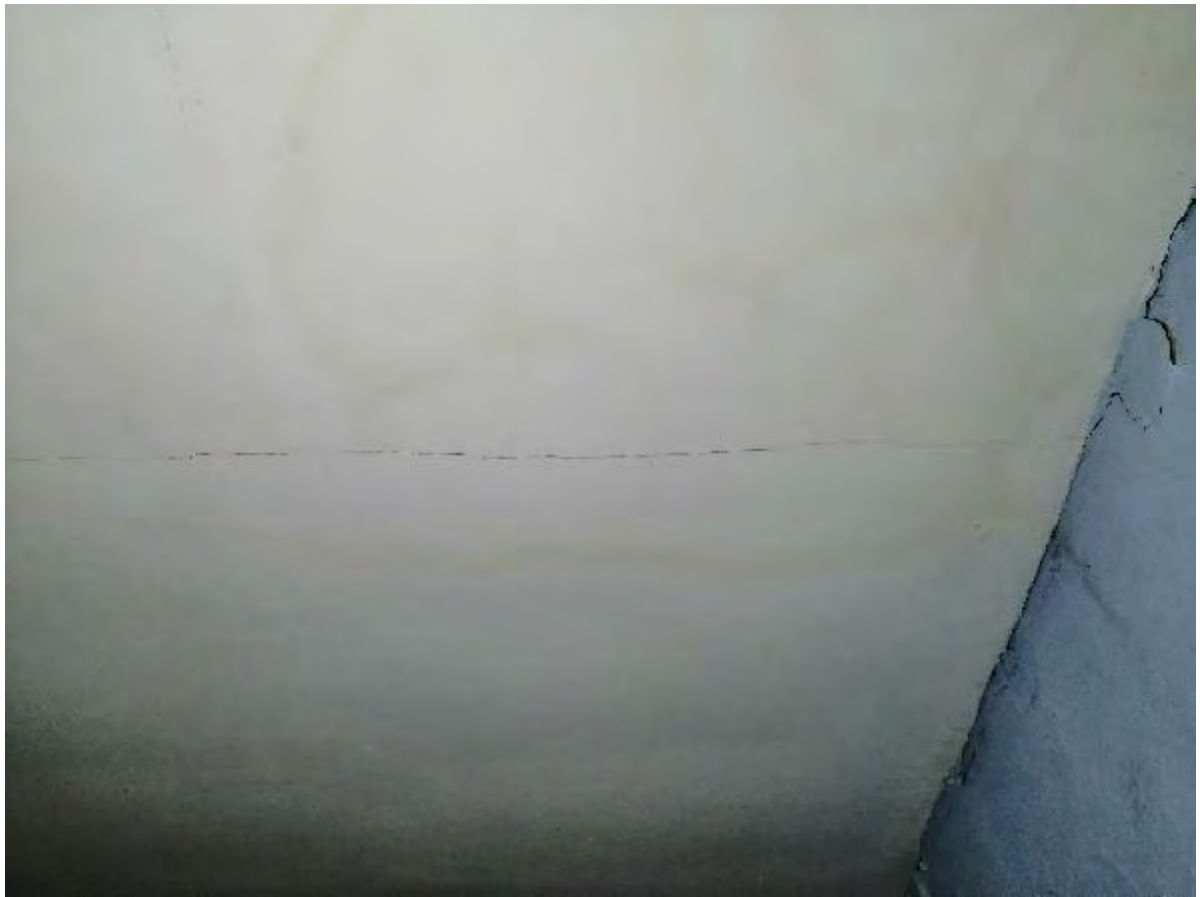
Photo 103 – Ceiling Cracking (Rear Room)
