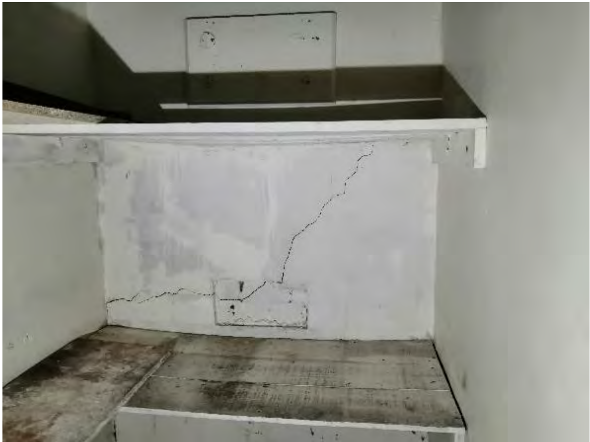
Photo 201 – Stepped Internal Wall Crack (Utility Room 2)
