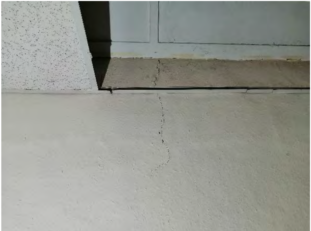
Photo 126 – Wall Plaster Crack (Front Room 1)
