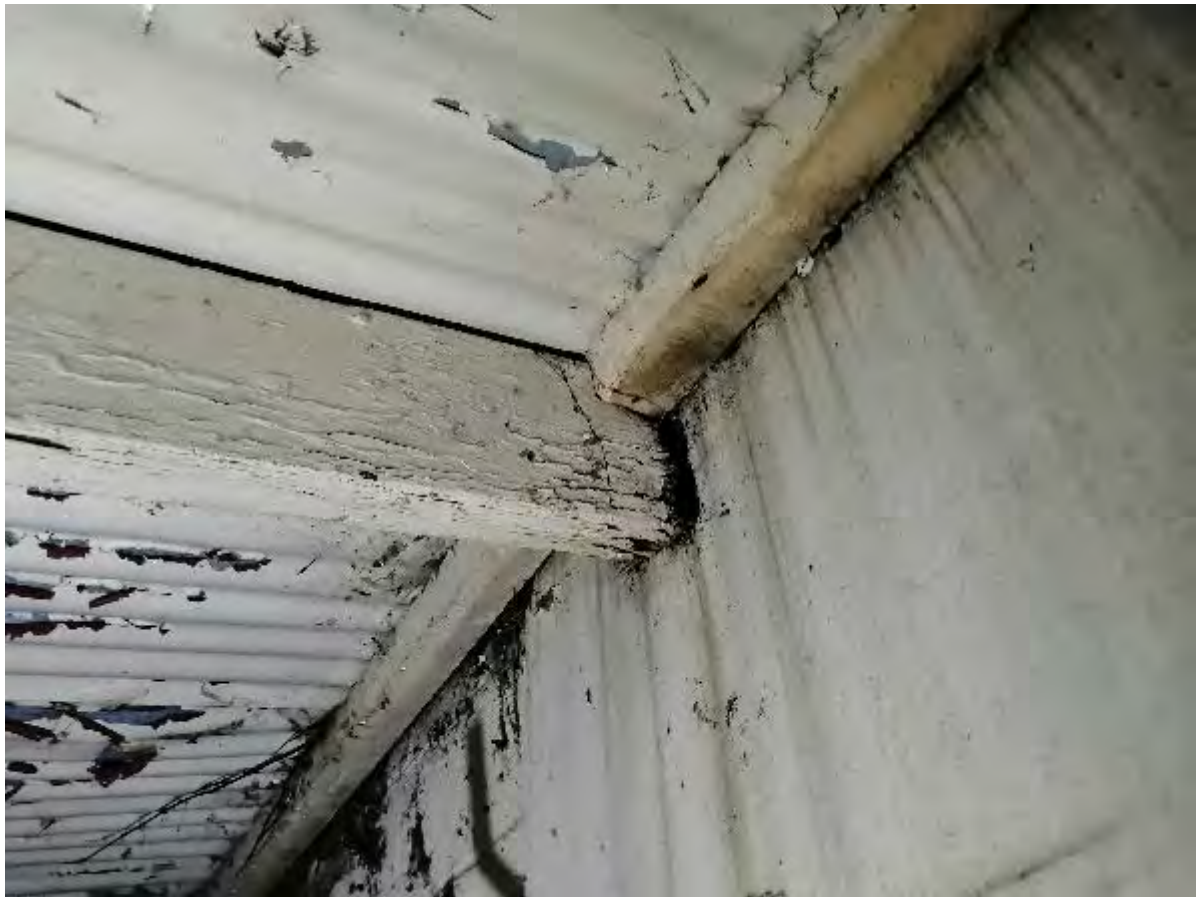
Photo 219 – Rot to Roof Purlin (Fire Exit Room)
