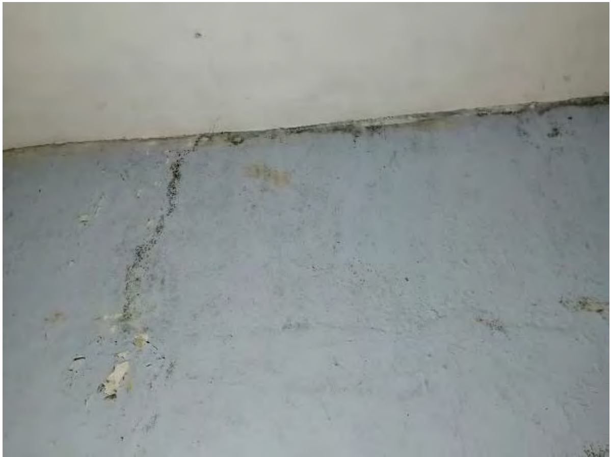
Photo 141 – Penetrating Damp (Rear Room)
