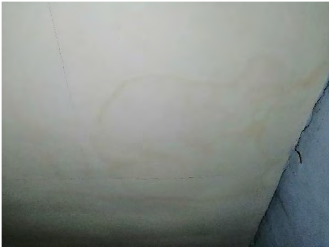
Photo 139 – Penetrating Damp (Rear Room)
