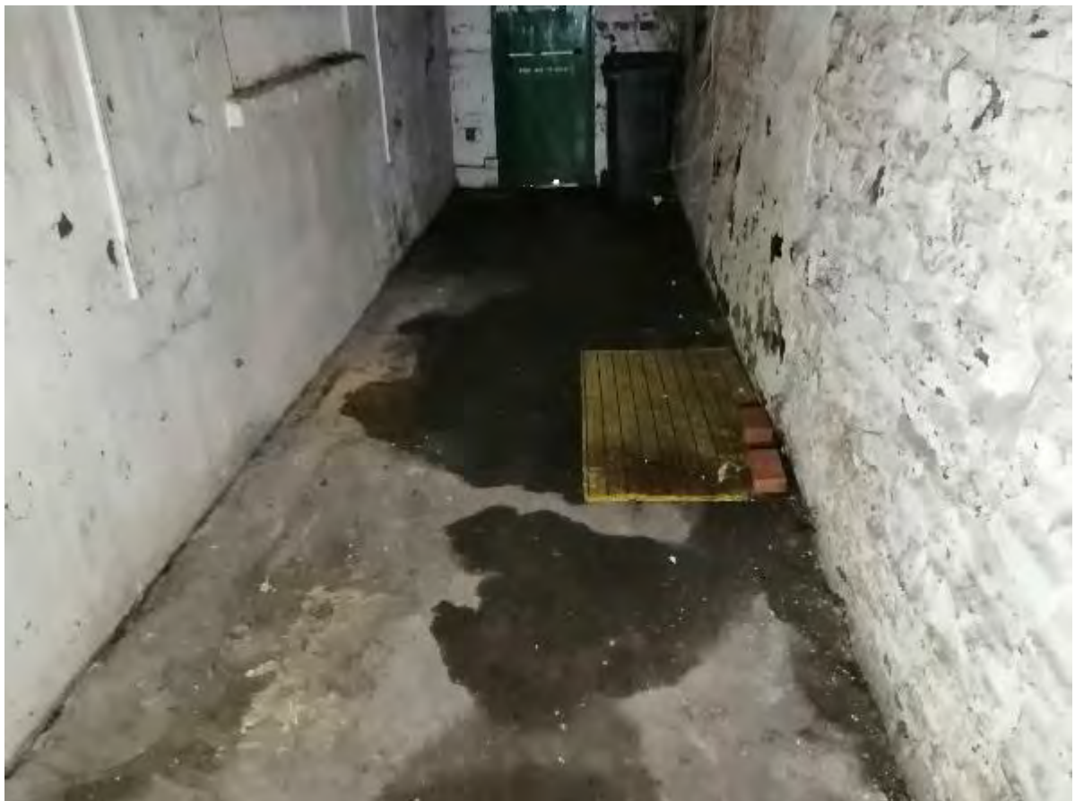
Photo 244 – Penetrating Damp (Fire Exit Room)
