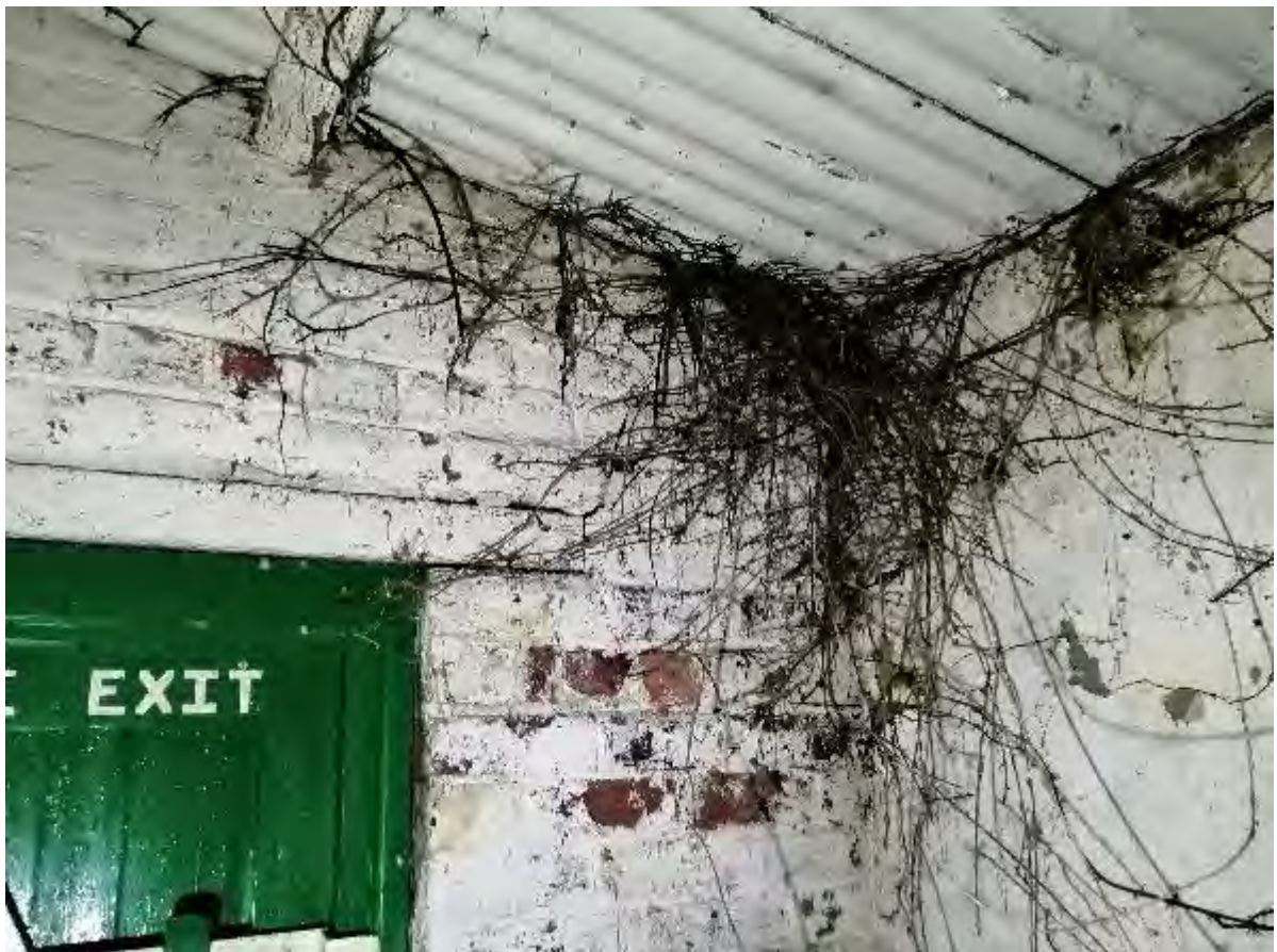
Photo 210 – Internal Vegetation Growth (Fire Exit Room)
