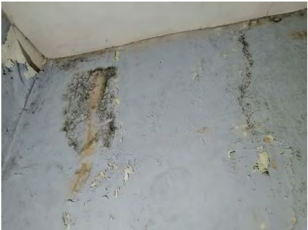
Photo 142 – Penetrating Damp (Rear Room)
