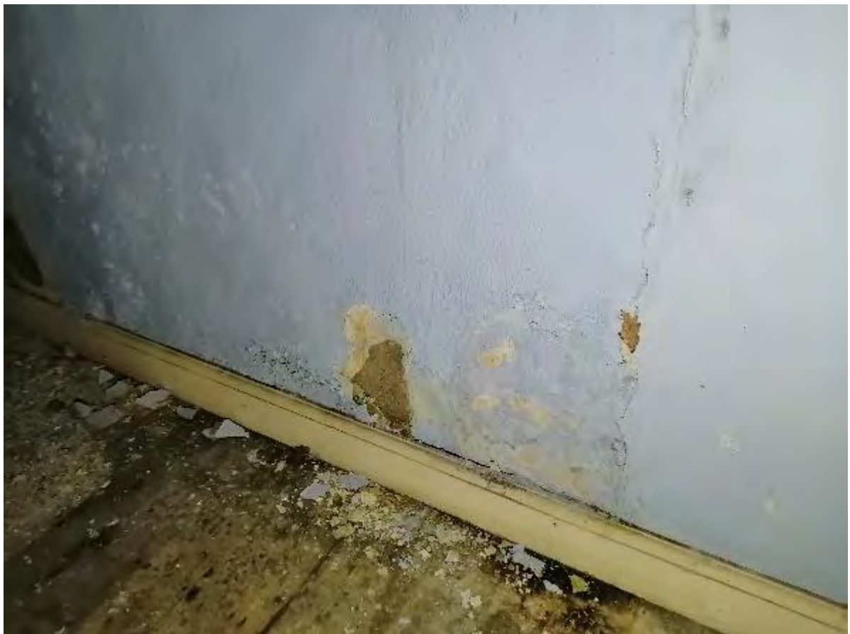
Photo 150 – Penetrating Damp (Rear Room)
