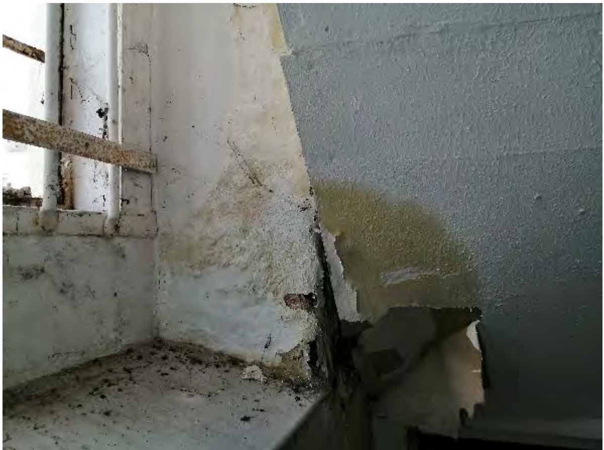
Photo 230 – Penetrating Damp (Side Room 1)
