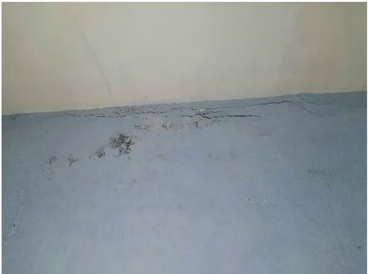
Photo 146 – Condensation Damp (Rear Room)
