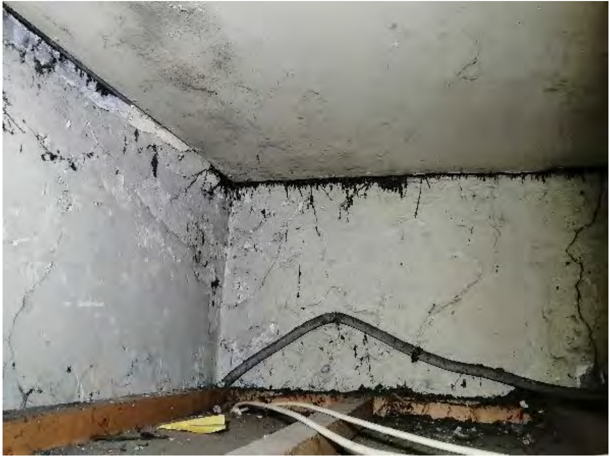
Photo 133 – Wall Plaster Crack (Front Room 1)
