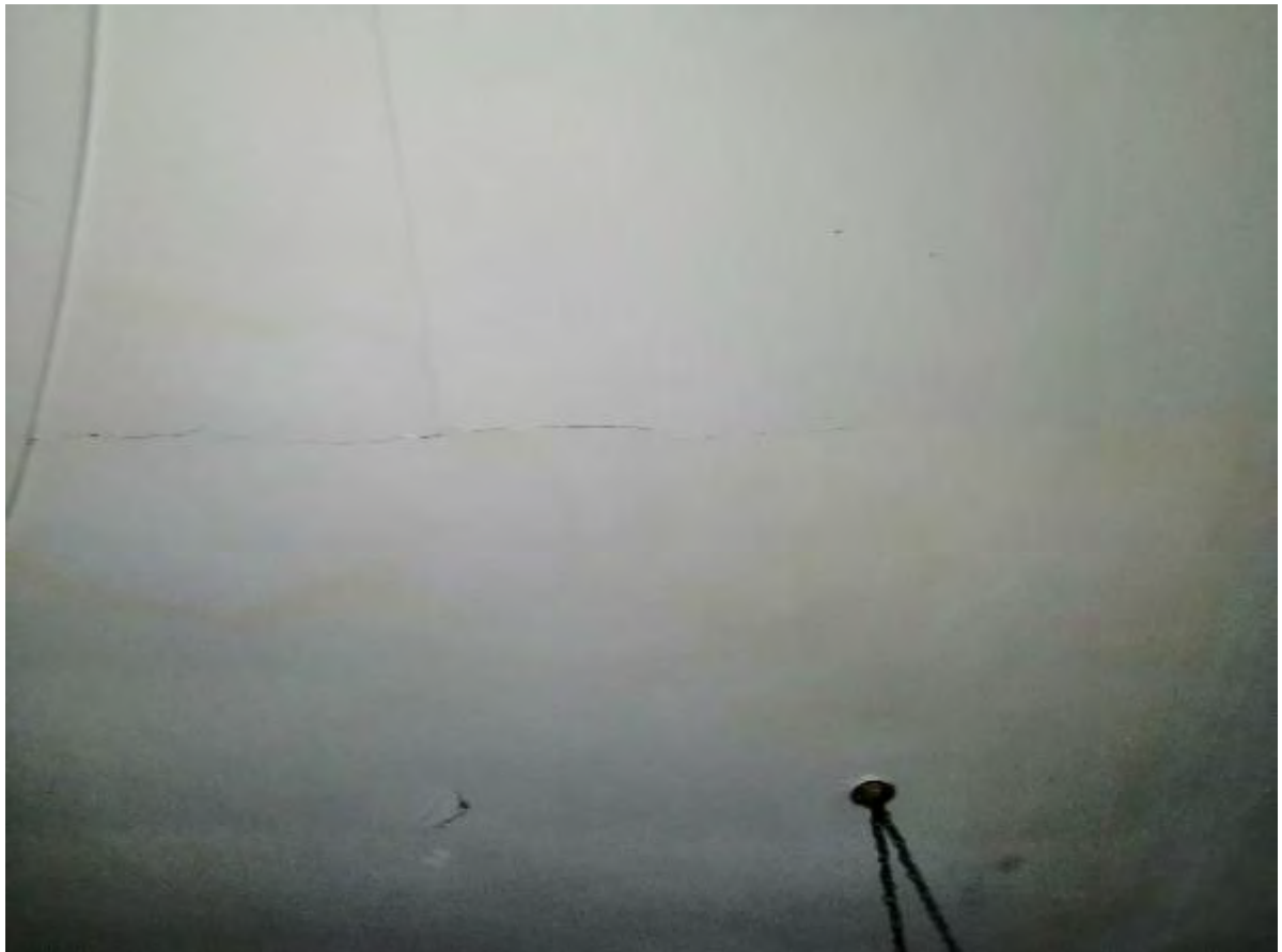
Photo 108 – Ceiling Cracking (Rear Room)
