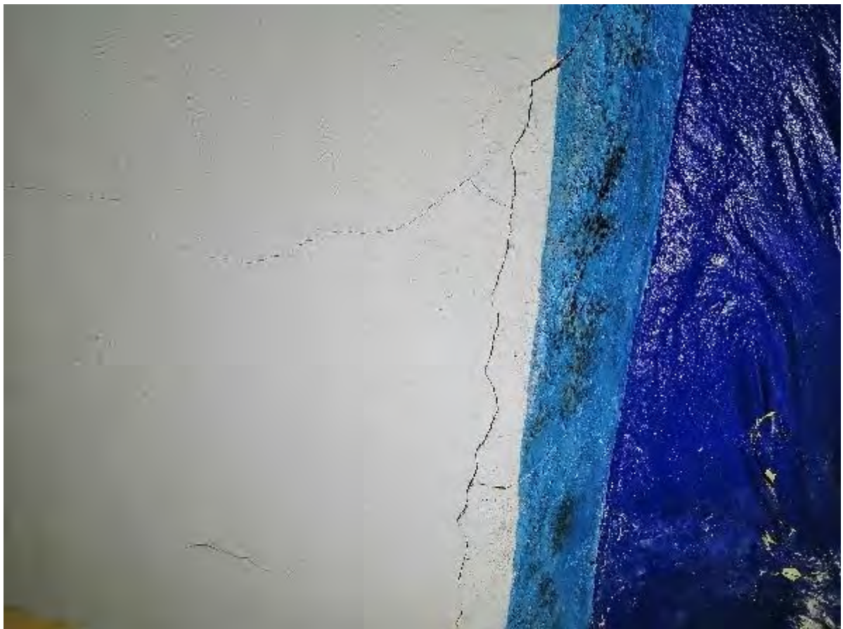
Photo 120 – Wall Plaster Crack (Rear Room)
