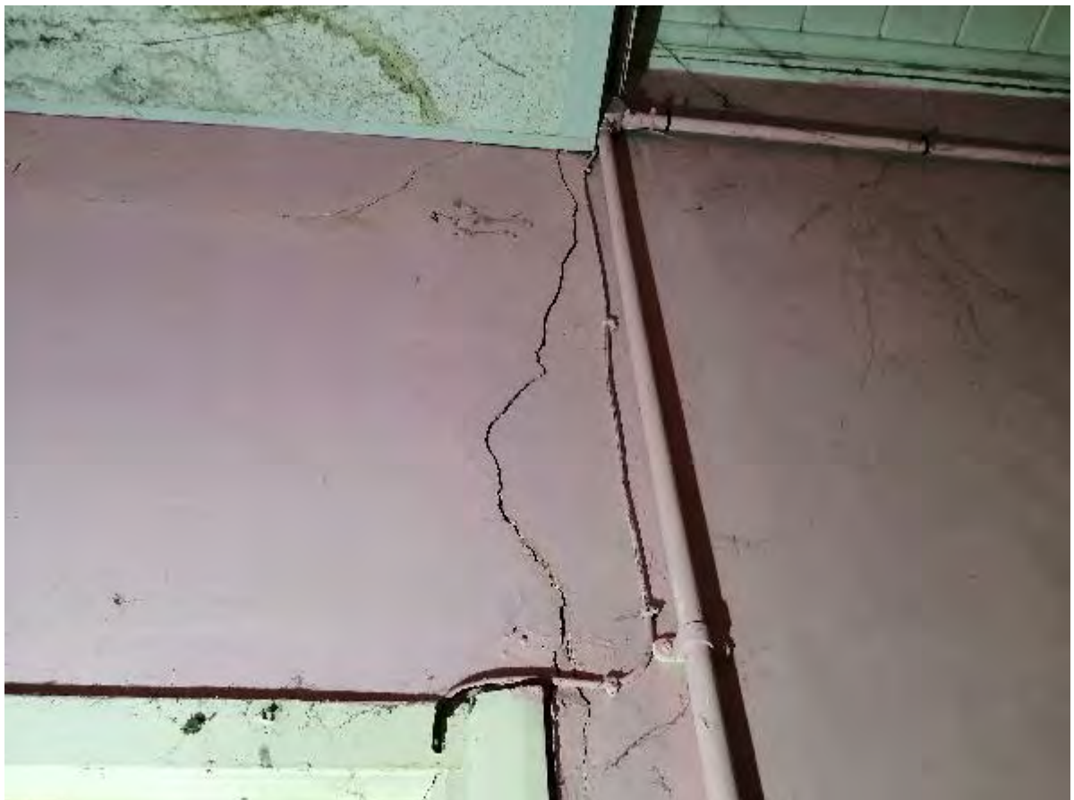
Photo 190 – Wall Plaster Cracking (Corridor 2)
