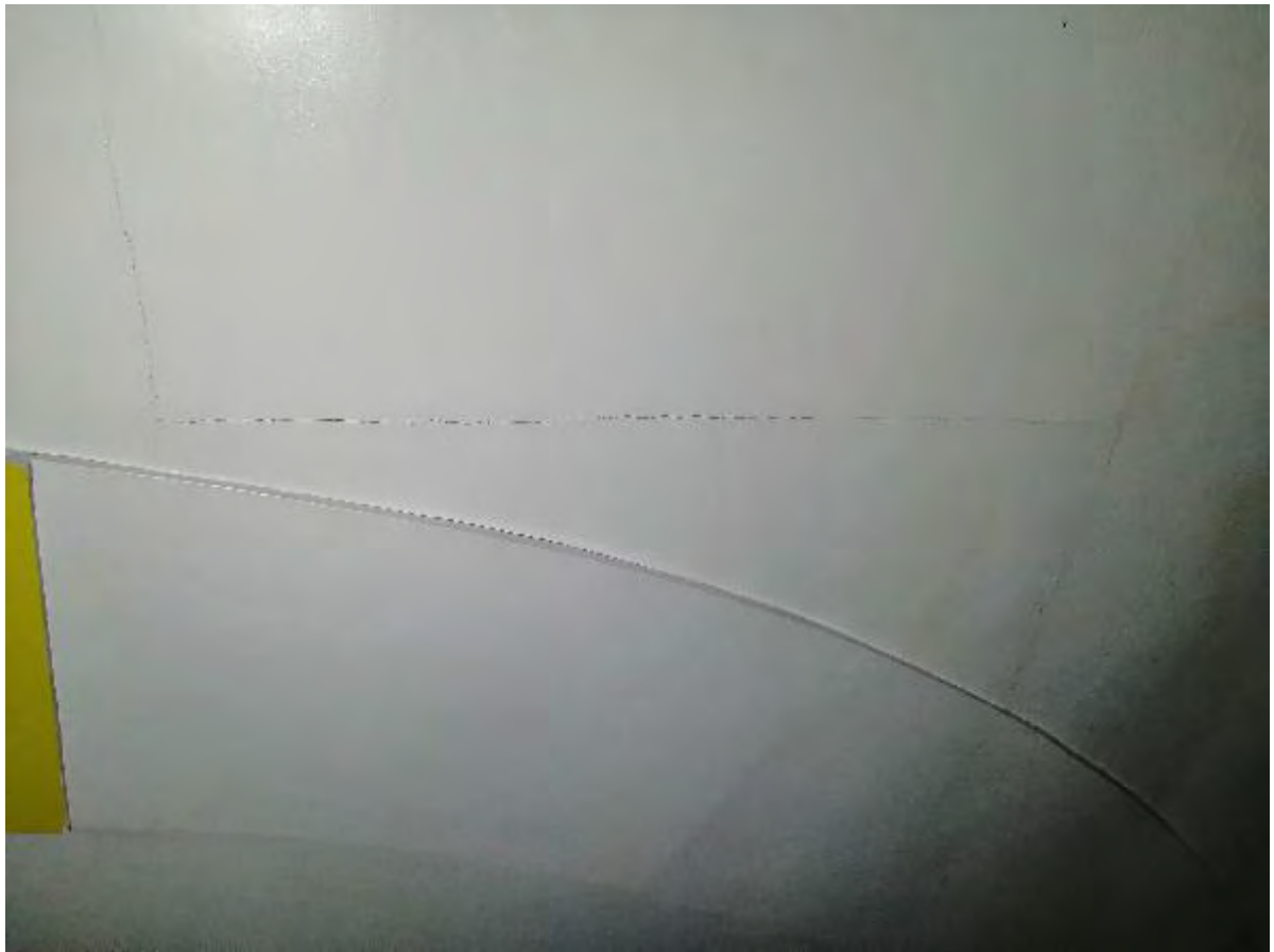
Photo 107 – Ceiling Cracking (Rear Room)
