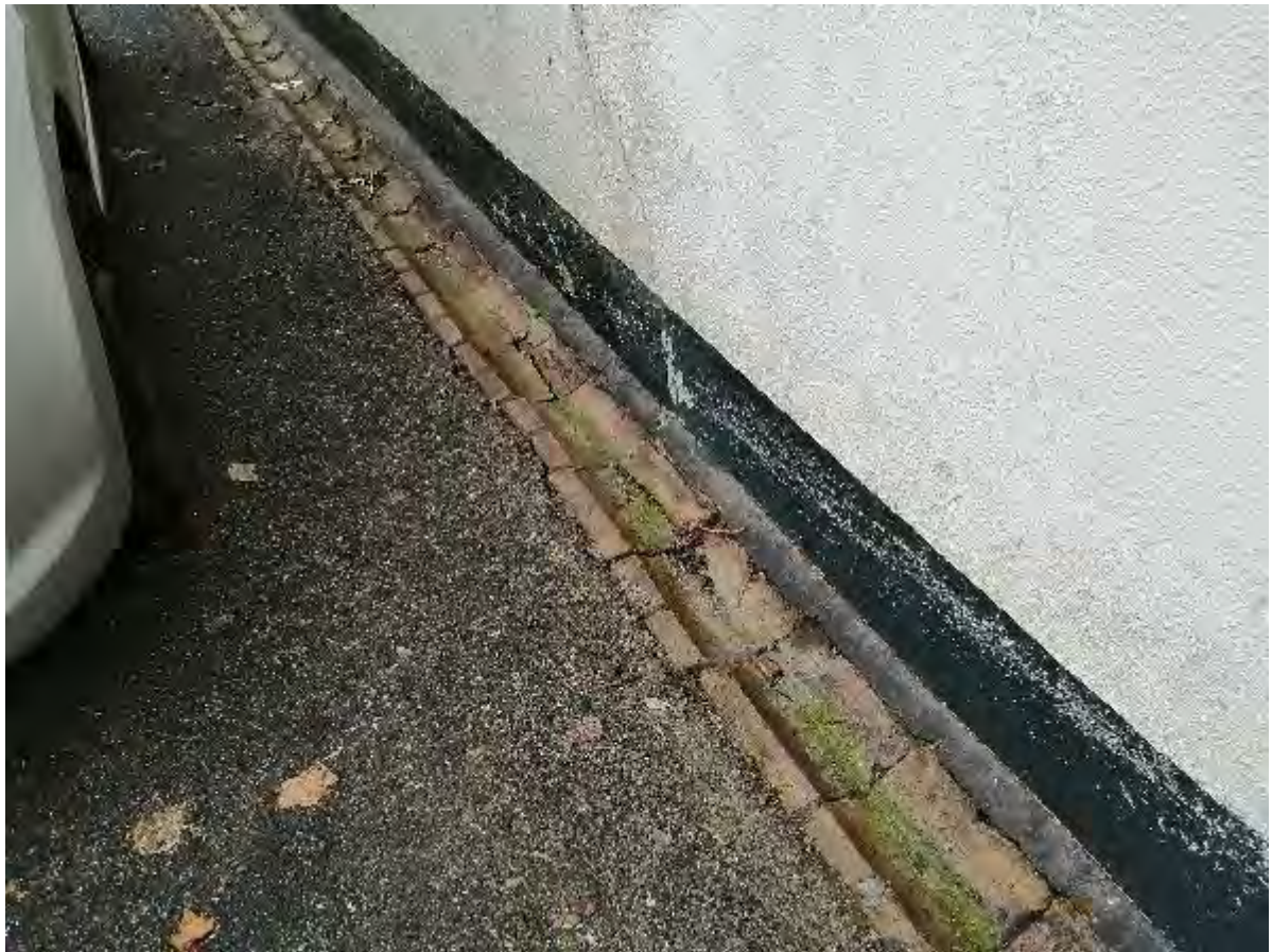
Photo 246 – Defective Drainage Chanel (Right Wall Elevation)
