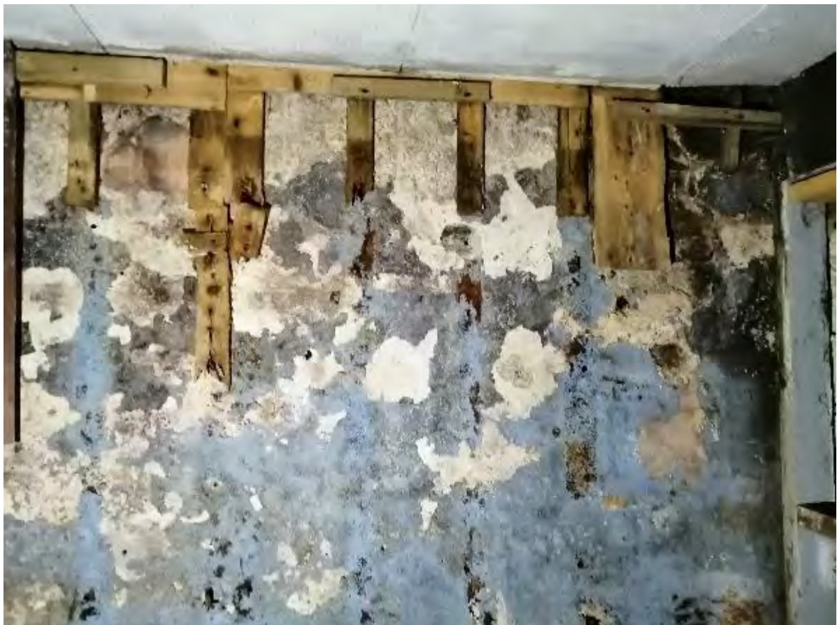
Photo 238 – Penetrating Damp (Hall)
