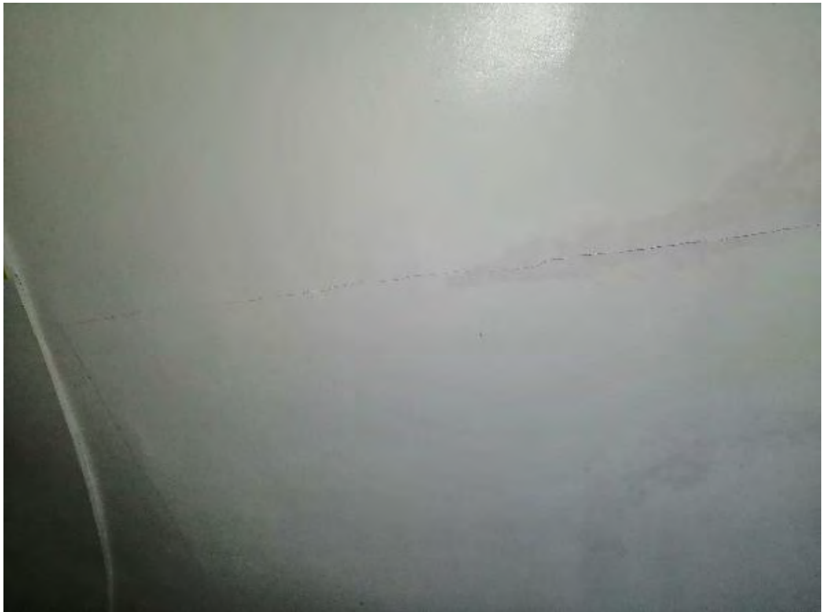
Photo 106 – Ceiling Cracking (Rear Room)
