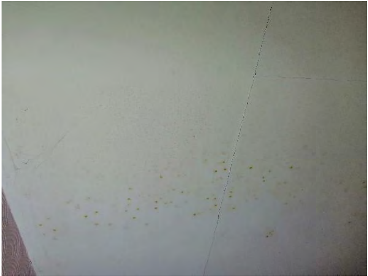
Photo 203 – Ceiling Cracking (Hall)
