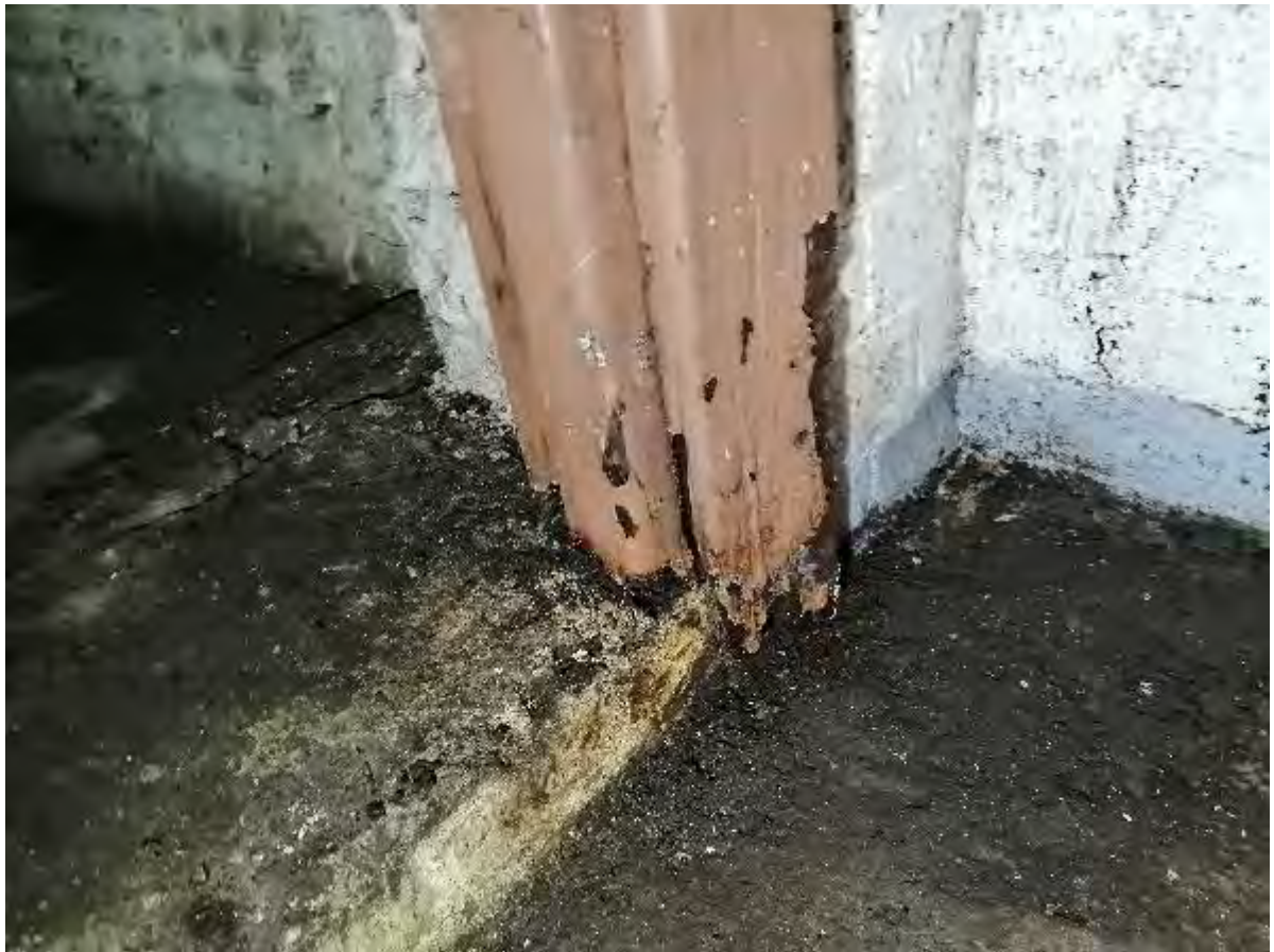
Photo 207 – Rot to Doorway Timber (Corridor 3)
