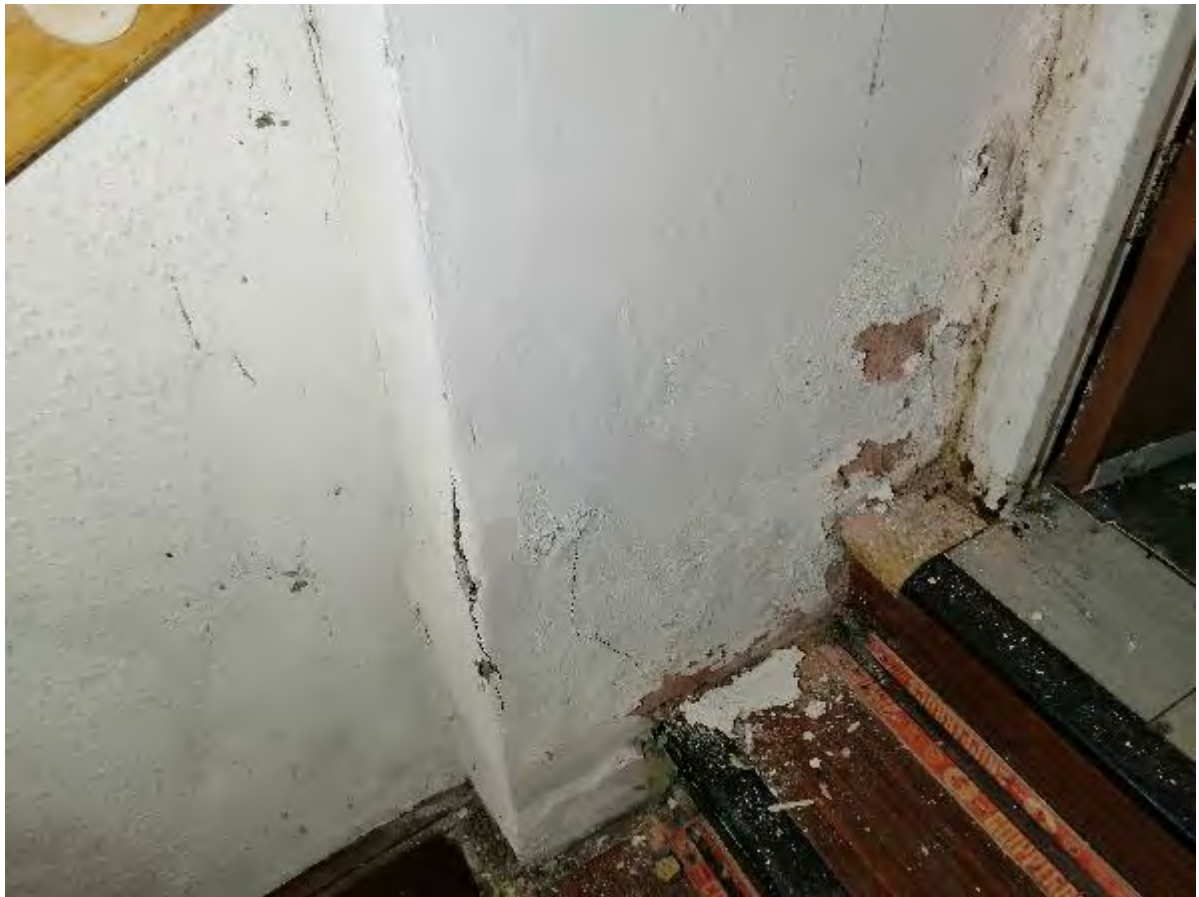
Photo 165 – Penetrating Damp (Staircase)
