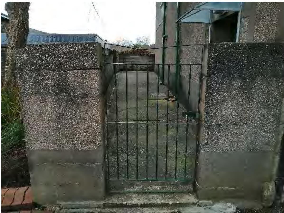
Photo 245 – Cracking to Wall Supporting Entrance Gate
