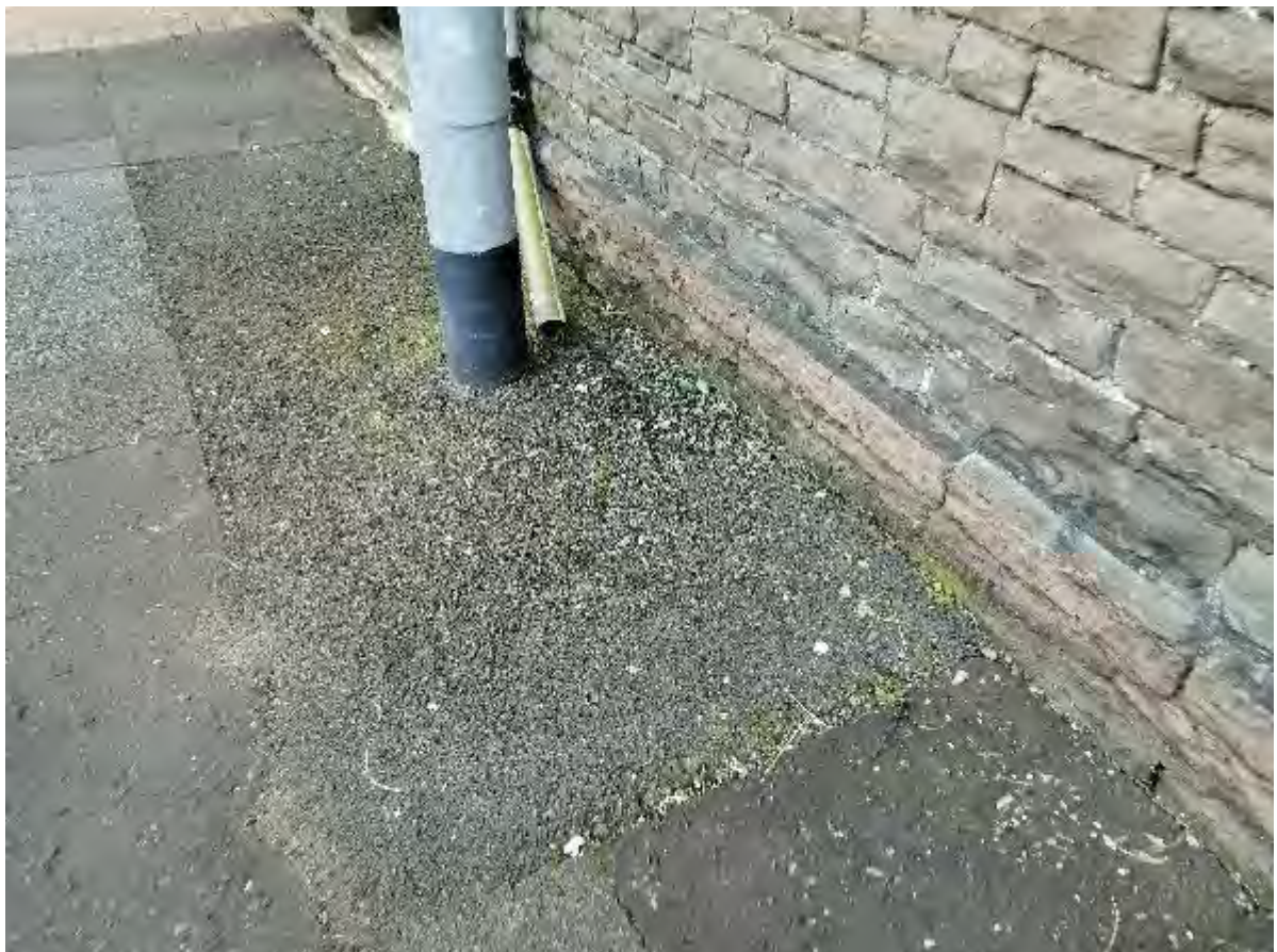
Photo 249 – No Drainage to Remove Water from Wall (Front Wall Elevation)
