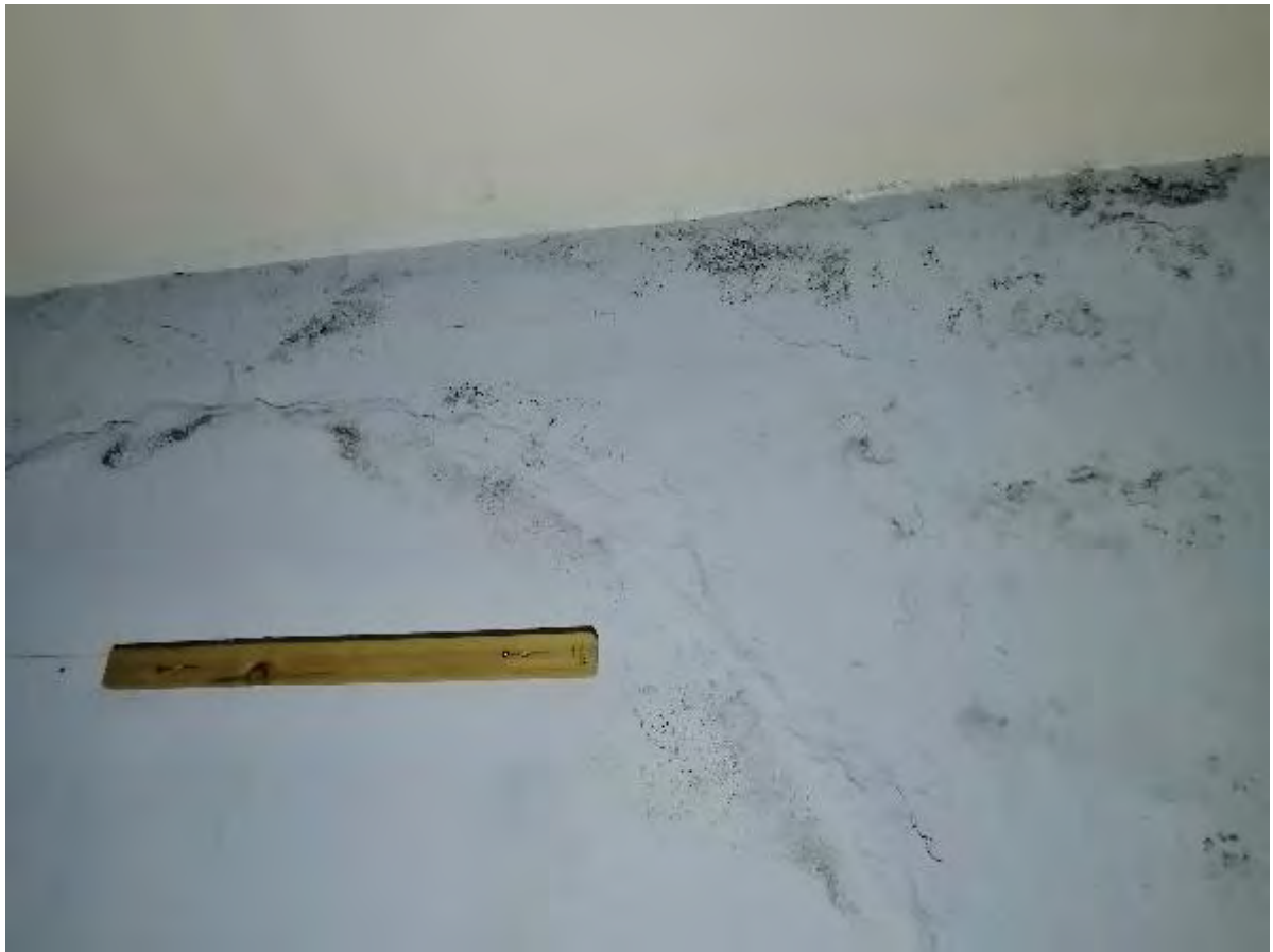
Photo 151 – Condensation Damp (Rear Room)
