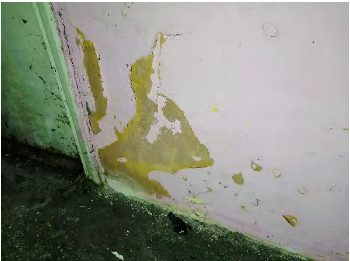
Photo 228 – Penetrating Damp (Corridor 2)
