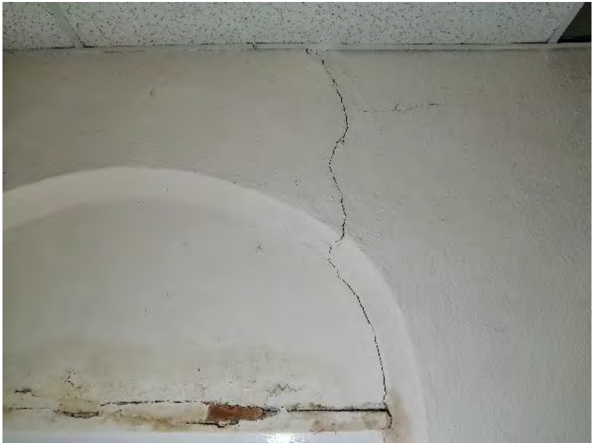
Photo 131 – Wall Crack Above Archway (Front Room 1)
