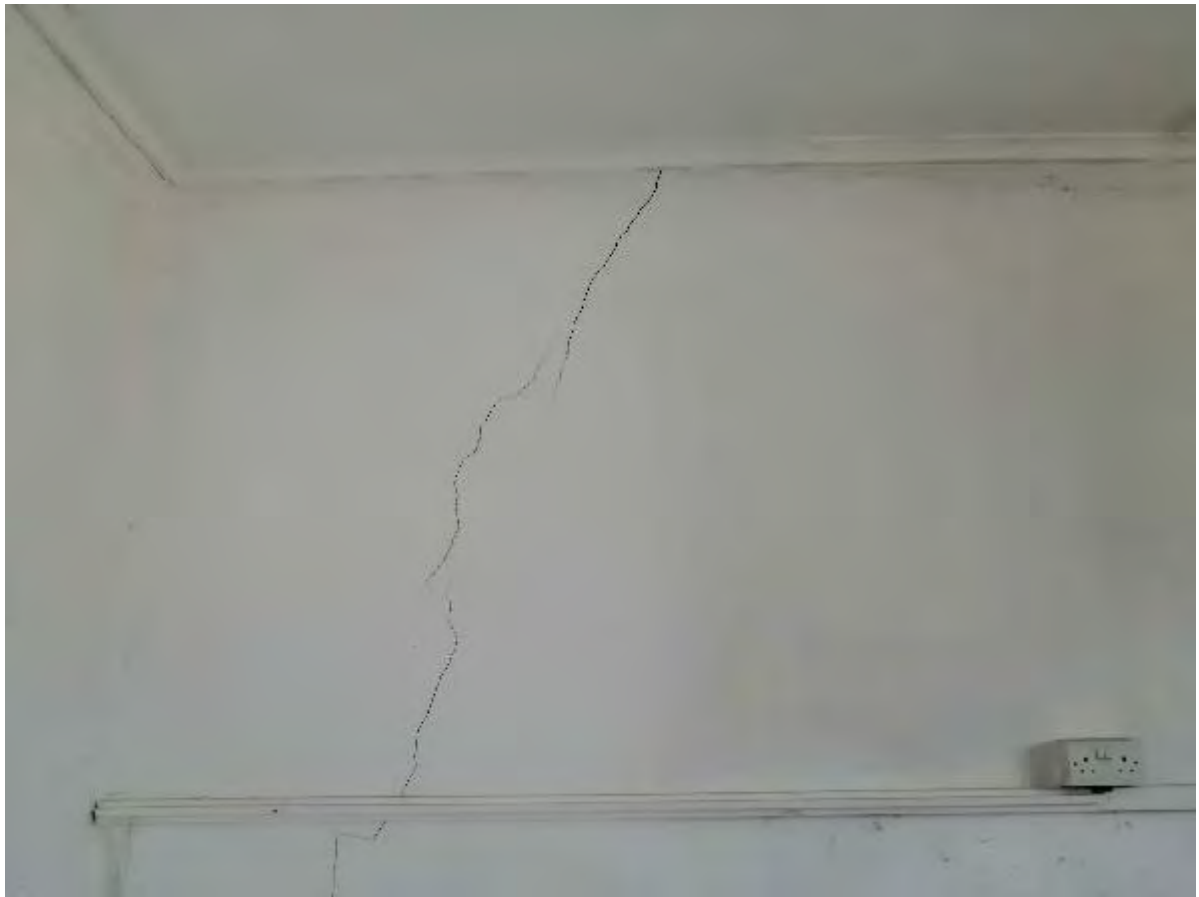
Photo 193 – Wall Plaster Cracking (Side Room 1)
