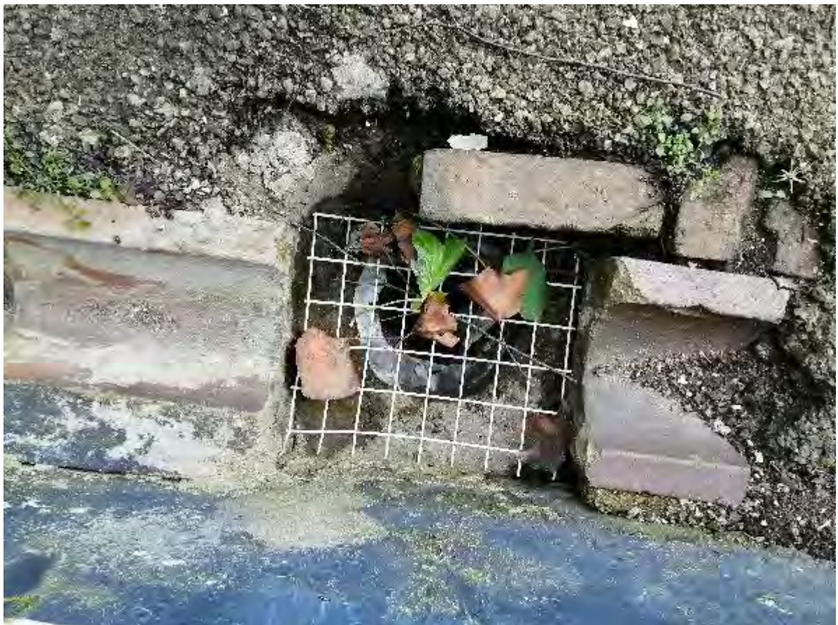
Photo 247 – No Drainage Gully (Right Wall Elevation)
