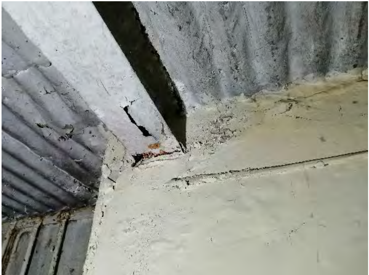
Photo 232 – Penetrating Damp (Utility Room 1)
