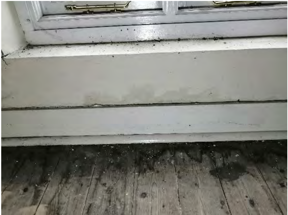
Photo 163 – Penetrating Damp (Front Room 1)
