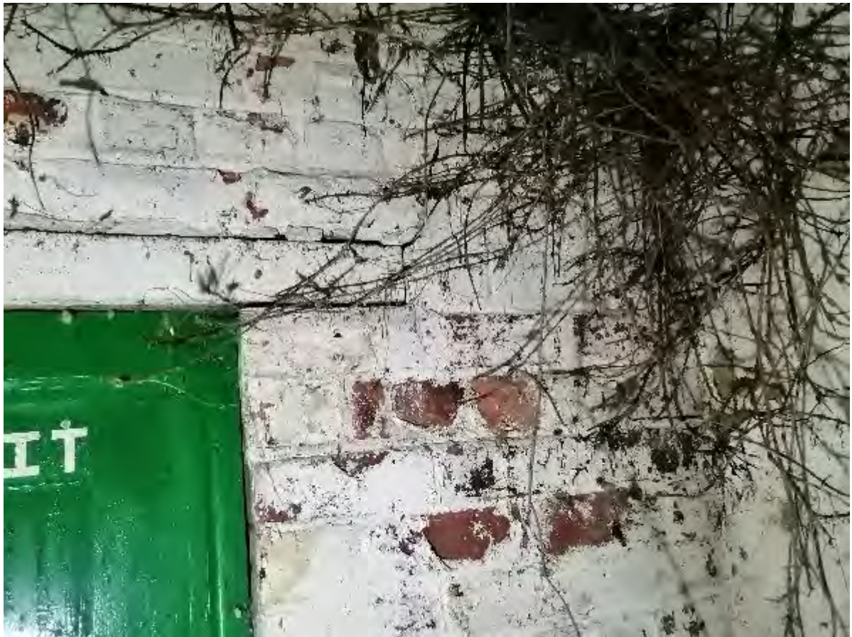
Photo 213 – Cracked Masonry (Fire Exit Room)
