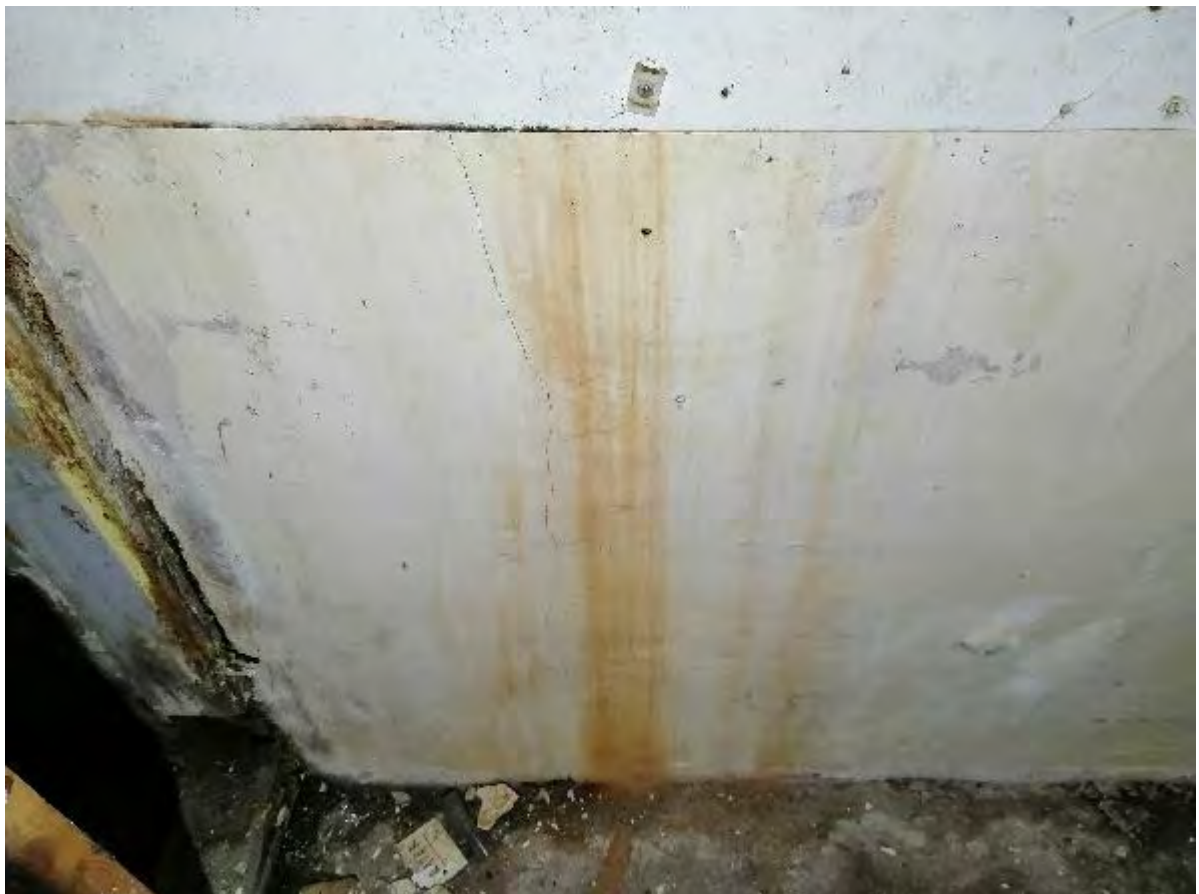
Photo 236 – Penetrating Damp (Utility Room 1)
