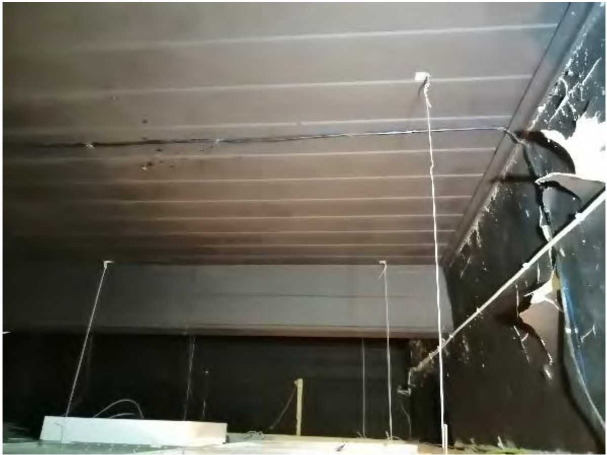
Photo 174 – Void Above Front Room
