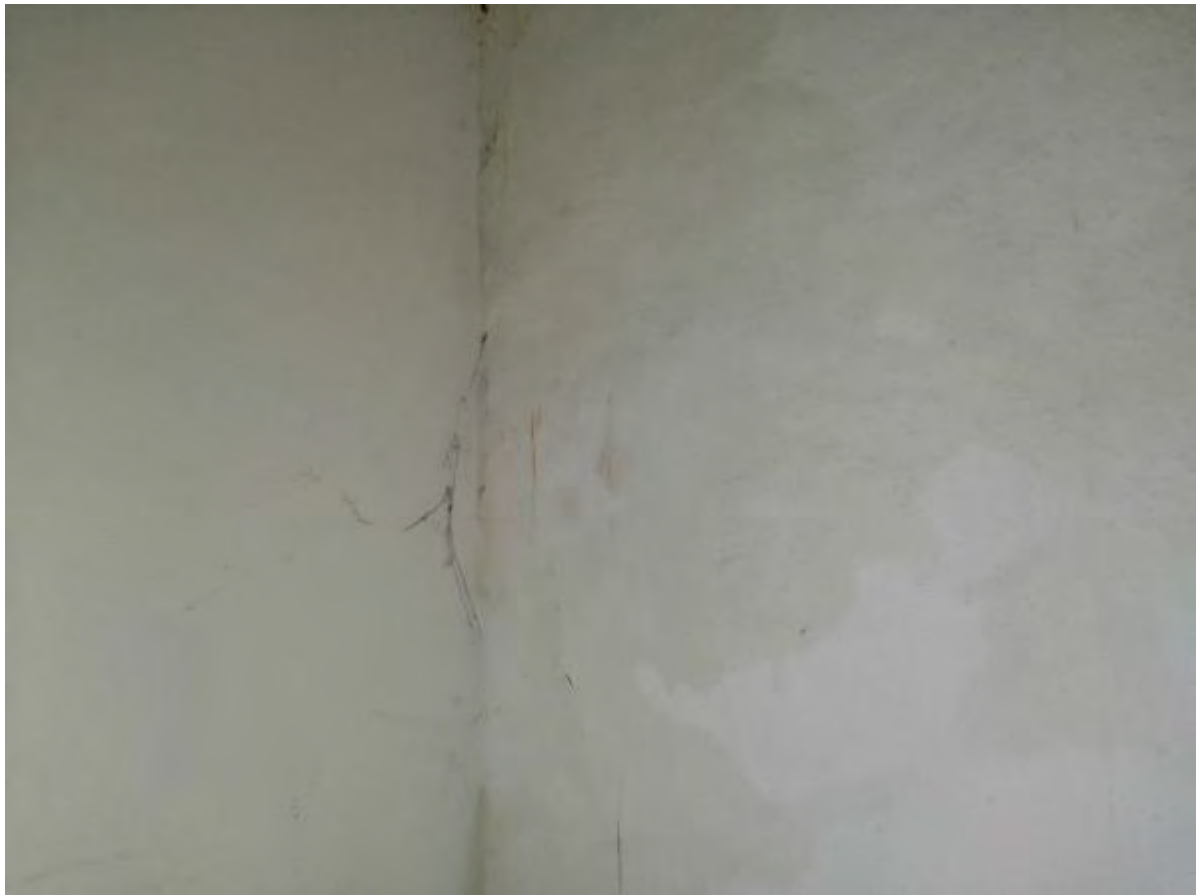
Photo 158 – Penetrating Damp (Front Room 1)
