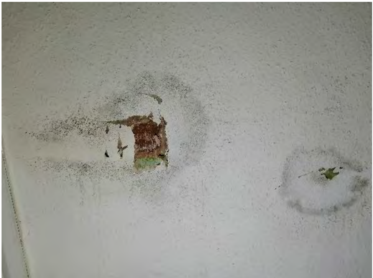
Photo 154 – Penetrating Damp (Front Room 1)
