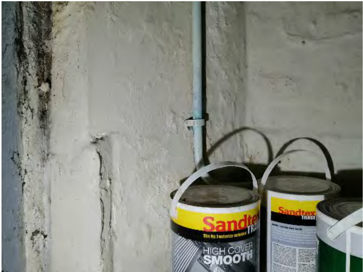
Photo 237 – Penetrating Damp (Utility Room 1)
