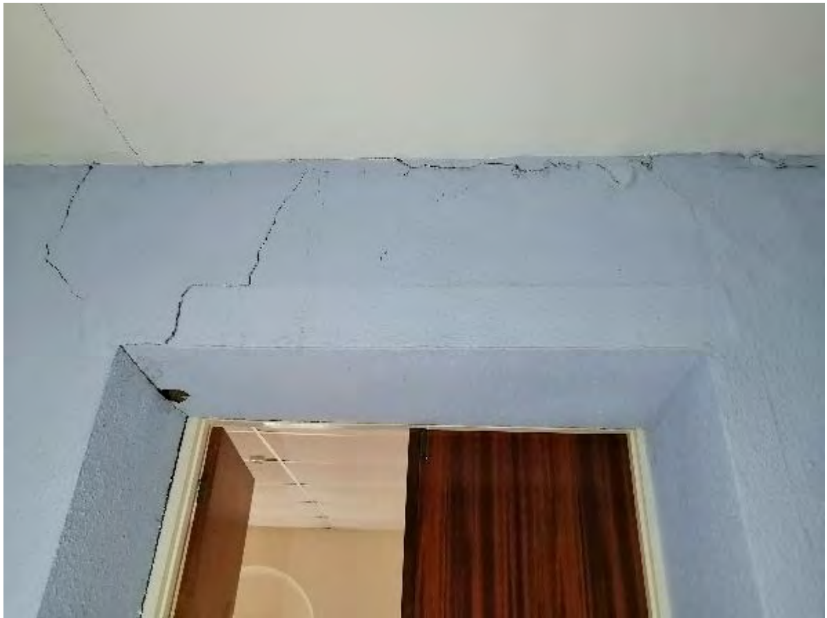
Photo 115 – Wall Plaster Crack (Rear Room)
