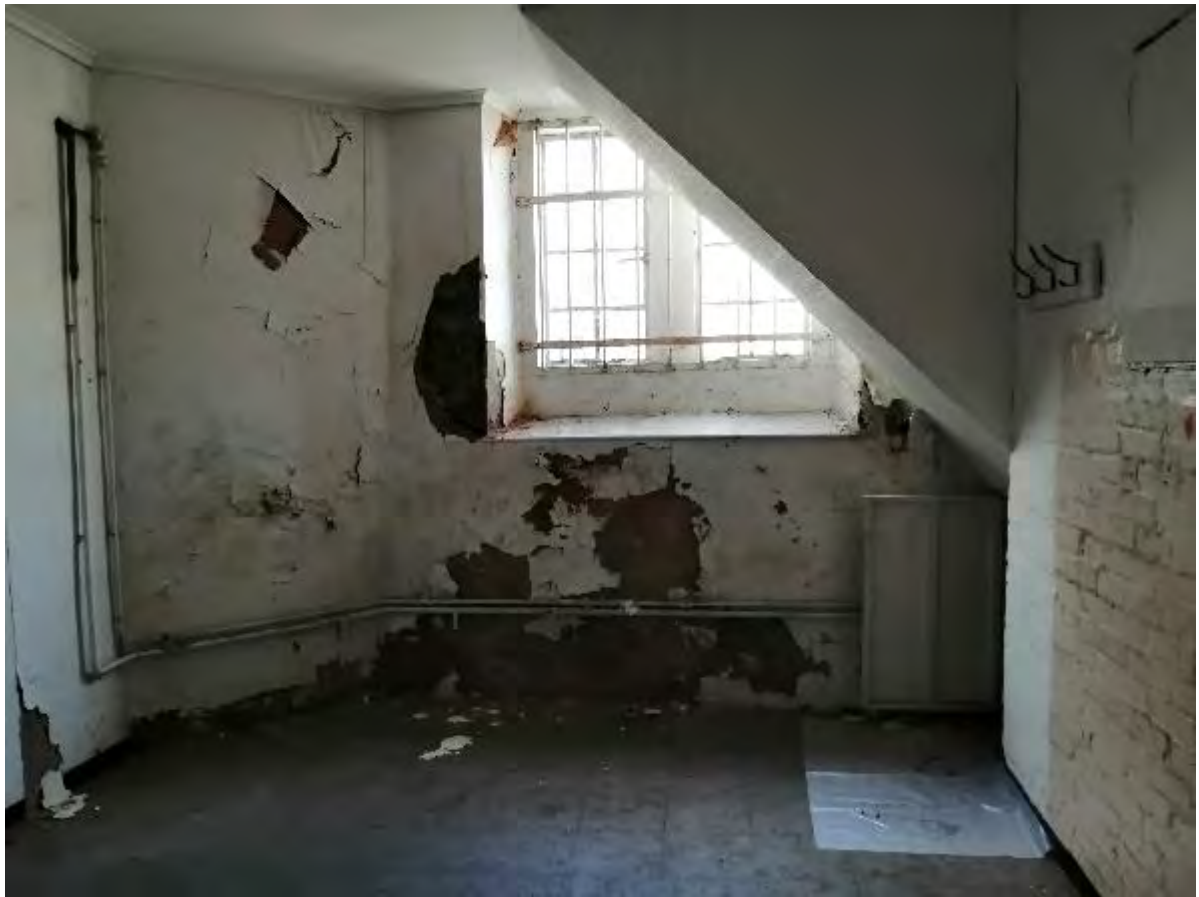
Photo 229 – Penetrating Damp (Side Room 1)
