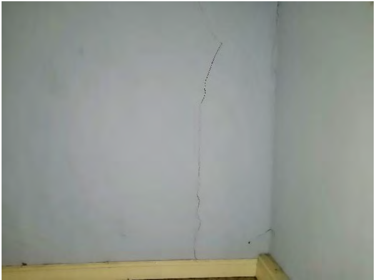
Photo 113 – Wall Plaster Crack (Rear Room)
