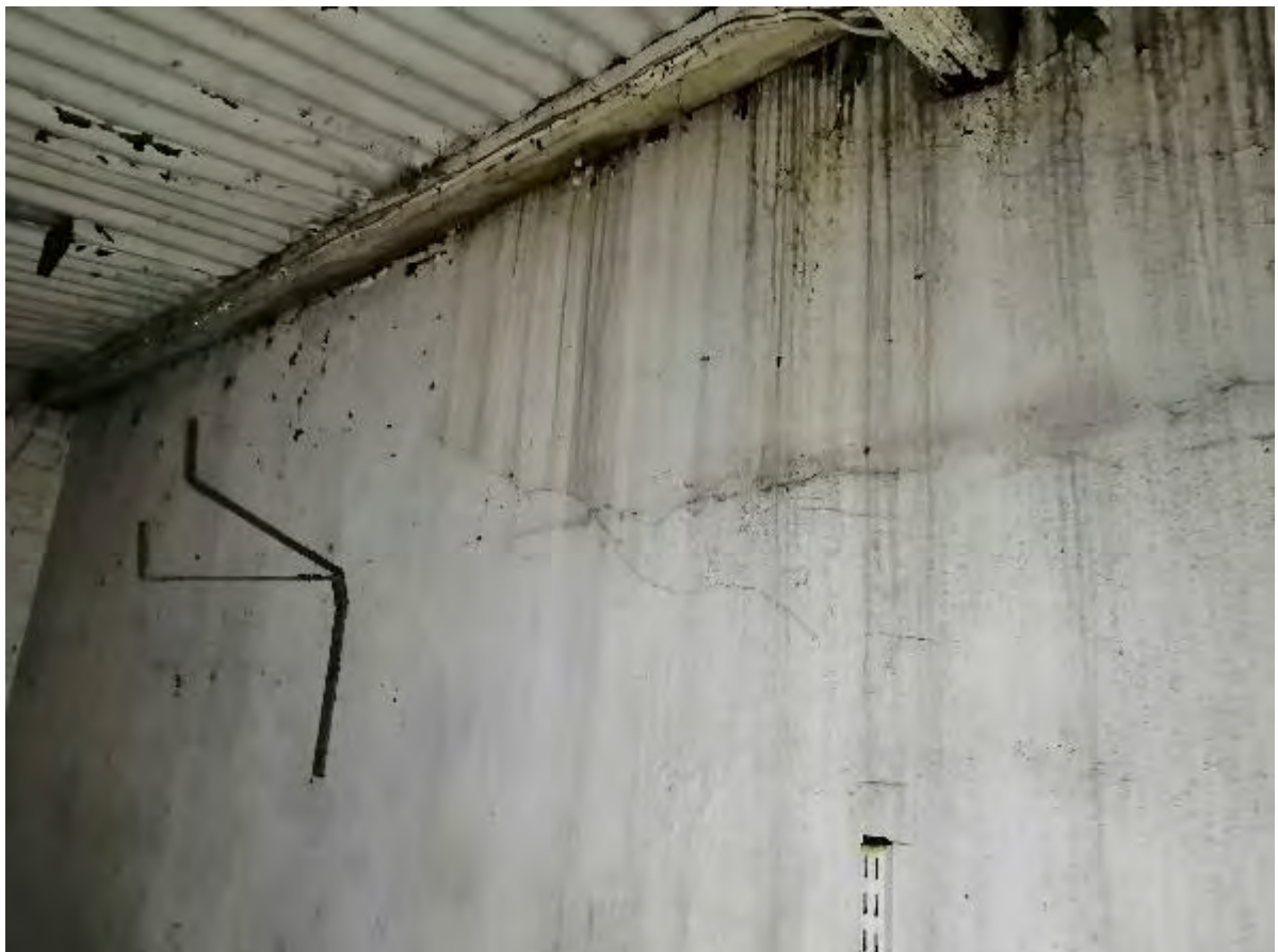
Photo 218 – Wall Plaster Crack (Fire Exit Room)
