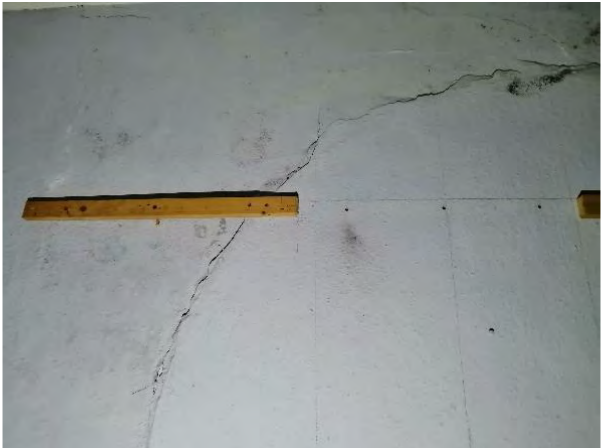
Photo 122 – Cracking Around Archway Infill (Rear Room)
