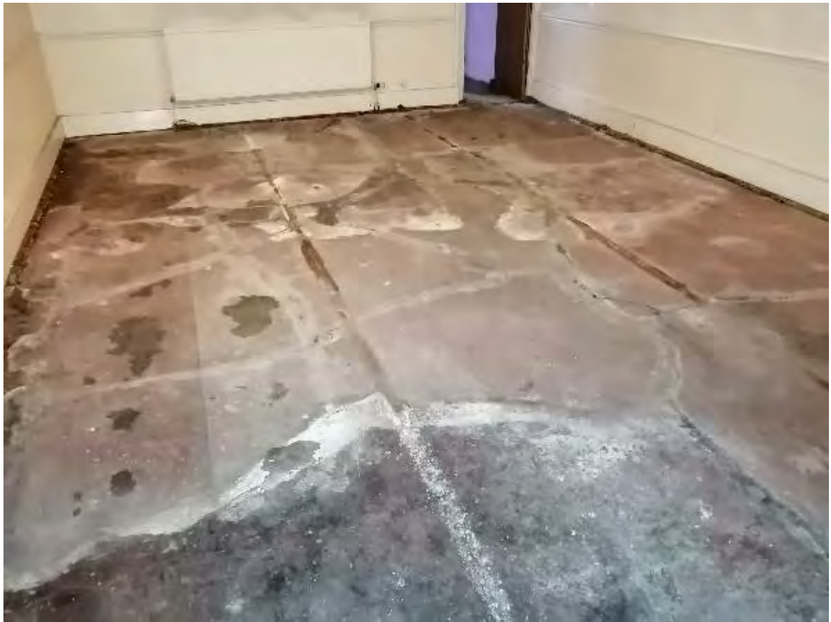
Photo 187 – Concrete Floor Cracking (Front Room)
