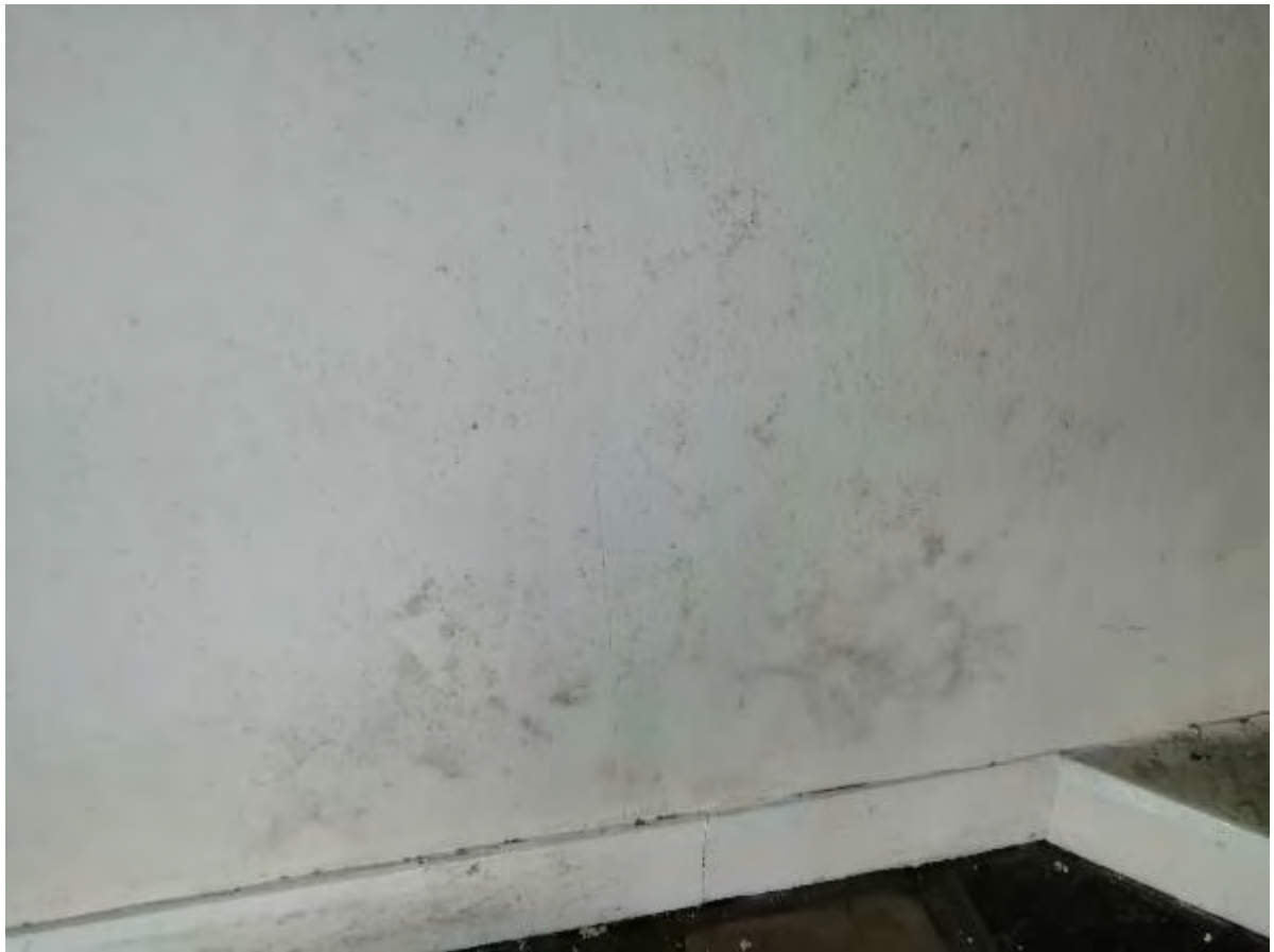
Photo 155 – Condensation Damp (Front Room 1)
