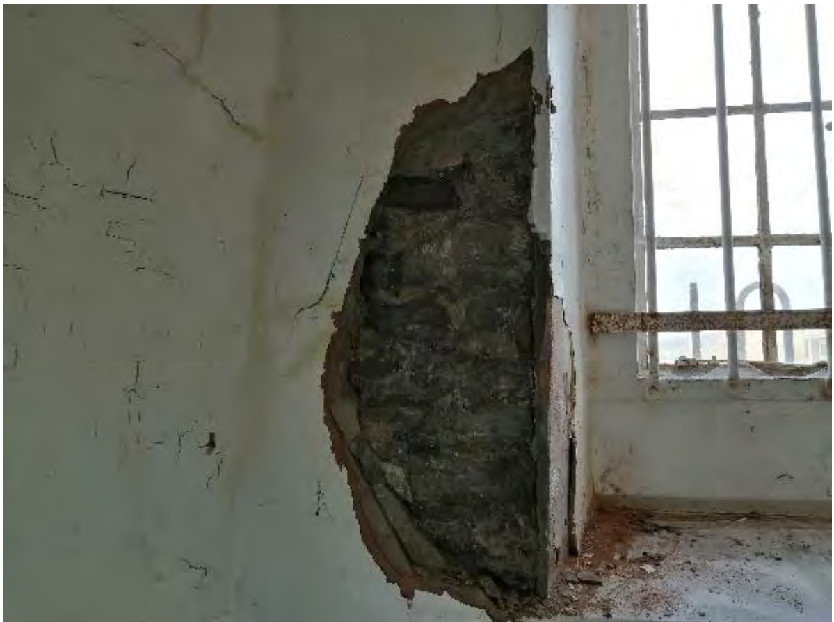
Photo 198 –Detached Plaster (Side Room 1)
