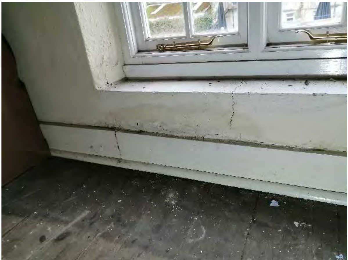
Photo 162 – Penetrating Damp (Front Room 1)
