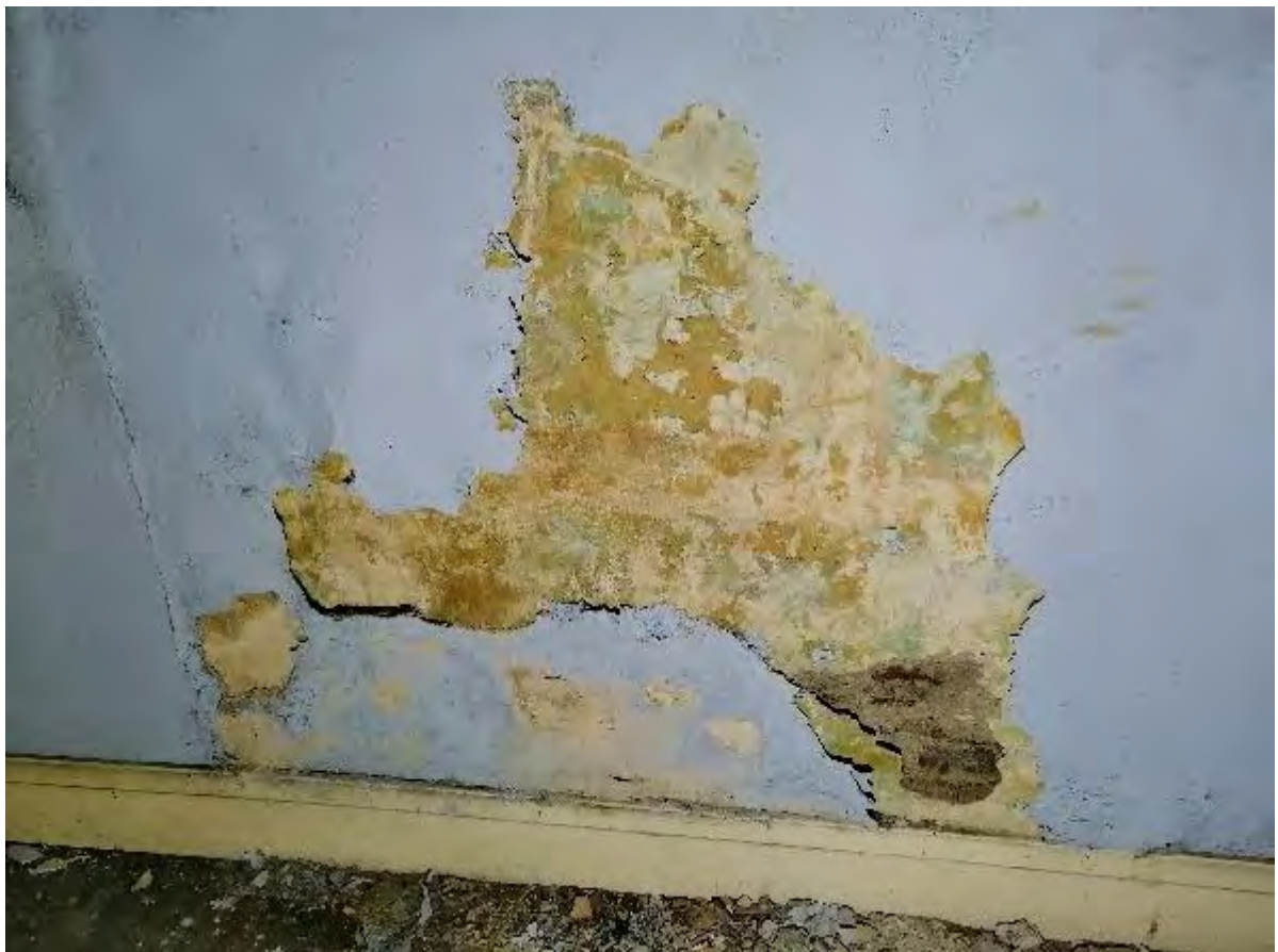
Photo 152 – Penetrating Damp (Rear Room)
