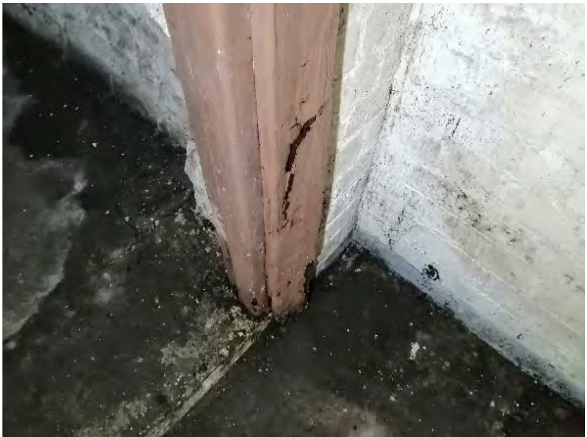
Photo 208 – Rot to Doorway Timber (Storage Room)
