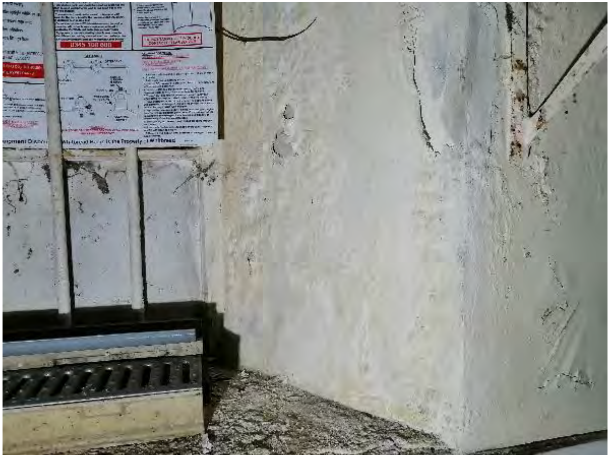
Photo 233 – Penetrating Damp (Utility Room 1)
