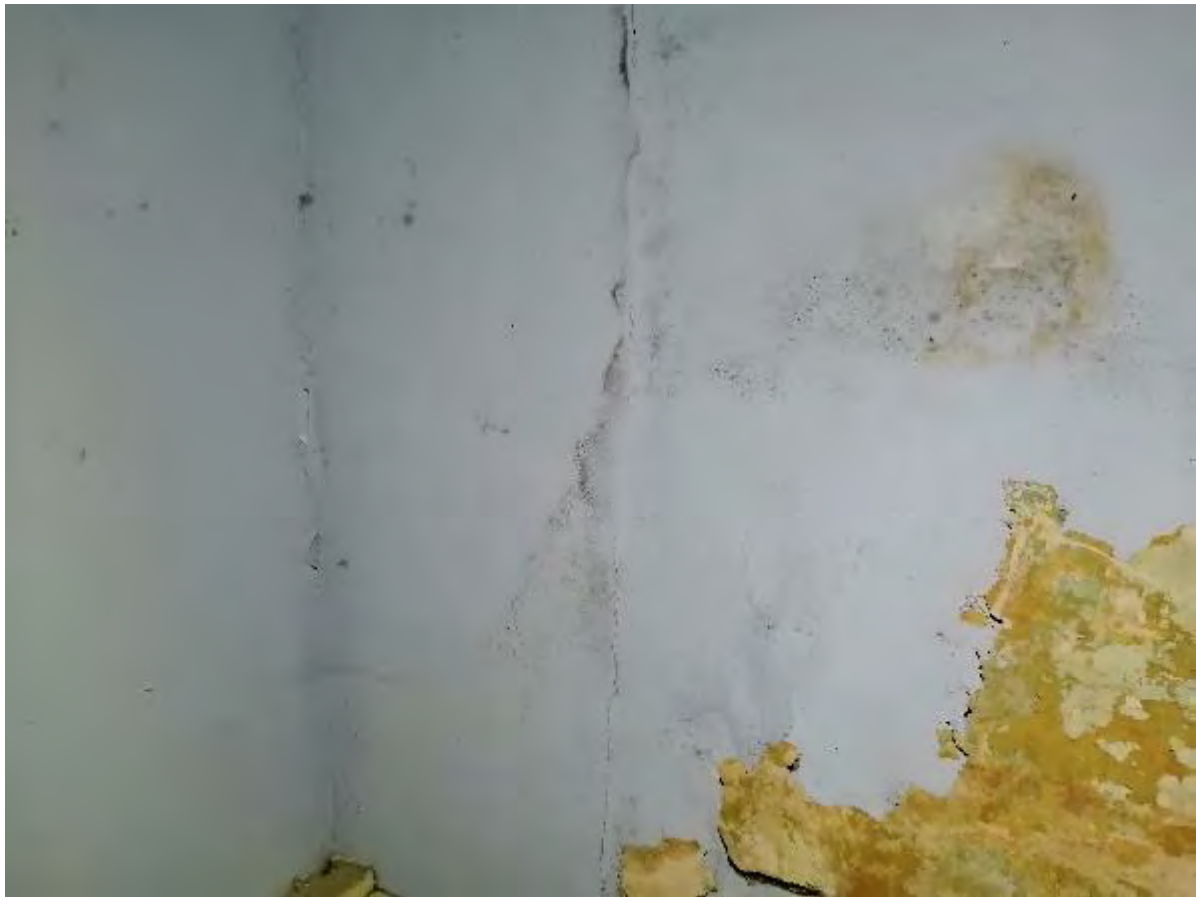
Photo 153 – Condensation Damp (Rear Room)
