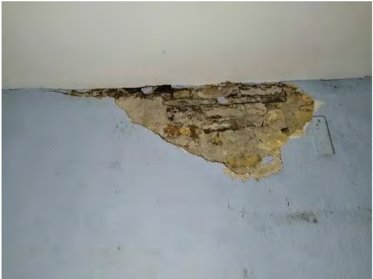
Photo 123 – Detached Wall Plaster (Rear Room)
