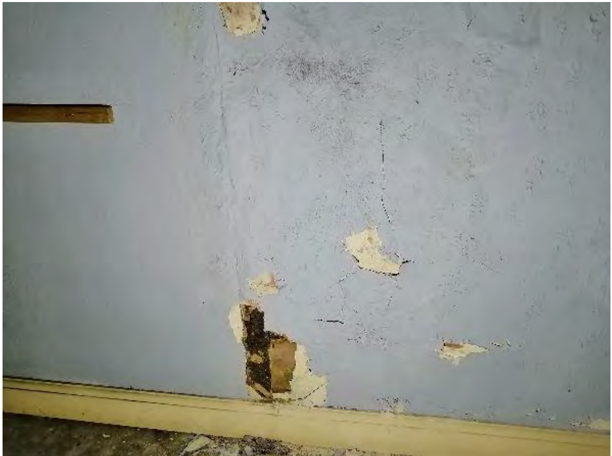
Photo 148 – Penetrating Damp (Rear Room)
