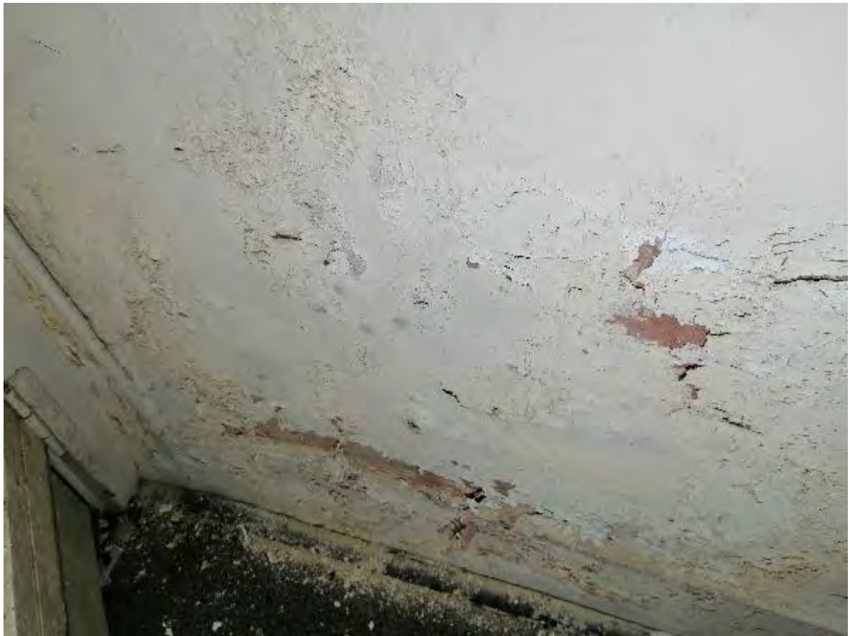
Photo 167 – Penetrating Damp (Male Toilets)
