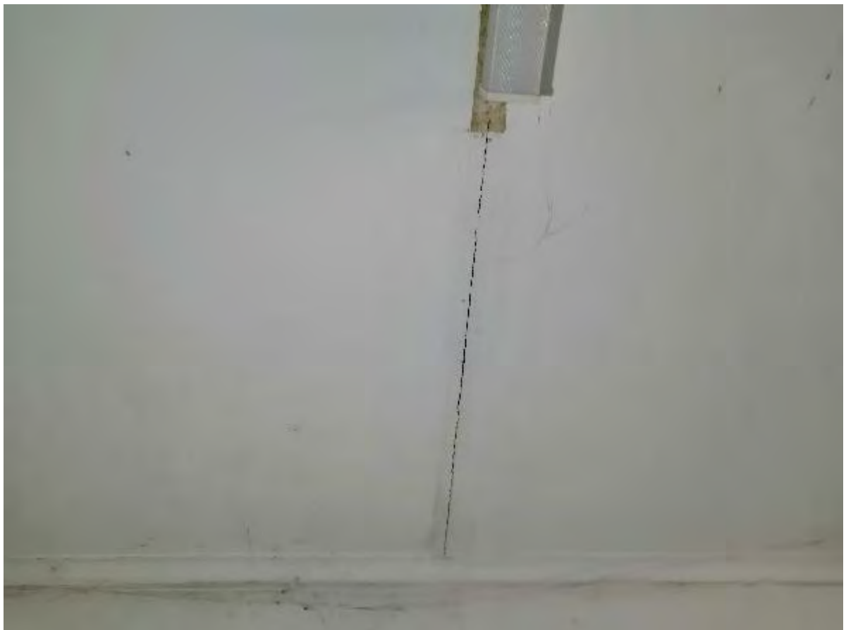
Photo 192 – Ceiling Cracking (Side Room 1)
