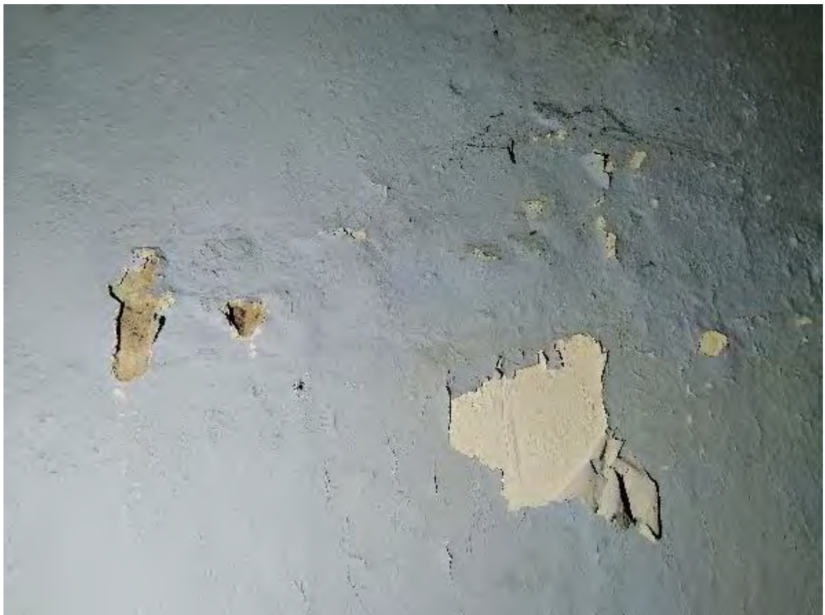
Photo 144 – Penetrating Damp (Rear Room)
