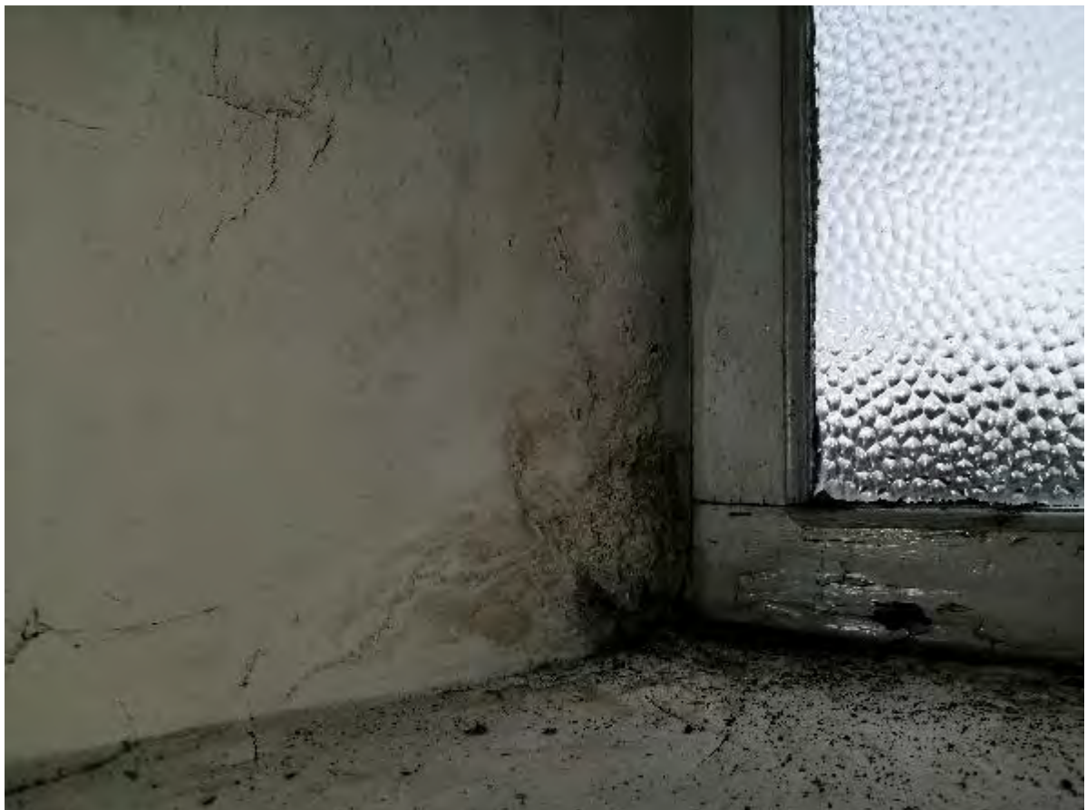
Photo 168 – Penetrating Damp (Male Toilets)
