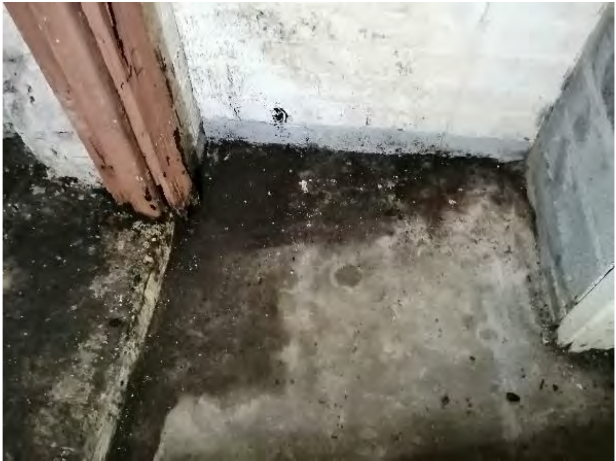
Photo 243 – Penetrating Damp (Corridor 3)
