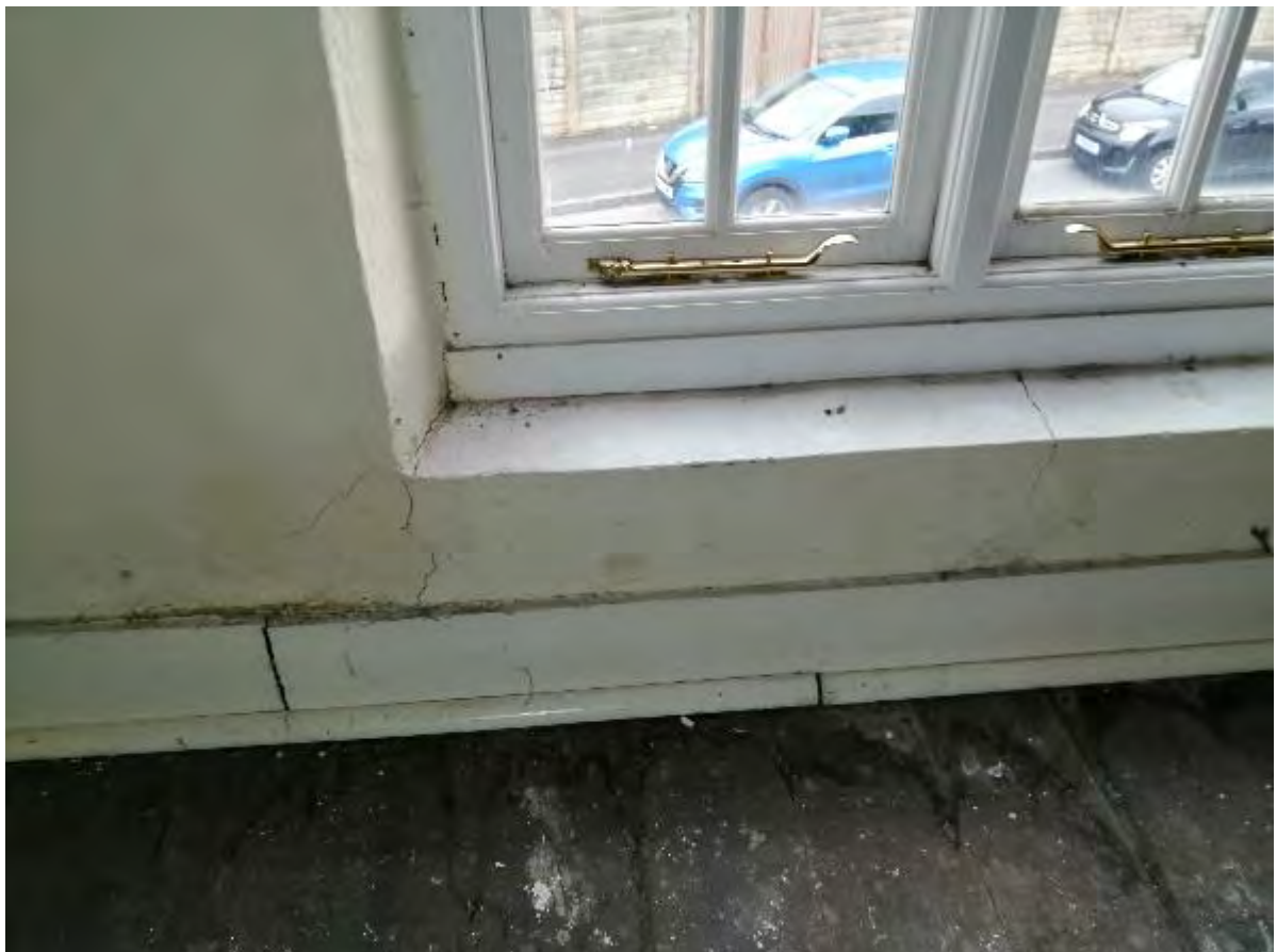
Photo 128 – Wall Plaster Crack (Front Room 1)
