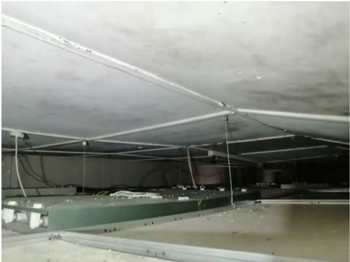
Photo 97 – Void Above Front Room 1
