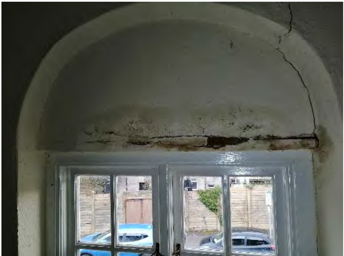
Photo 164 – Penetrating Damp (Front Room 1)
