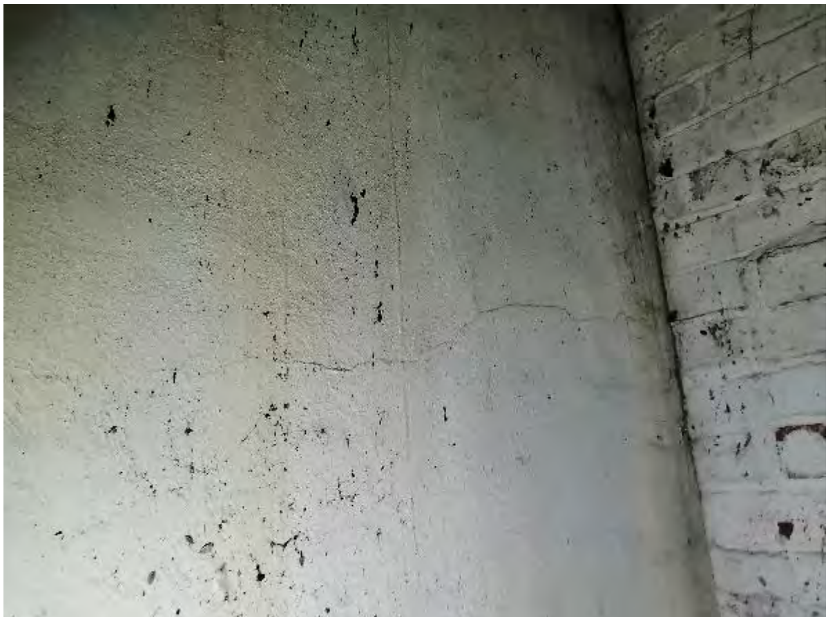
Photo 214 – Wall Plaster Crack (Fire Exit Room)
