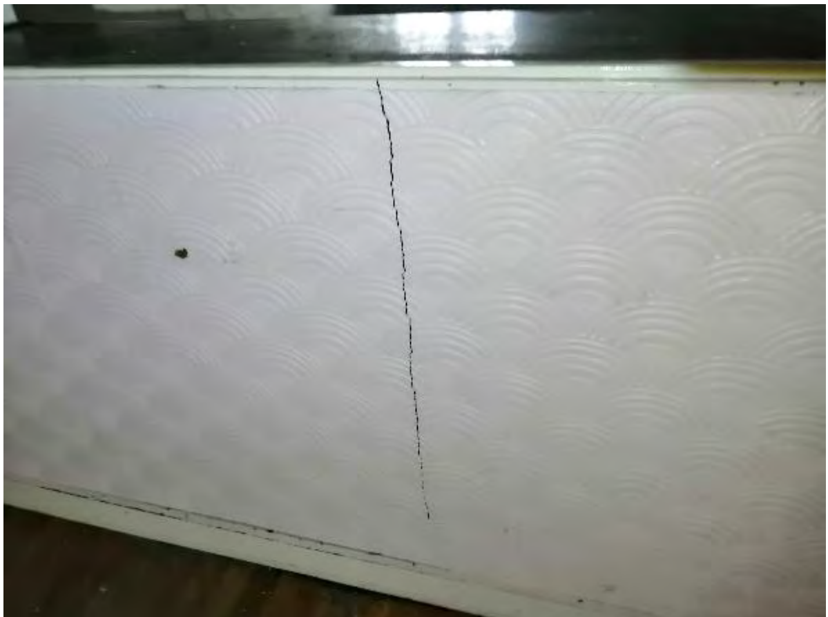
Photo 206 – Cracking to Studwork Wall (Hall)
