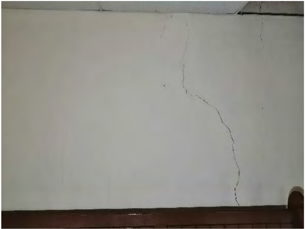
Photo 125 – Cracking Around and Above Archway Infill (Front Room 1)
