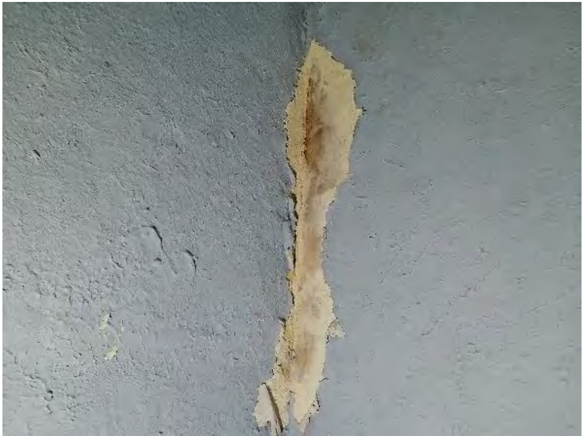
Photo 147 – Penetrating Damp (Rear Room)
