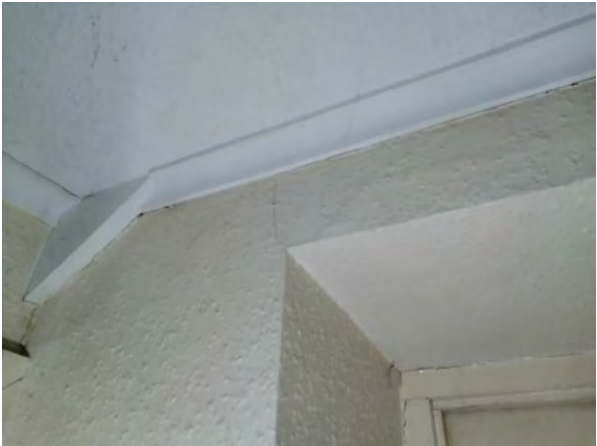
Photo 185 – Wall Plaster Crack (Corridor 1)
