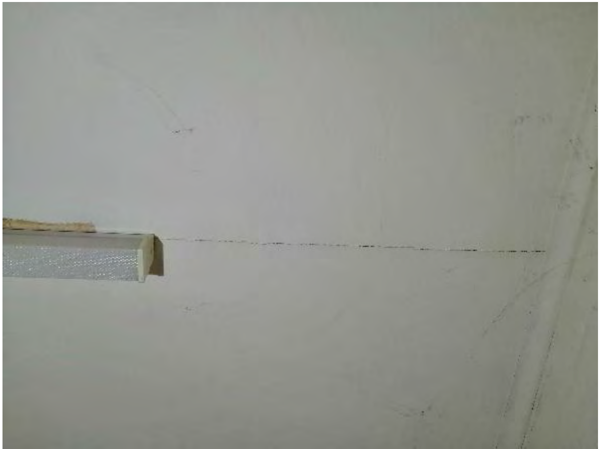
Photo 191 – Ceiling Cracking (Side Room 1)
