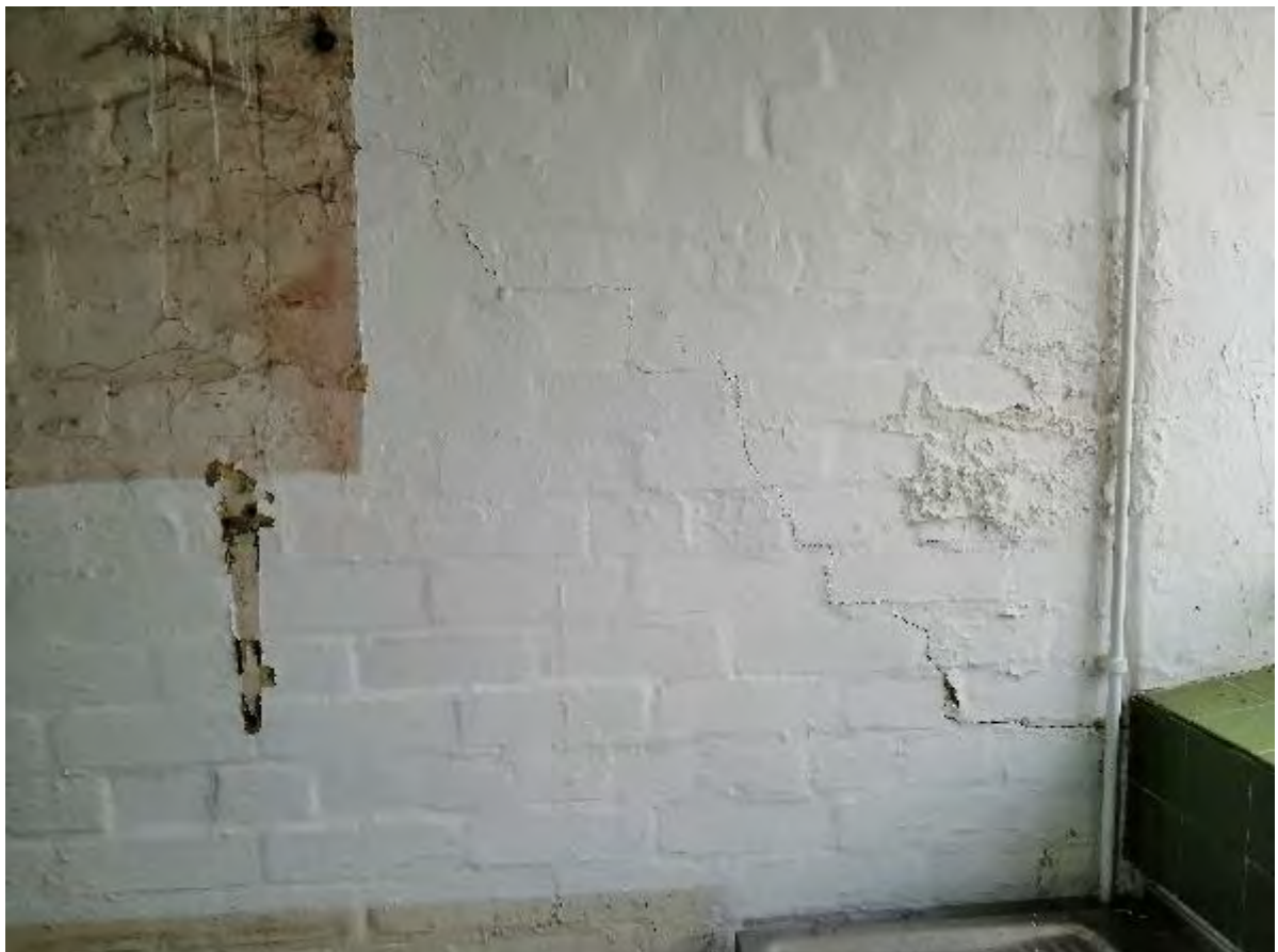
Photo 200 – Stepped Internal Wall Crack (Kitchen)
