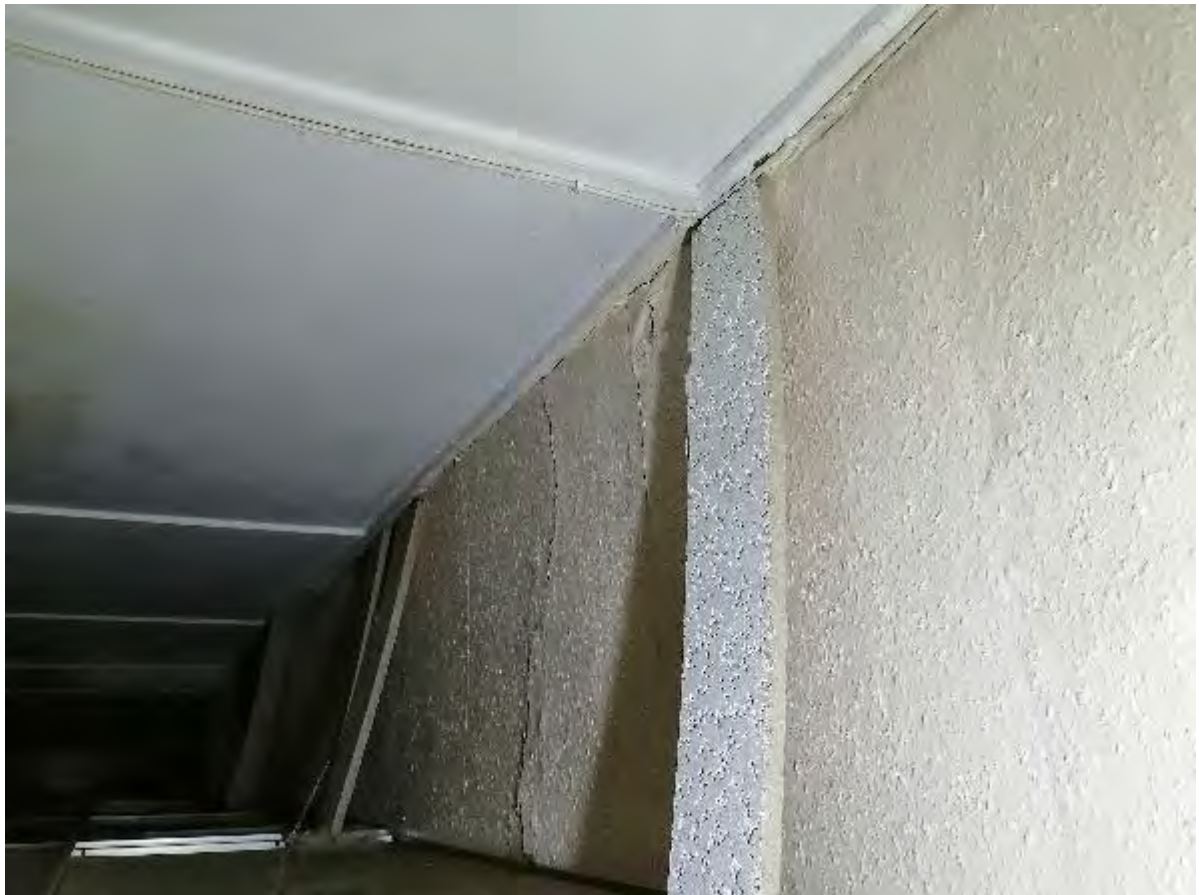
Photo 132 – Wall Plaster Crack (Front Room 1)
