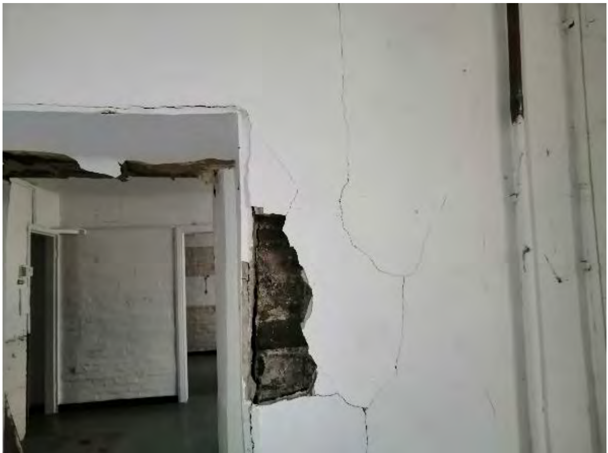
Photo 196 – Wall Plaster Cracking and Detached Plaster (Side Room 1)
