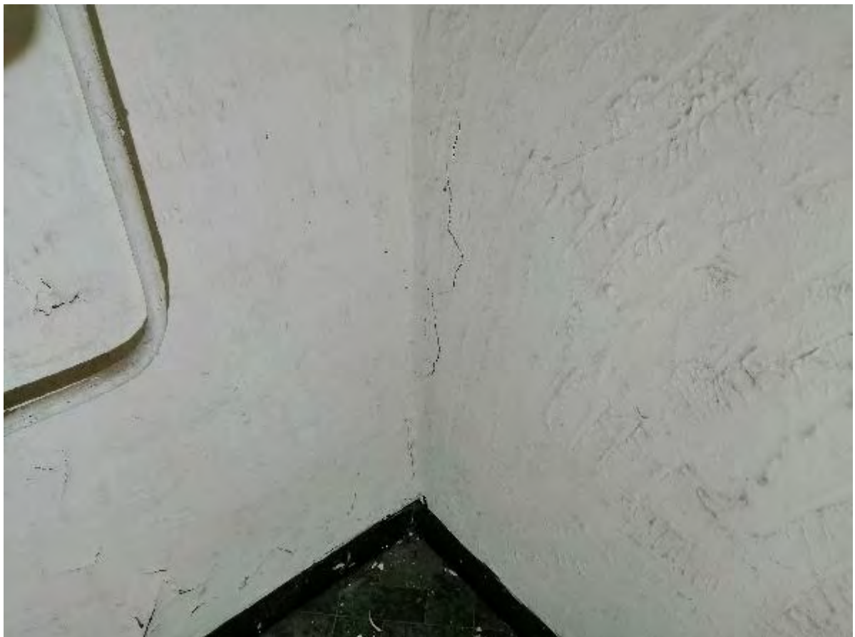
Photo 138 – Wall Plaster Crack (Male Toilet)
