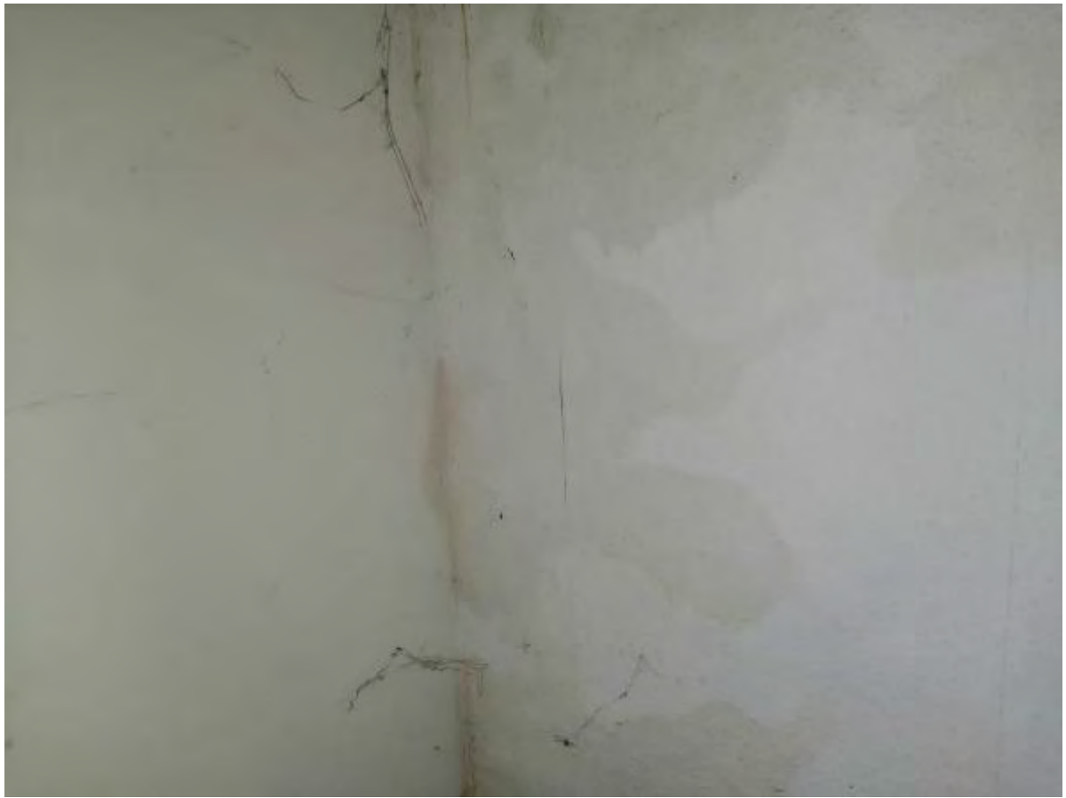
Photo 157 – Penetrating Damp (Front Room 1)
