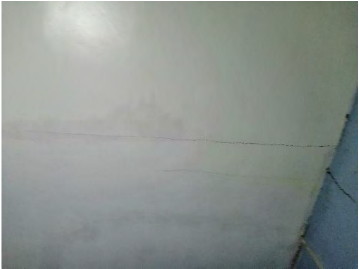
Photo 105 – Ceiling Cracking (Rear Room)
