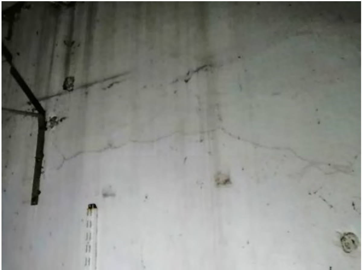
Photo 215 – Wall Plaster Crack (Fire Exit Room)
