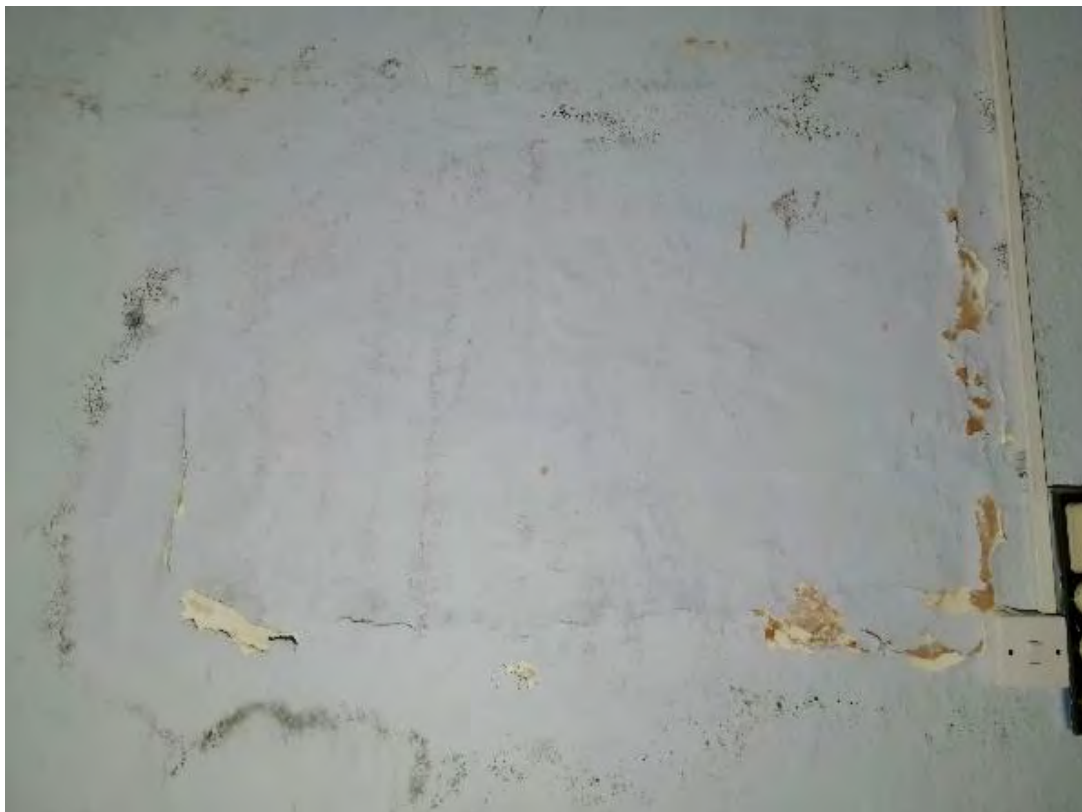
Photo 140 – Penetrating Damp (Rear Room)
