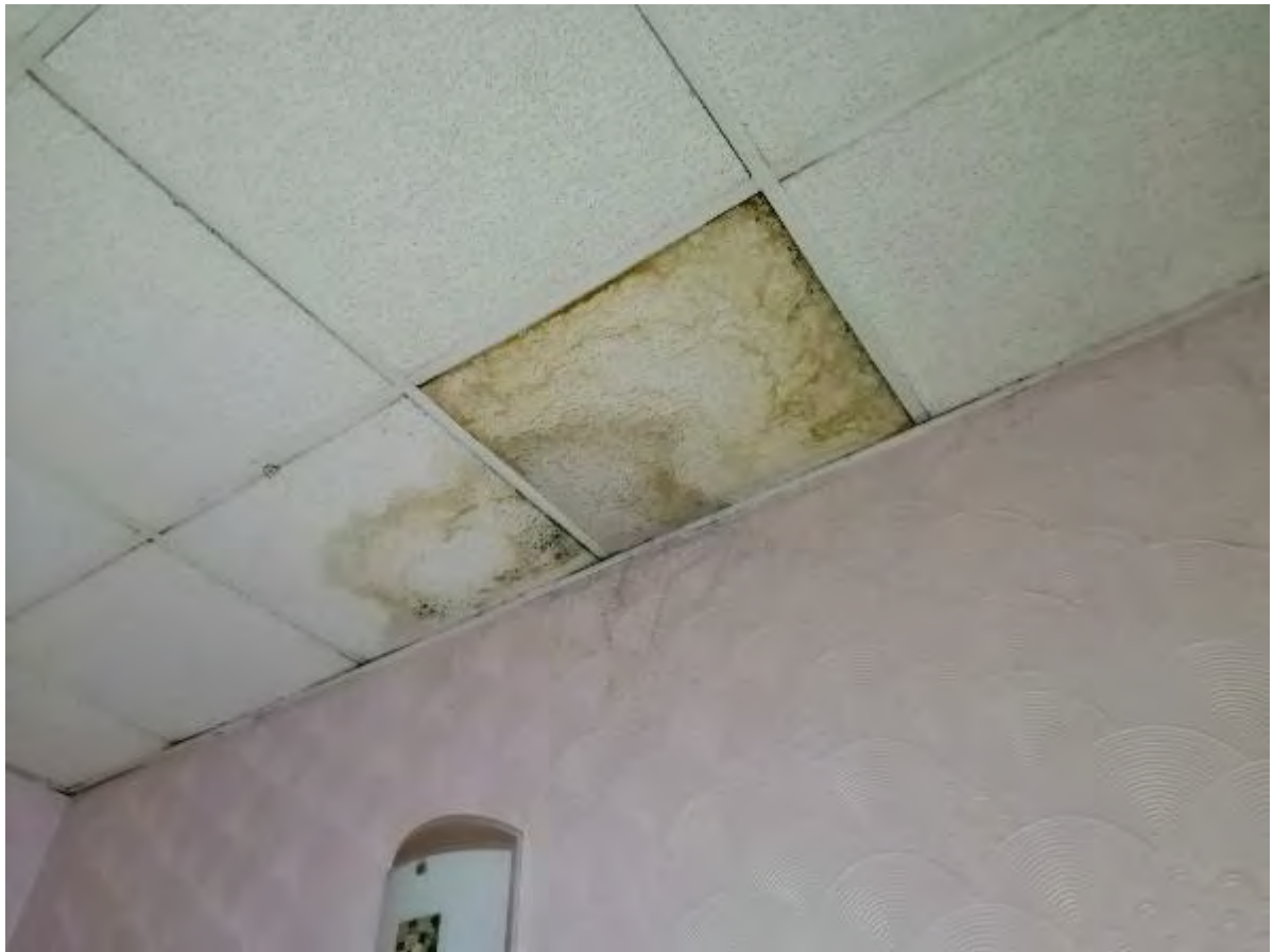
Photo 241 – Penetrating Damp (Hall)
