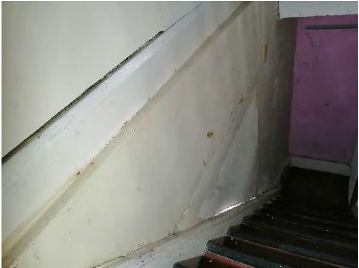
Photo 161 – Penetrating Damp (Front Room 1)
