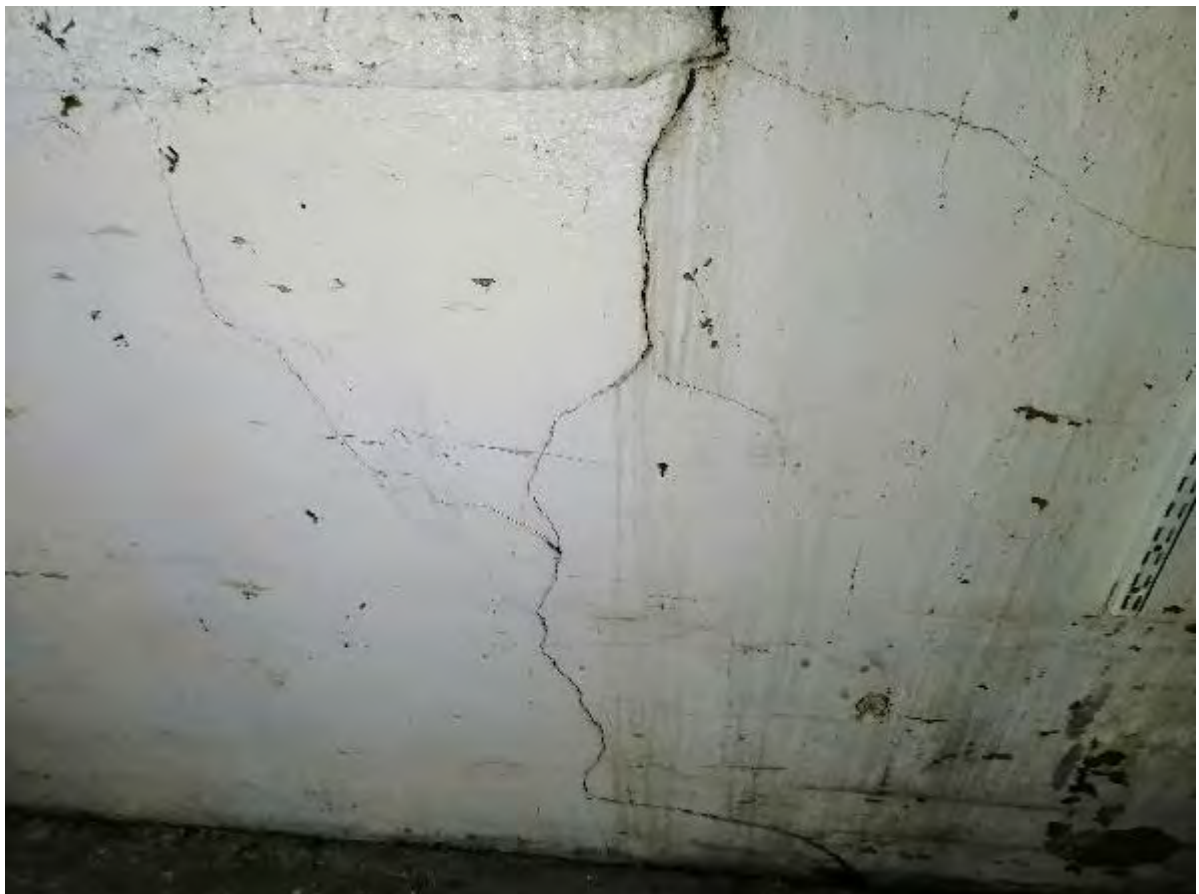
Photo 216 – Wall Plaster Crack (Fire Exit Room)
