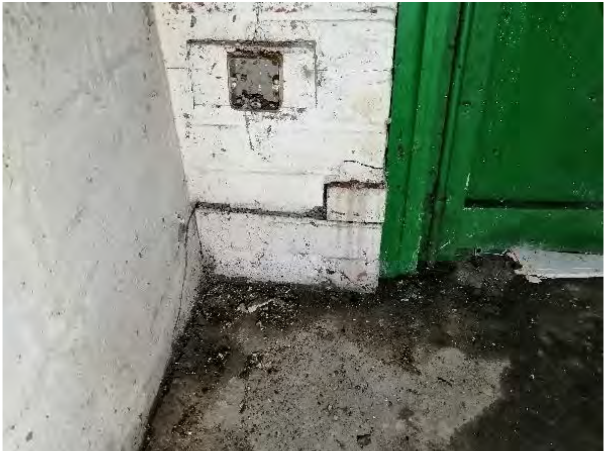
Photo 212 – Cracked and Displaced Masonry (Fire Exit Room)
