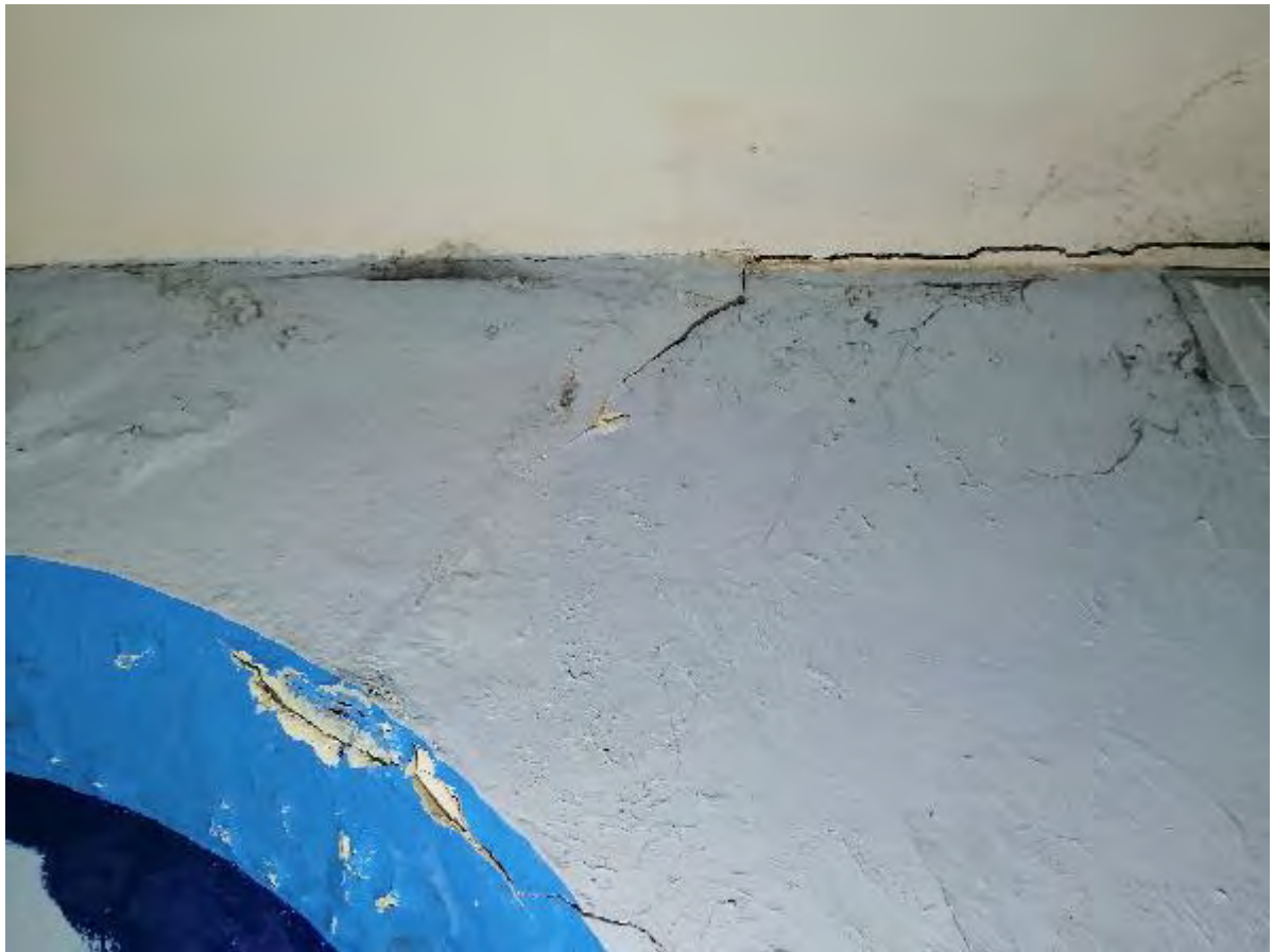
Photo 117 – Wall Plaster Crack (Rear Room)
