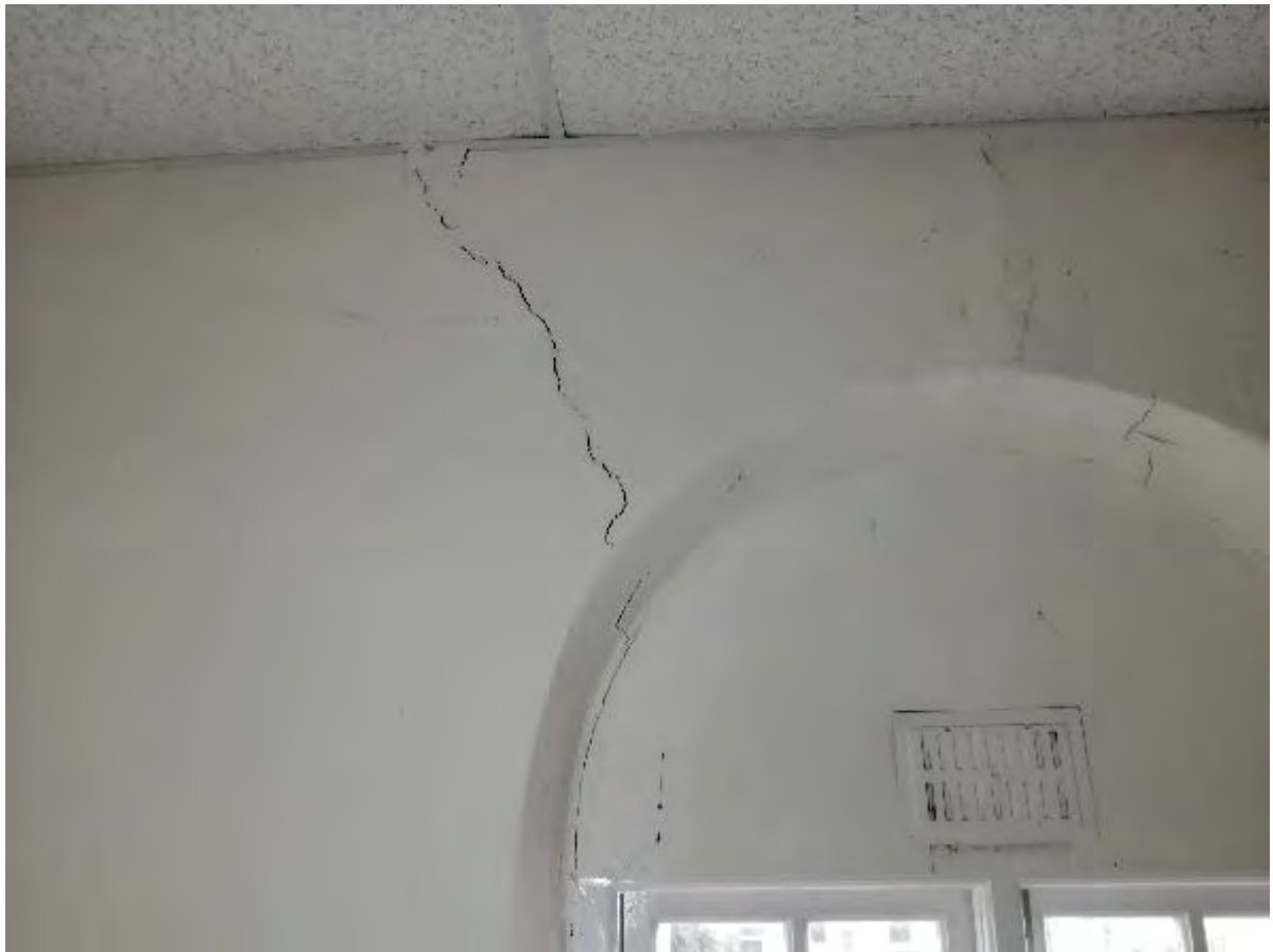
Photo 127 – Wall Crack Above Archway (Front Room 1)
