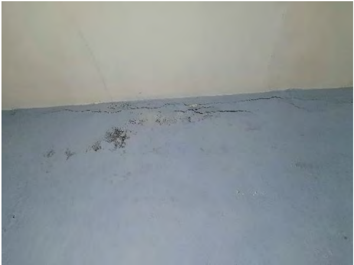
Photo 121 – Wall Plaster Crack (Rear Room)
