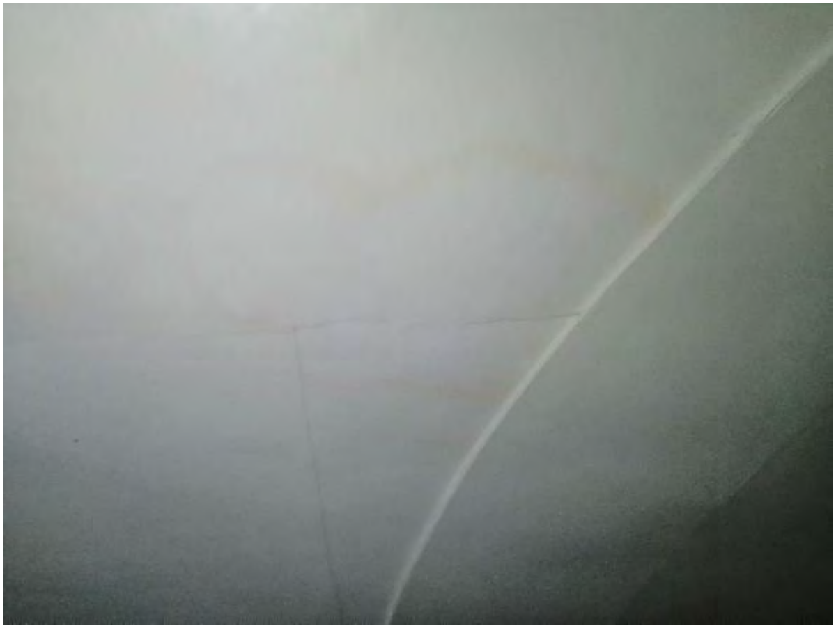
Photo 109 – Ceiling Cracking (Rear Room)
