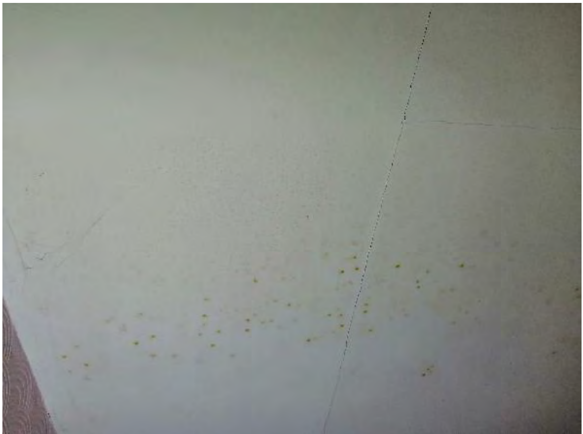
Photo 240 – Condensation Damp (Hall)
