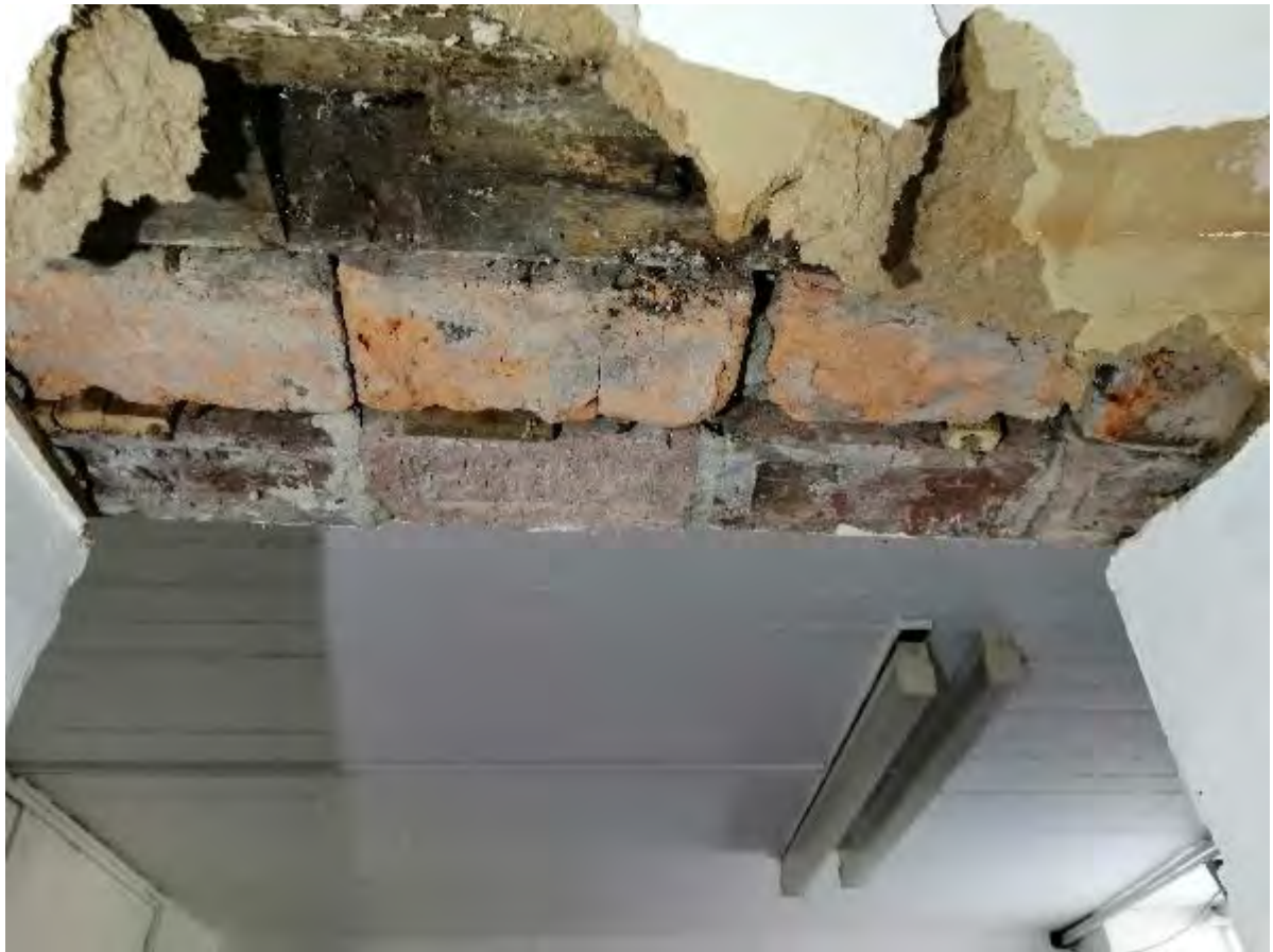
Photo 197 – No Doorway Lintel (Side Room 1)
