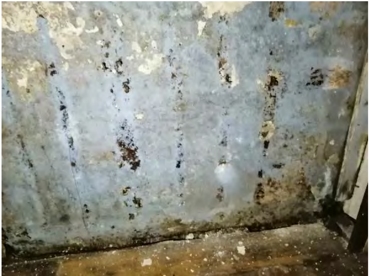
Photo 239 – Penetrating Damp (Hall)
