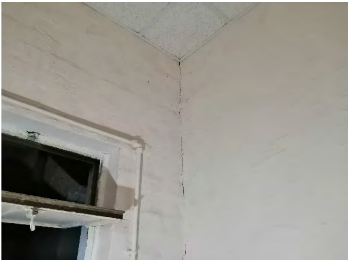
Photo 136 – Wall Plaster Crack (Male Toilet)
