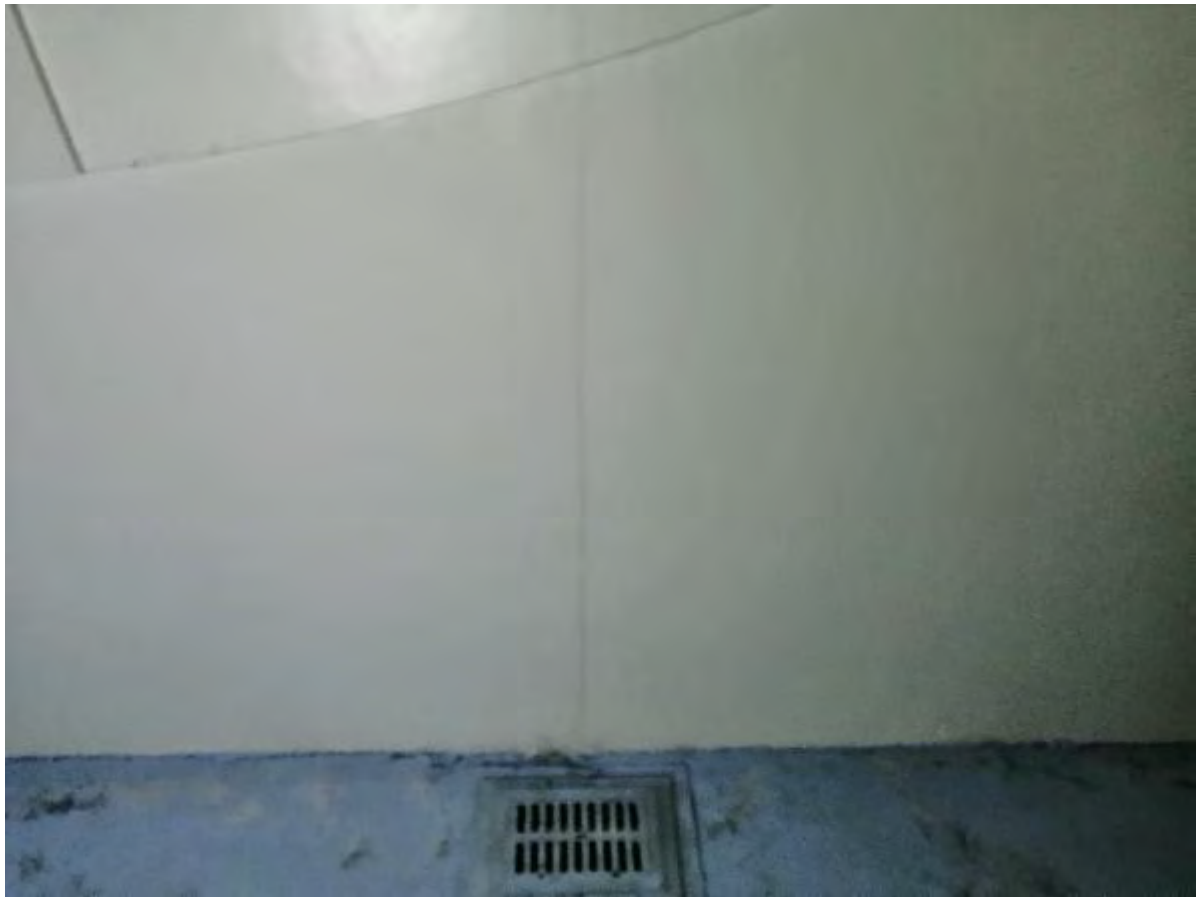
Photo 111 – Ceiling Cracking (Rear Room)
