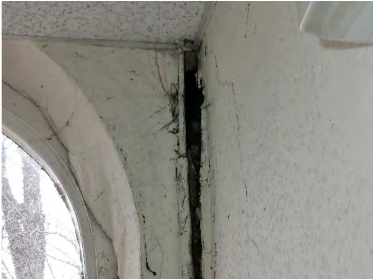
Photo 134 – Wall Plaster Crack (Staircase)
