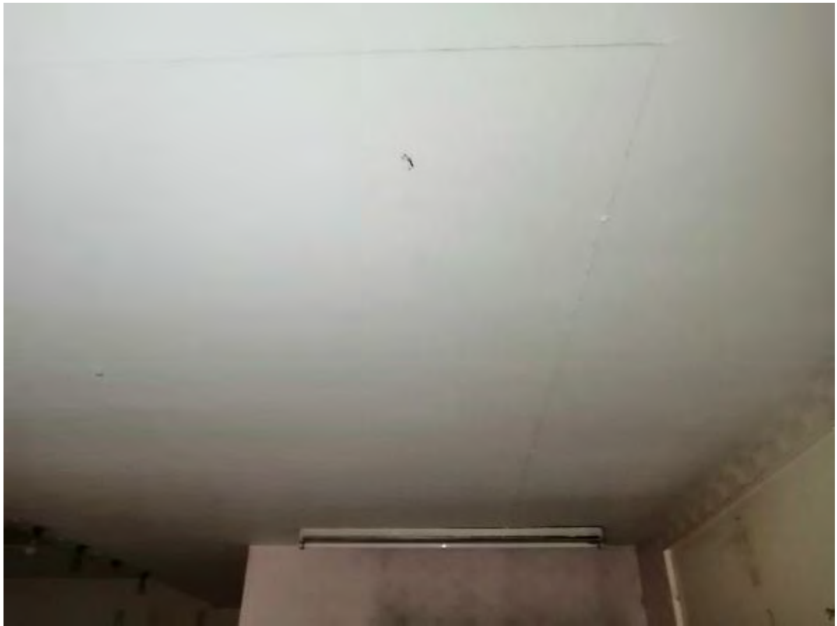
Photo 205 – Ceiling Cracking (Hall)
