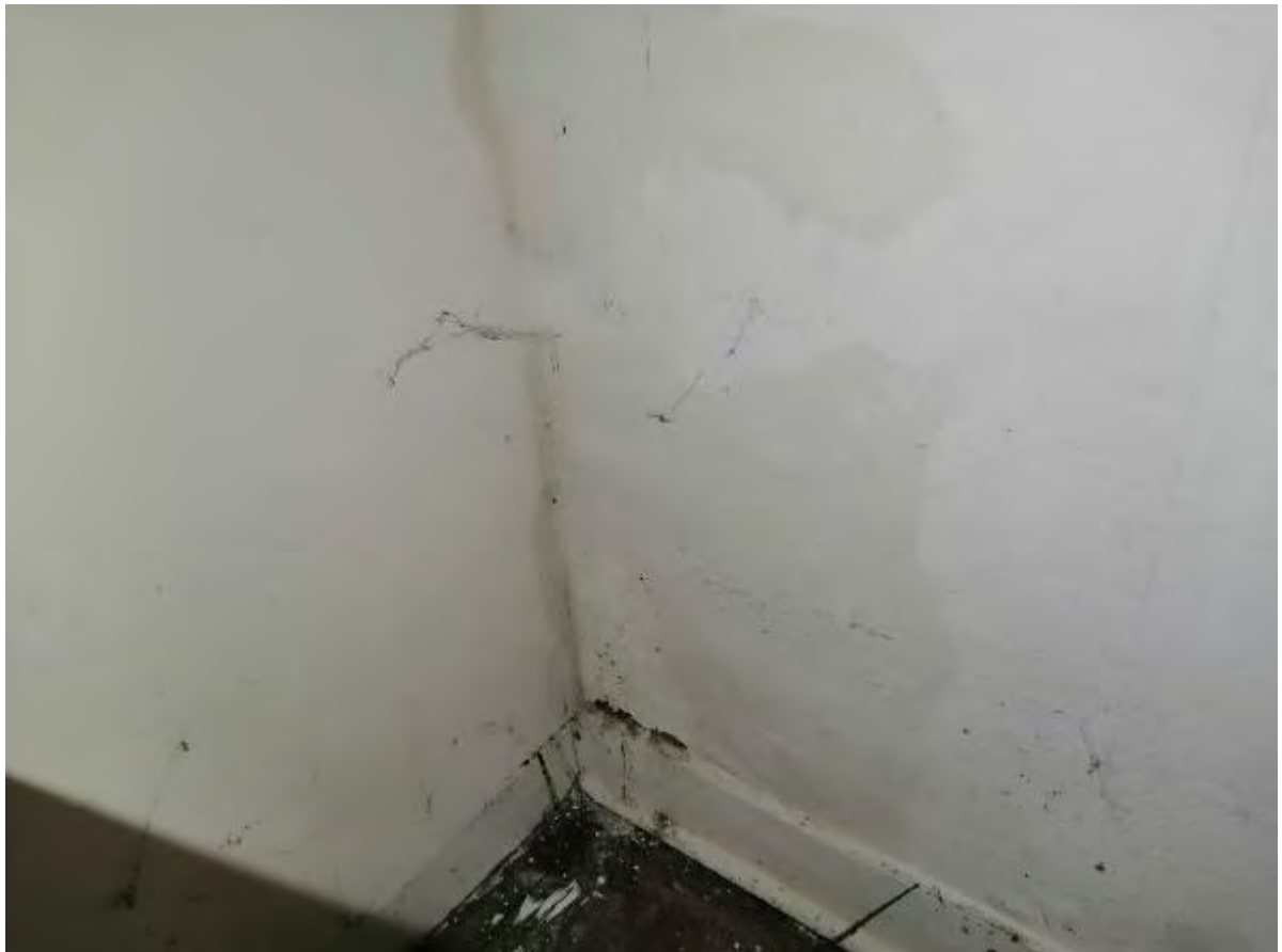
Photo 156 – Penetrating Damp (Front Room 1)
