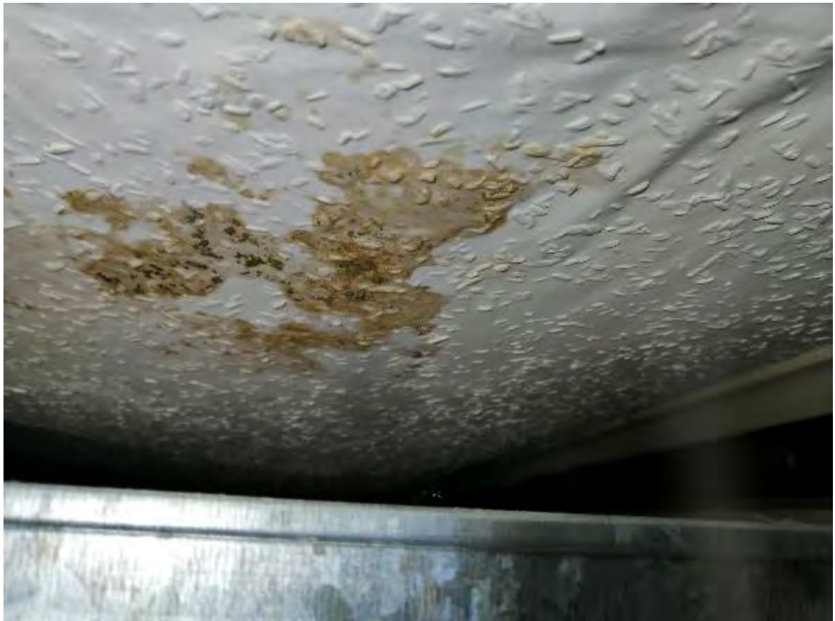
Photo 242 – Penetrating Damp (Hall)
