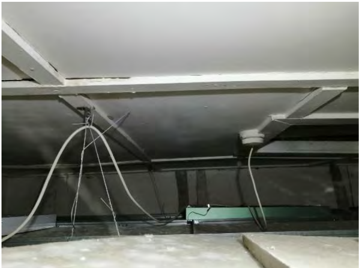
Photo 99 – Void Above Male Toilets
