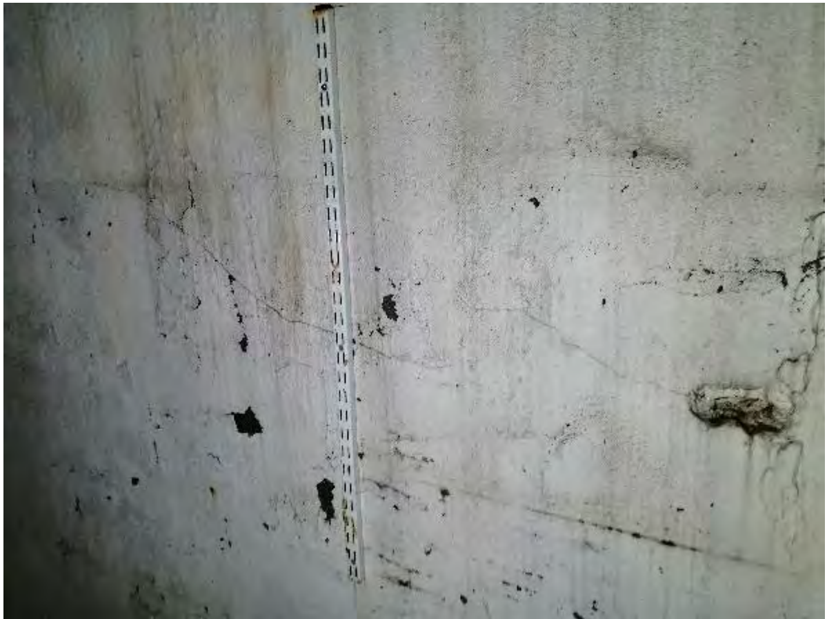
Photo 217 – Wall Plaster Crack (Fire Exit Room)
