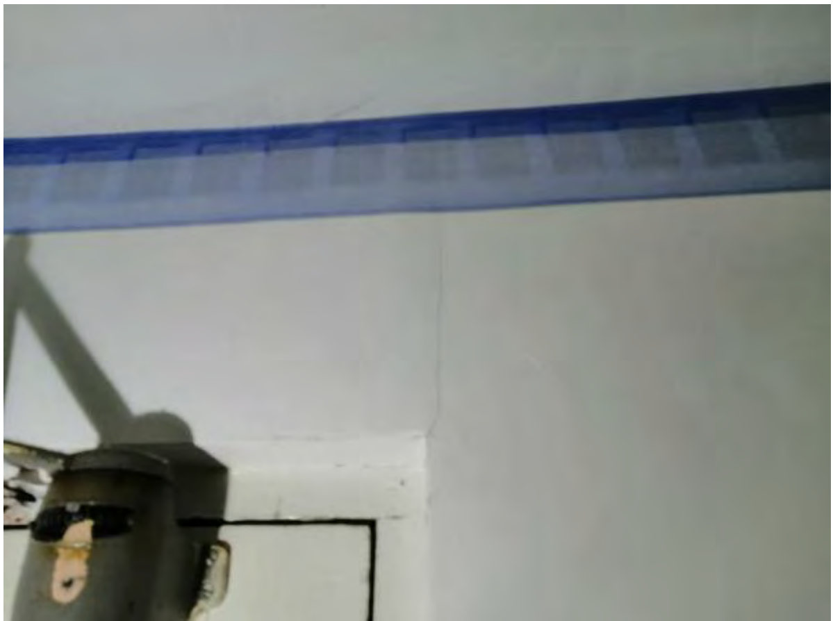
Photo 186 – Wall Plaster Crack (Female Toilets)
