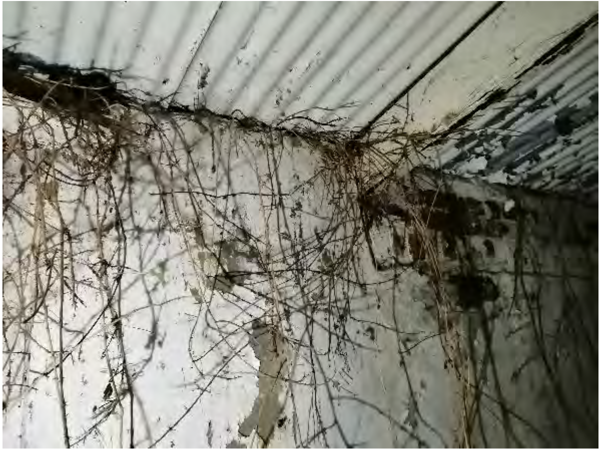
Photo 211 – Internal Vegetation Growth (Fire Exit Room)
