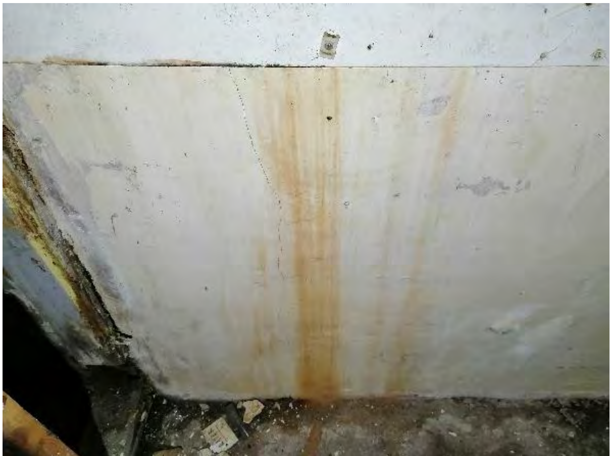
Photo 202 – Wall Plaster Crack (Utility Room 1)
