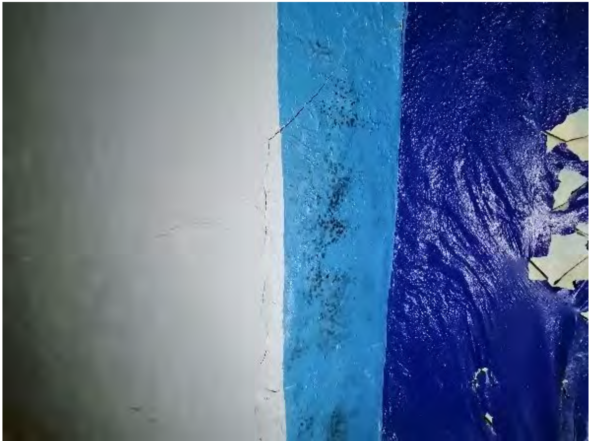
Photo 145 – Condensation Damp (Rear Room)
