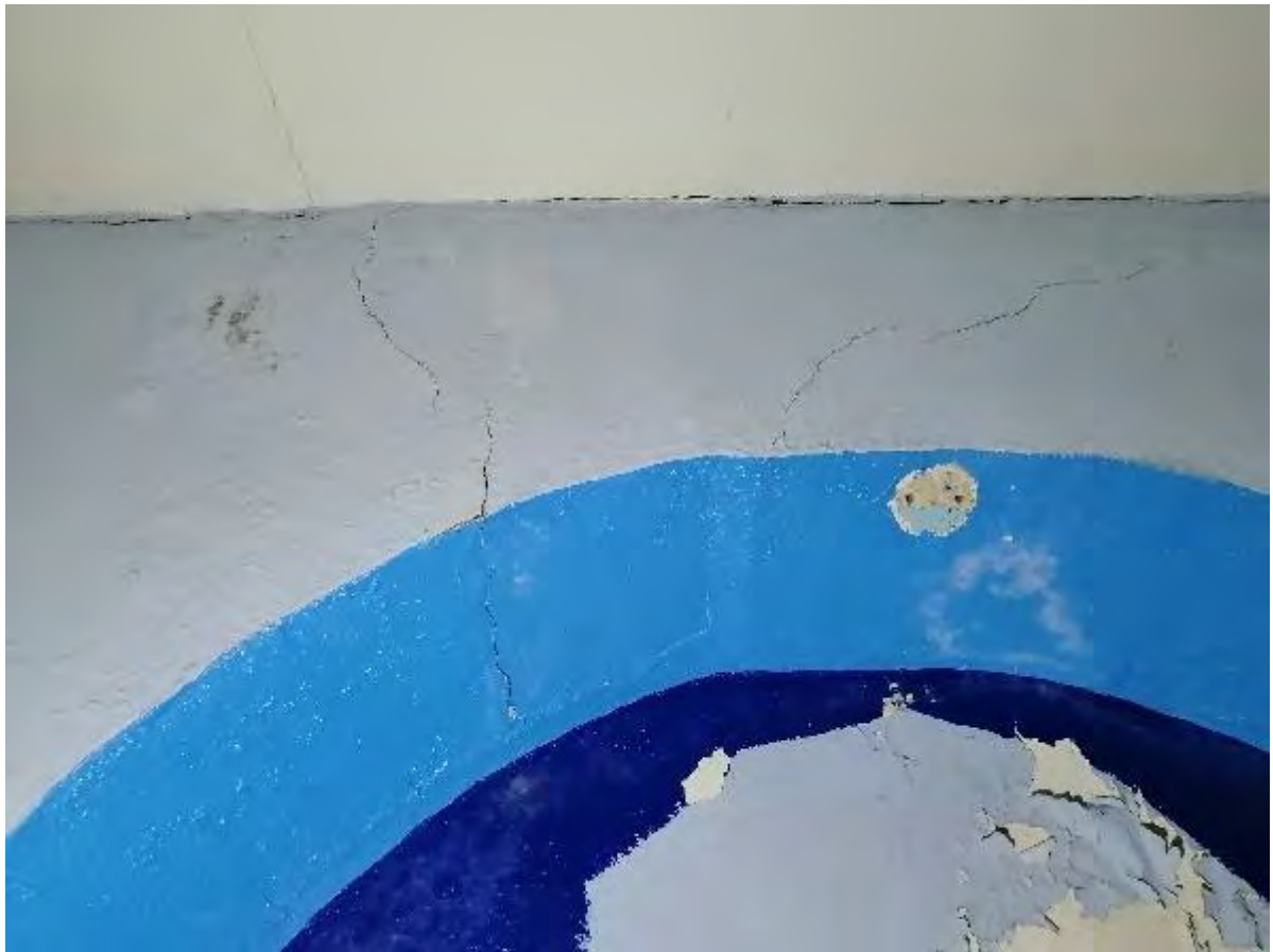
Photo 119 – Wall Plaster Crack (Rear Room)
