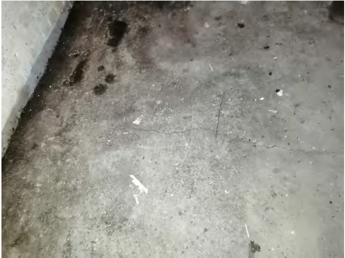
Photo 209 – Cracking to Concrete Floor (Storage Room)
