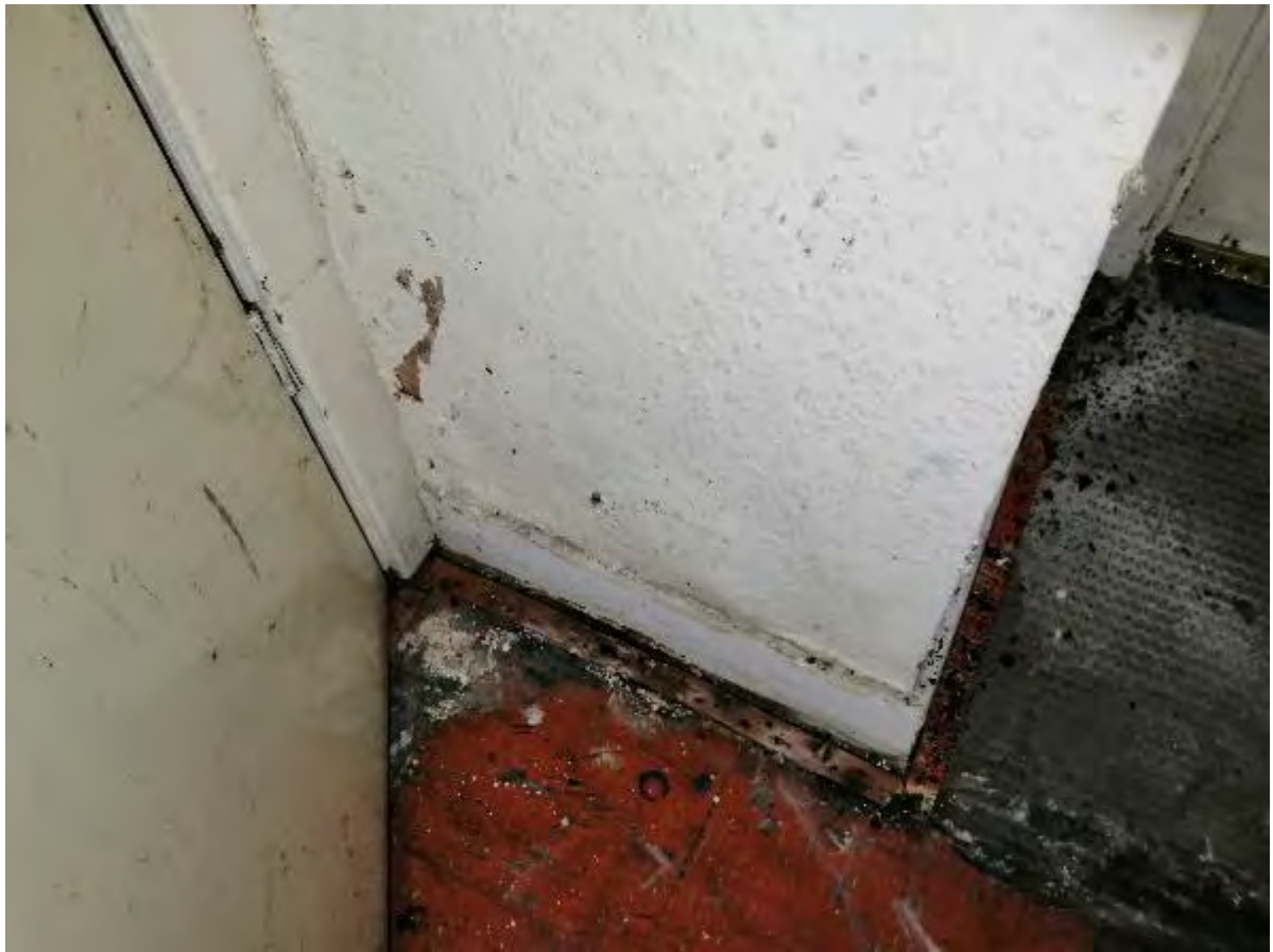
Photo 225 – Rising Damp (Corridor 1)
