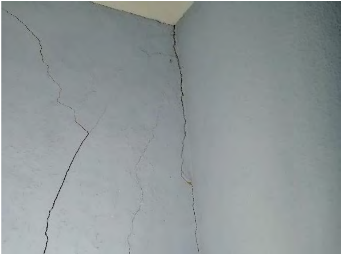
Photo 114 – Wall Plaster Crack (Rear Room)
