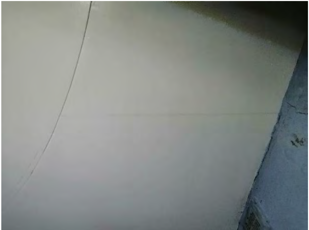
Photo 112 – Ceiling Cracking (Rear Room)
