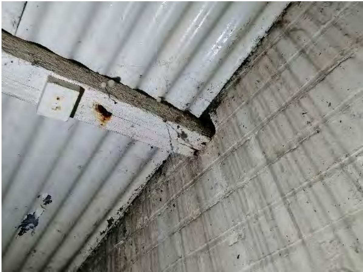
Photo 223 – Rot to Roof Purlin (Fire Exit Room)
