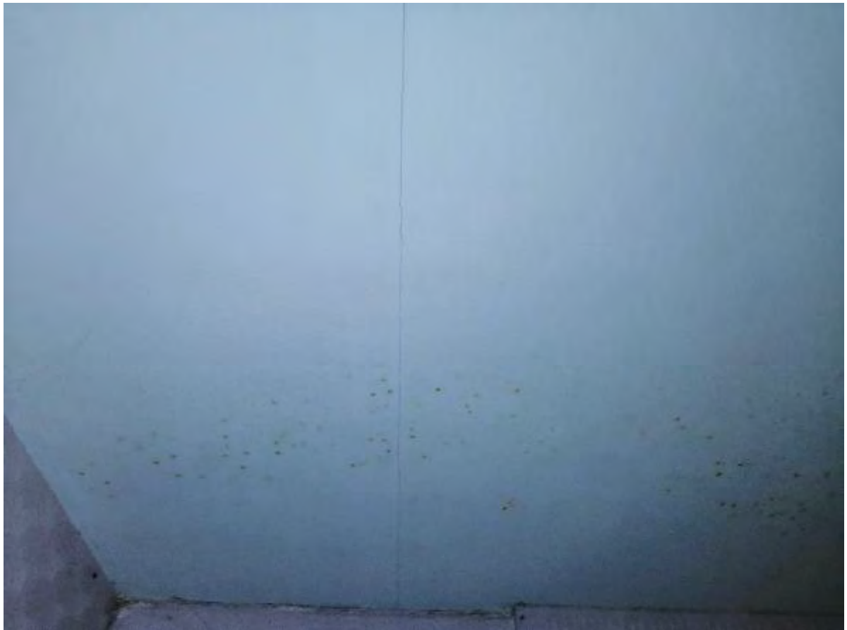
Photo 204 – Ceiling Cracking (Hall)
