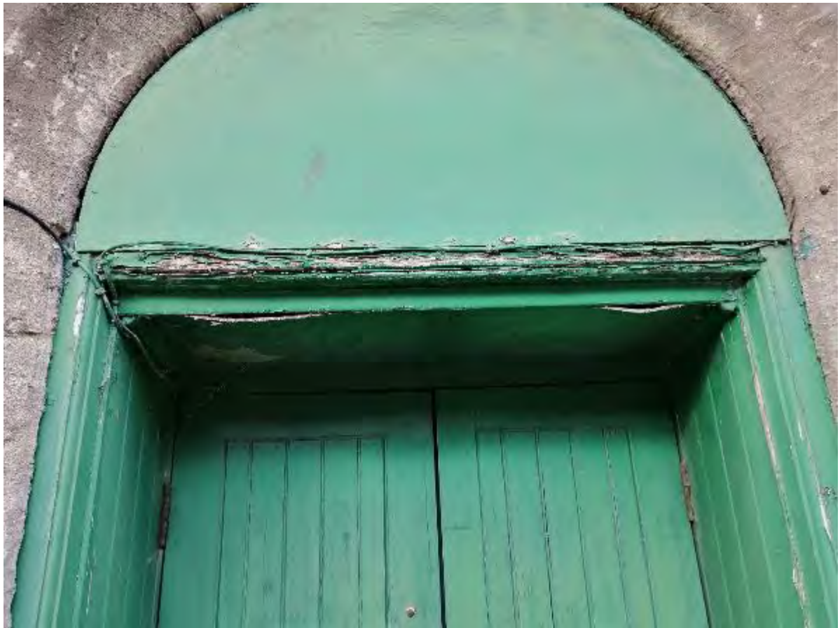
Photo 71 – Weathering and Rot to Timber Door Frame (Front Wall Elevation)
