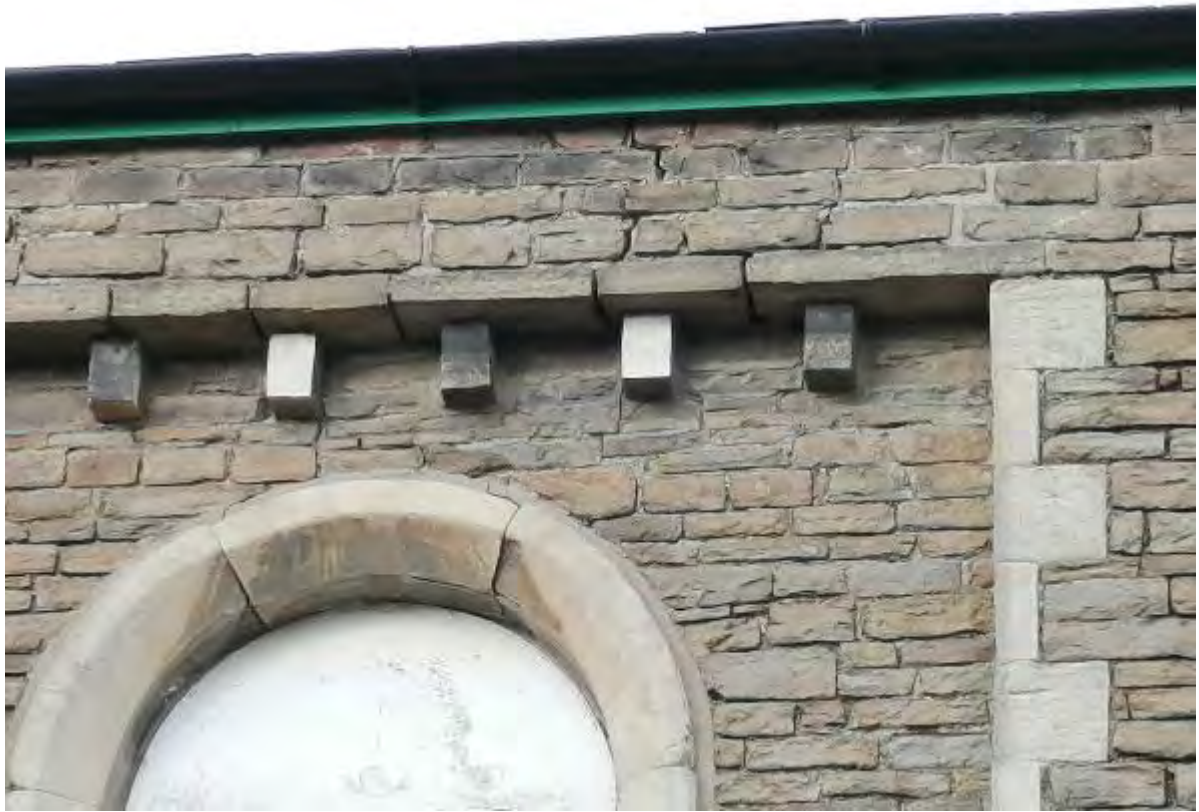
Photo 69 – Cracking to Mortar Above Archway (Front Wall Elevation)
