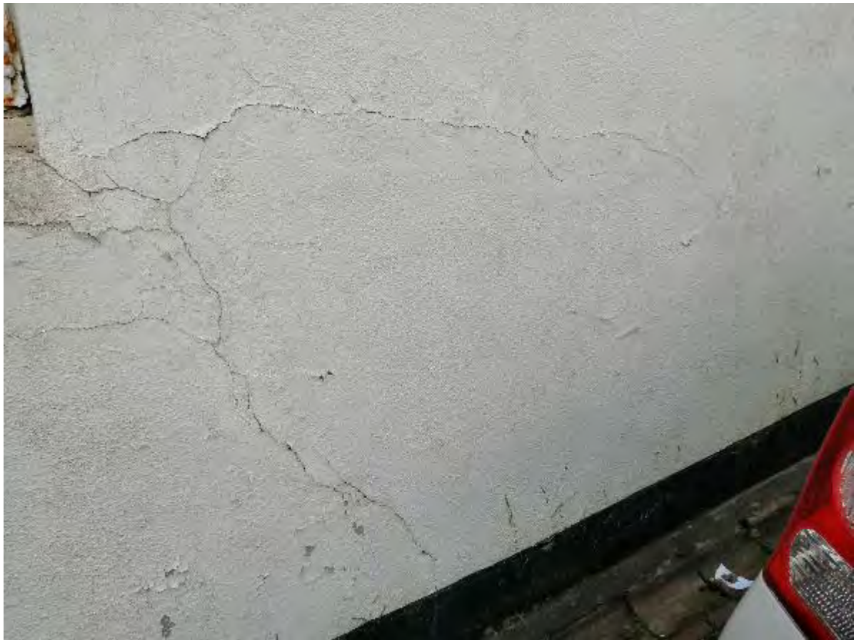
Photo 79 – Render Shrinkage Cracking (Right Wall Elevation)
