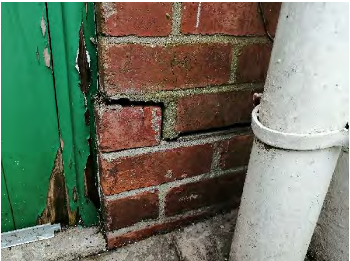
Photo 36 – Cracking to Mortar (Left Wall Elevation)
