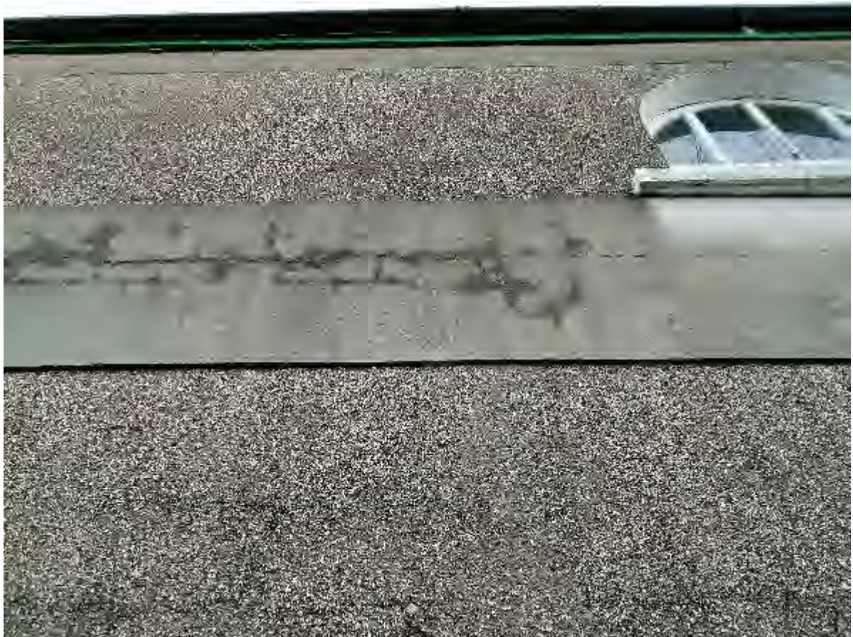
Photo 39 – Render Cracking Around Old Opening (Left Wall Elevation)
