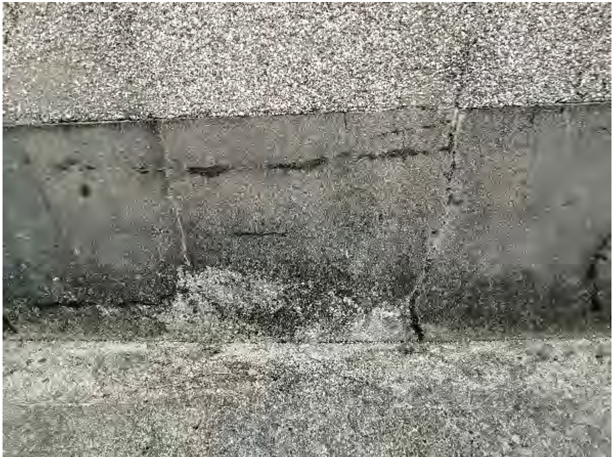
Photo 42 – Render Shrinkage Cracking (Left Wall Elevation)
