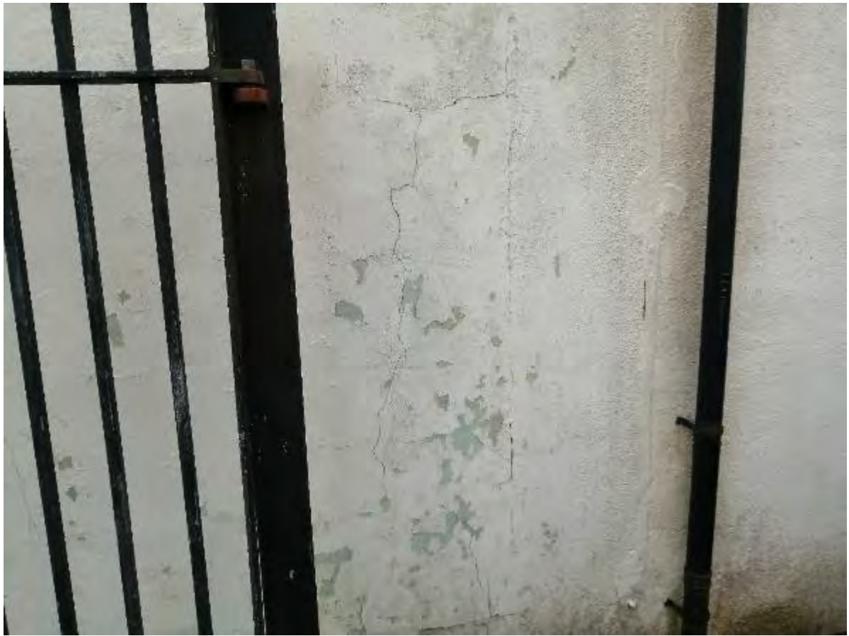
Photo 77 – Render Shrinkage Cracking (Right Wall Elevation)
