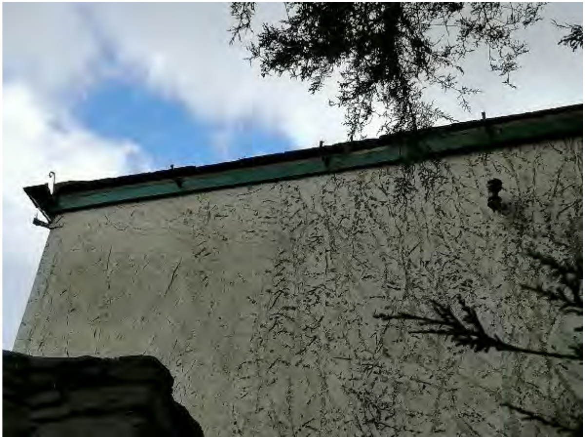
Photo 12 – Missing Guttering (Rear Roof Profile)
