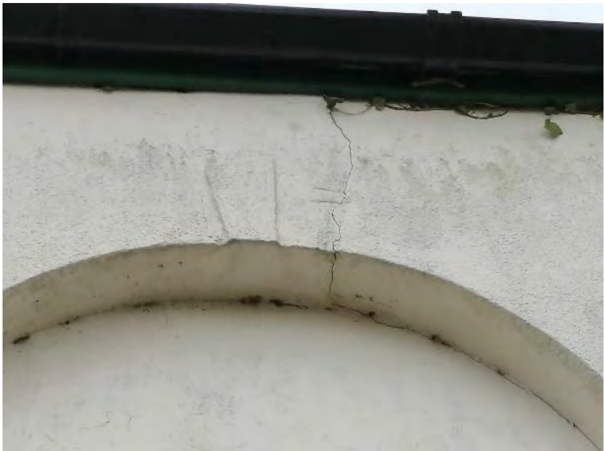
Photo 82 – Render Shrinkage Cracking (Right Wall Elevation)
