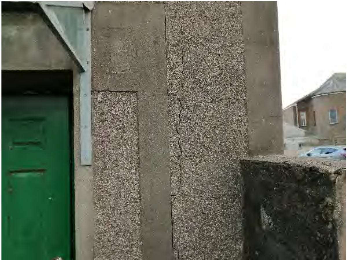
Photo 57 – Wall Crack (Left Wall Elevation)
