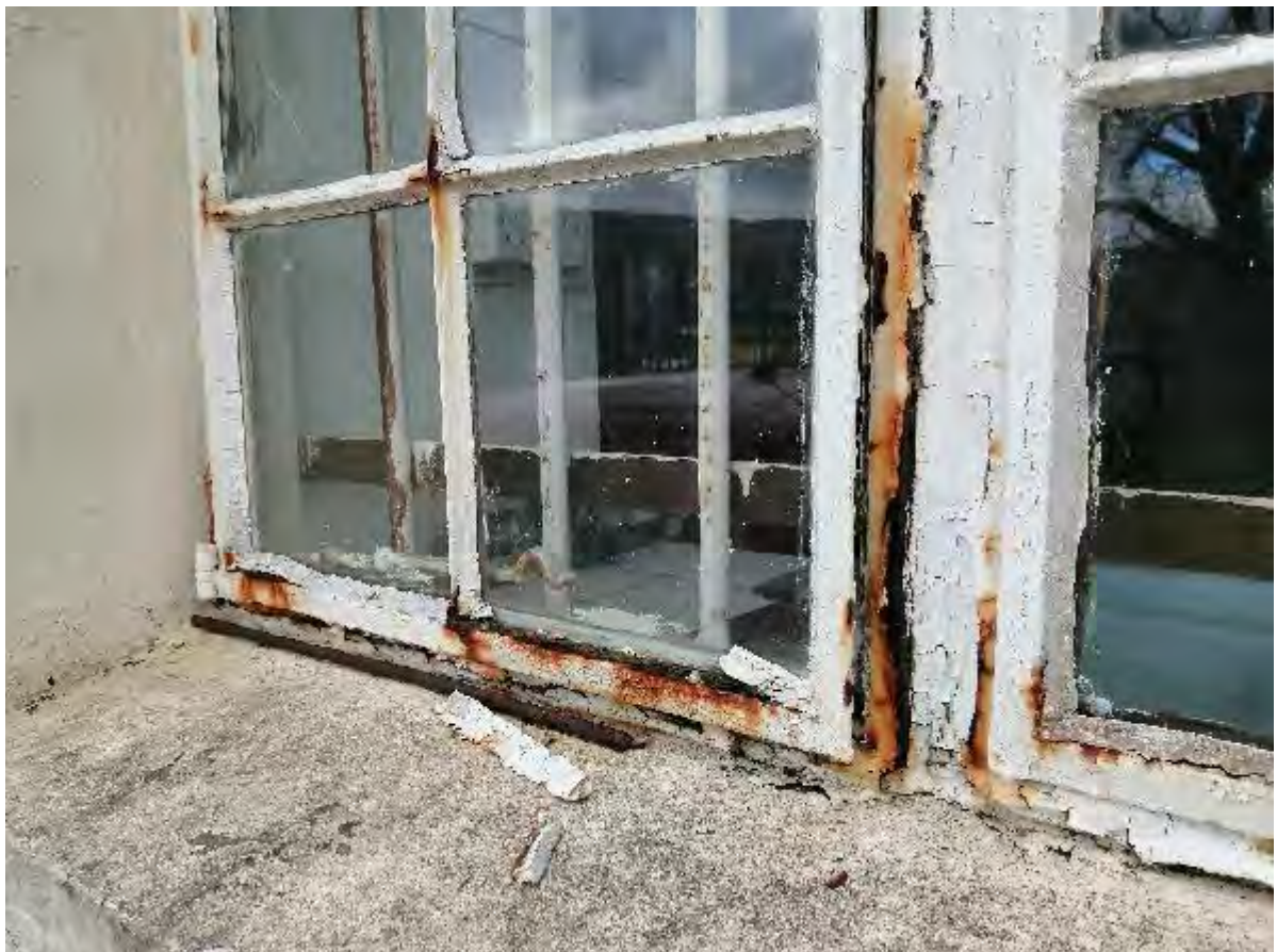
Photo 84 – Corrosion to Metal Window Frame (Right Wall Elevation)
