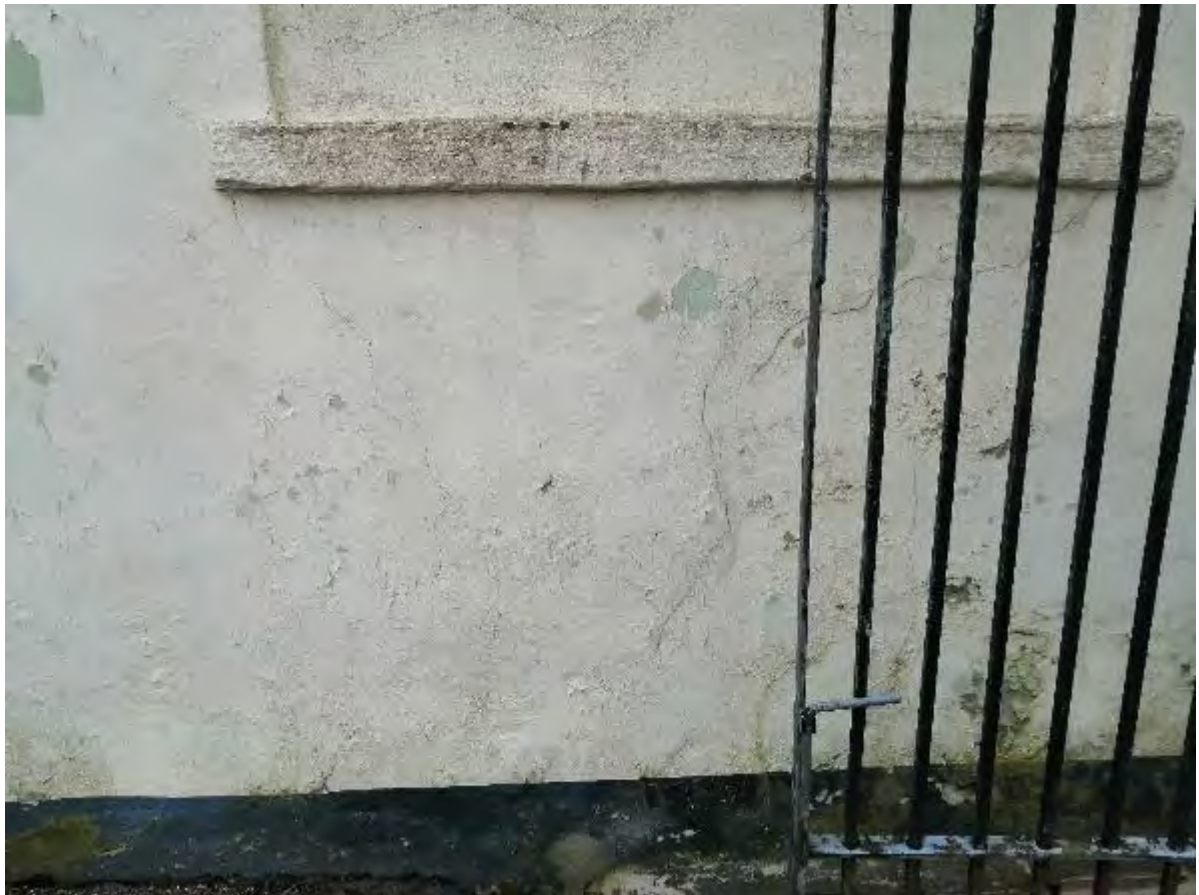
Photo 74 – Render Shrinkage Cracking (Right Wall Elevation)
