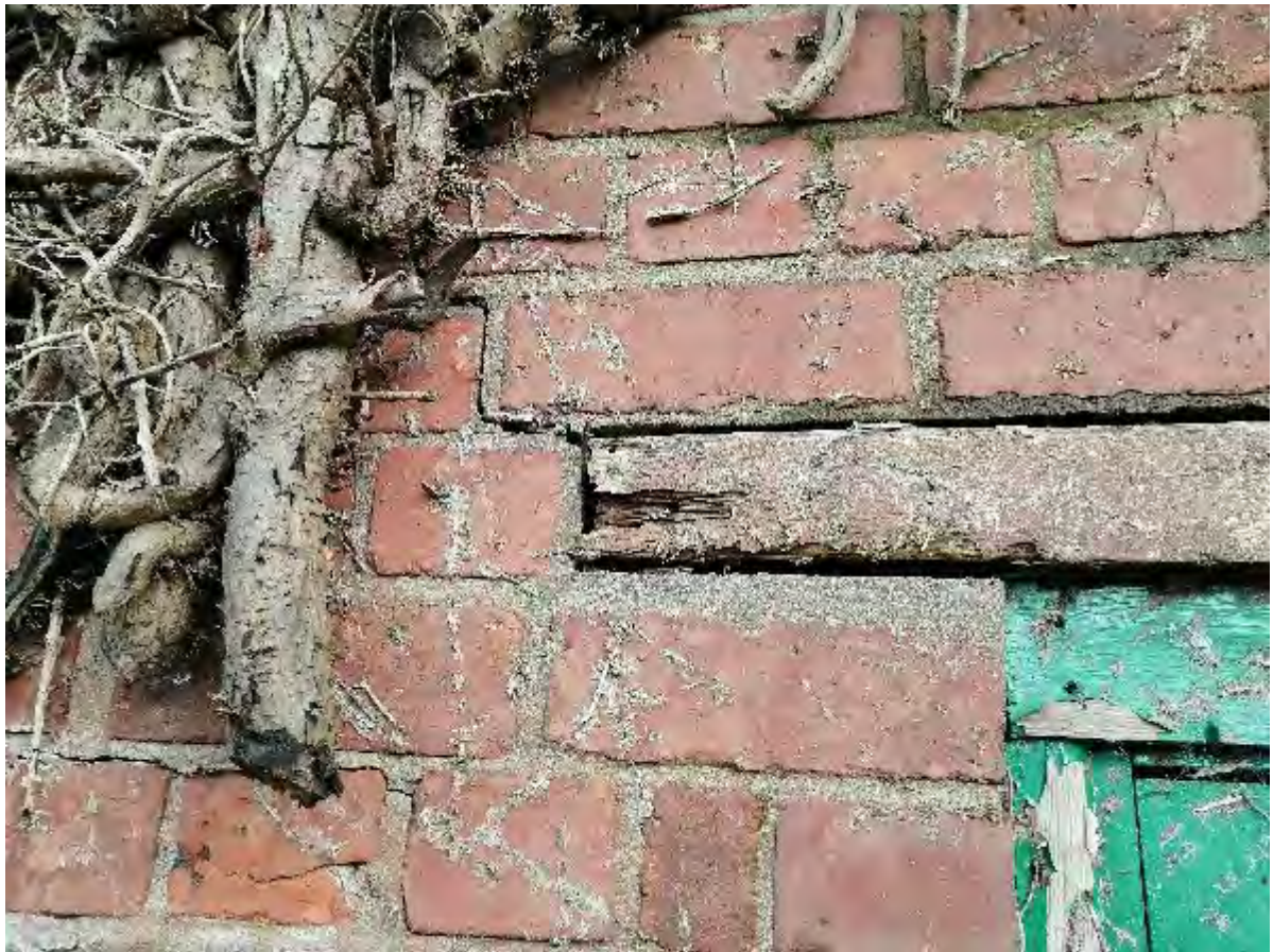
Photo 35 – Steped Cracking to Mortar and Rotten Doorway Lintel (Left Wall Elevation)
