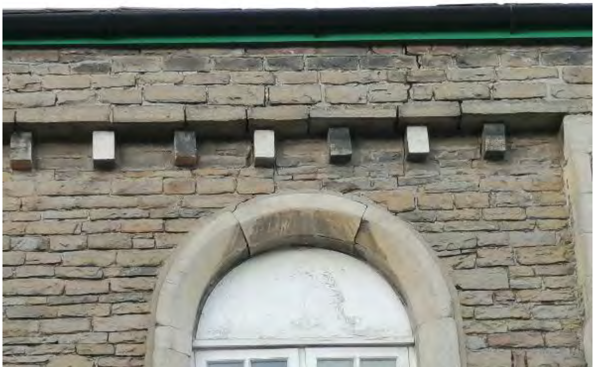
Photo 58 – Cracking to Mortar Above Archway (Front Wall Elevation)
