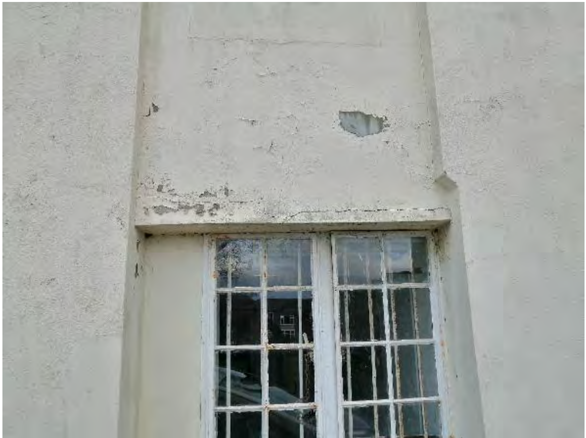
Photo 83 – Render Shrinkage Cracking (Right Wall Elevation)
