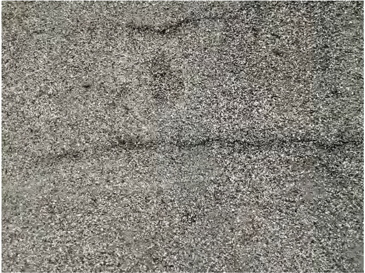
Photo 45 – Render Shrinkage Cracking (Left Wall Elevation)
