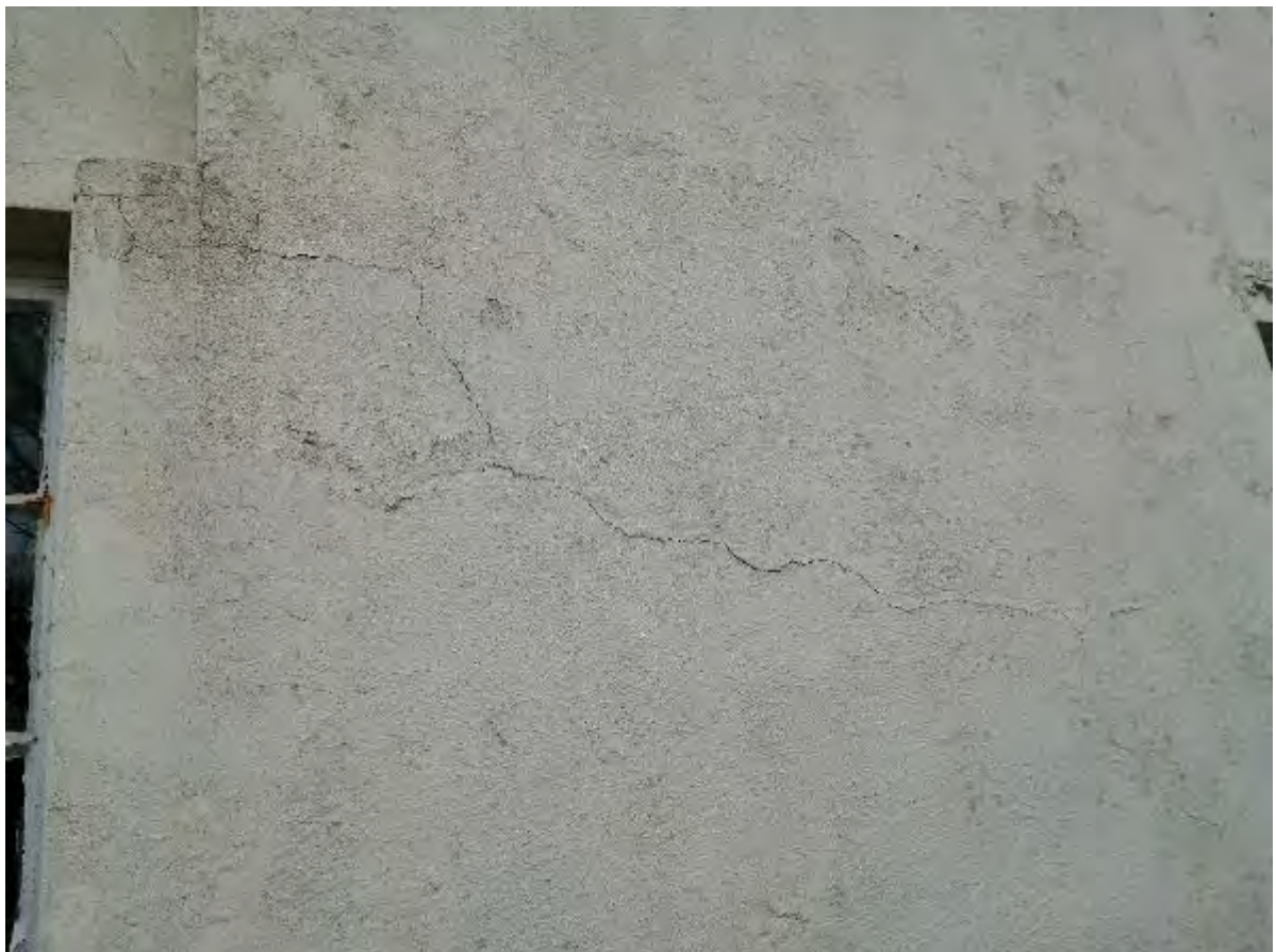
Photo 80 – Render Shrinkage Cracking (Right Wall Elevation)
