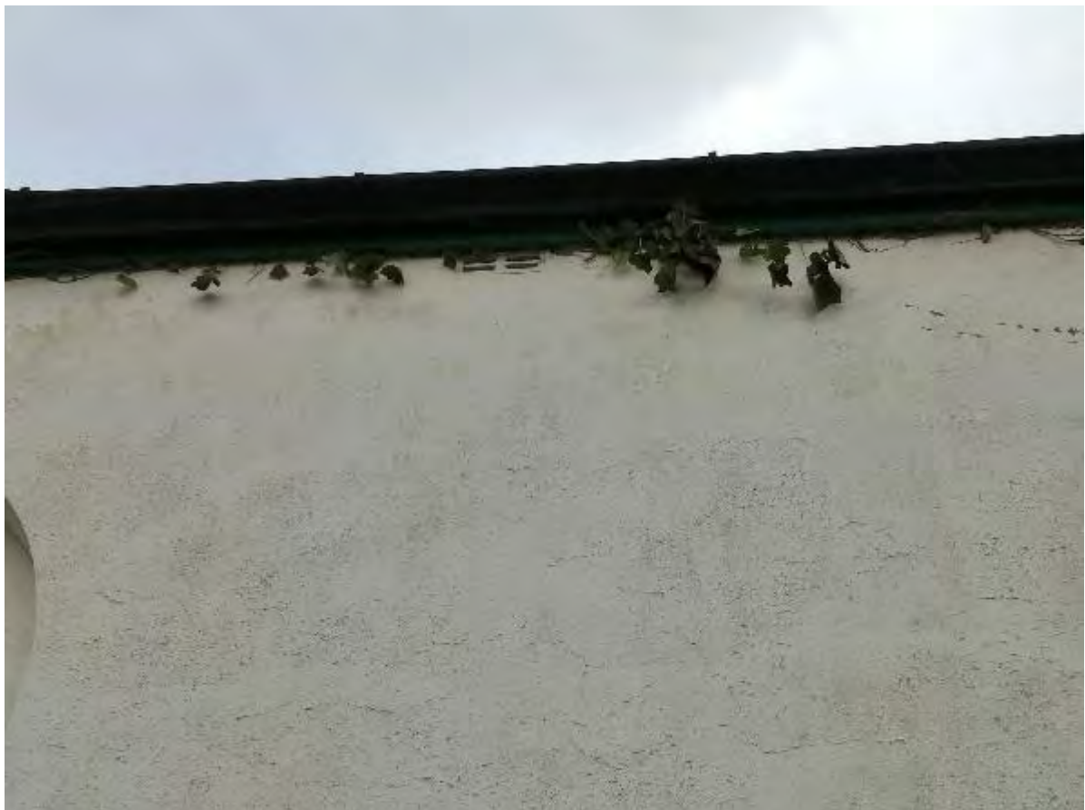
Photo 21 – Vegetation Growth (Right Roof Profile)
