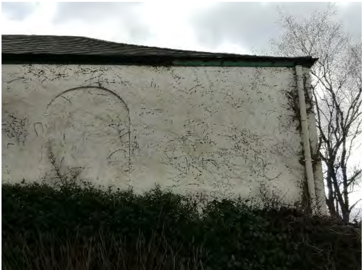
Photo 30 – Vegetation Growth (Rear Wall Elevation)
