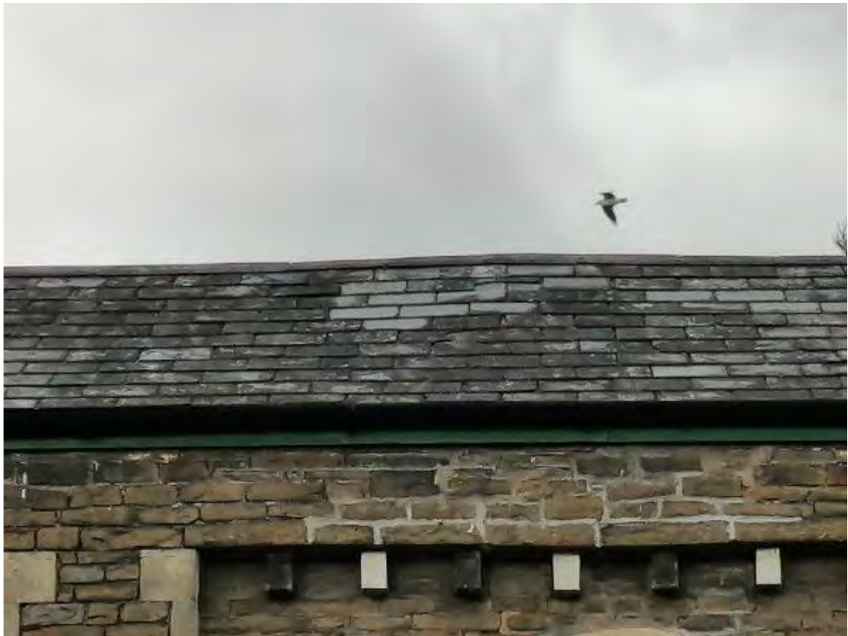
Photo 20 – Damaged Slate Tiles and Sagging to Roof (Front Roof Profile)
