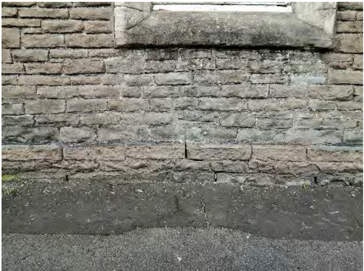
Photo 66 – Cracking to Mortar (Front Wall Elevation)
