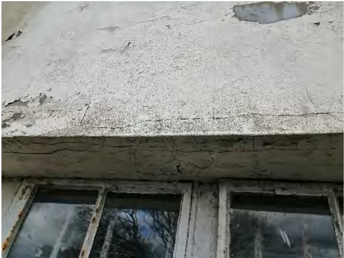
Photo 87 – Render Shrinkage Cracking (Right Wall Elevation)
