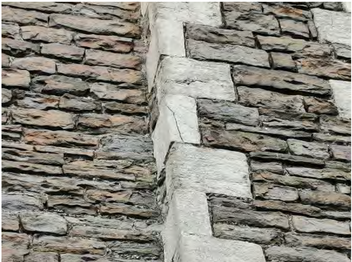
Photo 68 – Cracking to Stonework (Front Wall Elevation)
