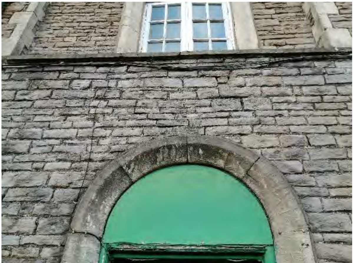
Photo 70 – Cracking to Mortar Above Archway (Front Wall Elevation)
