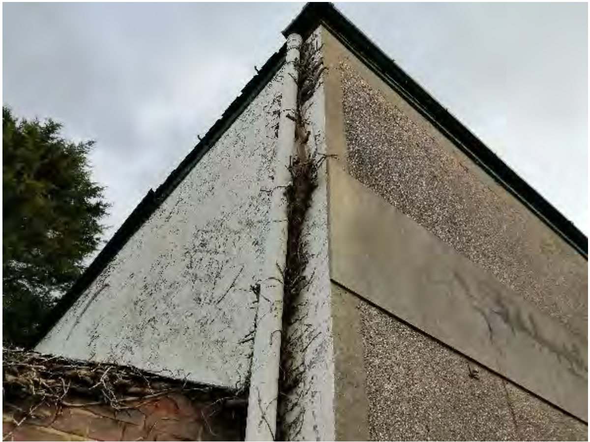
Photo 31 – Vegetation Growth (Rear Wall Elevation)
