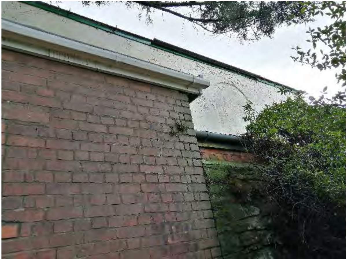
Photo 33 – Vegetation Growth (Rear Wall Elevation)
