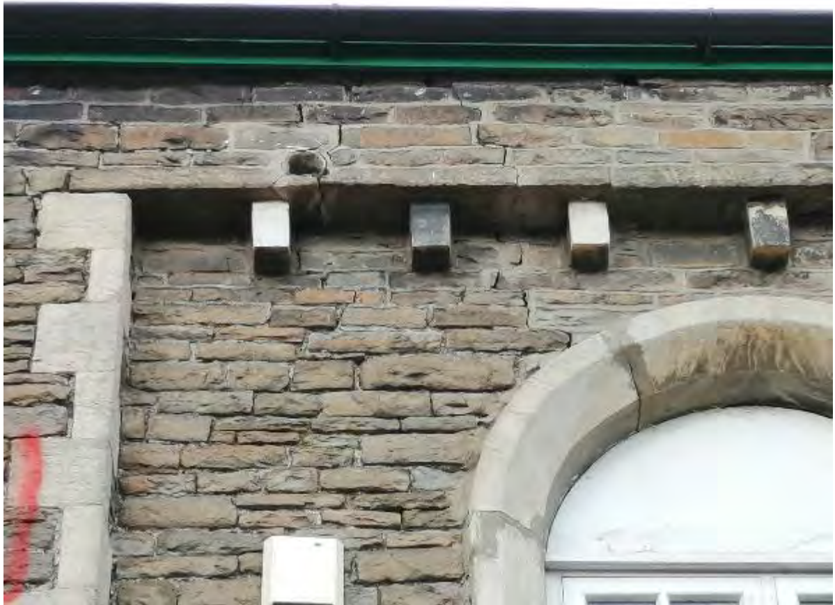
Photo 59 – Cracking to Mortar Above Archway (Front Wall Elevation)
