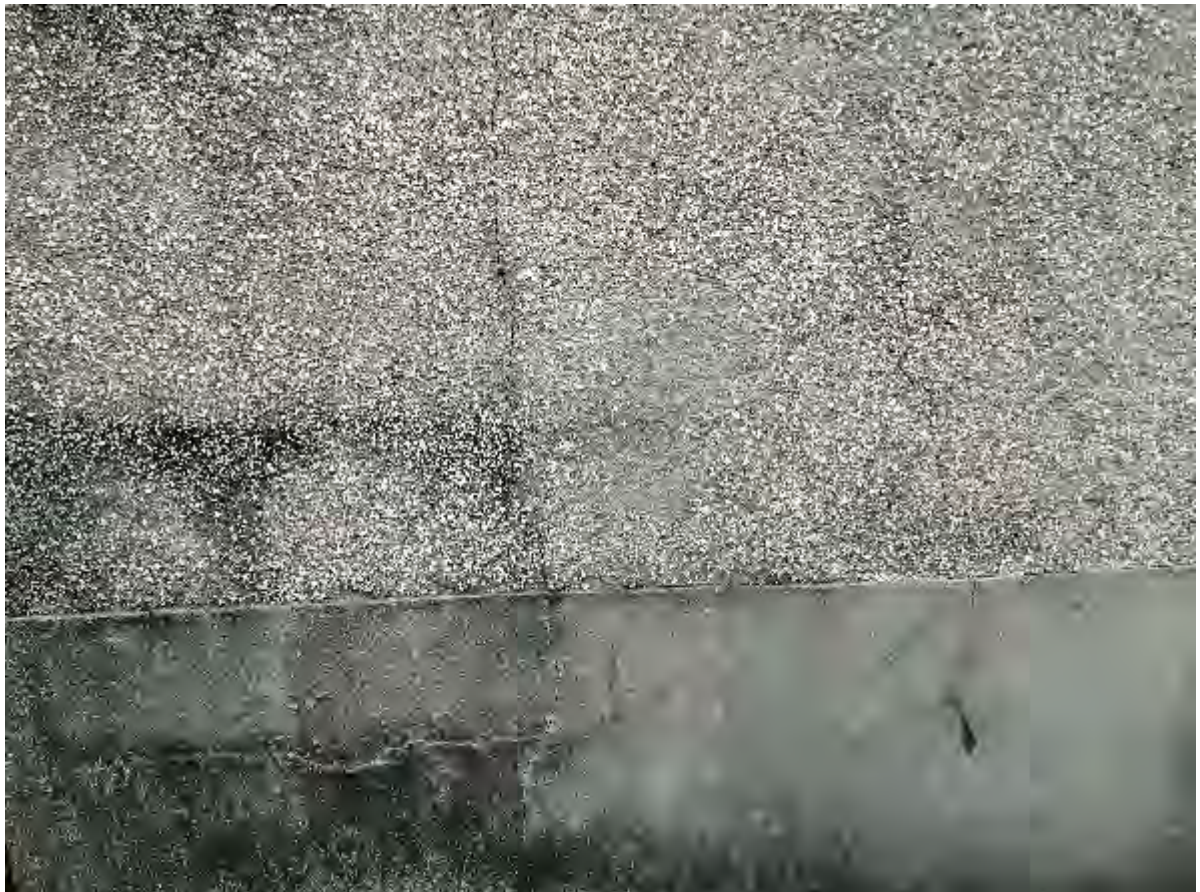
Photo 54 – Render Shrinkage Cracking (Left Wall Elevation)
