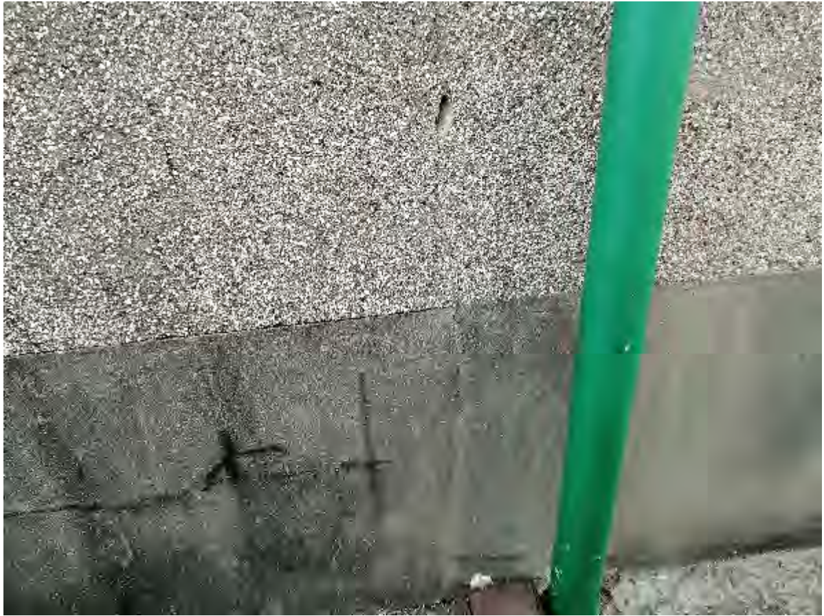
Photo 41 – Render Cracking Around Old Opening (Left Wall Elevation)
