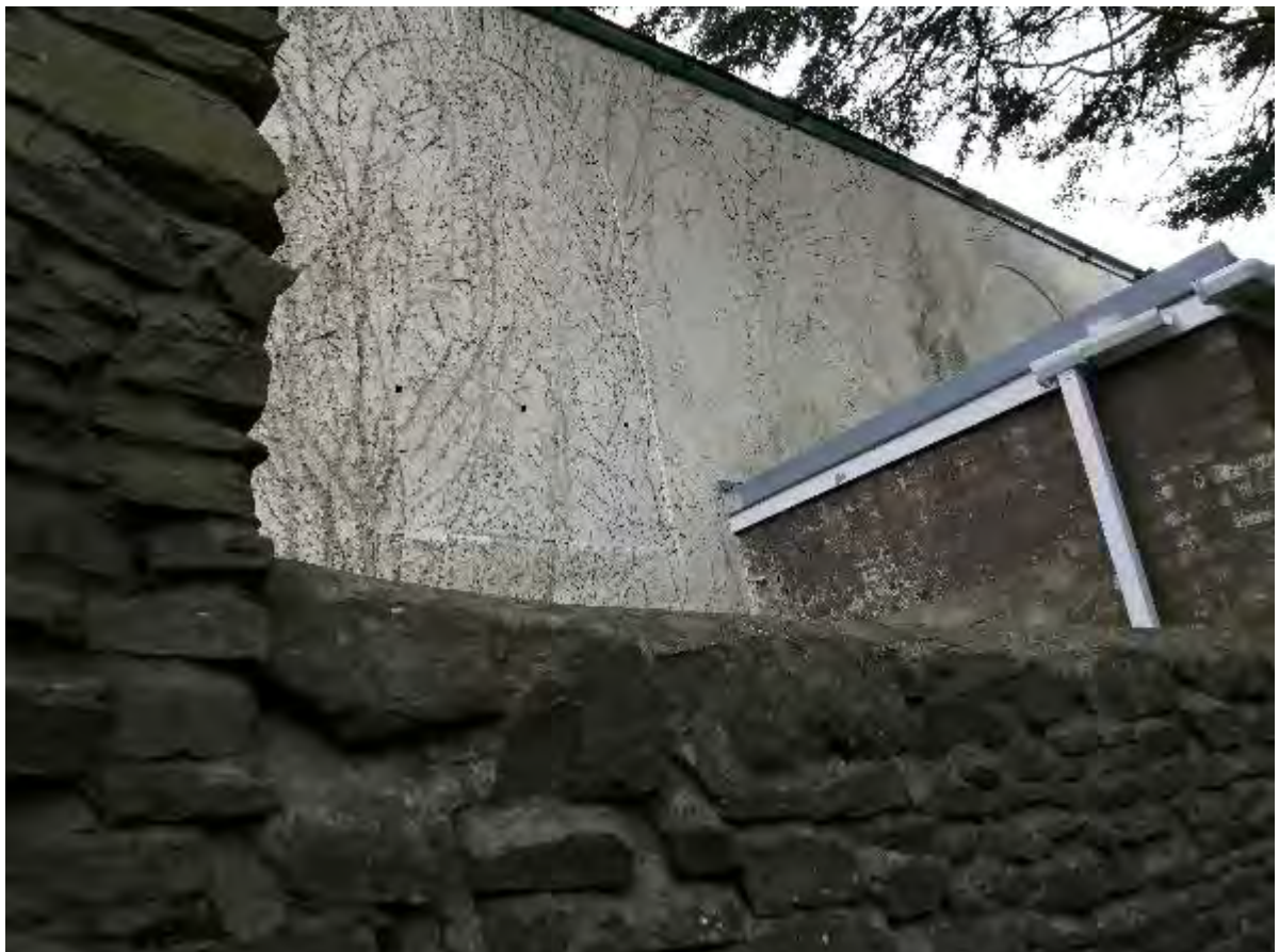
Photo 32 – Vegetation Growth (Rear Wall Elevation)
