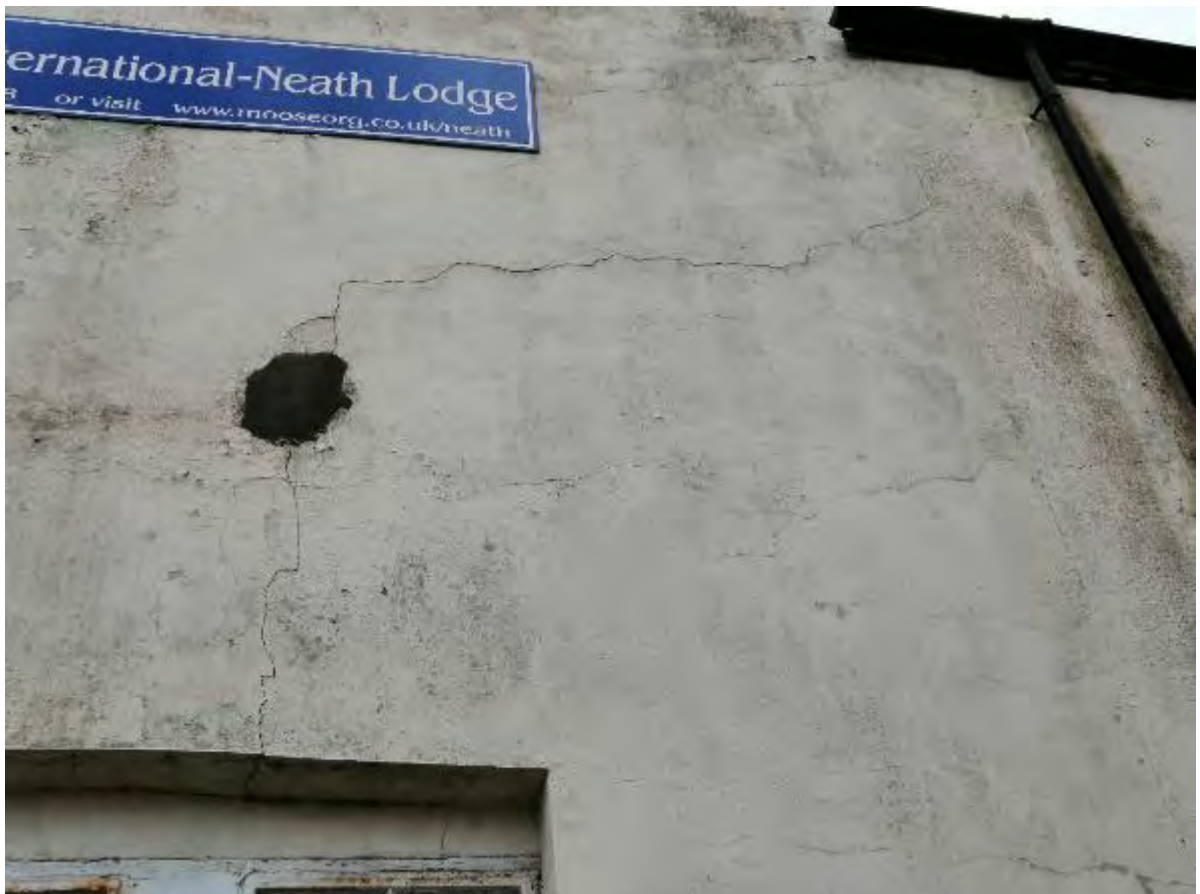
Photo 76 – Render Shrinkage Cracking (Right Wall Elevation)
