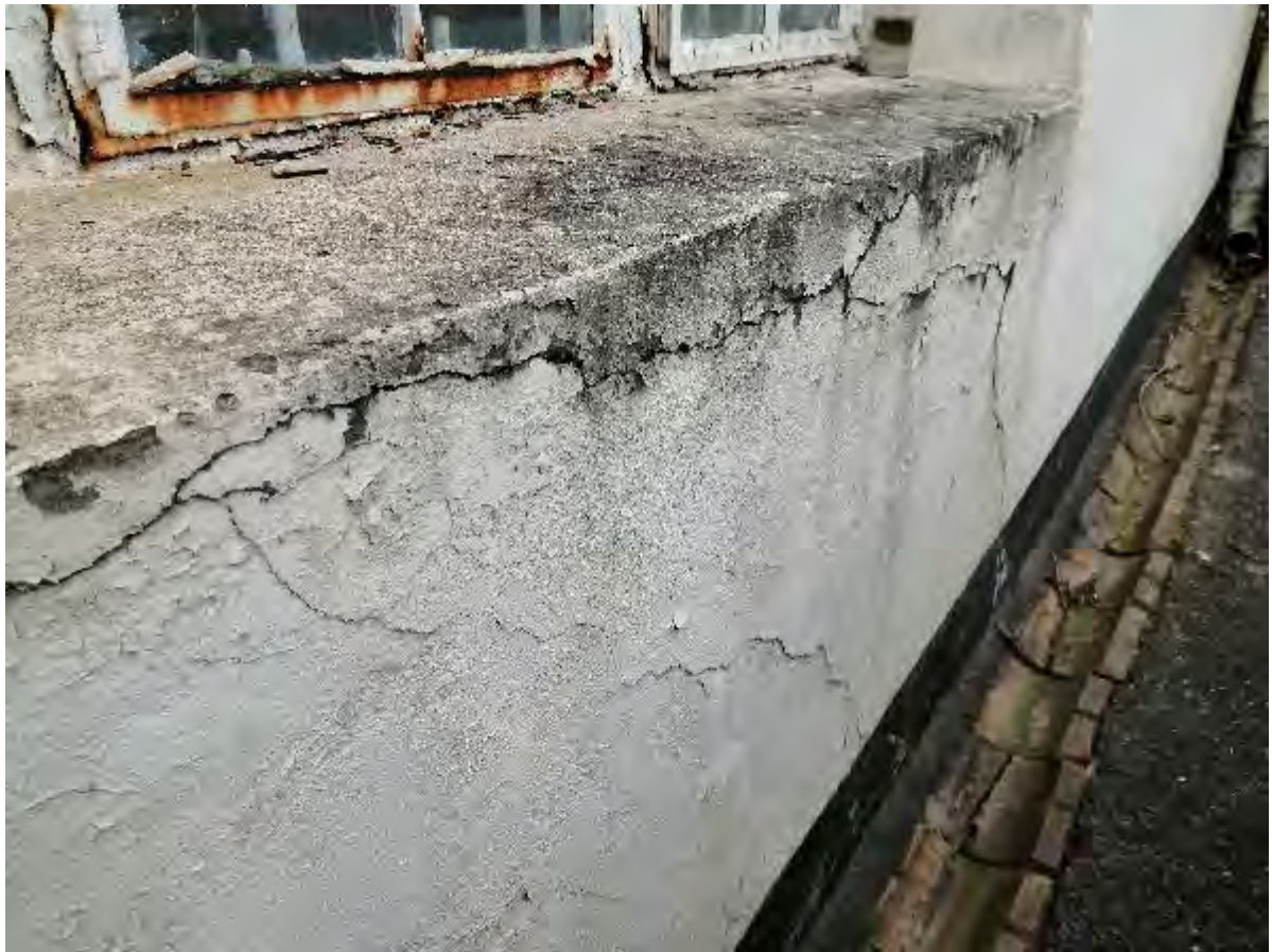
Photo 85 – Render Shrinkage Cracking (Right Wall Elevation)
