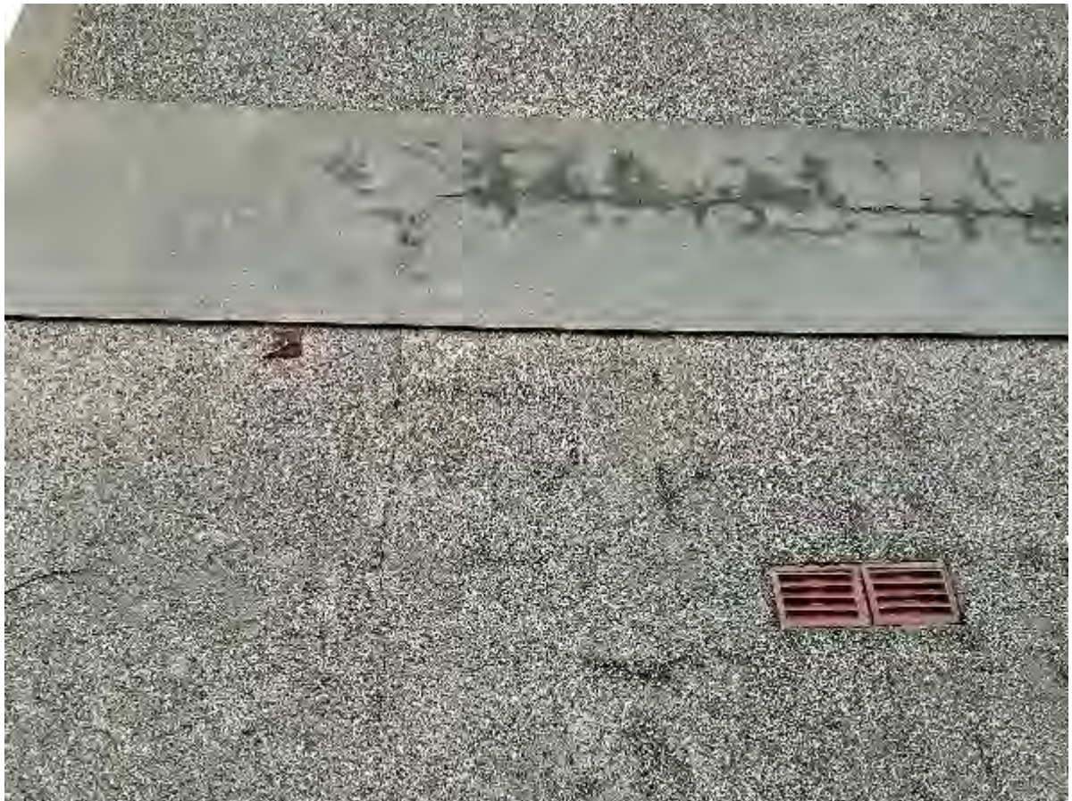
Photo 37 – Render Cracking Around Old Opening (Left Wall Elevation)
