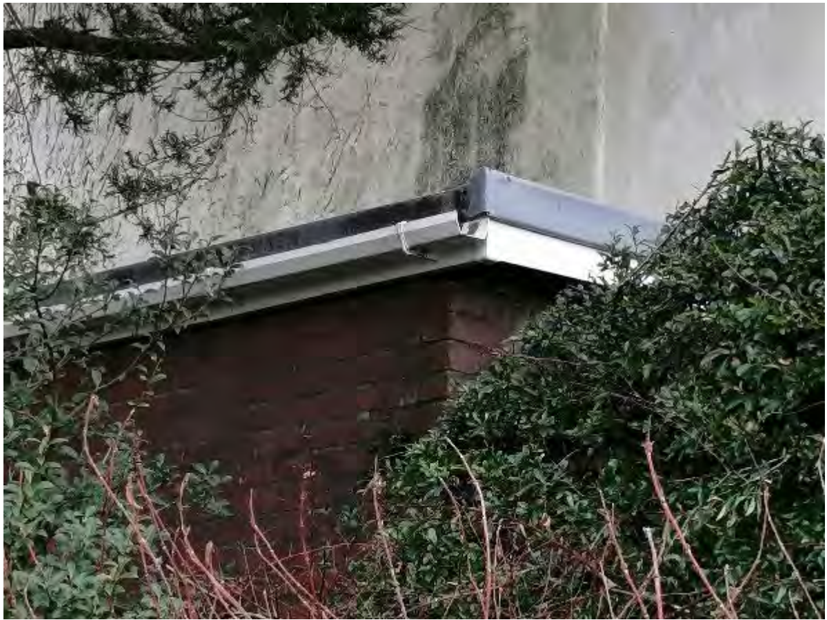
Photo 14 – Defective Guttering (Rear Roof Profile)
