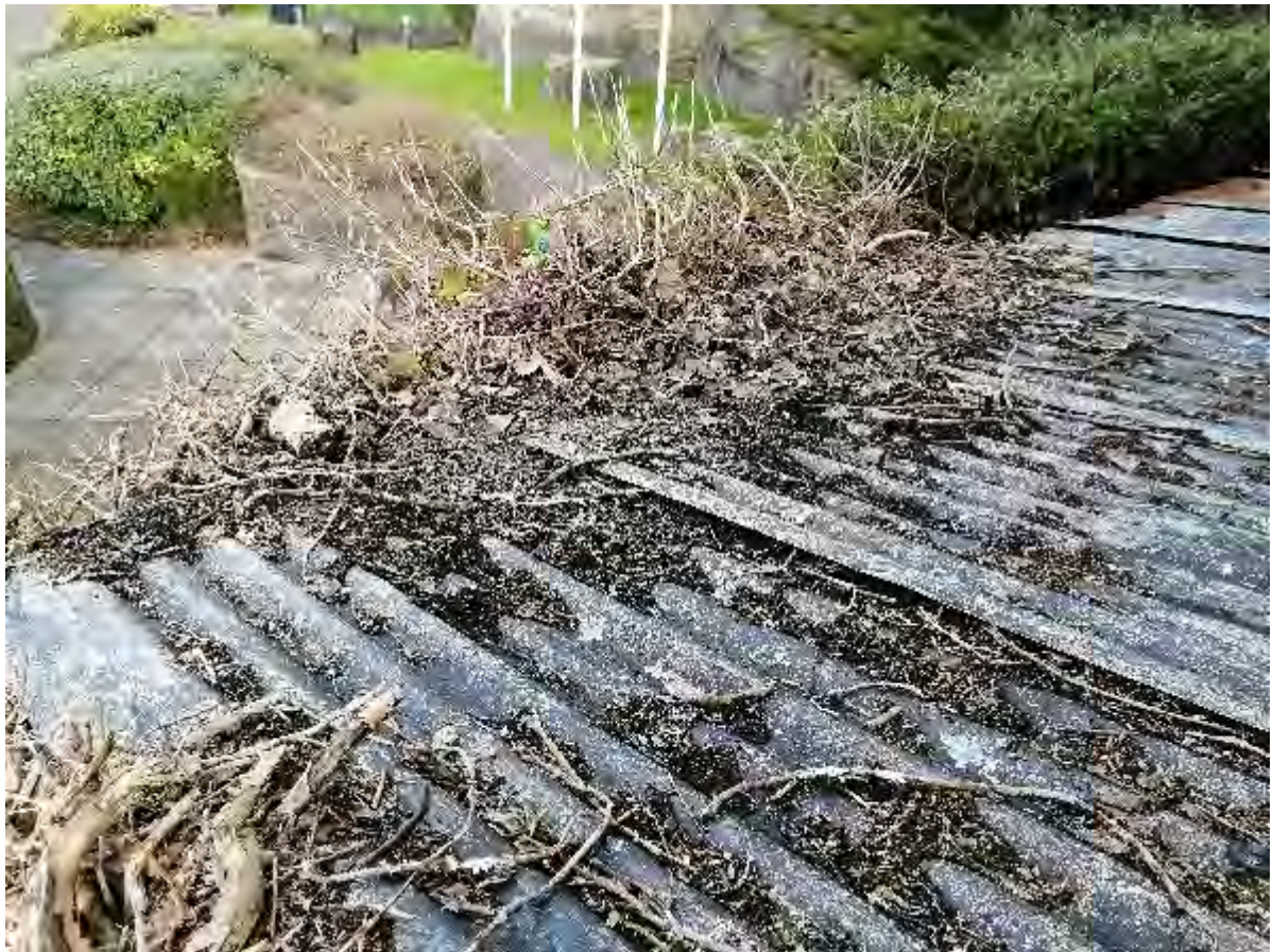
Photo 18 – Vegetation Growth and Corrosion to Sheeting Material (Rear Roof Profile)
