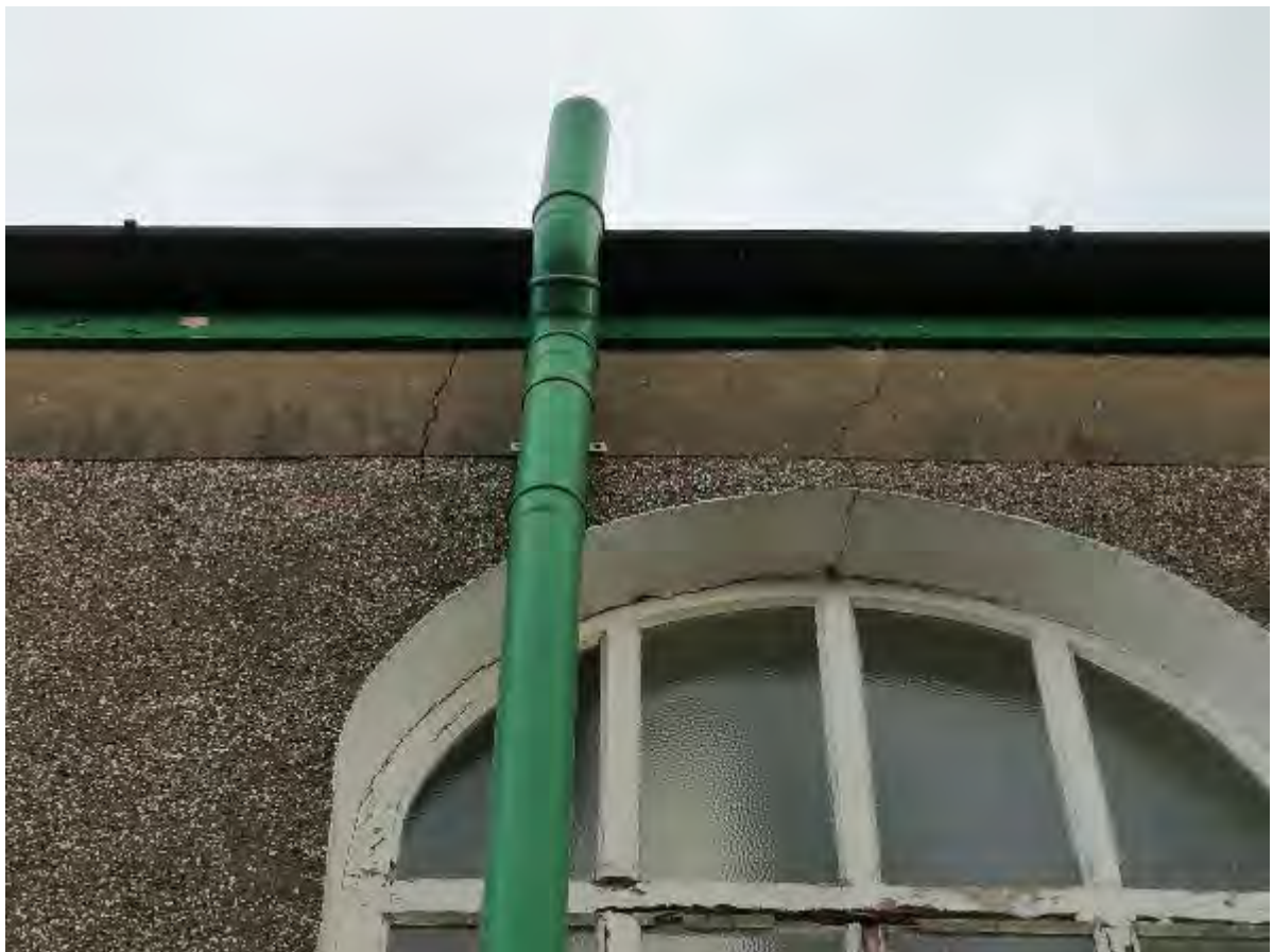
Photo 48 – Render Shrinkage Cracking (Left Wall Elevation)
