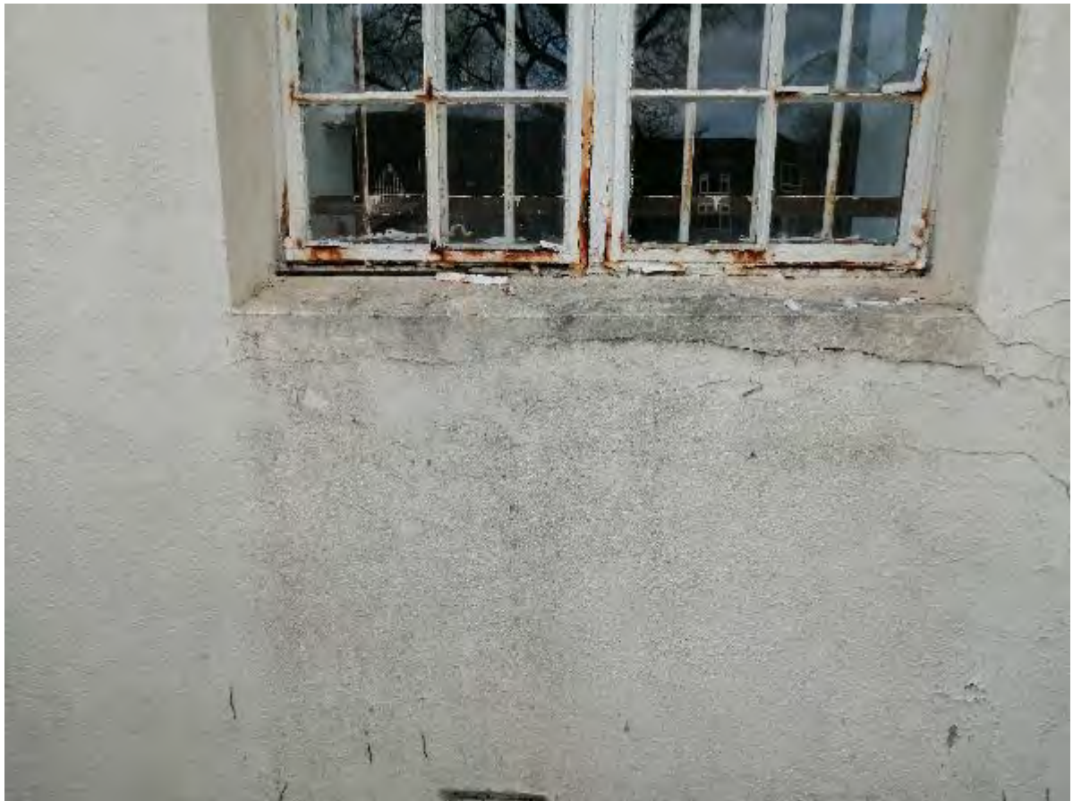
Photo 78 – Render Shrinkage Cracking (Right Wall Elevation)
