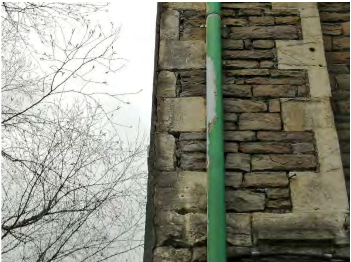
Photo 60 – Weathered Mortar and Exposed Render Edge (Front Wall Elevation)
