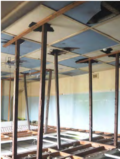
Fig 20: Void over lay-in-grid ceiling with cement tile ceiling, damaged by modern ceiling structure.
