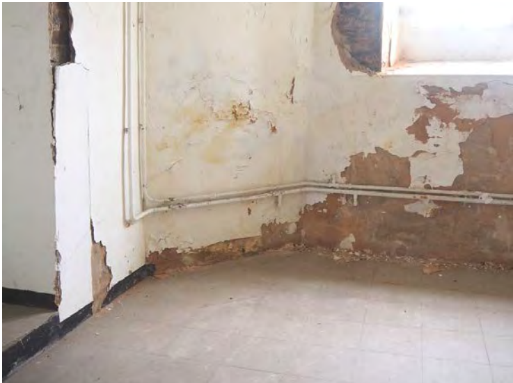
Fig 32: Kitchen store (ground floor) with modern plaster finish affected by damp and surface mounted pipework. Possible former chimney stack in corner.
