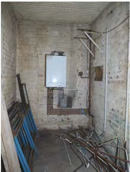
Fig 27: External store (east) housing gas fired boiler.
