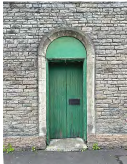
Fig 11: Principal entrance located on south elevation abutting Castle Street. Timber doors in poor condition throughout.
