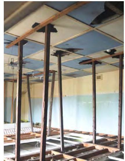
Fig 15: Void over lay-in-grid ceiling with cement tile ceiling, damaged by modern ceiling structure.
