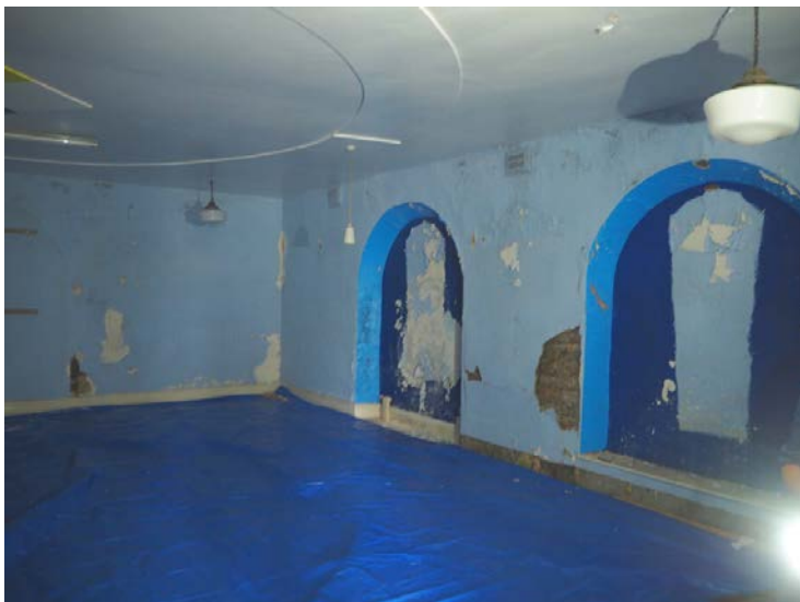
Fig 23: First floor ceremony room (within former chapel). Chapel window openings blocked and external walls covered with cementitious plaster. Boarded timber floor below tarpaulin.
