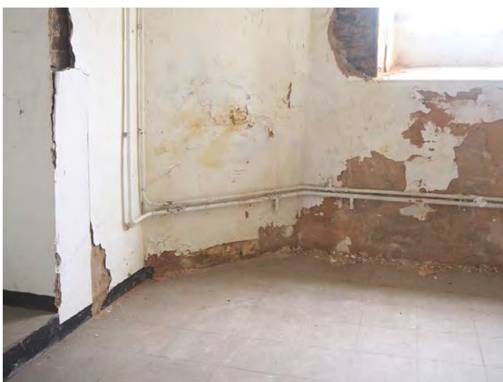
Fig 27: Kitchen store (ground floor) with modern plaster finish affected by damp and surface mounted pipework. Possible former chimney stack in corner.
