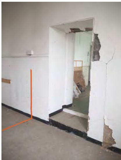
Fig 28: Access between kitchen and kitchen store through unsupported doorway.
