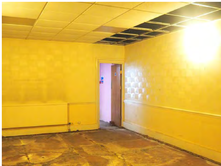
Fig 29: Ground floor social room with route through to kitchen store/stairs to first floor hallway. Image shows previous lay-in-grid ceiling/contemporary finishes and cracked concrete floor.
