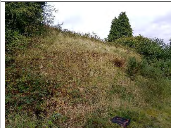
Plate 9: Photograph of minor slip present to the central eastern area of the site in fill batter.
