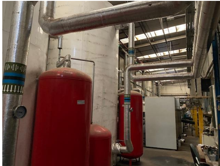
Photo 4 – internal floorspace dedicated to boiler apparatus which generates heat for the drying process
