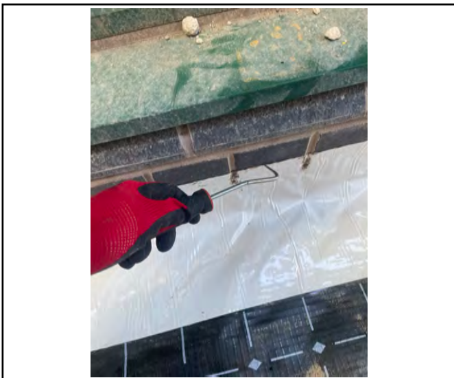
Pick and probe test carried out to the retro fit detail.
