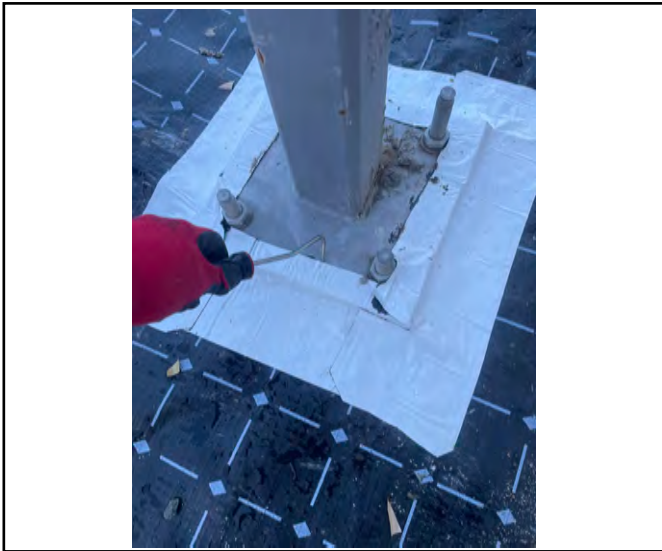
Pick and probe test carried out to a sealed steel column.
