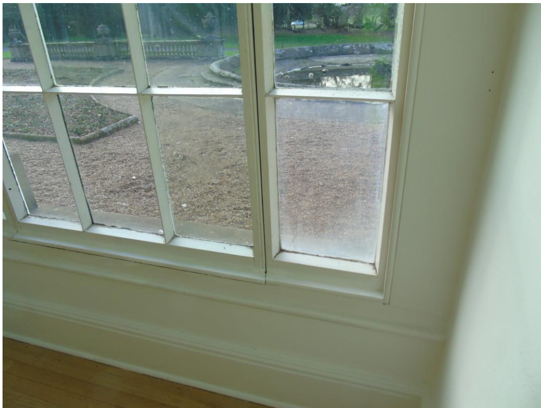
Figure 6: Inappropriate Replacement Glass
