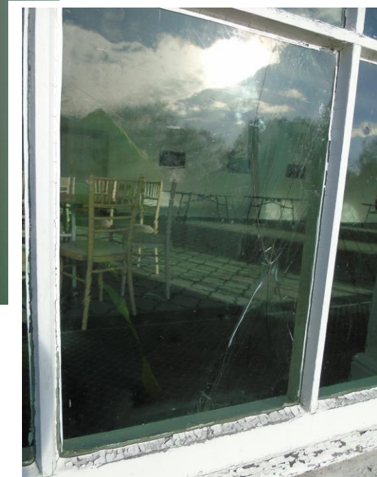
Figure 5: Cracked Cylinder Glass, Exterior
