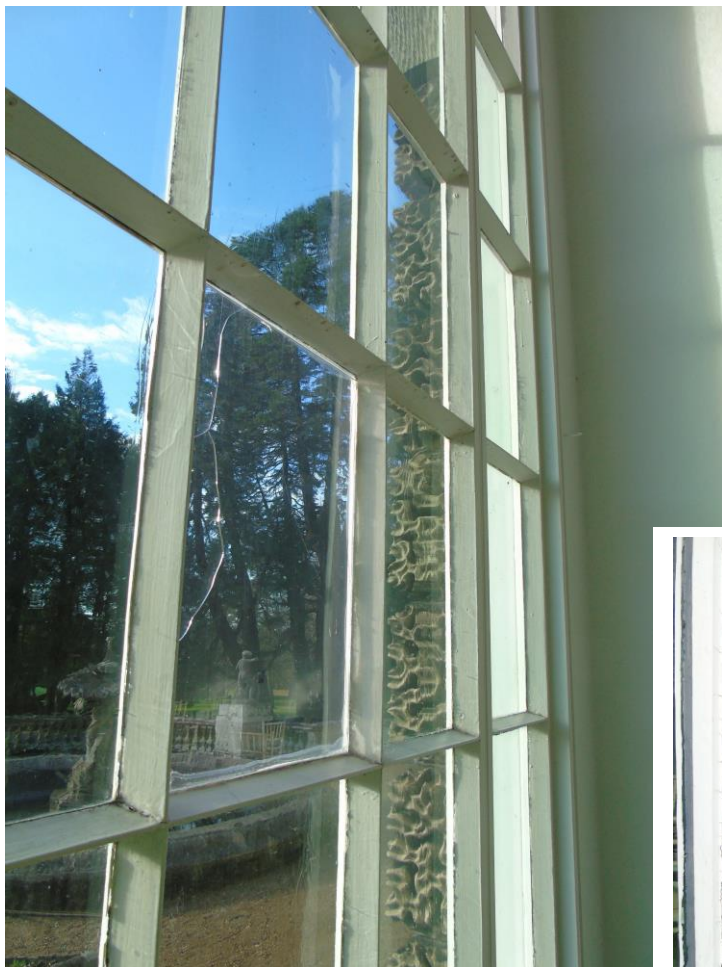
Figure 4: Cracked Cylinder Glass, Interior
