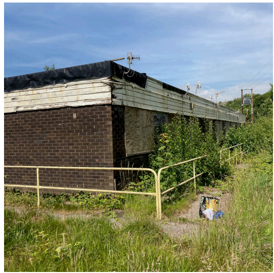
Figure 11. Damage to wooden cladding, south west corner.
