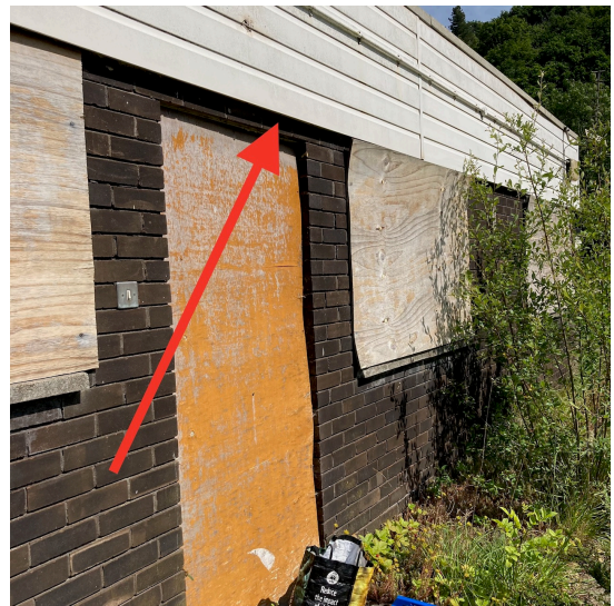
Figure 7. uPVC cladding – gaps underneath.
