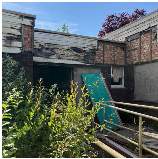
Figure 12. Damage to wooden cladding, eastern elevation.
