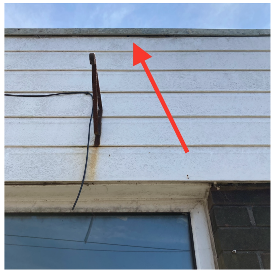
Figure 13. Suspected roost access point, dropping on window below.
