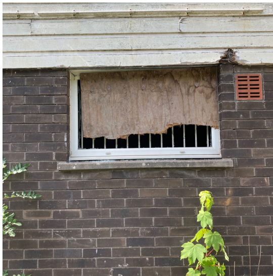
Figure 6. Window to the rear with missing glass.
