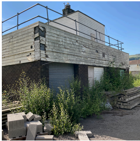
Figure 10. Damage to wooden cladding, south east corner.
