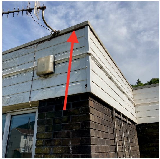
Figure 9. Gaps along roof verge at top of cladding.
