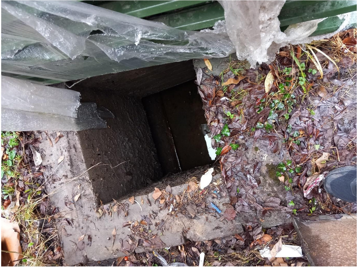
Existing Storm Water Inspection Chamber constructed and aproved by Local Authority on rebuild of garage structure that being Carters MOT Centre.
