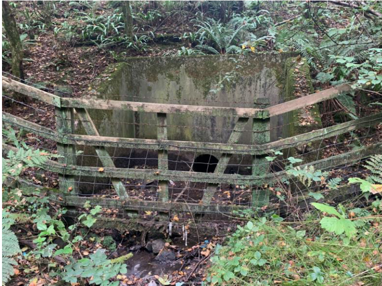
Figure 4: Original Watercourse Emanating from 450mm diameter Pipe under M4
