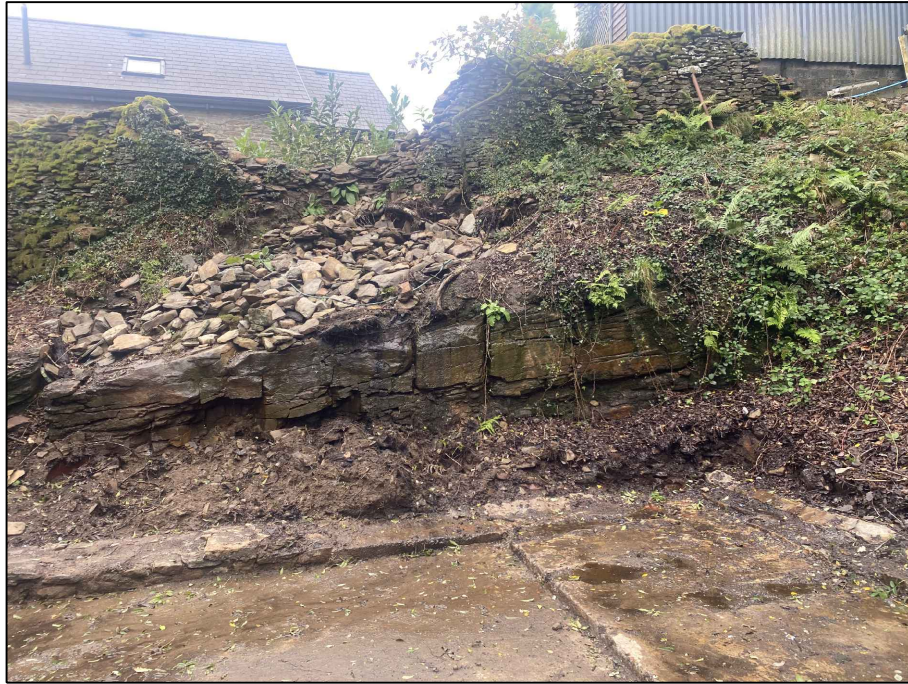
Pic.8 View of slab / perimeter toward North East. Note the close proximity of the rock face bank and level of vegetation earth above slab level
