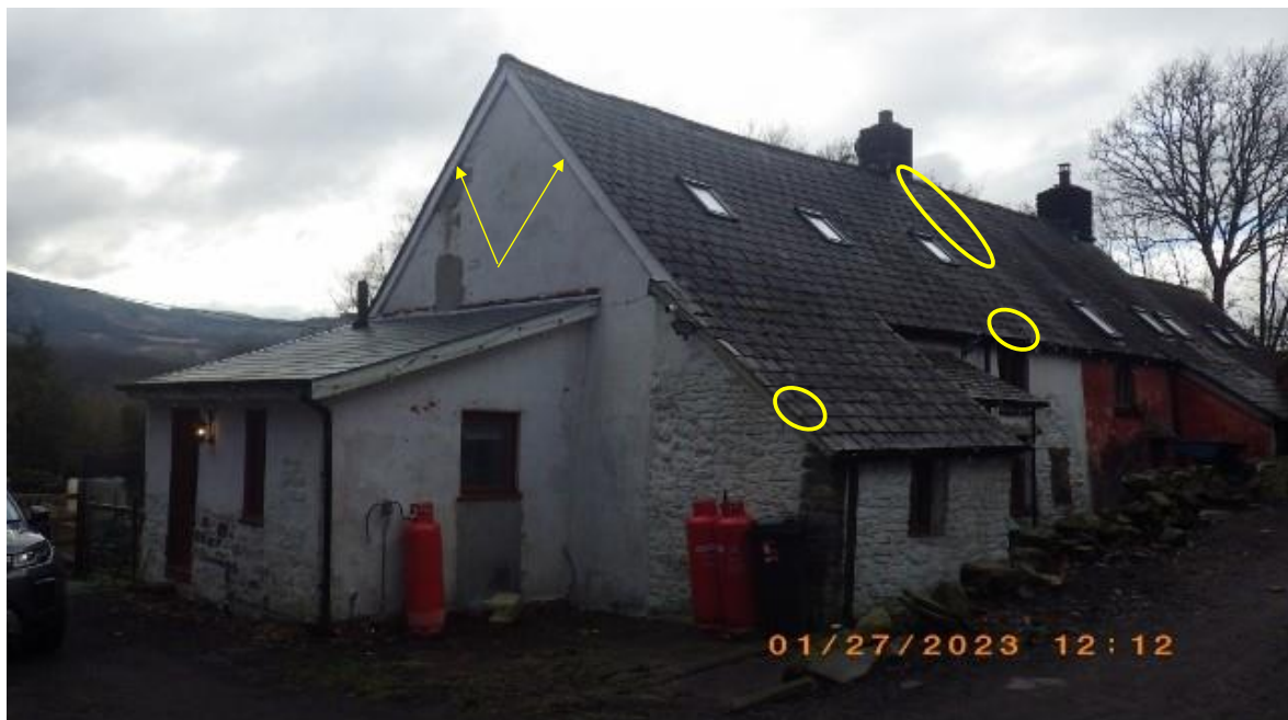
Gaps under roof tiles and eaves on the north and east elevation of the main house
