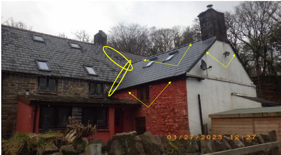
Gaps under roofing tiles, around roof valleys and gable eaves on the south and west elevation of the extension
