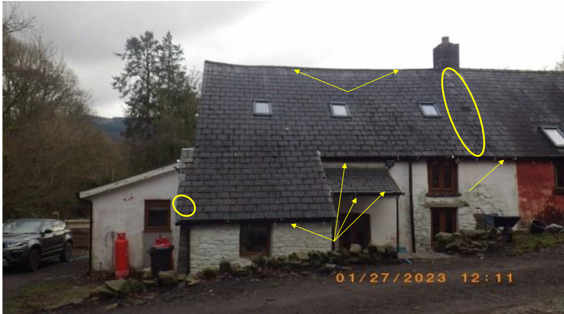
Gaps under roof tiles and eaves on the north elevation of the house
