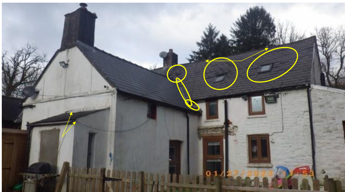
Gaps under roof tiles and around the roof valley on the south elevation of the main house
