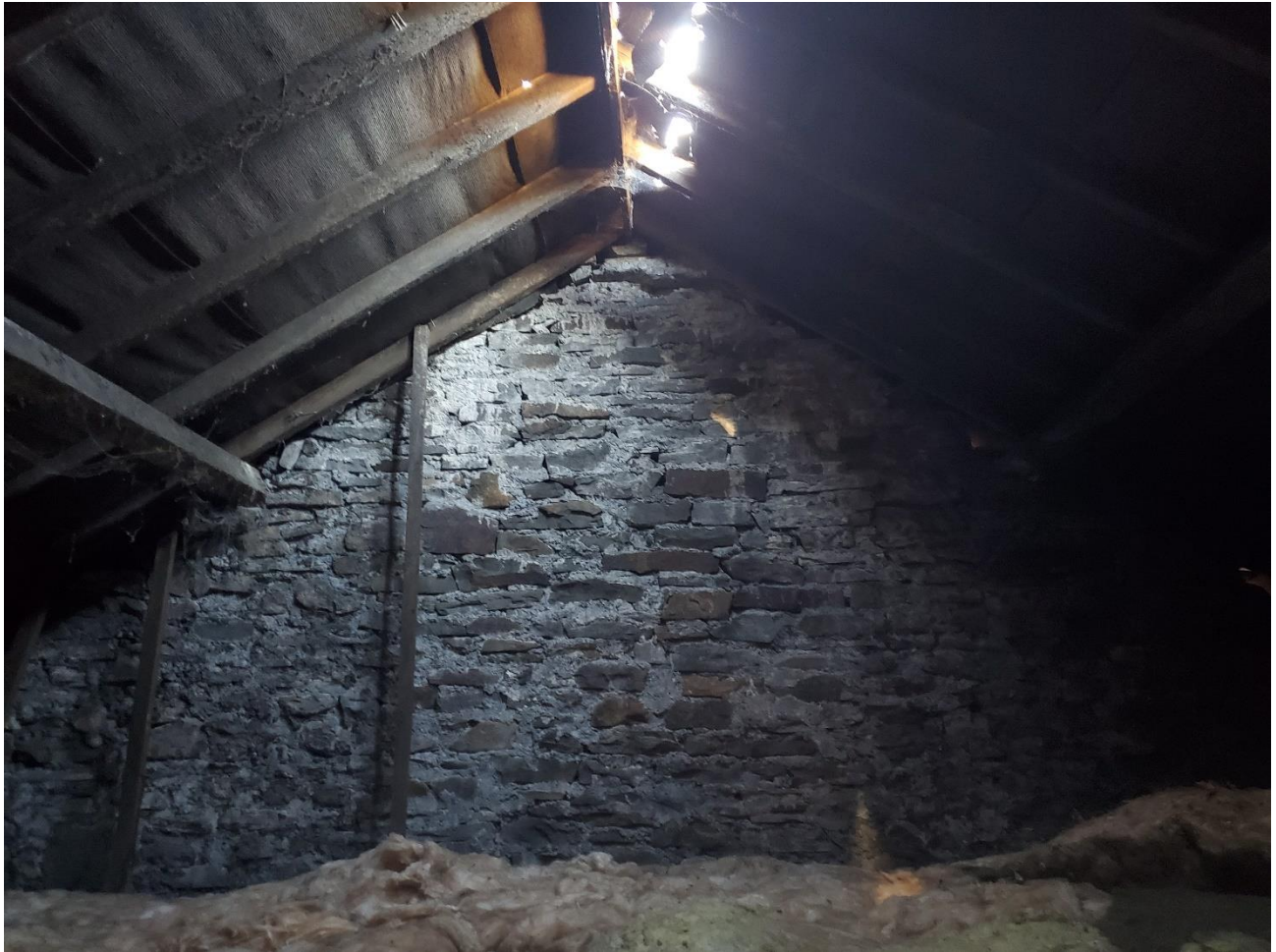
Figure 5: View from loft interior showing light spill from removed ridge tiles
