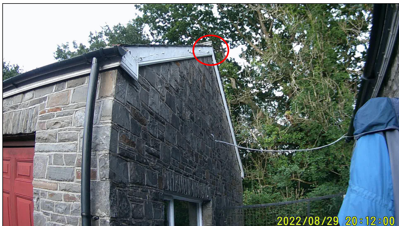
Photo 7: Location of Soprano Pipistrelle on southern gable end of garage.
