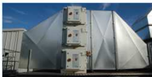
3 ESP Units Stacked in modular formation
