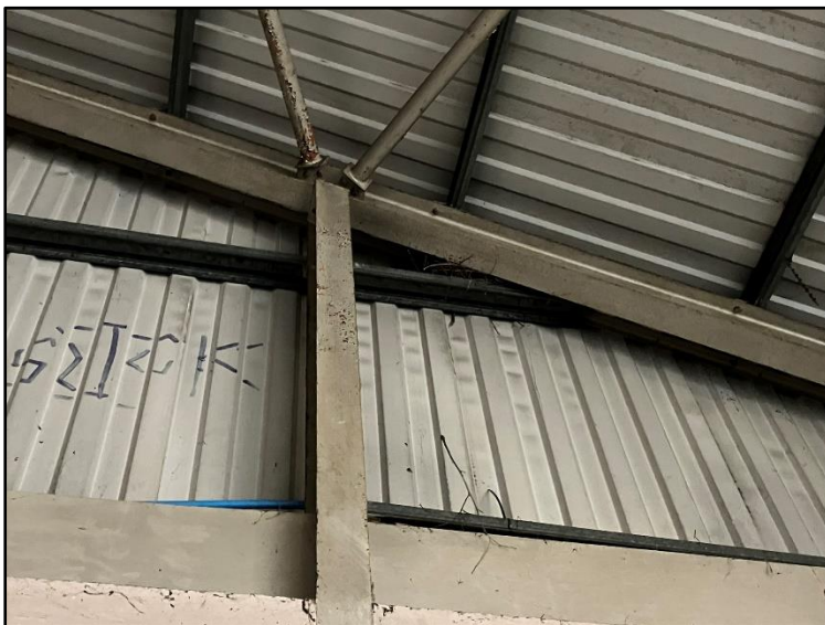
Plate 4 – Nest between corrugated roof and wall of eastern building
