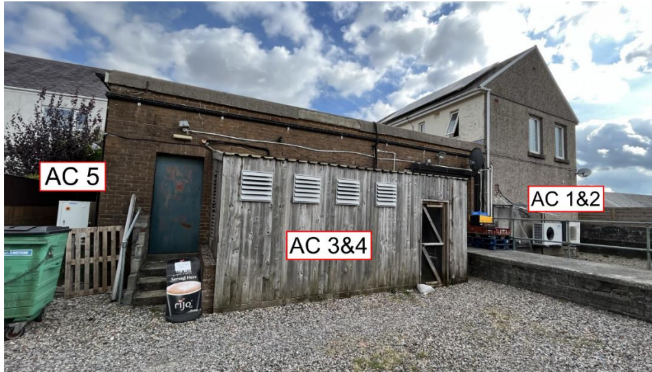
Figure 3.1 – Photo of A/C Units – Existing Scenario
