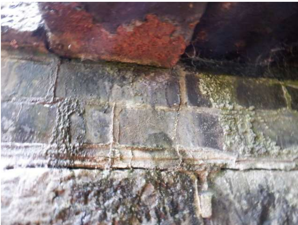
Photo 21: O/S Fracture to Downside Abutment (07.08.21)
