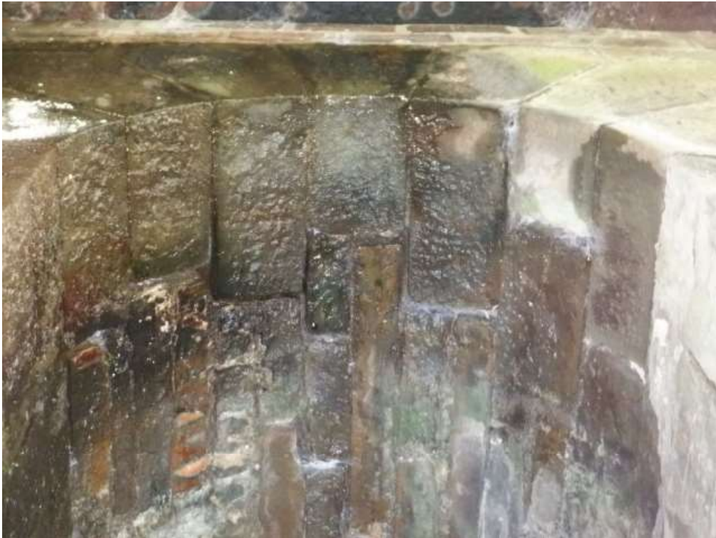
Photo 28: Typical View of Longitudinal Fracture to Relieving Arches (07.08.21)
