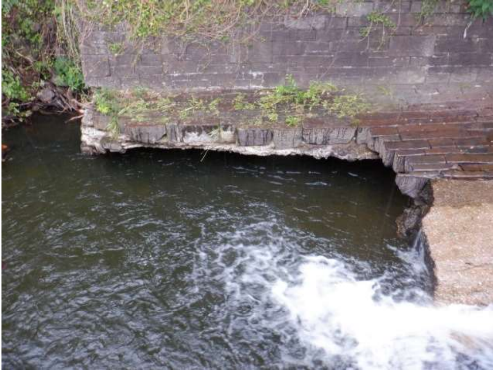
Photo 38: Undermining to Low Mileage End of Wier (07.08.21)
