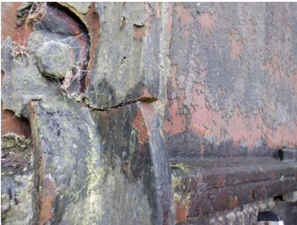
Photo 35: Horizontal Fracture & Displacement to Lower cranking (07.08.21)
