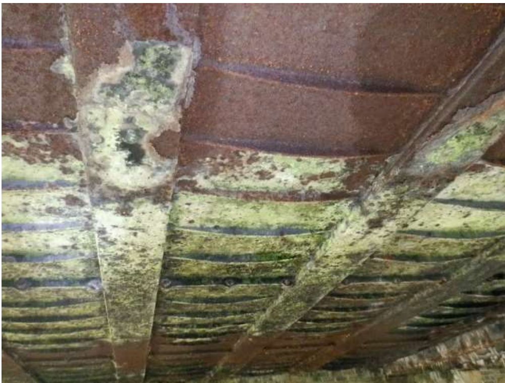
Photo 11: Corrosion to Deck Floor (07.08.21)
