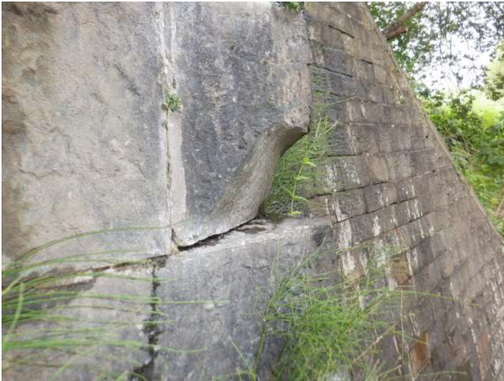
Photo 25: Spalling to Abutment Quoin (07.08.21)
