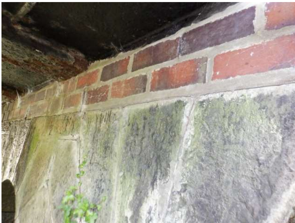
Photo 26: Horizontal Bed Joint Fracture (07.08.21)
