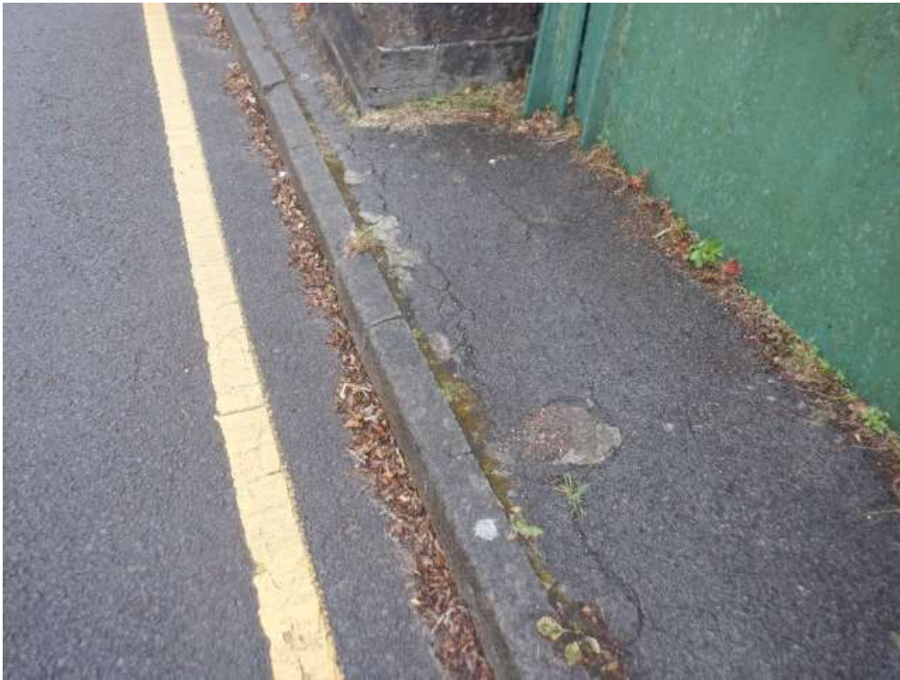
Photo 41: Cracks Present to Road & Pavement(07.08.21)
