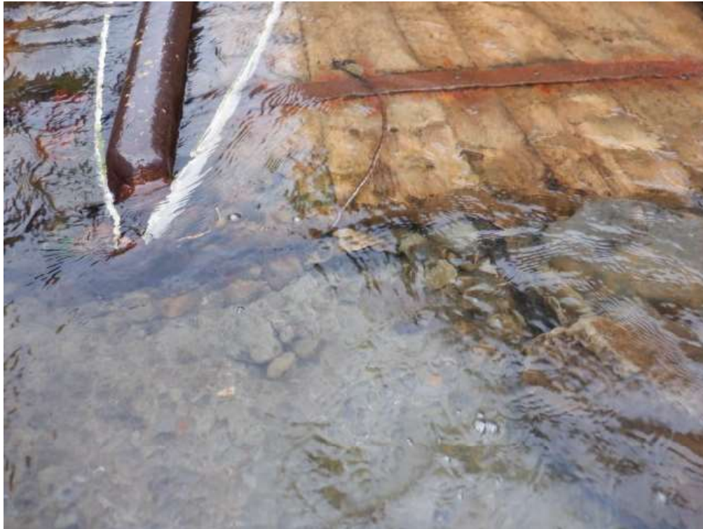
Photo 16: Debris Wedged at Timber Ends (07.08.21)
