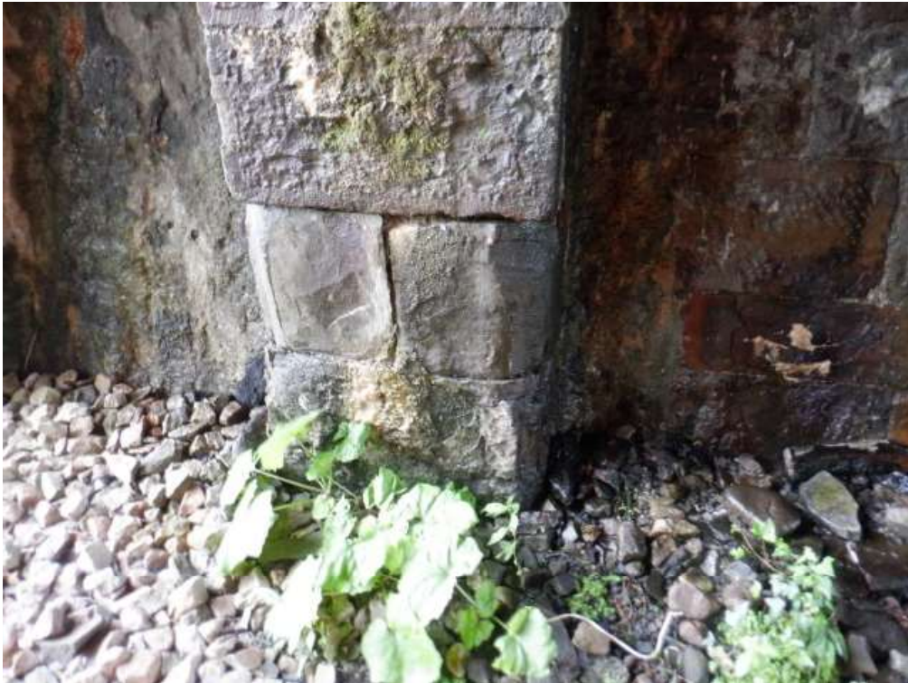
Photo 20: typical O/S Spalling to relieving Arches (07.08.21)
