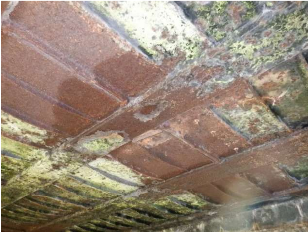
Photo 10: Corrosion Loss to MGI's (07.08.21)
