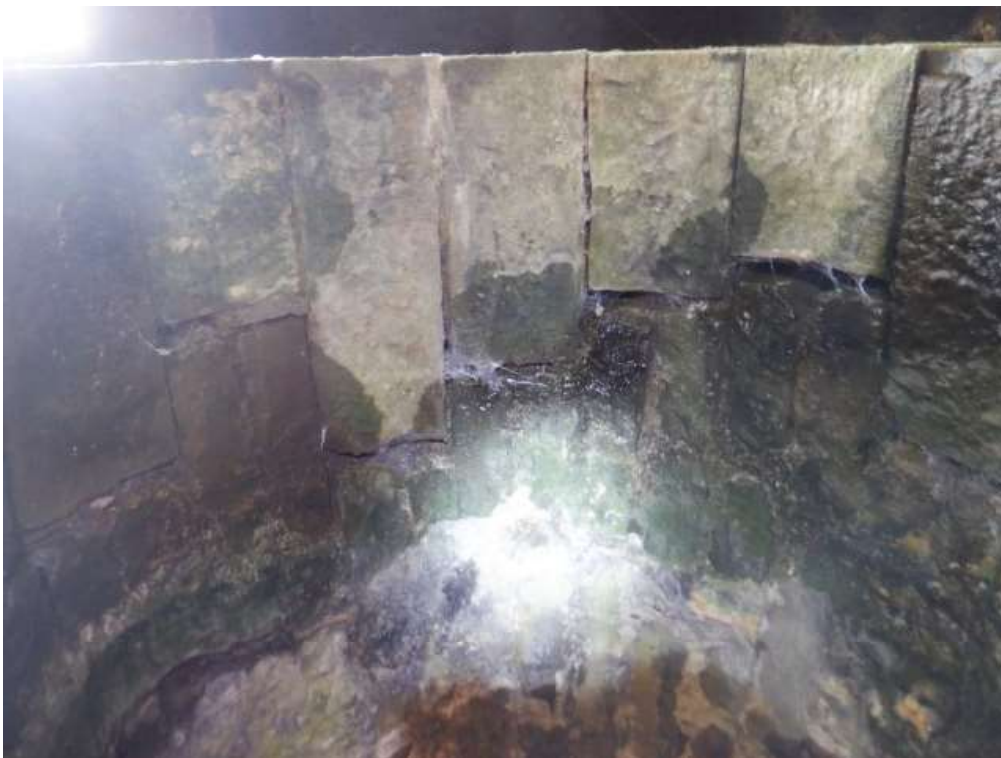
Photo 23: Typical View of Longitudinal Fractures to Relieving Arches (07.08.21)
