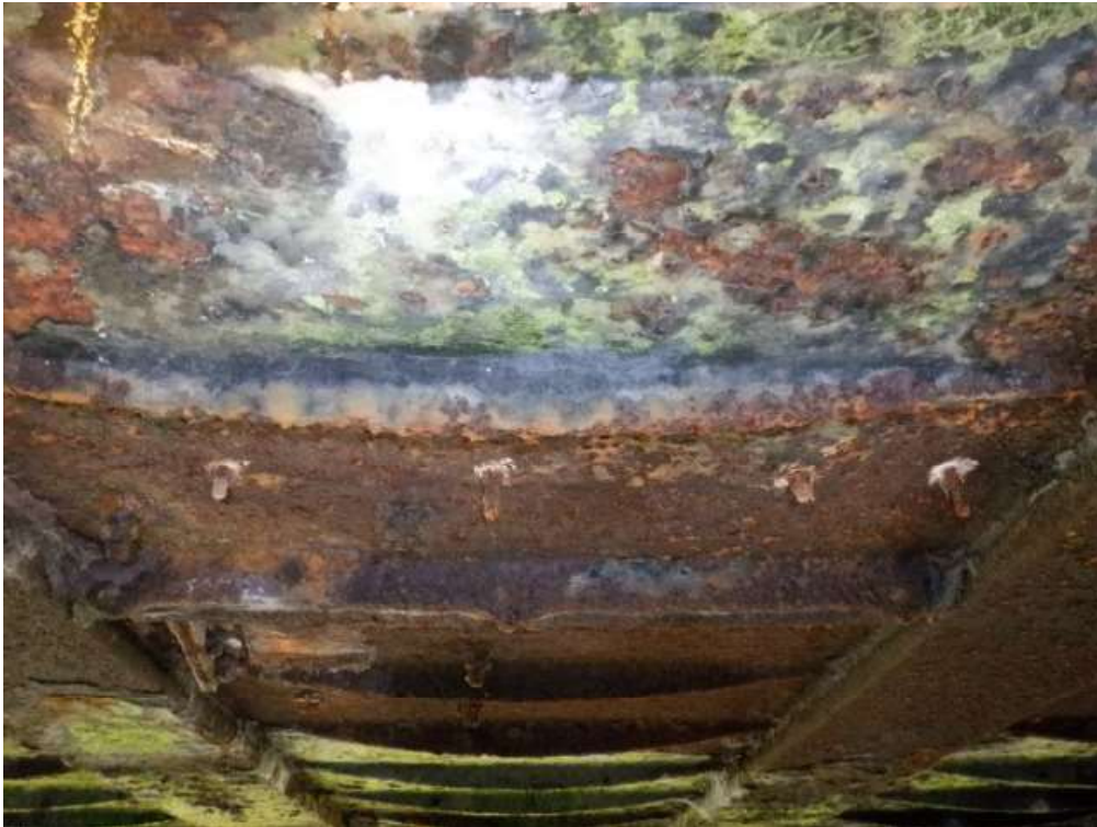
Photo 12: Loss to Ribbed Plate (07.08.21)
