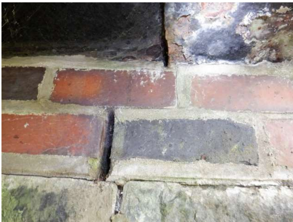
Photo 27: Vertical Fracture to Brickwork Below Low Mileage Girder (07.08.21)
