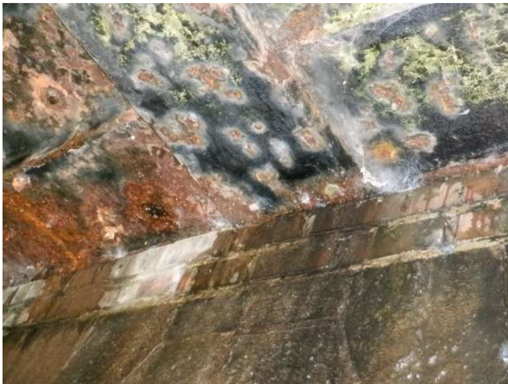
Photo 9: Corrosion Loss to MGI's (07.08.21)
