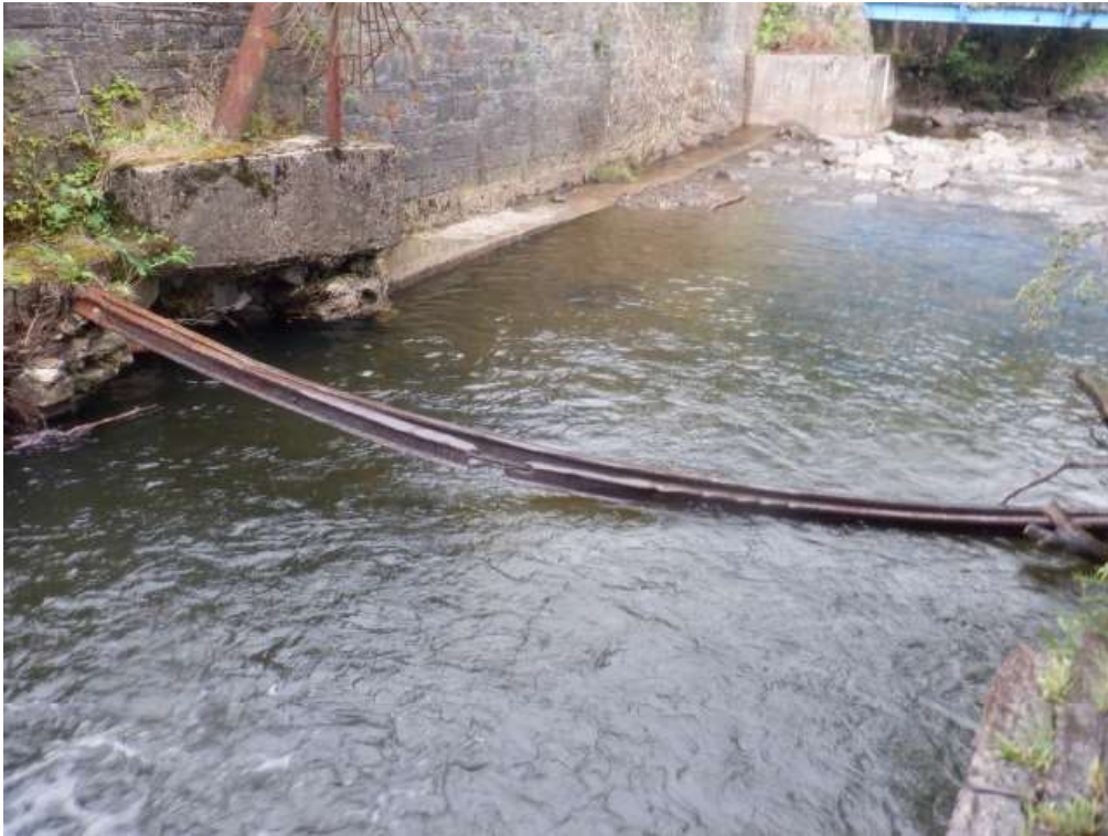
Photo 40: Detached & Bent Rail Retainer (07.08.21)
