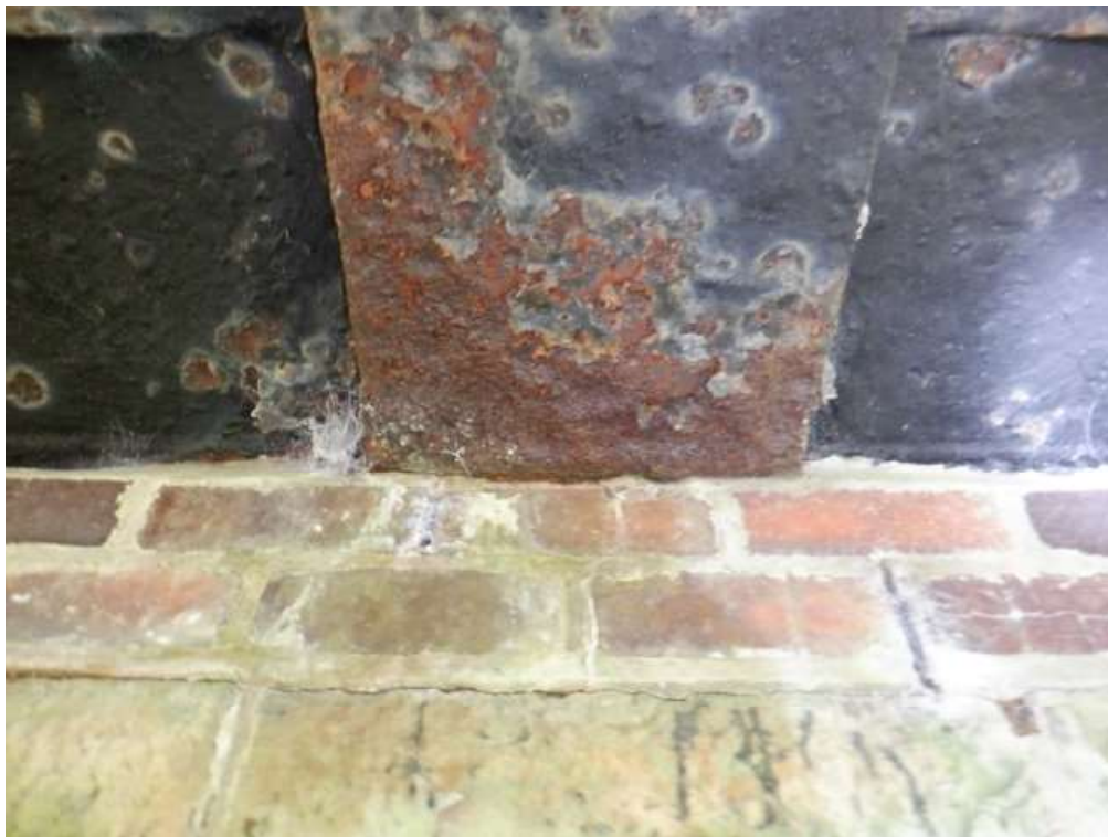
Photo 8: Corrosion Loss to MGI's (07.08.21)
