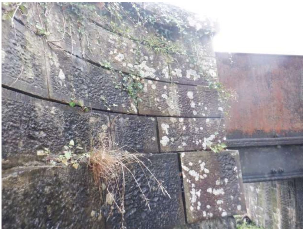
Photo 36: Displaced Stonework to Downside Pilaster (07.08.21)
