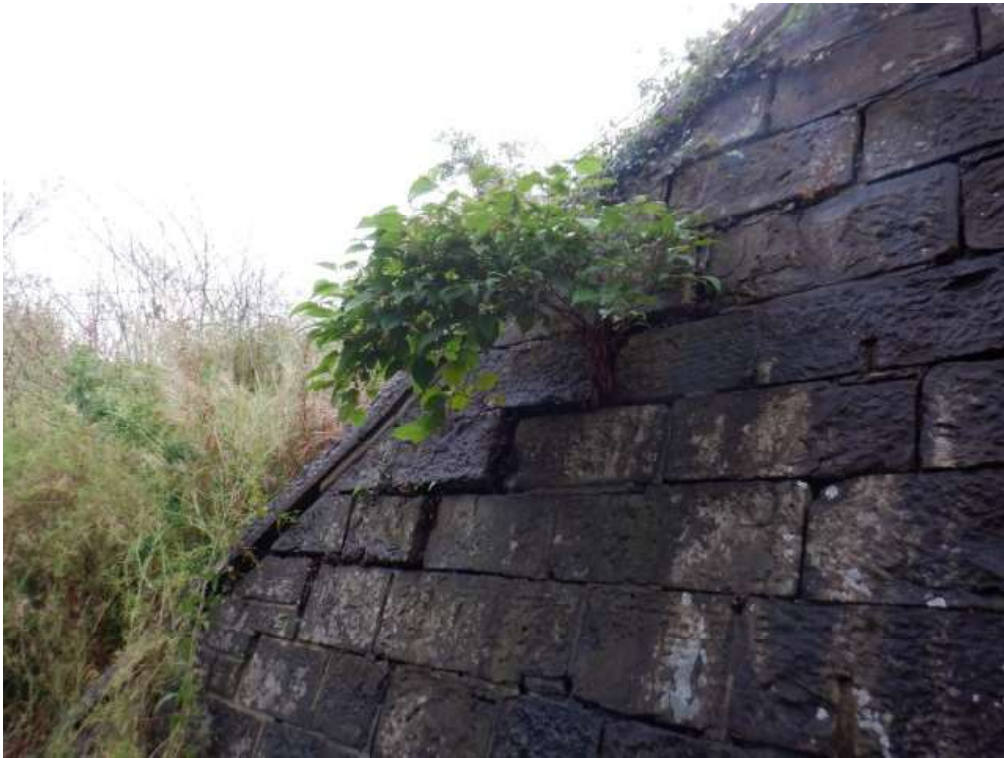
Photo 31: LTH & Displaced Stonework (07.08.21)
