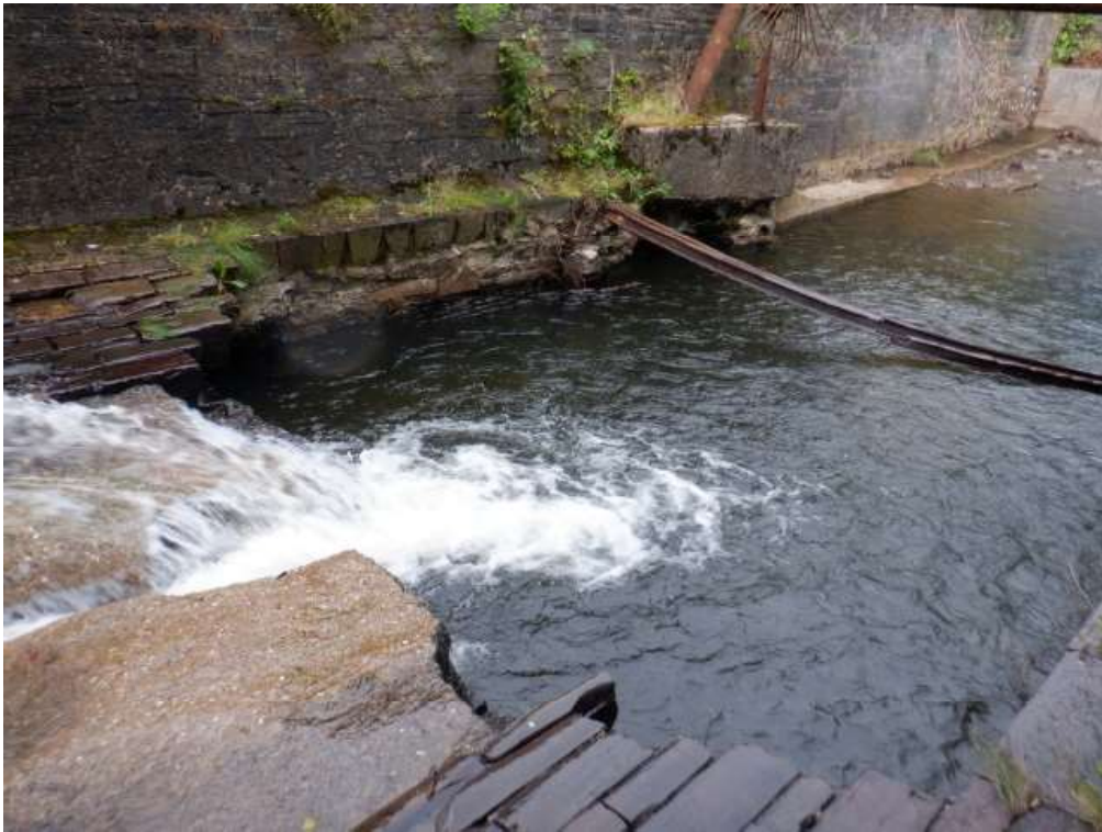
Photo 39: Undermining to High Mileage End of Weir (07.08.21)
