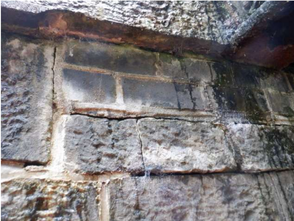
Photo 22: Horizontal Bed-Joint Fracture & LTH Stonework (07.08.21)
