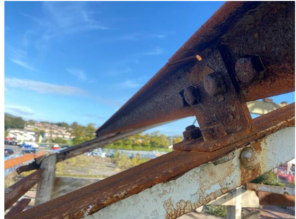
Photo B1- D6- Corrosion to purlins and truss
