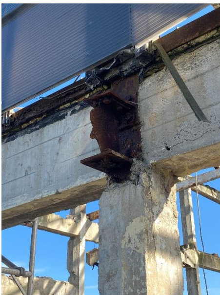
Photo B1- D9- Canopy member not fully removed
