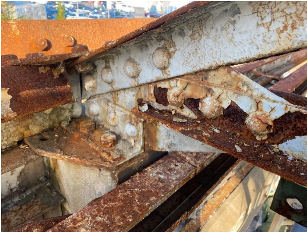
Photo B1- D5- Truss end connection – Typical spalling paint and light corrosion
