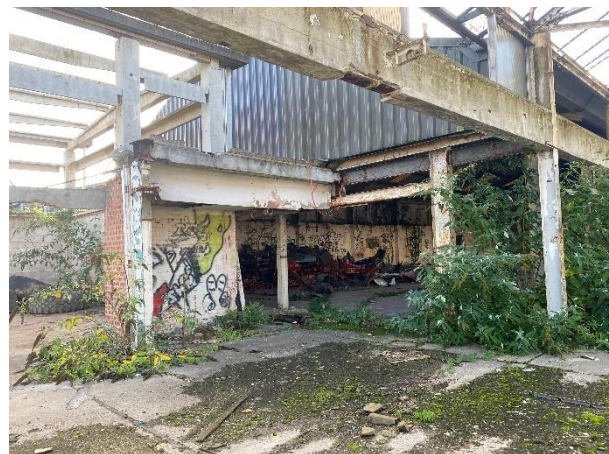
Photo B2-GA10 – Redundant steelwork outside building 3 and connected into building 2
