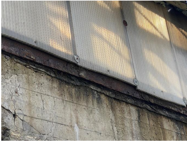
Photo B1- D11- Corroded bottom cladding rail
