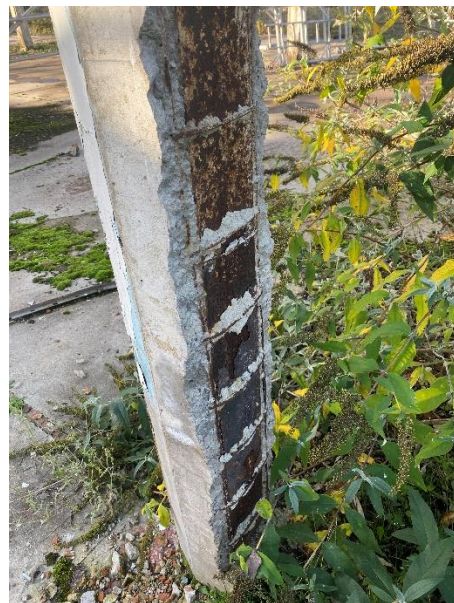
Photo B1- D2 – Concrete encasement spalled
