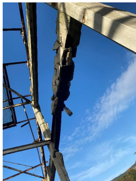
Photo B1- D4 – Damaged and missing concrete encasement
