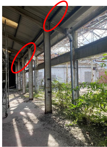
Photo B2- D5 – Missing eaves beams
