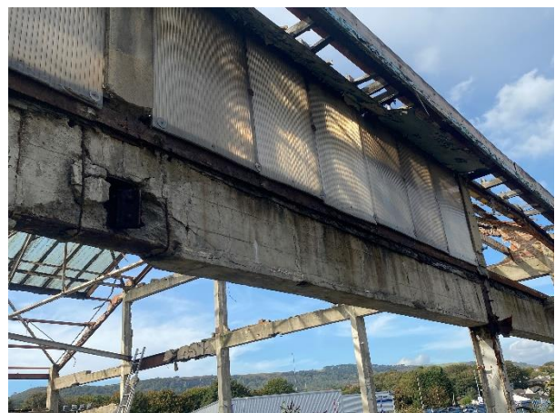
Photo B1 - GA8 - Side wall lights
