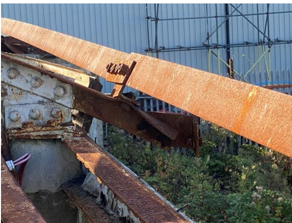
Photo B1- D7- Twisted end to truss
