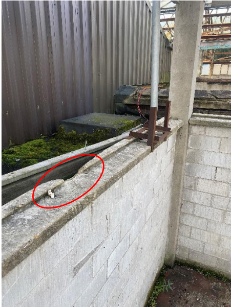
Photo B3- D5 – Spalled 'lip' to cladding rail
