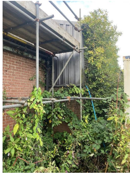
Photo B2- D2 – Heavy vegetation along boundary wall
