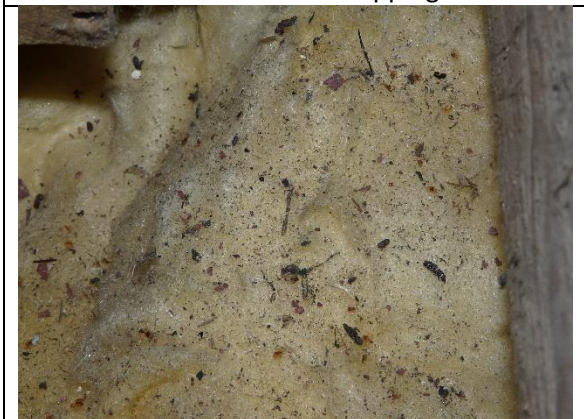
Photo 27: Close up view of bat droppings
