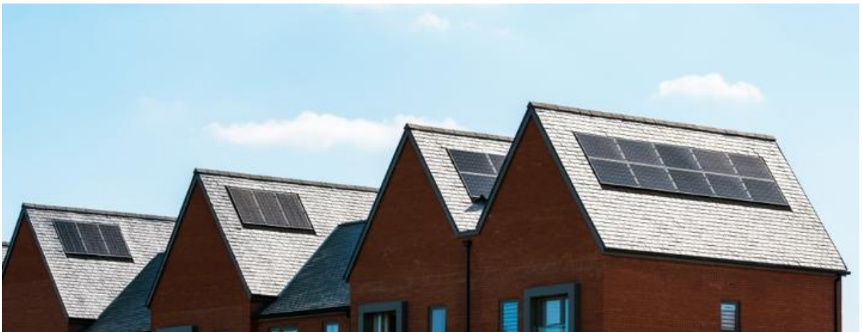
Figure 5: Domestic PV array image
