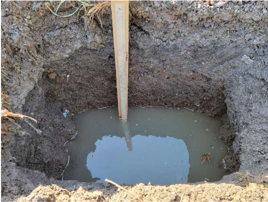
Picture 7 – Condition of Test pit 1 the morning of testing following heavy rain.
