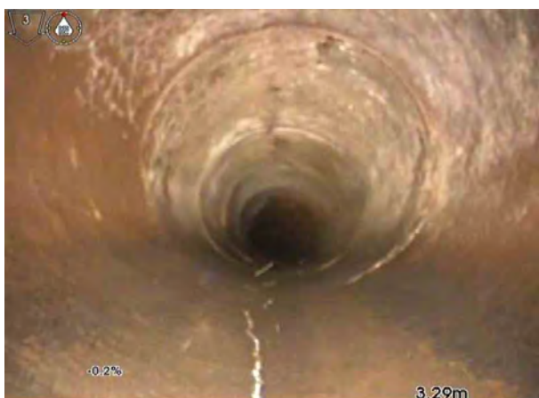
CMH1X_e4d0d78b-eefa-4dd0-a6c2-c070fd18919c_20220719_132531_413.jpg, 00:00:25, 3.15 m Crack, longitudinal at joint at 6 o'clock
