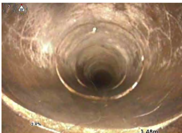
CMH1X_79a3eba9-7235-4626-9a07-8de68ec9bb5c_20220719_132455_071.jpg, 00:00:17, 1.44 m Cracks, multiple at joint from 9 o'clock to 5 o'clock
