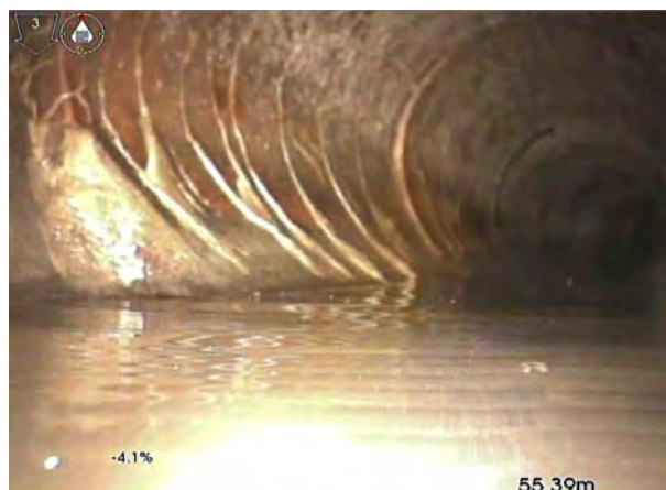
CMH1X_c25398c8-9cab-414a-9f26-2a7f2fc9a407_20220719_132036_588.jpg, 00:02:10, 55.39 m Cracks, multiple at joint from 7 o'clock to 9 o'clock
