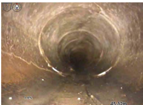
CMH1X_45e314fc-b6c1-4fbe-8aae-eed6d34c8893_20220719_122749_513.jpg, 00:00:41, 45.32 m Crack, longitudinal at joint at 8 o'clock
