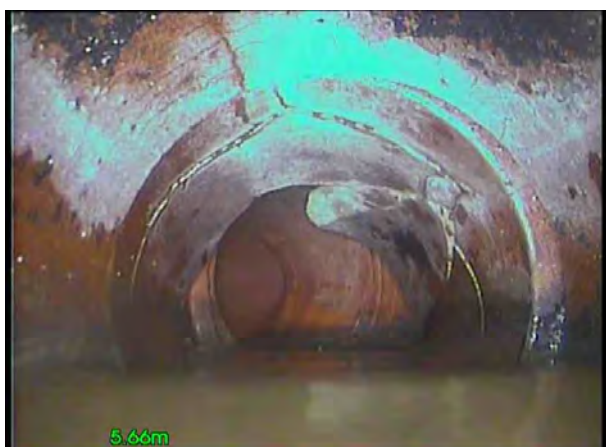
MH1X_e22f26e8-9fea-4220-a785-75829cdce594_20220719_102536_335.jpg, 00:00:40, 5.66 m Joint displaced, medium (between 1.0 and 1.5 times the pipe wall thickness)
