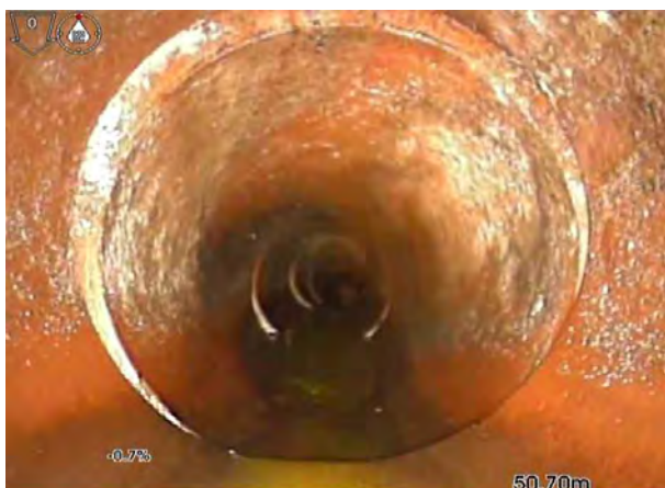
SMH1X_c9756ae9-7474-49f5-a008-c138a565df65_20220719_105926_330.jpg, 00:06:35, 50.70 m Joint displaced, medium (between 1.0 and 1.5 times the pipe wall thickness)
