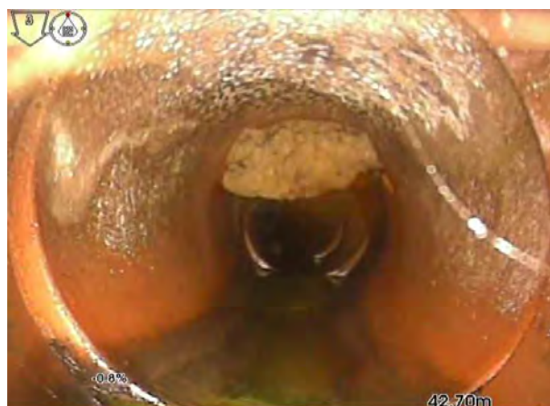
SMH1X_a768c2ae-1ae9-4f7c-a708-5cb530ed3402_20220719_104728_997.jpg, 00:04:49, 42.70 m Joint displaced, medium (between 1.0 and 1.5 times the pipe wall thickness)
