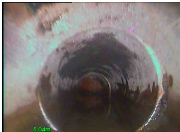
MH1X_477a9be3-cc3c-4335-ad93-83c09bcec28f_20220719_102453_801.jpg, 00:00:36, 5.04 m Joint displaced, medium (between 1.0 and 1.5 times the pipe wall thickness)
