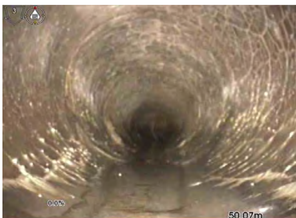
CMH1X_e1258b56-ab67-4f49-964f-38183c96be60_20220719_131533_565.jpg, 00:01:18, 50.07 m Cracks, multiple at joint from 7 o'clock to 5 o'clock
