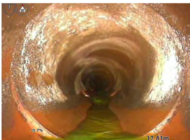
SMH1X_f92ca79e-53b3-4d47-887d-68a5be7a452c_20220719_103536_333.jpg, 00:02:21, 17.81 m Joint displaced, medium (between 1.0 and 1.5 times the pipe wall thickness)
