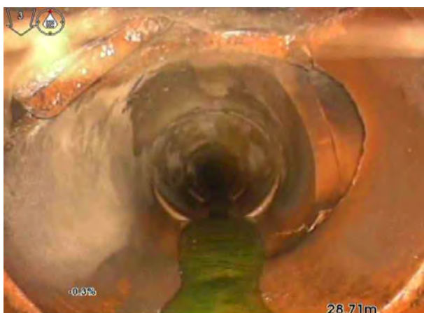
SMH1X_08197eb3-2e41-4746-a179-c65fda0d987c_20220719_103938_946.jpg, 00:03:11, 28.71 m Broken sewer at joint from 9 o'clock to 1 o'clock
