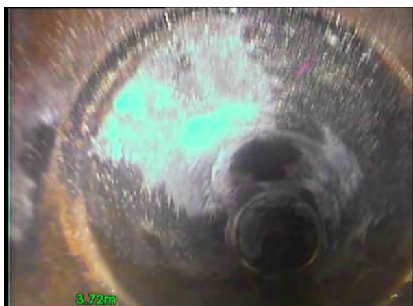
MH1X_bfa6a2ae-05b9-4013-944a-ce73e46ab4cb_20220719_102126_708.jpg, 00:00:31, 3.72 m Joint displaced, medium (between 1.0 and 1.5 times the pipe wall thickness)
