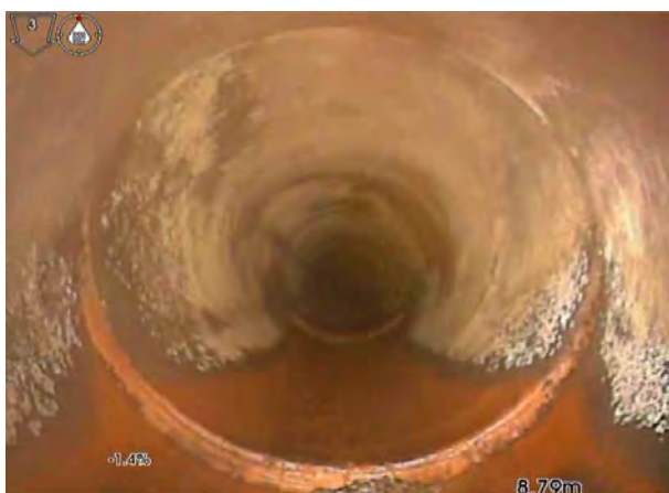
SMH1X_991156c6-c930-4b20-a70c-0a7b7d79ccfb_20220719_103122_509.jpg, 00:00:48, 8.79 m Joint displaced, medium (between 1.0 and 1.5 times the pipe wall thickness)
