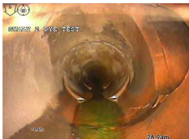
SMH1X_6ba71695-2bea-4a47-8214-2e20b8661d8e_20220719_104032_953.jpg, 00:03:15, 28.94 m Junction at 3 o'clock, 150mm diameter, Gully coming into main line.
