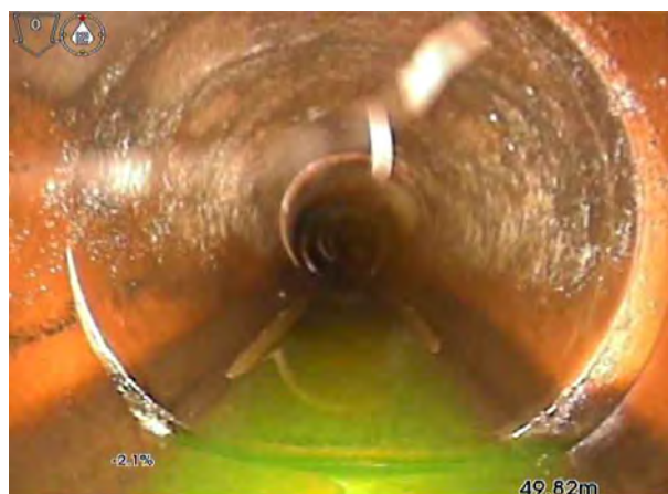
SMH1X_9445edbe-fada-433b-998c-6e3624088dc6_20220719_105901_218.jpg, 00:06:30, 49.82 m Joint displaced, medium (between 1.0 and 1.5 times the pipe wall thickness)
