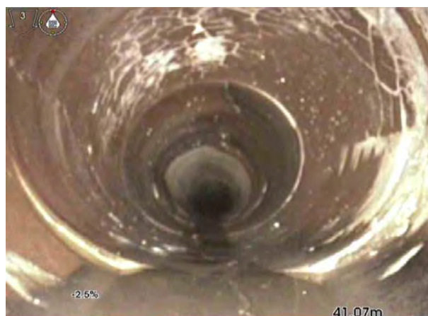
CMH1X_d52fe99e-2010-4b86-b3a5-692ec5cfc662_20220719_111404_809.jpg, 00:00:13, 40.97 m Cracks, multiple at joint from 9 o'clock to 4 o'clock
