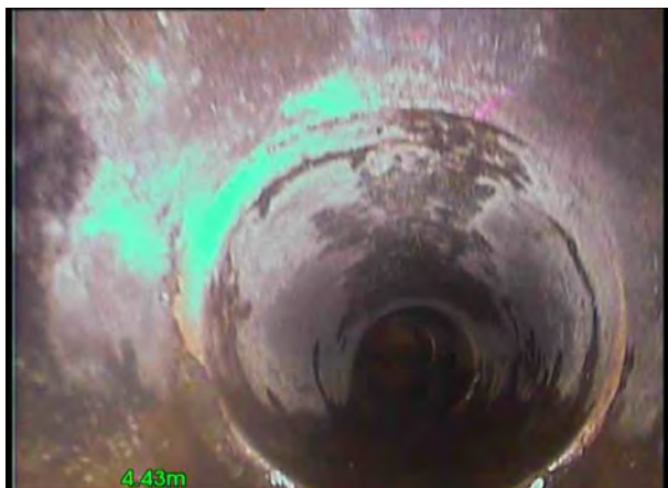
MH1X_60254934-20c9-4a15-bc4b-028e3730e26f_20220719_102146_948.jpg, 00:00:34, 4.35 m Joint displaced, medium (between 1.0 and 1.5 times the pipe wall thickness)
