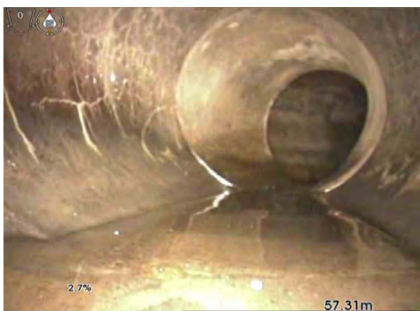
CMH1X_da2fb8fe-7d74-4e1c-b099-19255886b6ae_20220719_132209_613.jpg, 00:03:15, 57.31 m Cracks, multiple at joint from 8 o'clock to 11 o'clock
