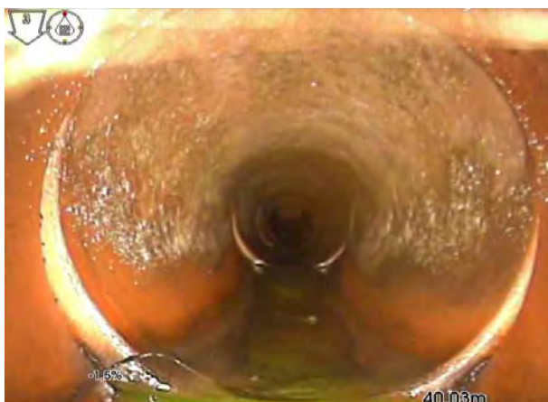
SMH1X_29679ca9-ad34-4a37-aa49-2cf5cfe874d0_20220719_104600_597.jpg, 00:04:35, 40.03 m Joint displaced, medium (between 1.0 and 1.5 times the pipe wall thickness)
