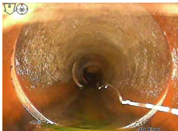
SMH1X_35a003be-02b4-492a-8c26-50edb8210f50_20220719_104640_575.jpg, 00:04:39, 40.83 m Joint displaced, medium (between 1.0 and 1.5 times the pipe wall thickness)
