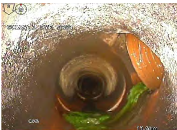
SMH1X_452ded66-a8bd-45a6-bf06-2eabbaf84c40_20220719_103405_437.jpg, 00:01:15, 13.65 m Junction at 3 o'clock, 150mm diameter, Gully coming into main storm line.
