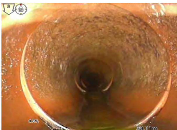
SMH1X_78db930b-fe2f-441f-a342-35a0c260ba97_20220719_104519_999.jpg, 00:04:26, 38.11 m Joint displaced, medium (between 1.0 and 1.5 times the pipe wall thickness)
