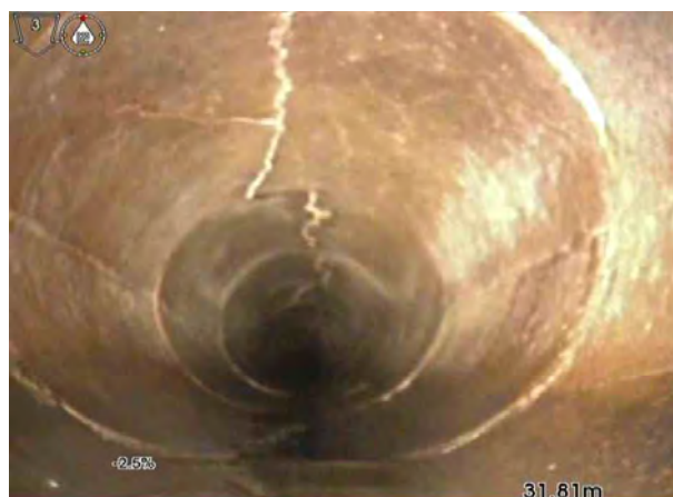
CMH1X_1aa01f2c-435b-4161-b06c-21360a938e73_20220719_133157_987.jpg, 00:02:39, 31.81 m Crack, longitudinal at joint at 12 o'clock
