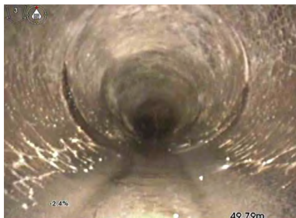
CMH1X_343aa71f-1ccd-4dd4-b85a-2276139aa498_20220719_131510_744.jpg, 00:01:12, 49.70 m Cracks, multiple at joint from 7 o'clock to 4 o'clock
