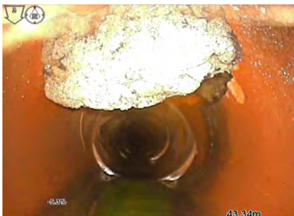
SMH1X_0991fb30-f8cd-45af-9bb6-baa5ac977309_20220719_105414_798.jpg, 00:04:52, 43.34 m Encrustation, heavy at joint from 9 o'clock to 2 o'clock
