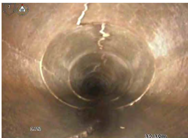
CMH1X_fe776423-a662-4269-934e-854f3dabd5ca_20220719_133225_674.jpg, 00:02:45, 32.39 m Fracture, longitudinal at joint at 7 o'clock
