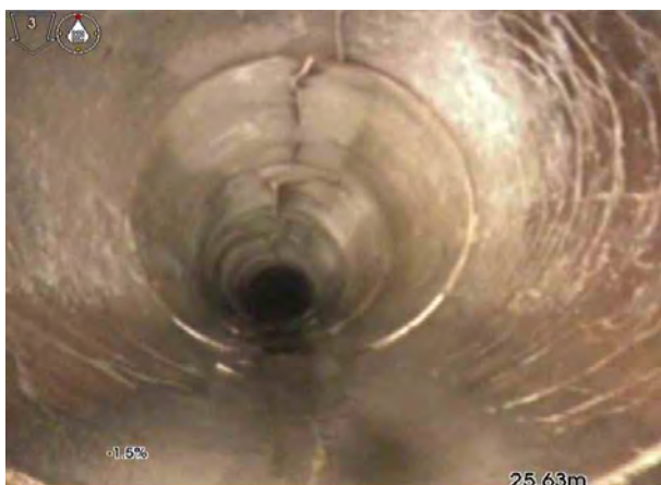
CMH1X_4d5620eb-5315-4bd6-baee-b84f84f942d3_20220719_133024_340.jpg, 00:02:09, 25.63 m Cracks, multiple at joint from 11 o'clock to 7 o'clock
