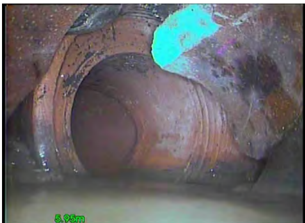
MH1X_5d2a9960-5d72-4562-b4e2-6fcc3b41231b_20220719_102617_849.jpg, 00:00:43, 5.95 m Broken sewer at joint from 7 o'clock to 4 o'clock
