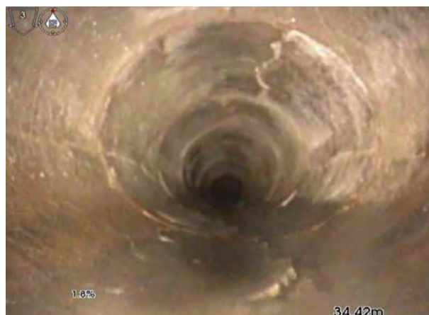
CMH1X_c5f1144c-7e4d-465e-89df-0abc384fcca8_20220719_133255_624.jpg, 00:02:57, 34.42 m Fracture, longitudinal at joint at 6 o'clock
