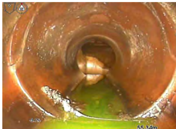
SMH1X_f6aff482-66af-443c-86ea-92f373434d74_20220719_110428_546.jpg, 00:06:59, 55.34 m Joint displaced, medium (between 1.0 and 1.5 times the pipe wall thickness)
