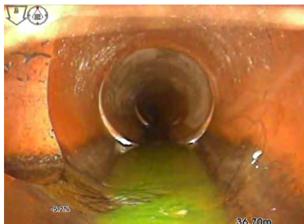
SMH1X_2e7141a8-7bc3-45fc-bbb0-ae63c5aebb67_20220720_082312_618.jpg, 00:04:19, 36.70 m Junction at 9 o'clock, 150mm diameter, Point where MH1 discharges into main line.
