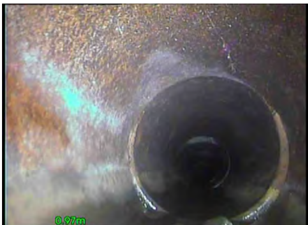
MH1X_b744a960-7a20-4b56-8a30-1d33e5686fc5_20220719_102008_611.jpg, 00:00:14, 0.97 m Joint displaced, medium (between 1.0 and 1.5 times the pipe wall thickness)
