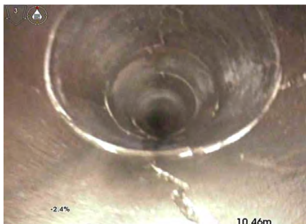
CMH1X_fd2ca93c-05ea-45de-a7db-d6ecc455912a_20220719_132641_868.jpg, 00:00:57, 10.46 m Fracture, longitudinal at joint at 6 o'clock
