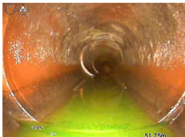
SMH1X_dbea6608-f440-4ef0-bffc-94a86a080fee_20220719_10021_131.jpg, 00:06:41, 51.75 m Joint displaced, medium (between 1.0 and 1.5 times the pipe wall thickness)
