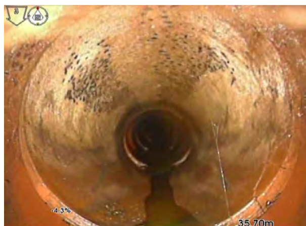
SMH1X_1e9fa716-6acc-4fff-8261-7748a058d3a6_20220719_104320_722.jpg, 00:04:13, 35.52 m Joint displaced, medium (between 1.0 and 1.5 times the pipe wall thickness)
