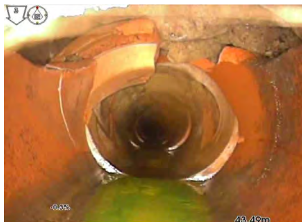
SMH1X_3ea32942-d369-4b15-8271-72f77b7ee6fc_20220719_105543_877.jpg, 00:04:58, 43.49 m Broken sewer from 9 o'clock to 3 o'clock
