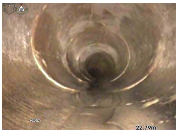
CMH1X_ed703122-72fe-4839-898c-2d52828b7e33_20220719_132933_843.jpg, 00:01:55, 22.79 m Crack, longitudinal at joint at 5 o'clock
