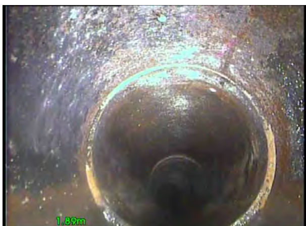
MH1X_09a68e6f-ac20-44e5-bb86-31d93af89045_20220719_102045_537.jpg, 00:00:22, 1.89 m Joint displaced, medium (between 1.0 and 1.5 times the pipe wall thickness)
