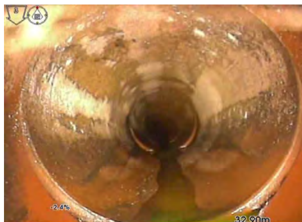
SMH1X_d89dceba-2ce3-49bd-9031-cc1f10aed6ff_20220719_104239_588.jpg, 00:04:01, 32.80 m Joint displaced, medium (between 1.0 and 1.5 times the pipe wall thickness)
