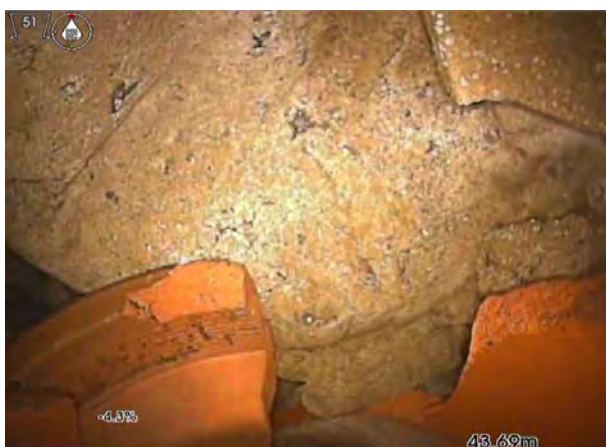
SMH1X_4996abcc-367f-4644-a34a-1bcbda12a709_20220719_105612_839.jpg, 00:04:58, 43.49 m Broken sewer from 9 o'clock to 3 o'clock
