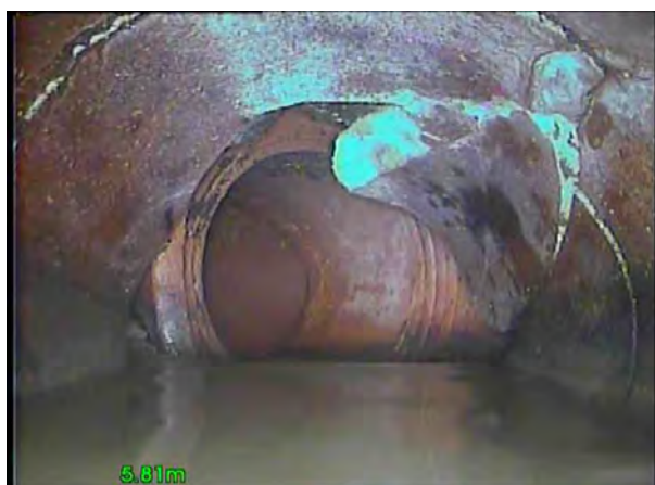
MH1X_4c46204d-9123-4a63-8f59-36ef4e7a8eda_20220719_102558_320.jpg, 00:00:42, 5.81 m Fractures, multiple at joint from 8 o'clock to 4 o'clock
