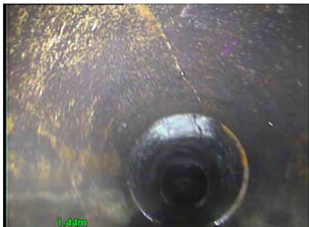
MH1X_9328158e-ab0f-47cd-8b6a-c4d7b4eede58_20220719_102027_722.jpg, 00:00:18, 1.44 m Crack, longitudinal at joint at 12 o'clock
