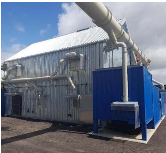
Building structure with demo/attack unit
