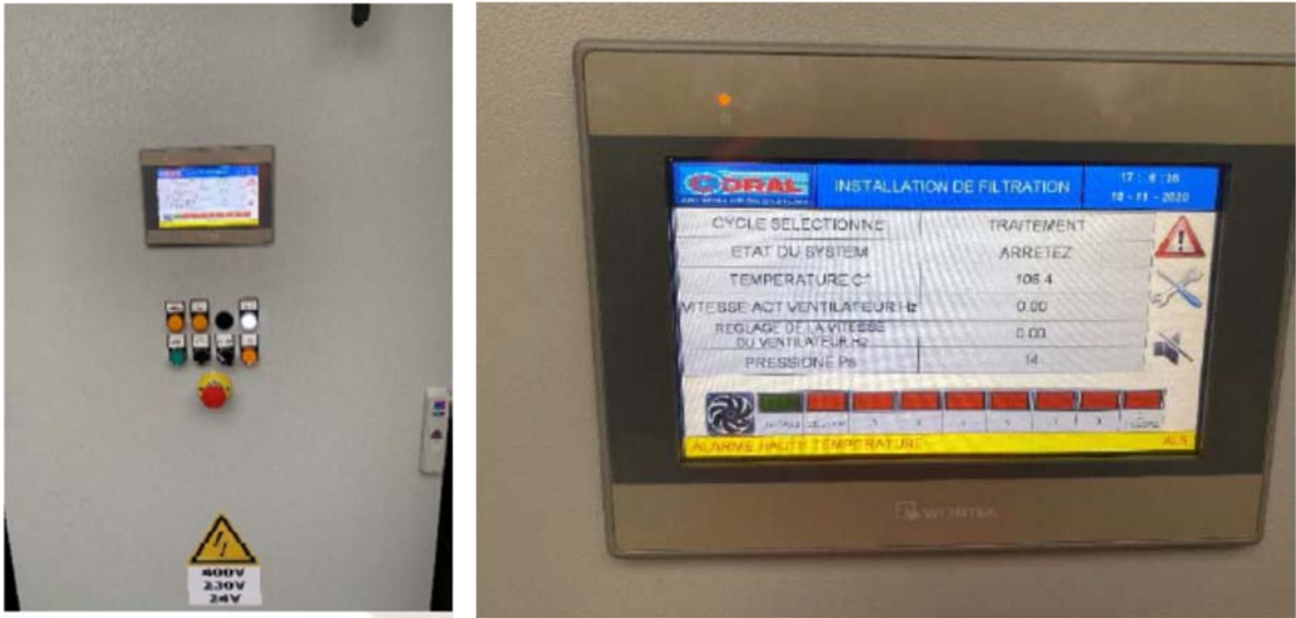
Touchscreen in the switchboard A1 for failure analysis and maintenance of the smoke cleaning system.
