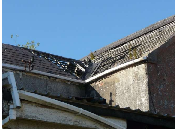
Image 5: Roof - viewed from south - large gaps
