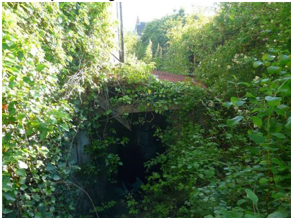
Image 14: Flooded shed / basement to north of building
