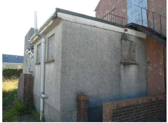
Image 4: Single storey extensions to south - gaps around soffits
