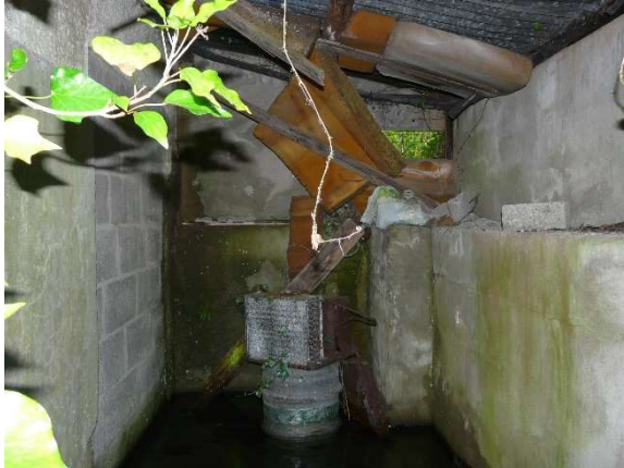
Image 7: Flooded basement / cellar
