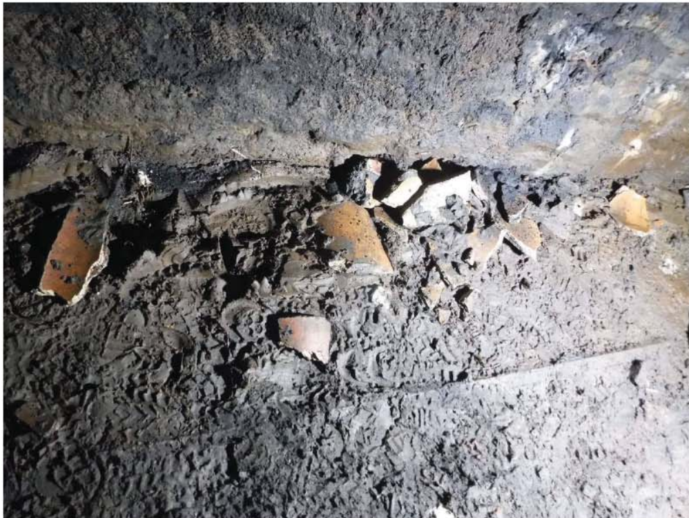
Photo No.43: Full length of tunnel, Solum Up & Down, drainage WIP, smashed track drainage pipes, poor underfoot conditions, hazard (typical example found at 071+11 cess down).
