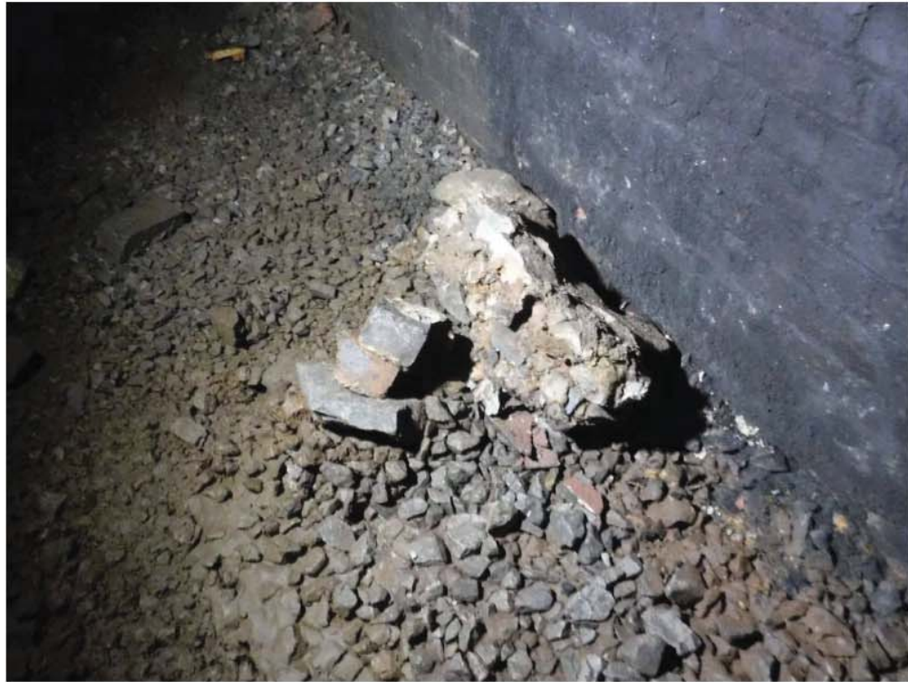
Photo No.34: 043+17 Solum Up, broken out catch-pit dumped in cess.
