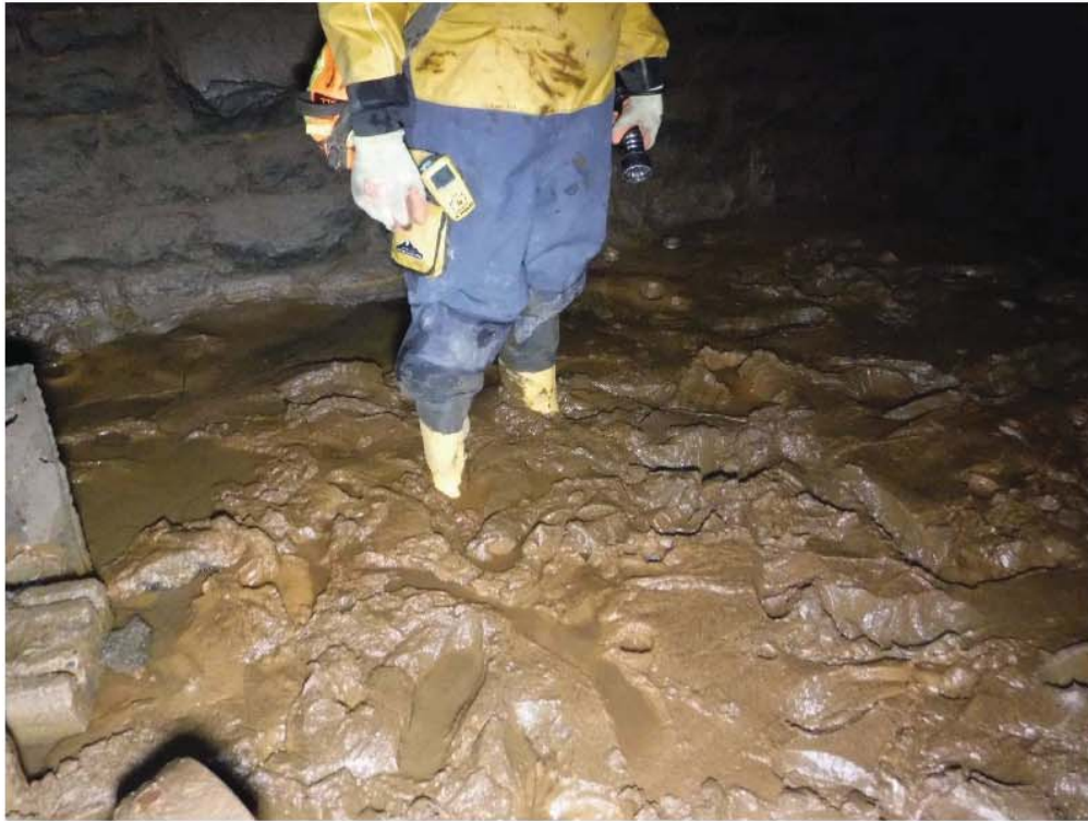
Photo No.44: 071+19 to 072+15 Solum Up & Down, Mud and flooding, depth 3".
