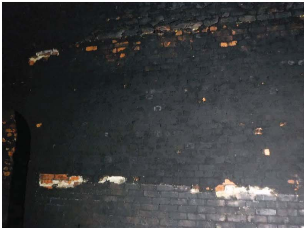
Photo No.35: 046+00 to 048+20 Sidewall & Haunches Up & Down, Brickwork, bulging 75mm with random vertical and longitudinal fractures, max. width 1mm, hollow, area 20sq.m.
