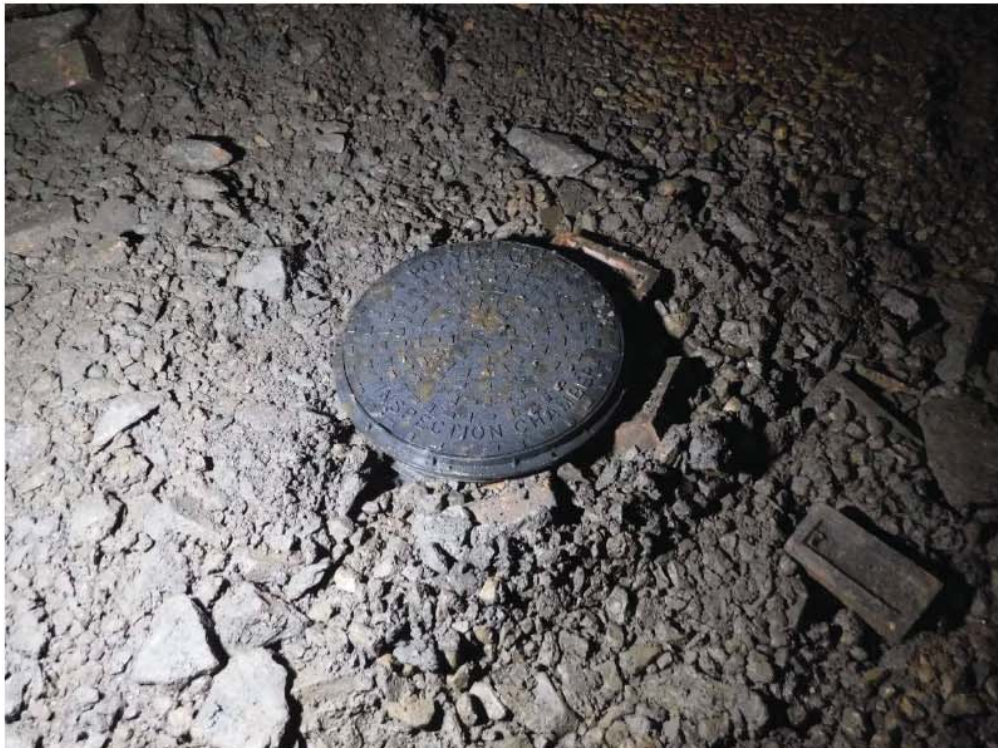
Photo No.41: 062+15 to 073+05 Solum Up & Down, drainage WIP, catch-pits and/or earthenware pipes broken out, new inspection chambers fitted proud on solum, hazard.
