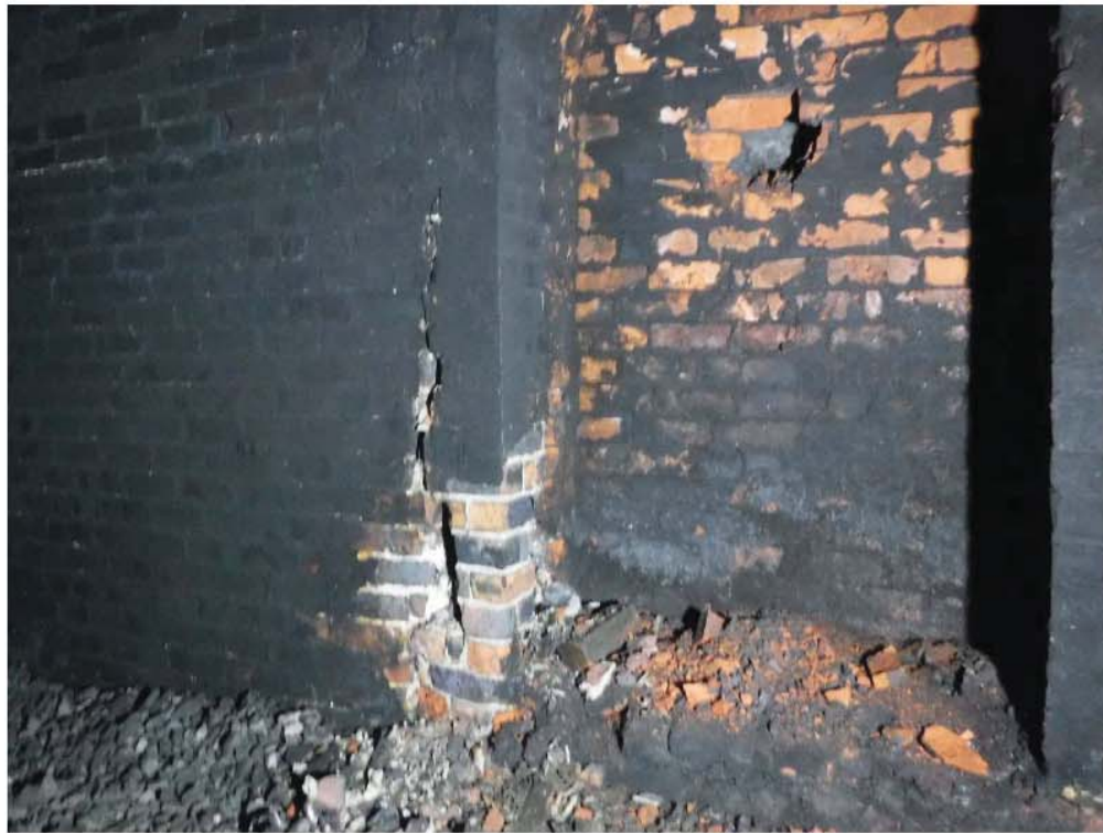
Photo No.36: 046+10 Refuge Down, Brickwork, spalling, depth 100mm, area 2sq.m., vertical fractures, length 1.6m to both Quoins, hollow.
