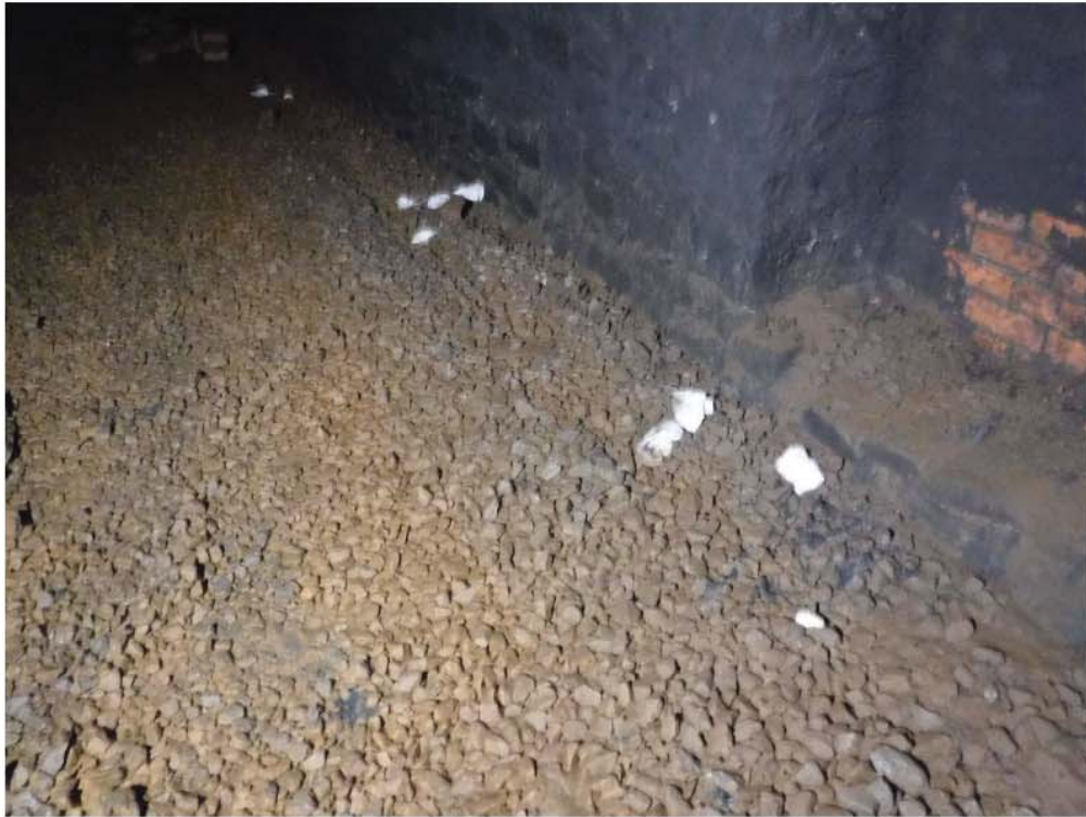
Photo No.38: 062+00 Solum Up, workman toilet waste, hazard.
