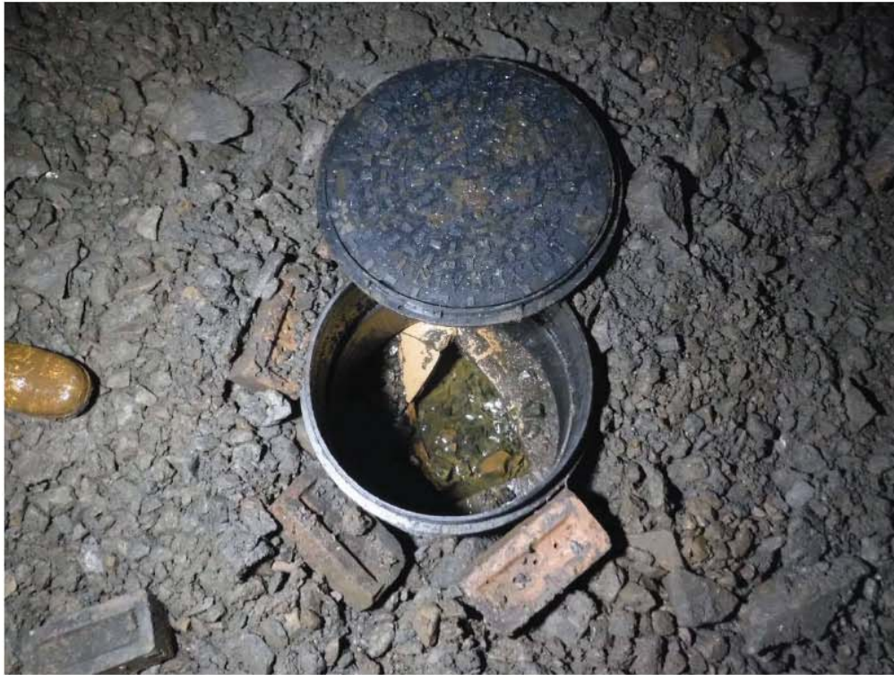
Photo No.40: 062+15 to 073+05 Solum Up & Down, drainage WIP, catch-pits and/or earthenware pipes broken out, new inspection chambers fitted proud on solum, hazard.
