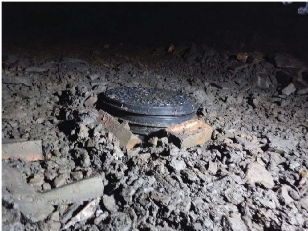
Photo No.39: 062+15 to 073+05 Solum Up & Down, drainage WIP, catch-pits and/or earthenware pipes broken out, new inspection chambers fitted proud on solum, hazard.
