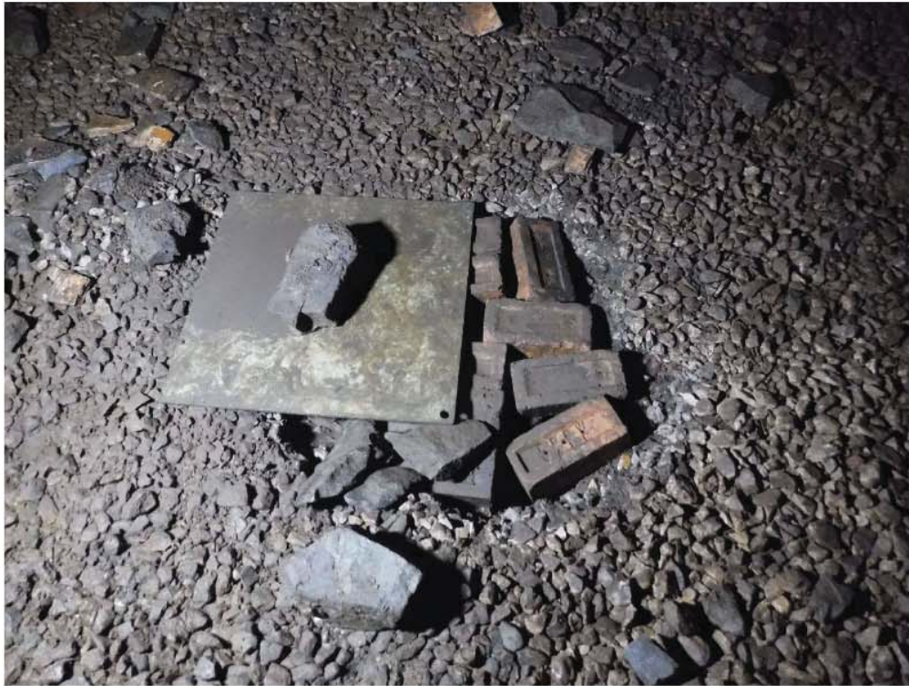
Photo No.42: 063+10 Solum Up & Down, Open catch-pit to six-foot with water welling up from inside. New cover fitted but displaced/ill-fitting. Now not surcharging.
